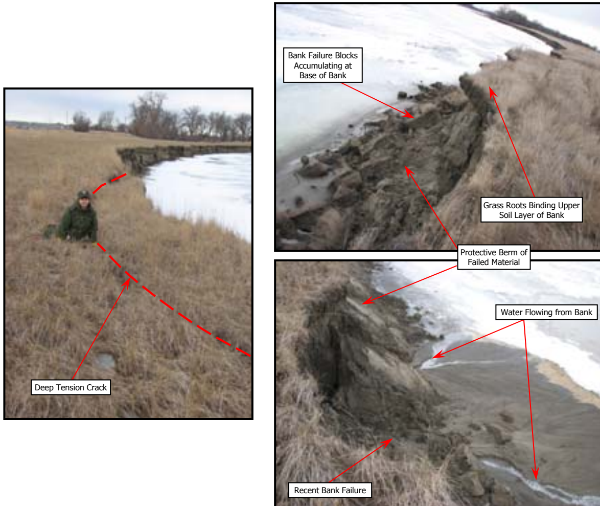
Figure 4.3 Photographs Taken by NPS Employees on 9 March 2007 Shortly before Ice-Out, showing: a) Deep Tension Crack Approx. 7 ft from Bank Edge; b) Cantilever Overhang and Recent Bank Failure; c) Water Flowing from Bank and Recent Bank Failure.
