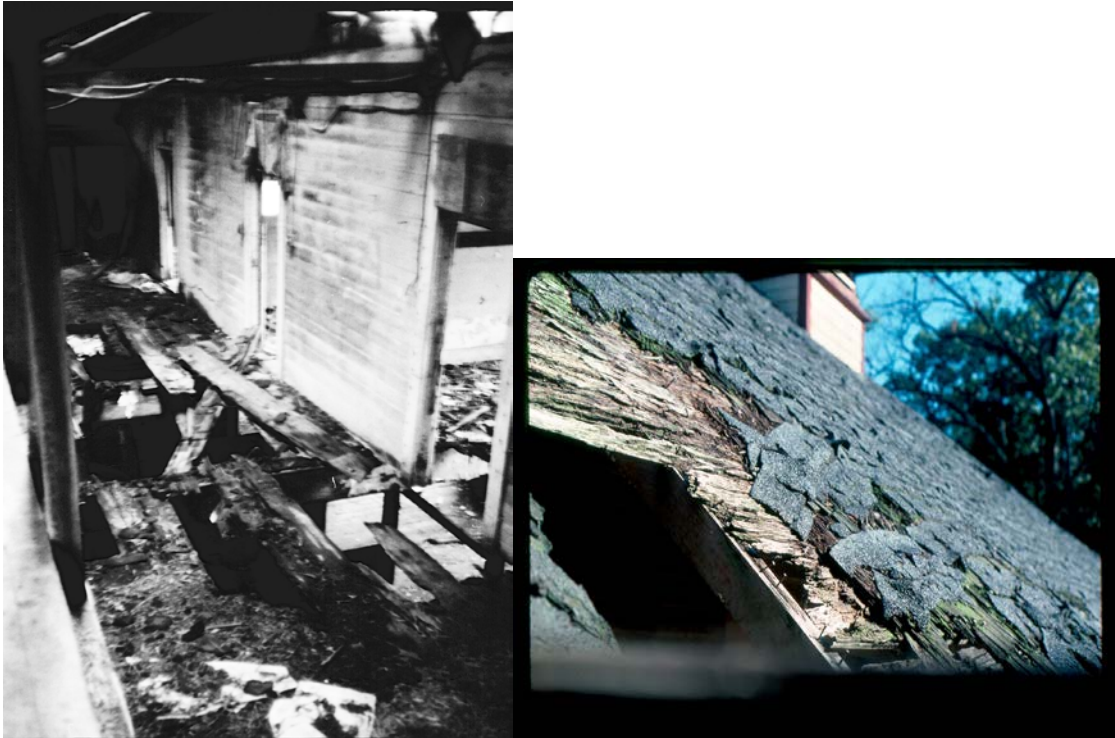
Fig. 2: Deterioration at Goddard State Park in Warwick, Rhode Island. The barn was demolished after deteriorating from lack of maintenance (Rhode Island Historic Preservation and Heritage Commission. Photographs on file).
