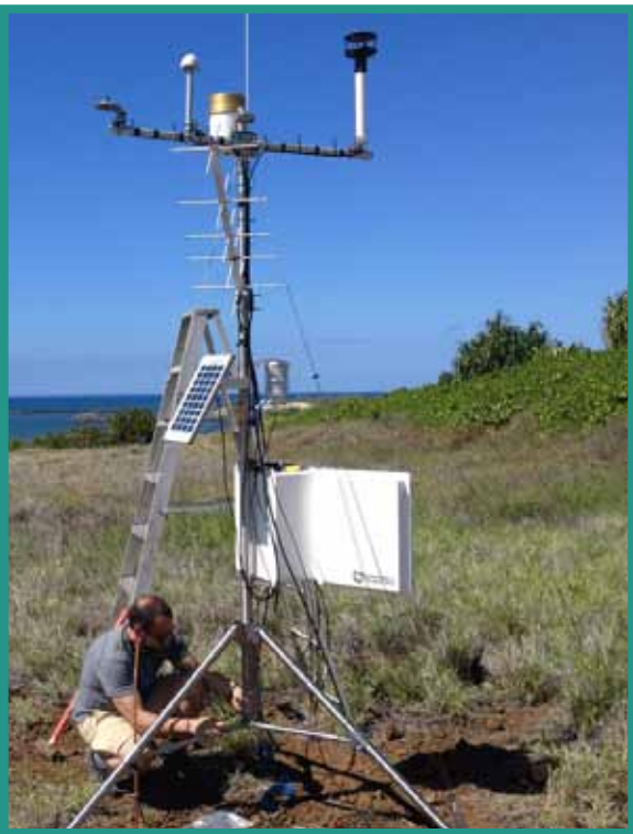
In June of 2013, the RAWS climate station at Pu'ukoholā Heiau National Historic Site (PUHE) was vandalized. A new station (above) was installed in January, 2015.
