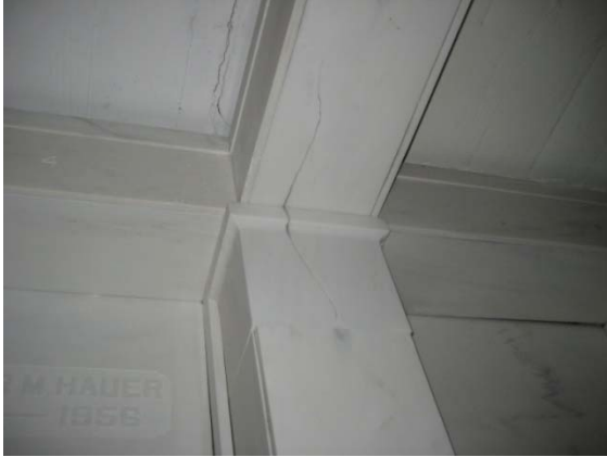
31 (Cracks at pilaster & beam.)
