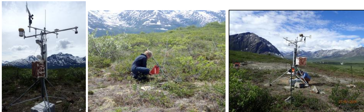
Figure 13. Tana Knob station June 20, 2016. Some cables (left) and the electric fence (middle) were damaged upon arrival. The station was functioning properly after completion of the field visit (right).
