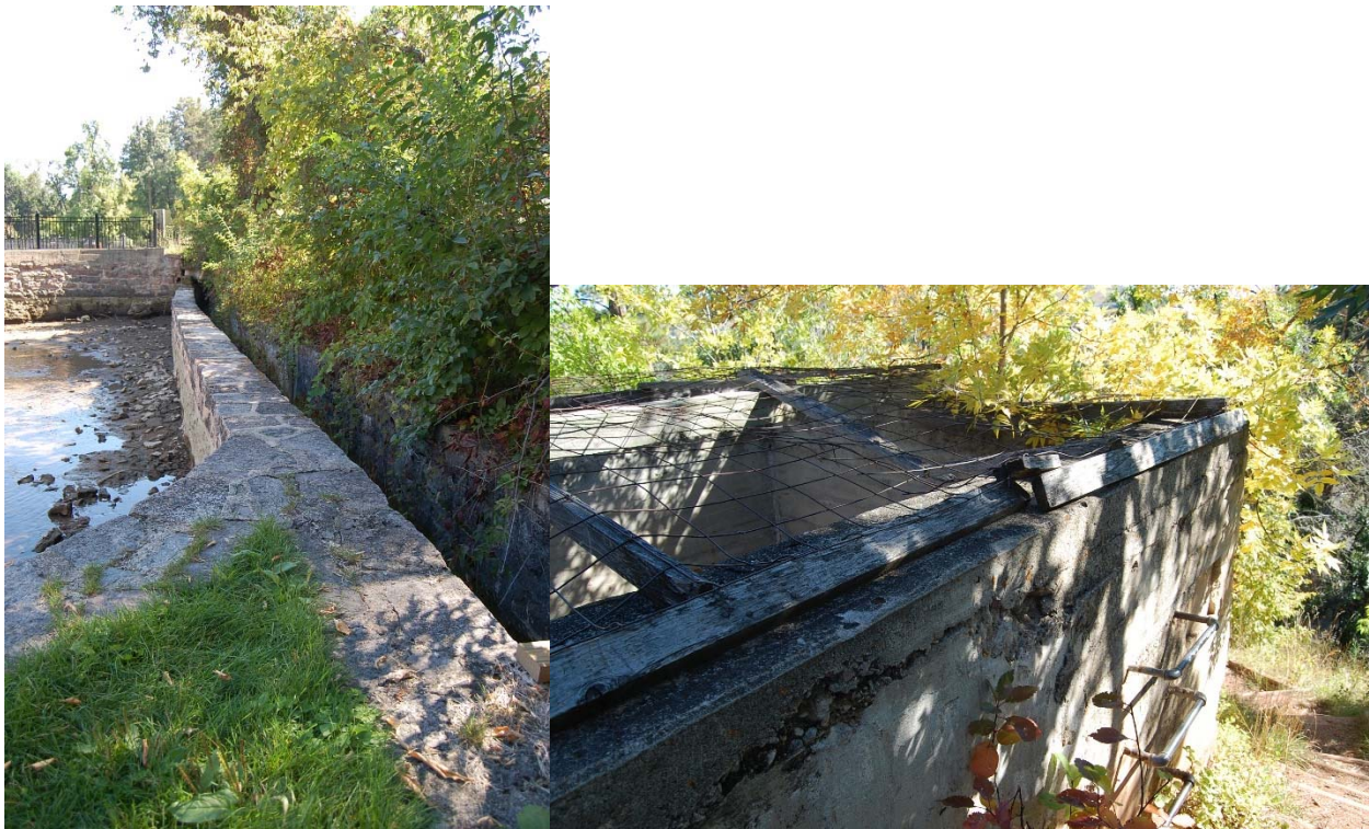
Figure 11. Storm Channel, Facing N; Holding Reservoir, Facing NE
