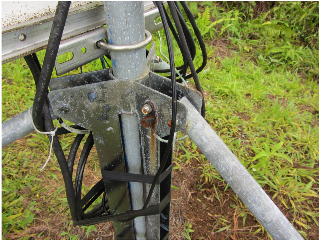
Figure 2 - Corrosion on the grounding system - Toa Ridge.
