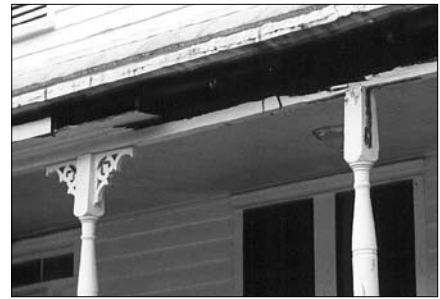
Replace missing original details in kind.
