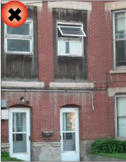
Inappropriate reduction in window size.
