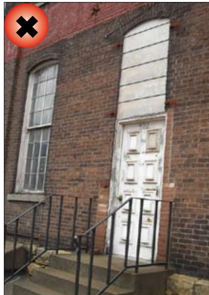
Inappropriate door and transom replacement.
