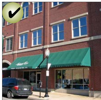
Appropriate installation of an operable awning.
