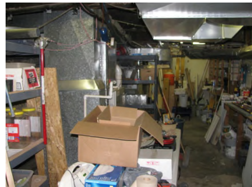
Existing workshop (multiple furnaces installed)
