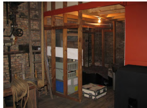
Existing furnace installed on stage=right
