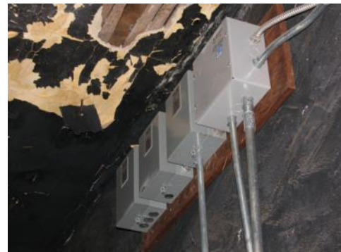
Marquee Lighting Contactors
