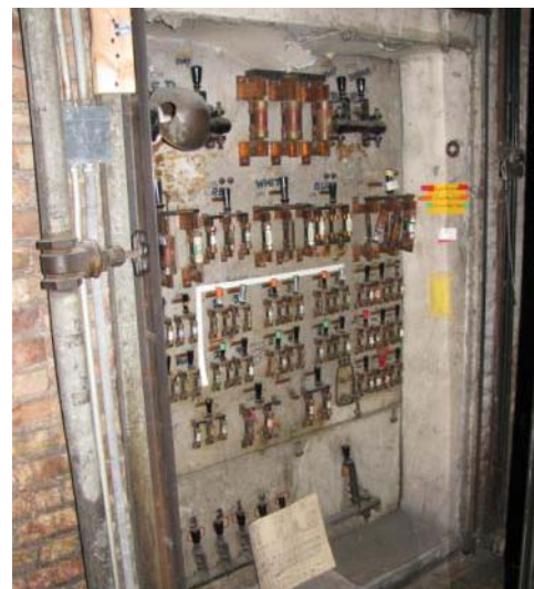
Stage Right Theatre Switchboard
