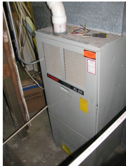
Existing basement furnace
