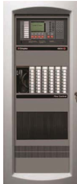
Fire Alarm Control Panel
