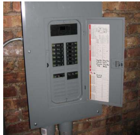
Stage Left Auxiliary Power Panel
