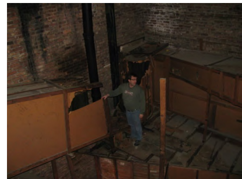
Existing supply ductwork above Auditorium
