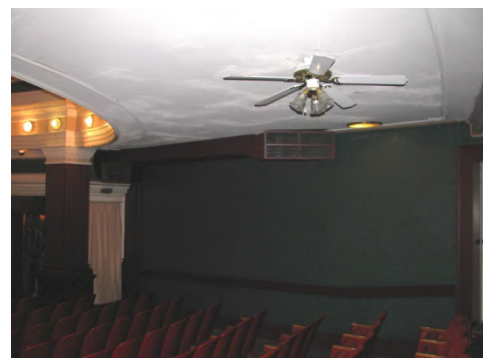
Existing supply air ductwork in Auditorium (House-right)
