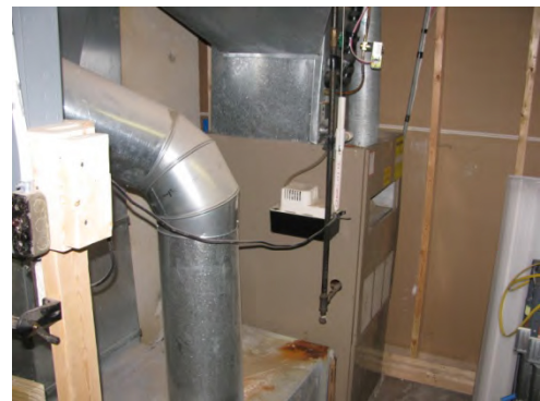
Existing basement furnace
