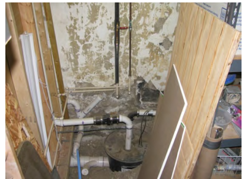
Existing sump pump/sewage ejector
