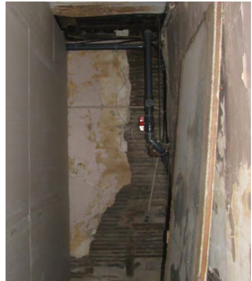
Existing domestic water service
