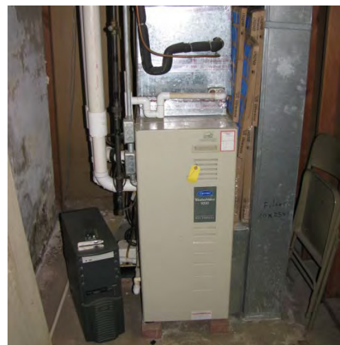
Existing basement furnace
