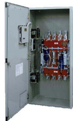
Automatic Transfer Switch
