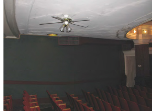
Existing supply air ductwork in Auditorium (House-left)
