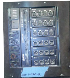
Typical Production Panel
