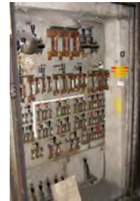
Existing lighting control panel
