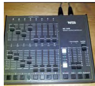
Existing front wash lighting controller
