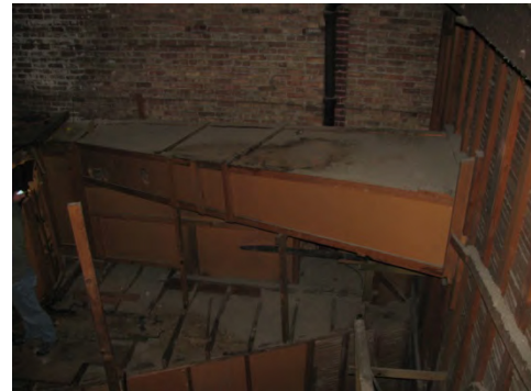
Existing supply ductwork above Auditorium
