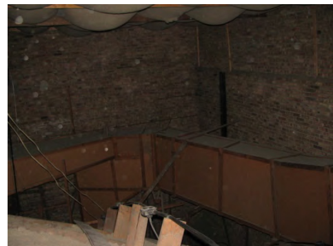
Existing supply ductwork above Auditorium
