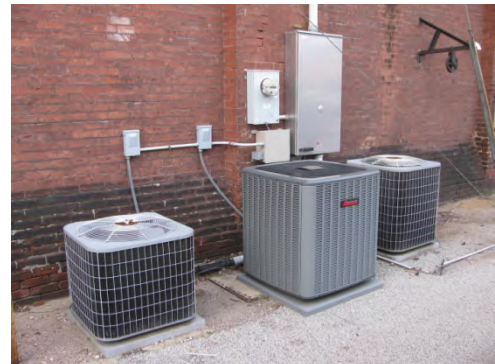
Existing air-cooled condensing units in alley
