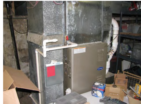
Existing basement furnace
