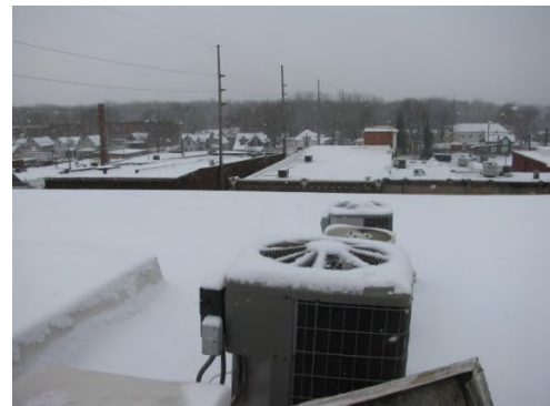
Existing air-cooled condensing units on roof
