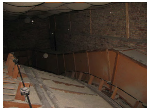
Existing supply ductwork above Auditorium
