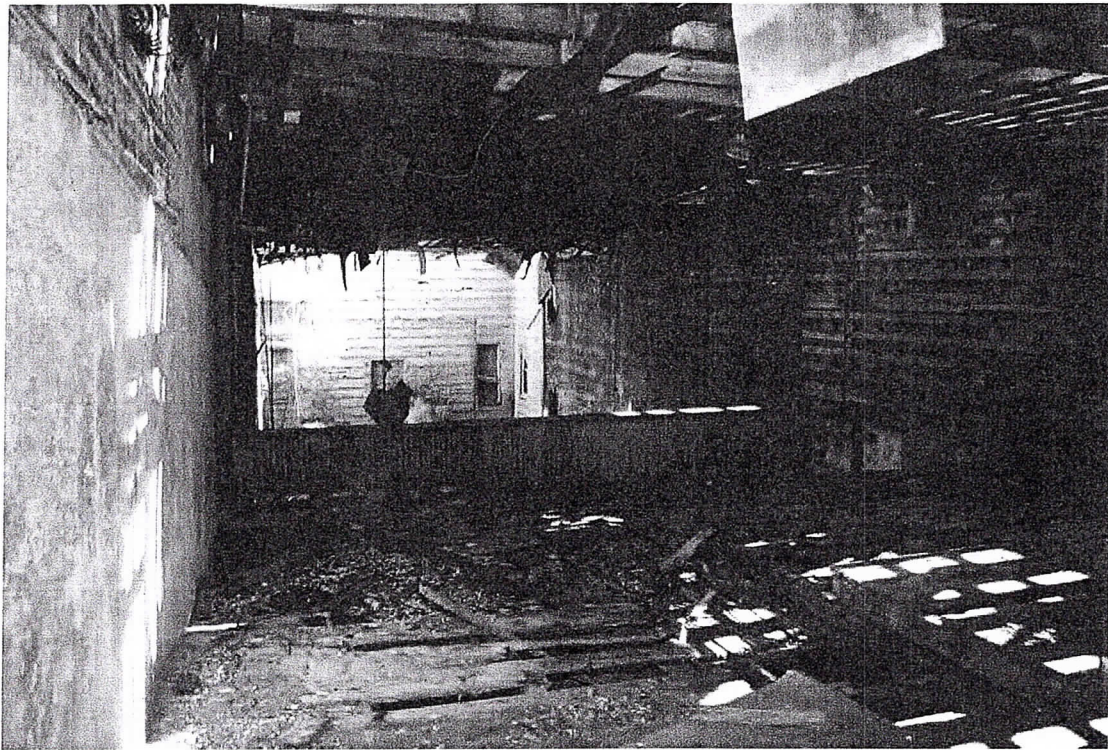
Upstairs Balcony area – note sunlight at rear building and over balcony (roof collapse)
