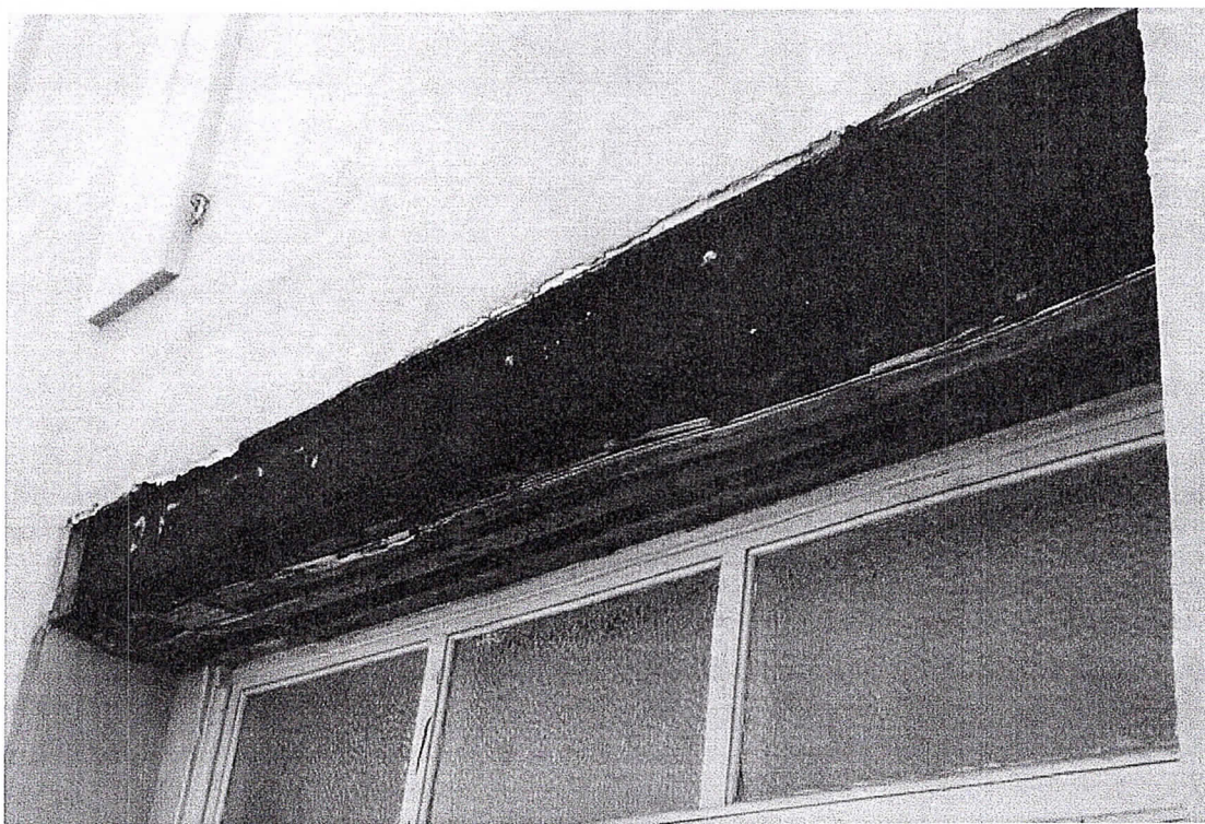
Steel Beam corrosion
