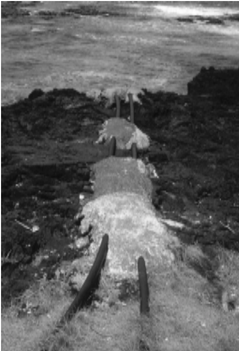
Figure 8. Seawater intake pipe at a giant clam hatchery in American Samoa (Simon Ellis).
