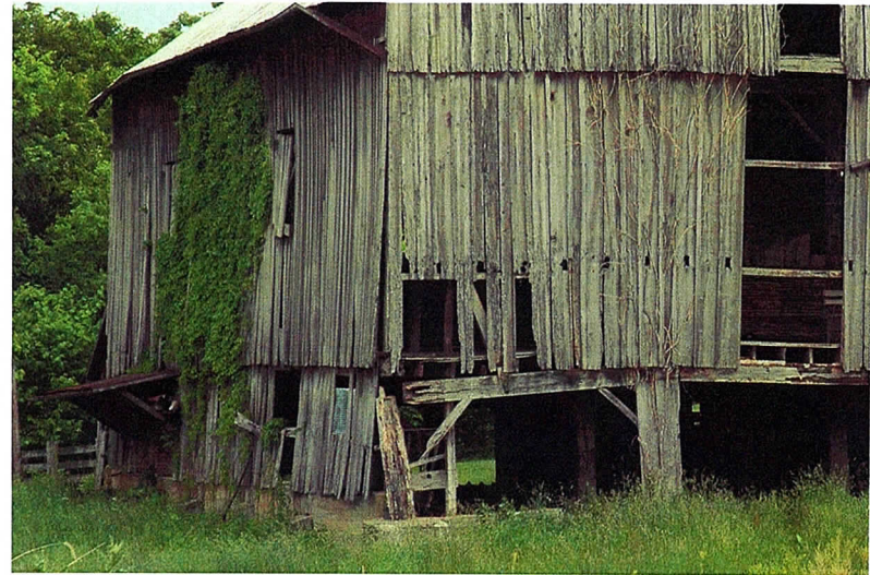
When roofs and siding no longer prevent water entry, barn structures will fail rapidly.
