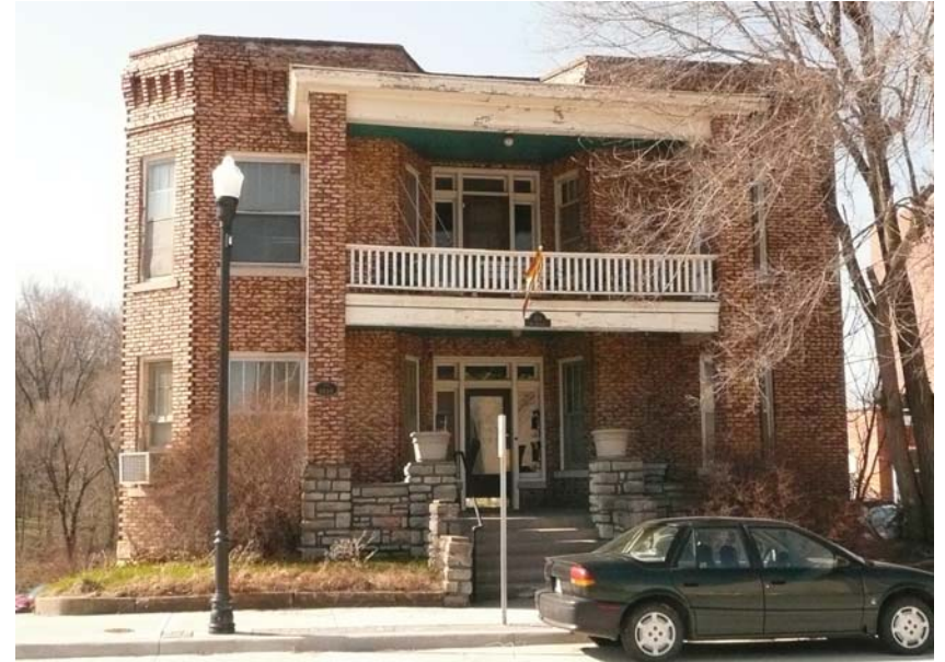
Historic Wood Porch Requiring Maintenance
