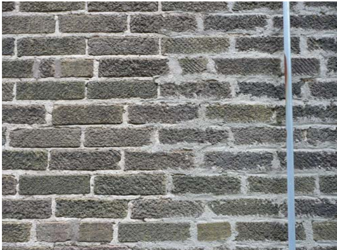
Incompatible Mortar Joint. These joints do not match the original joints in color, size or joint profile.
