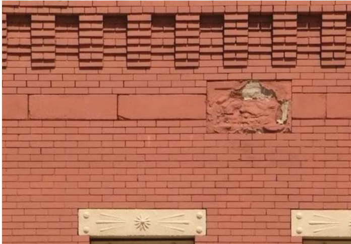
Historic Stone Unit Requiring Replacement
