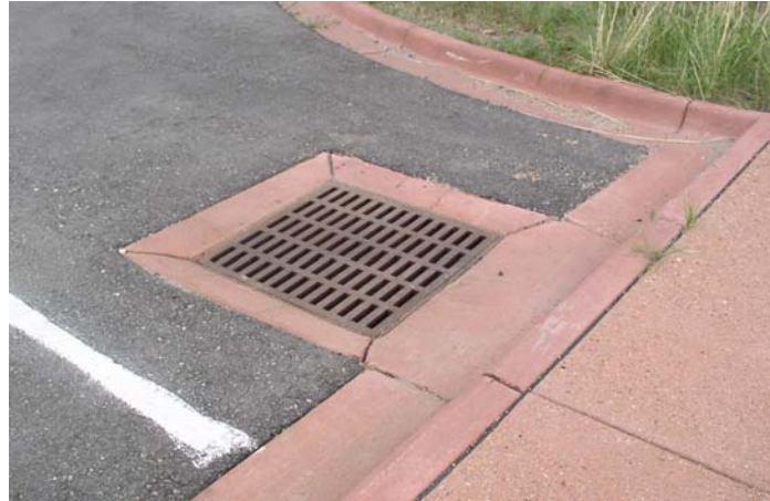
Steel drains match the color of the building's structural steel. (NPS-ROMO photo)
