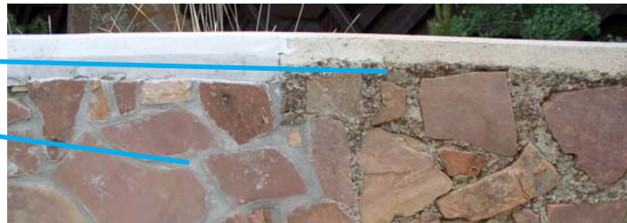
below: The original retaining wall at right has crumbled stone set in the mortar. The new retaining wall at left has a lighter colored concrete and lacks the crushed stone. (NPS-ROMO photos)
