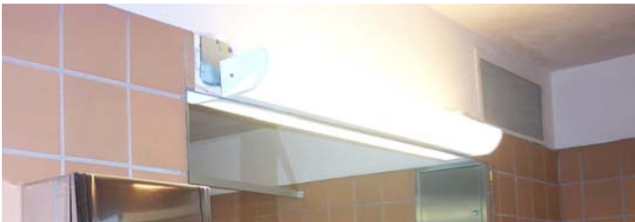
left: Original bathroom fixtures were of a simple, fluorescent design. (NPS-ROMO photos)
