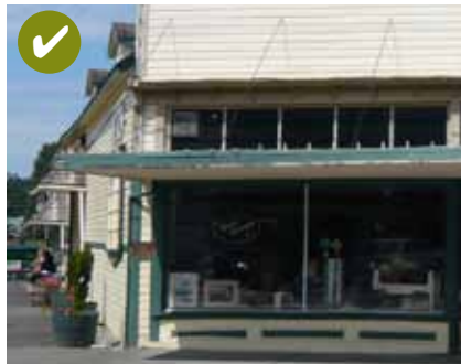
This fixed canopy is appropriately attached and located below the transom to maintain its operability.
