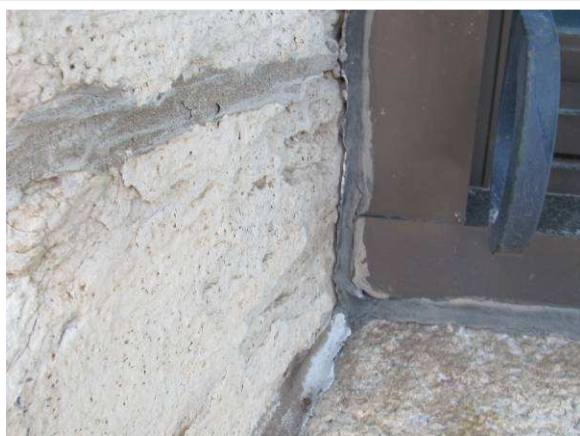
Failed mortar and sealant
