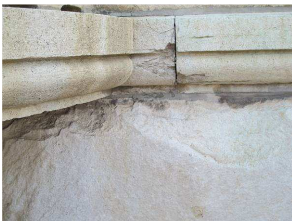
Failed mortar and deteriorating stone
