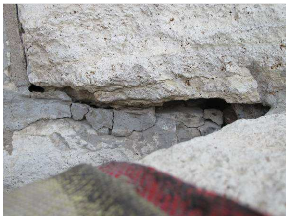
Broken mortar in joint
