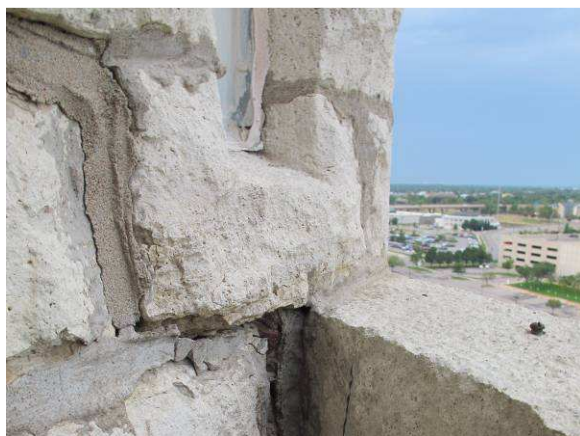
Failing mortar at balcony
