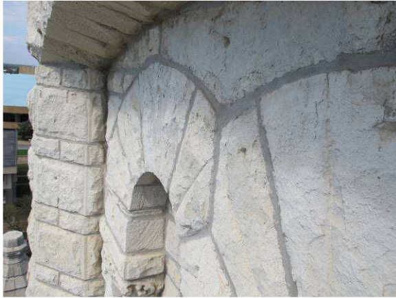
Loss of detail at arch
