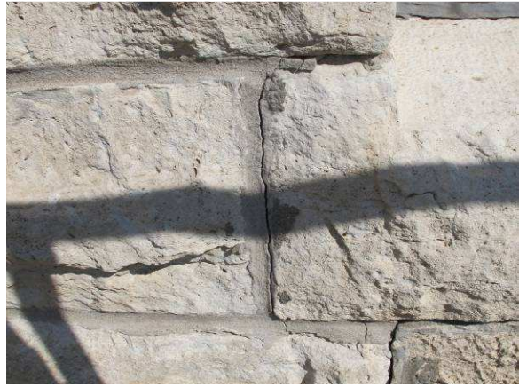
Debonded mortar joint and failed mortar
