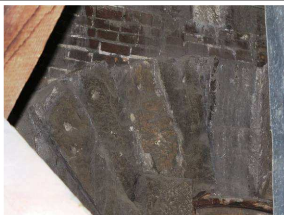
Smoke damage on interior stone arch
