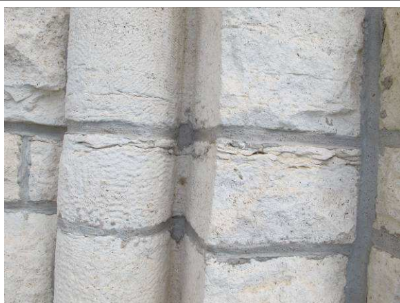
Delaminating naturally bedded stone
