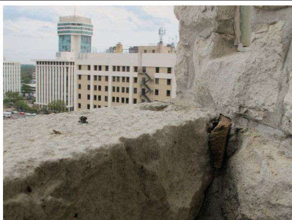
Exposed brick at balcony corner
