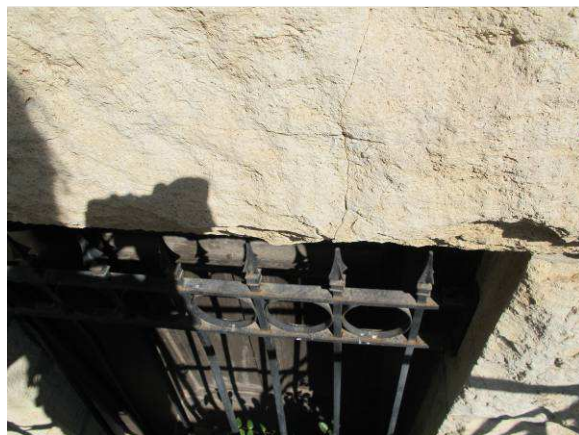
Crack in stone above window
