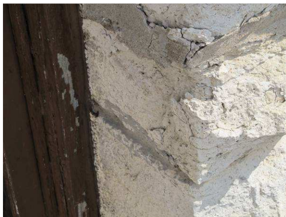
Deteriorating stone and mortar
