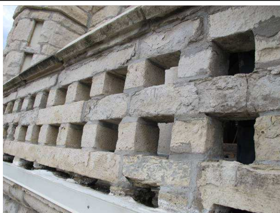
Delaminating stone at balcony
