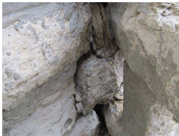
Deteriorating stone at balcony corner
