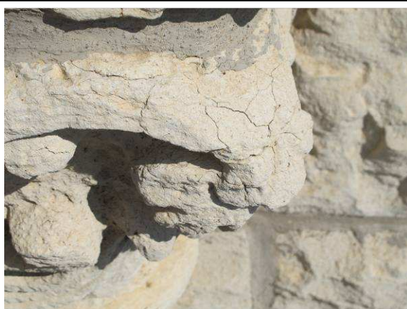
Deteriorating carved detail
