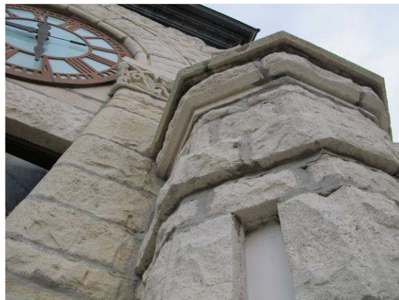
Poor mortar installation
