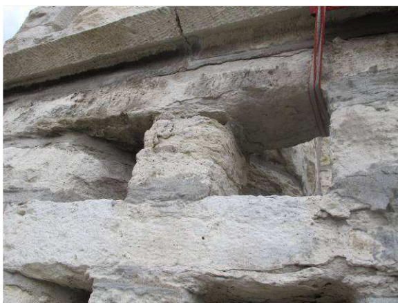
Deteriorating limestone at balcony
