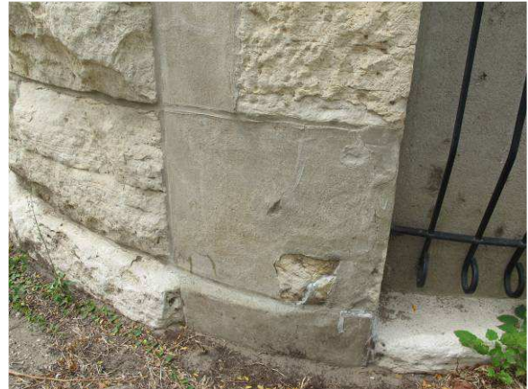
Failed parging on limestone
