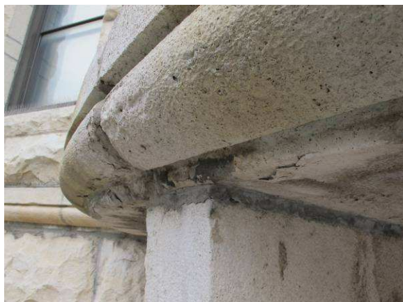
Deteriorating stone on underside of balcony
