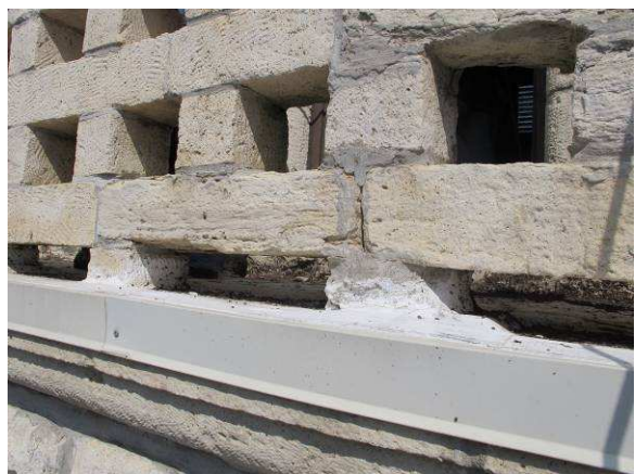
Poor repairs and deteriorating stone at balcony
