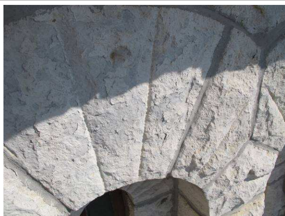
Loss of surface detail at arch
