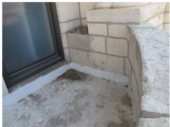
Extensive sealant around balcony
