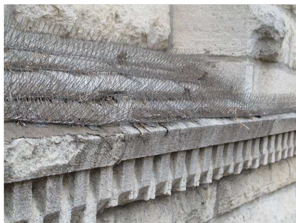
Spalled stone above dentil
