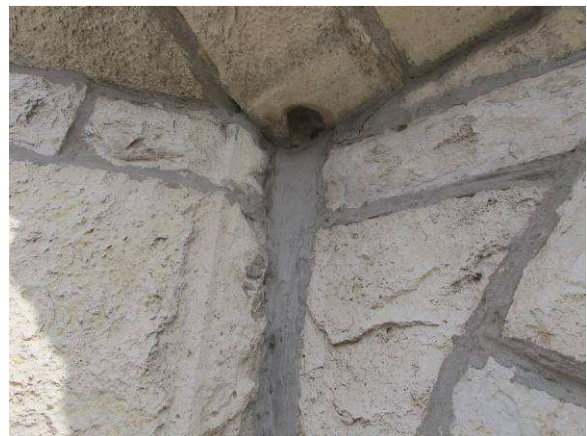
Poor mortar installation
