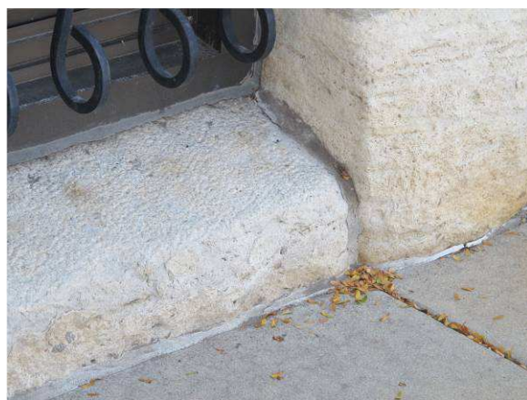
Failed sealant at window and sidewalk
