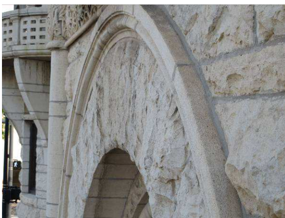
Loss of stone detail above main entry
