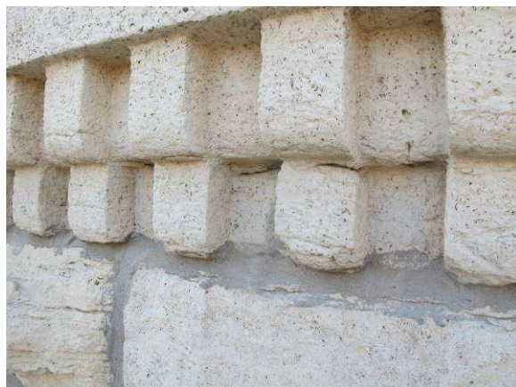
Poor mortar installation
