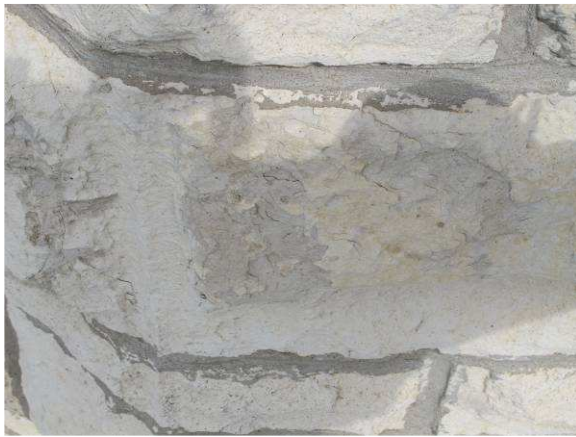
Spalled face of stone
