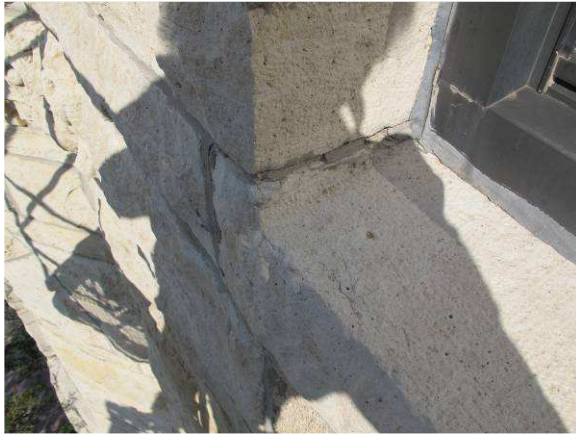
Failed mortar and sealant at window
