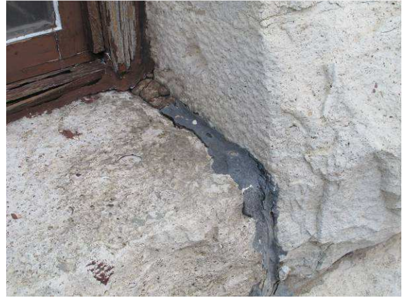
Failed caulking and deteriorated wood
