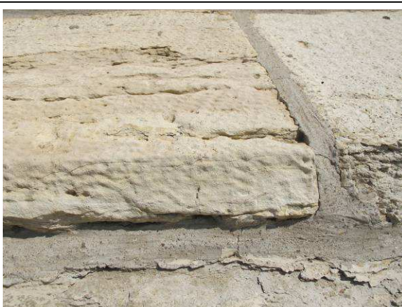
Deteriorating mortar and limestone
