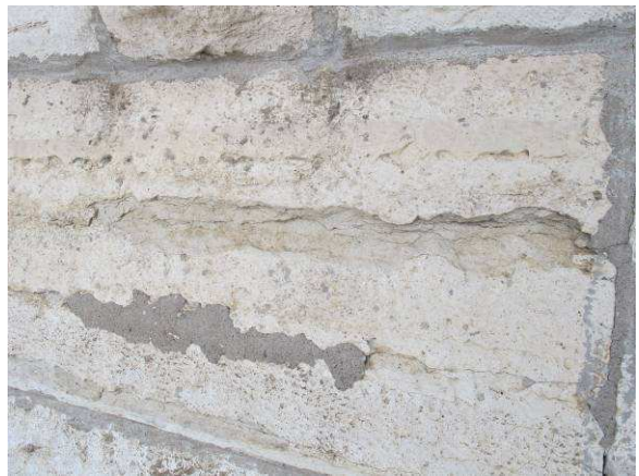
Deteriorating stone and poor repair below column
