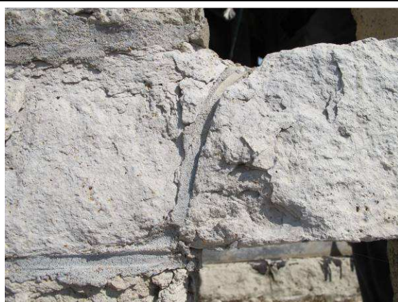
Poor repairs at balcony rail
