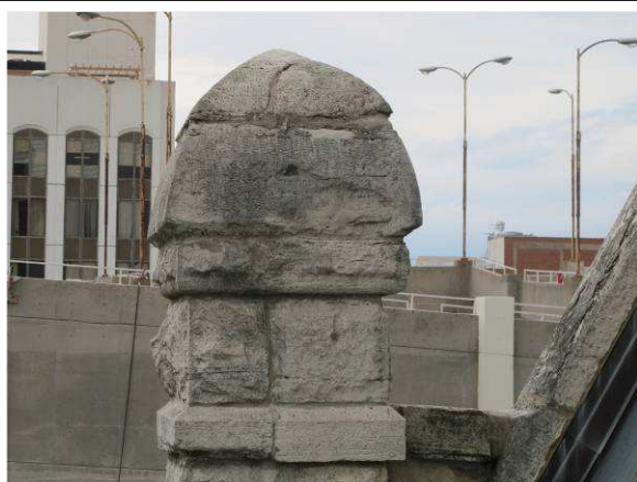
Mortar failing at spire
