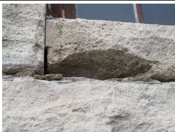
Missing stone and mortar
