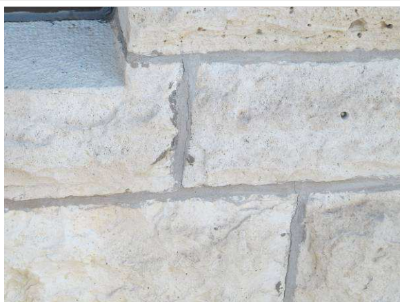
Cracked vertical mortar joints
