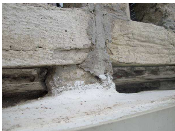
Poor mortar installation
