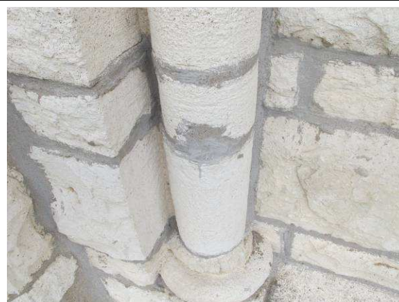
Poor mortar installation
