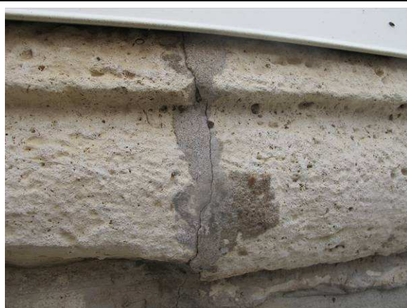
Crack in mortar joint
