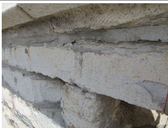
Deteriorated stone and mortar at balcony
