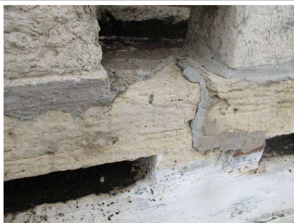
Deteriorated stone and failed mortar joint
