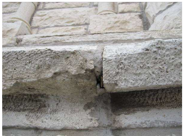
Deteriorated stone at joint
