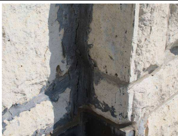
Poor mortar installation at return
