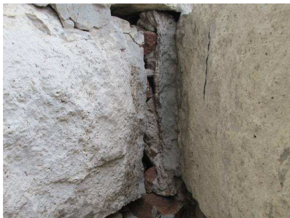
Exposed brick at balcony corner
