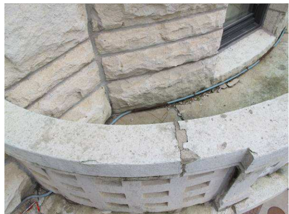
Failed mortar repair
