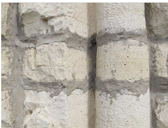
Poor mortar installation
