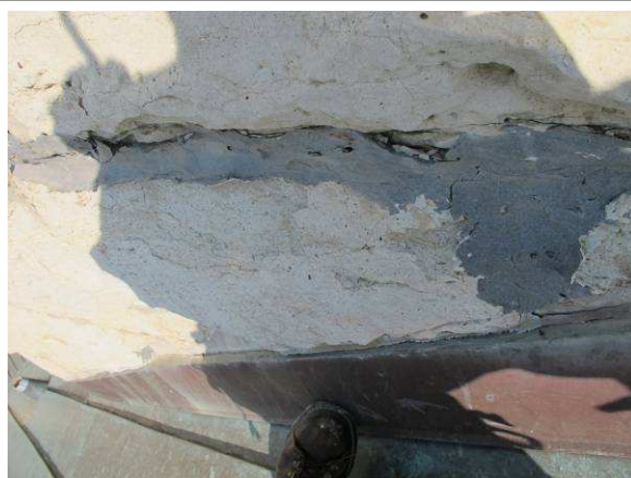
Deteriorating mortar near flashing
