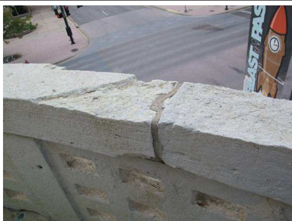
Deteriorated balcony rail
