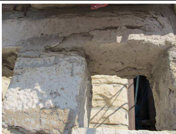
Deteriorating limestone at balcony rail
