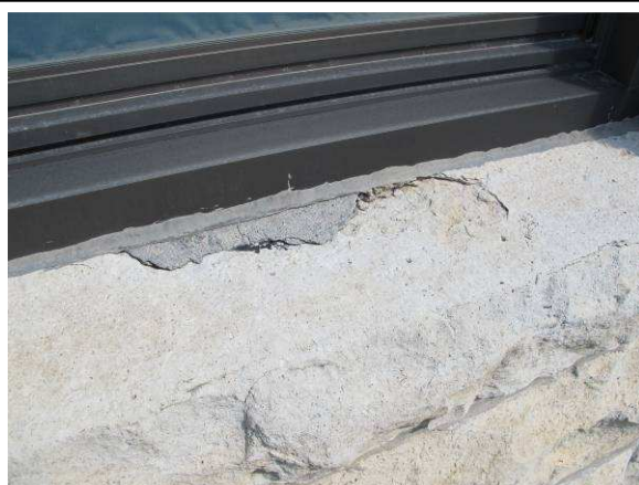
Exfoliating window ledge and failed repair
