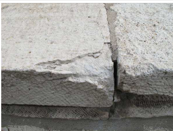
Failed mortar joint and spalled stone
