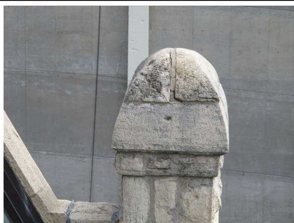
Failing mortar at roof edge spire
