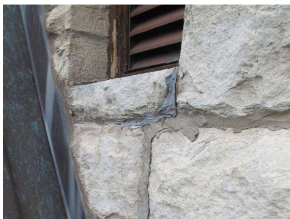
Failed caulking and separated mortar
