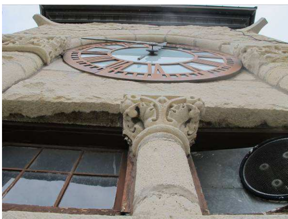
Water evidence at window headers
