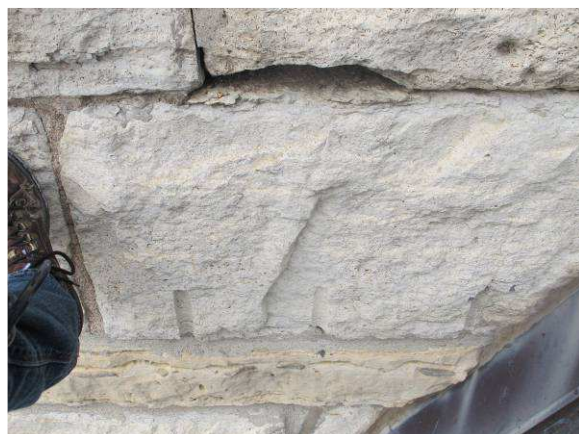
Missing mortar above flashing
