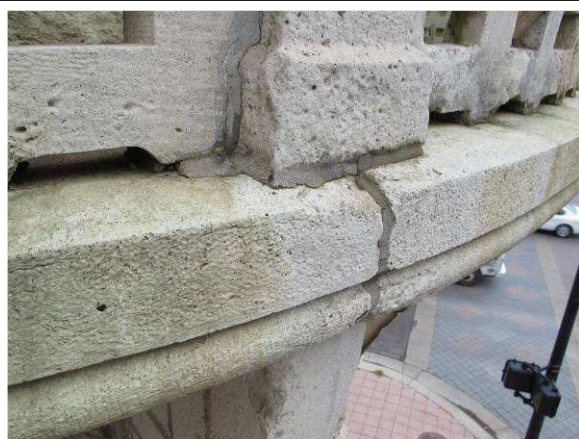
Poor mortar installation
