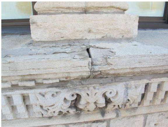
Damaged stone and open skyfacing joint
