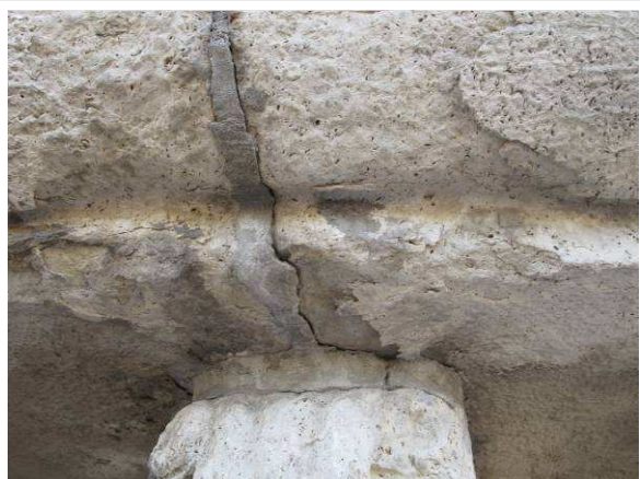
Failed joint and deteriorated stone
