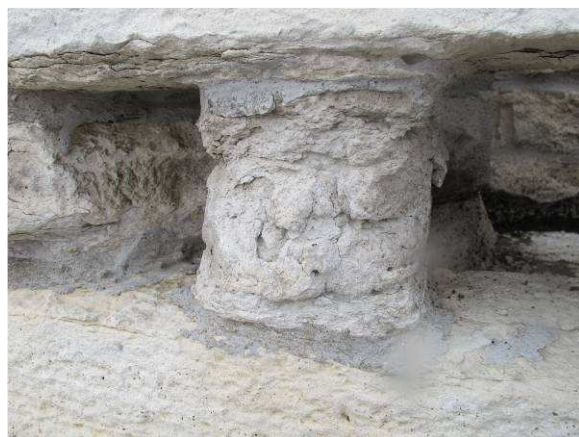
Deteriorating stone at balcony
