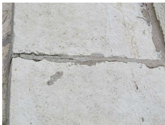
Separated mortar joint
