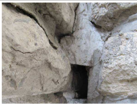
Missing brick at balcony corner
