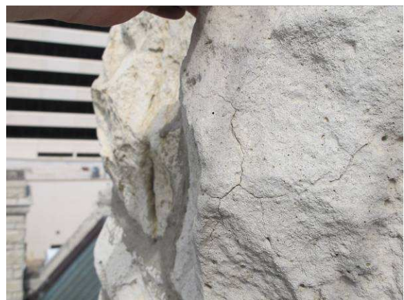
Deteriorating and spalling stone
