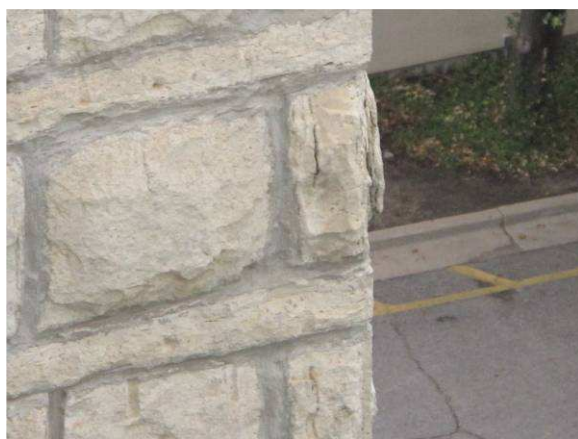
Spalling stone on opposite side of chimney
