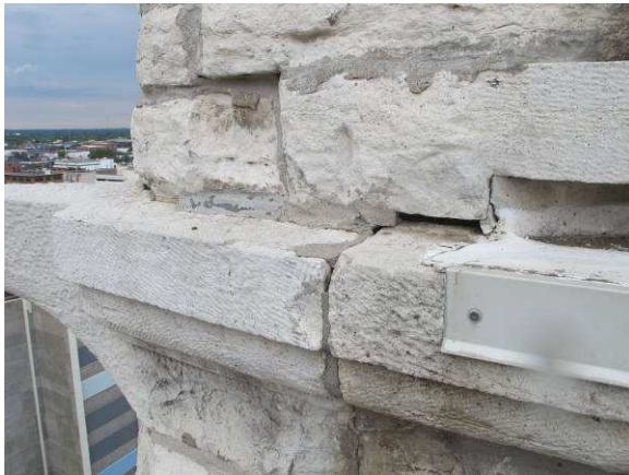
Failed mortar and deteriorating stone
