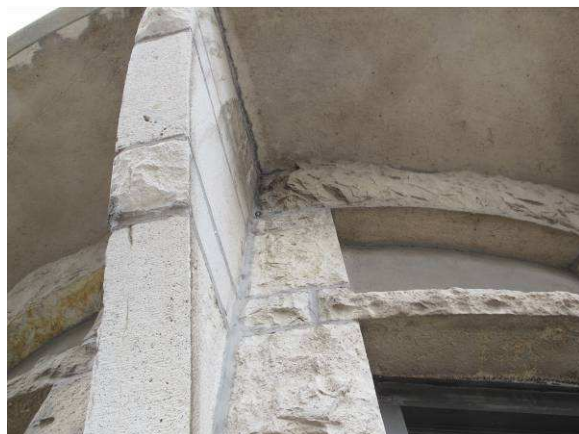
Deteriorating stone on underside of balcony
