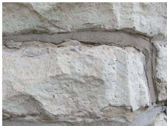
Failing mortar at balcony
