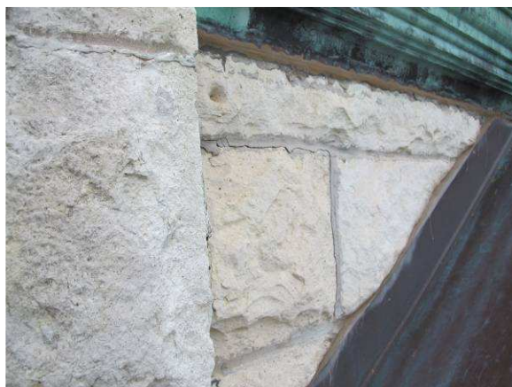
Failing mortar joints near roof sealant
