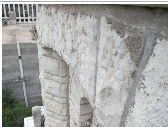
Deteriorated limestone and poor mortar
