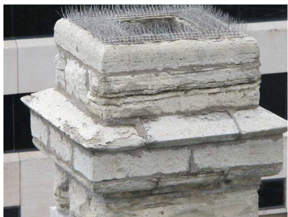
Mortar loss and deteriorating stone
