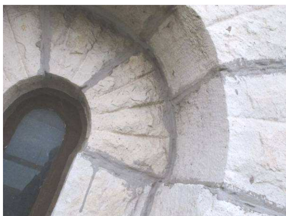
Poor workmanship and failing joints
