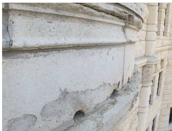
Deteriorated stone at balcony face
