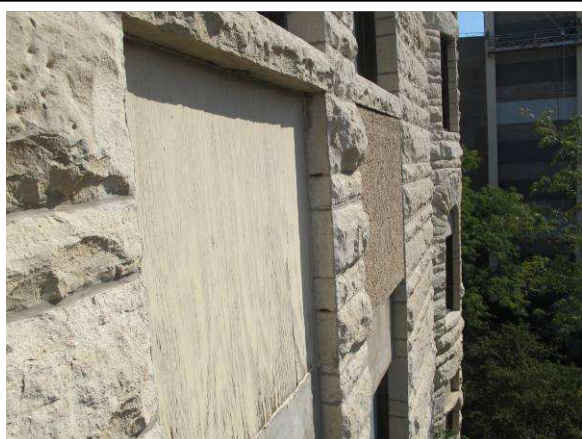
Missing cement board
