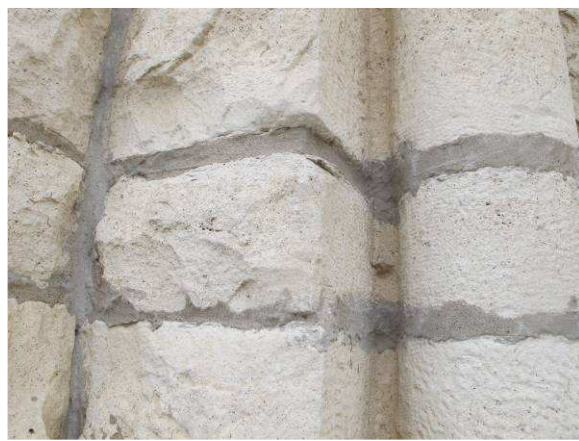
Poor mortar installation
