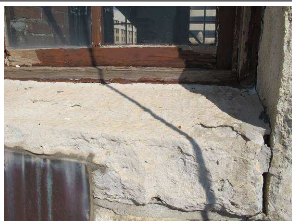
Deteriorating window, limestone and mortar
