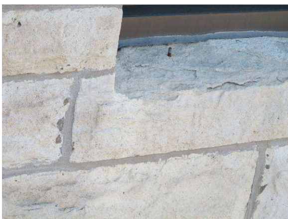
Deteriorating stone ledge
