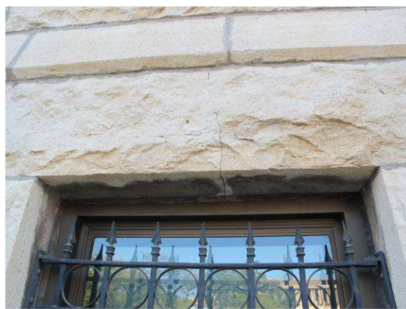
Cracked header stone
