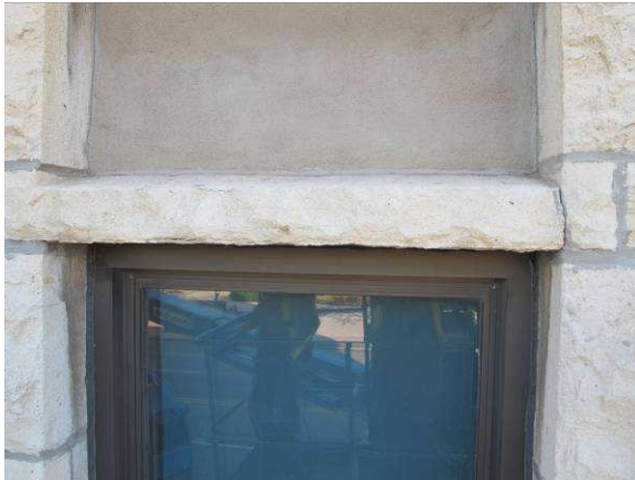
Failed mortar joint at header
