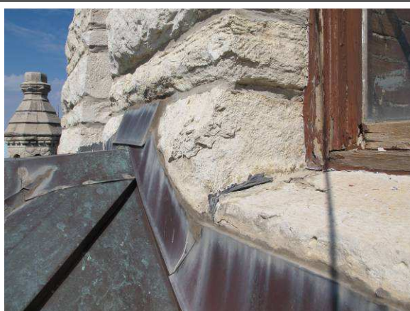
Deteriorating window, limestone and mortar
