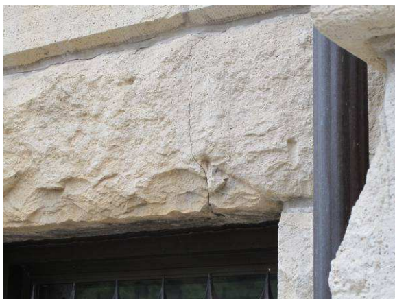
Cracked header stone
