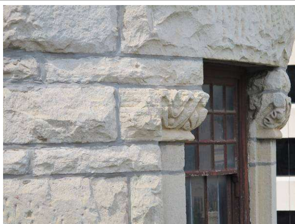
Deteriorating wood window
