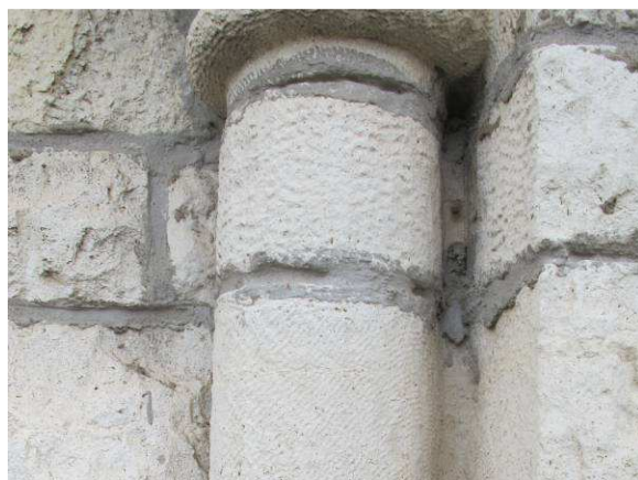
Poor mortar installation
