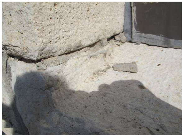
Failed joint at window
