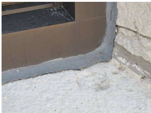
Failed window sealant
