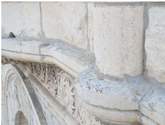
Close up of deteriorating stone
