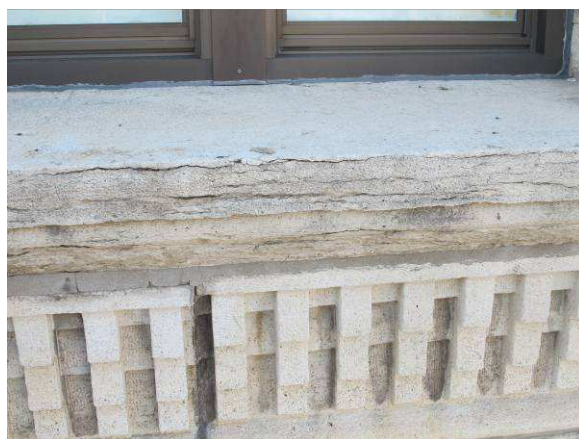
Delaminating stone ledge
