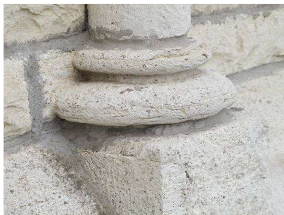
Loss of mortar at column base
