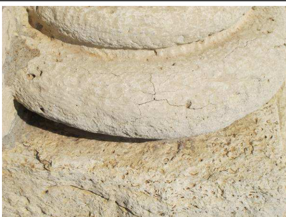
Deteriorating stone at column base
