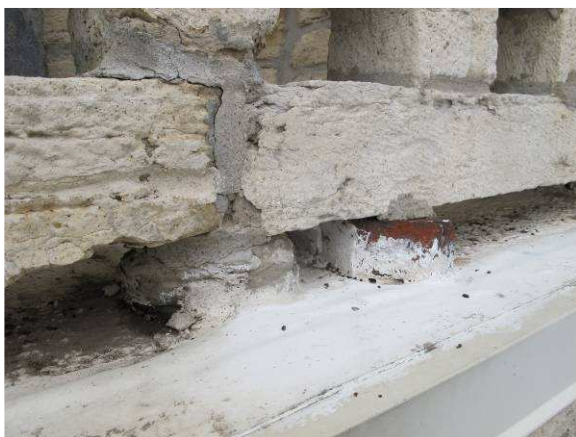
Missing stone and deteriorated mortar
