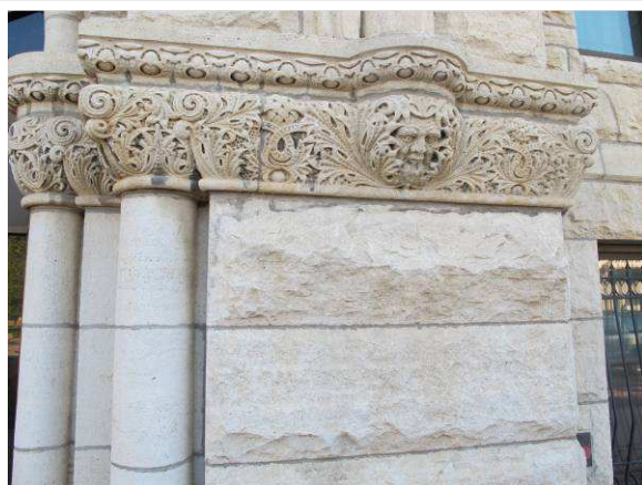
Poor mortar installation below carving
