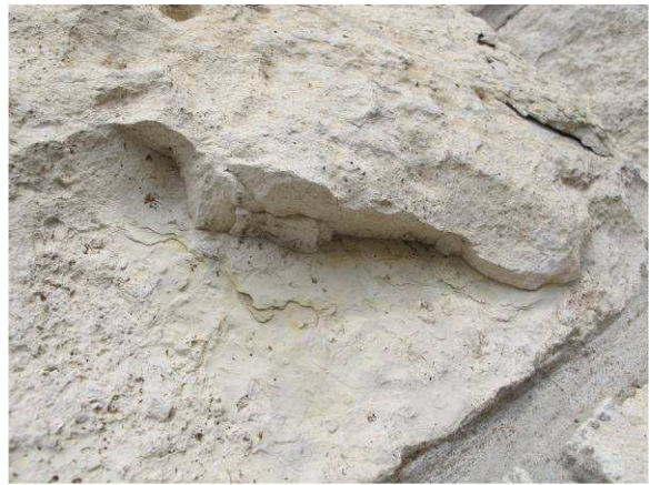
Partially spalled stone
