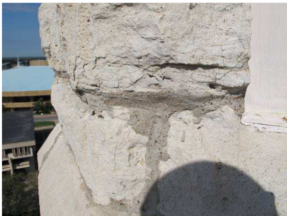
Poorly installed mortar and deteriorated limestone
