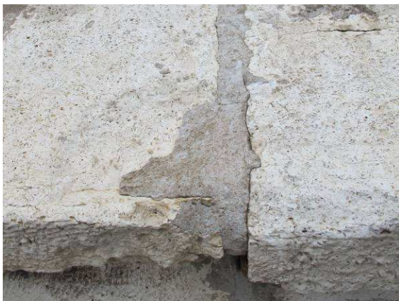
Separated mortar joint
