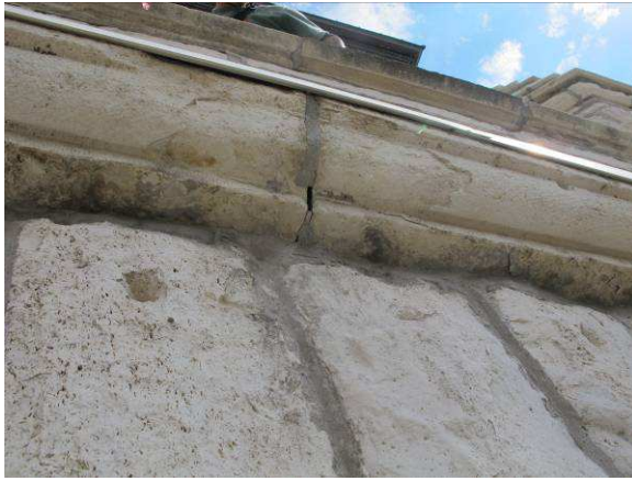
Open mortar joint and spalling stone
