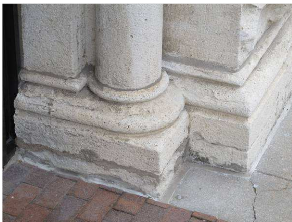
Delaminating stone at grade
