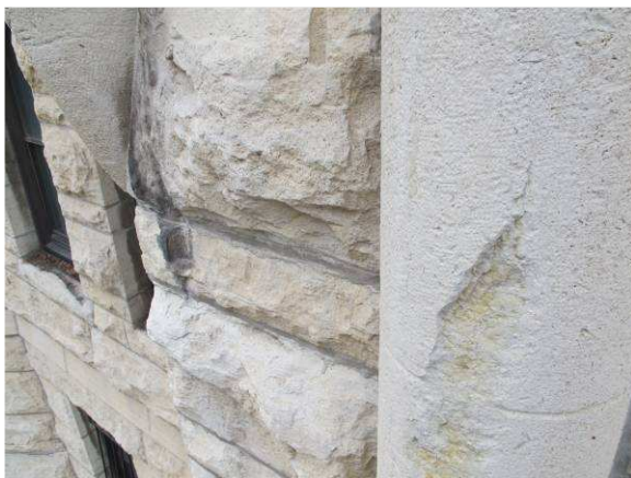
Damaged stone column
