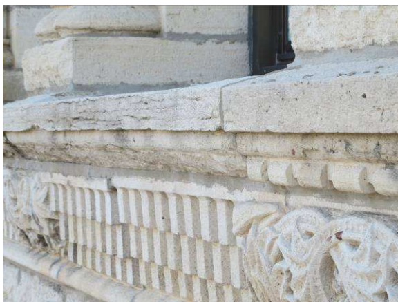
Delaminating and exfoliating stone
