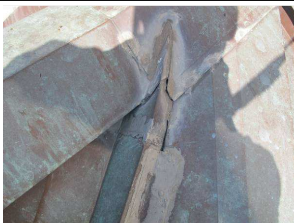
Poor flashing detail
