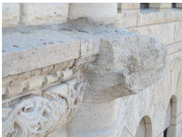
Damaged stone detail
