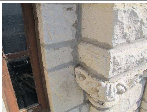
Poor mortar installation and decaying wood
