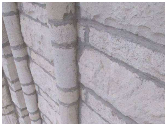
Poor mortar installation
