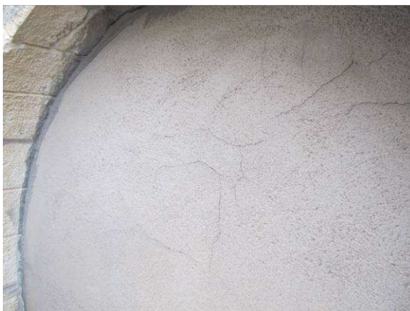
Cracked cement board
