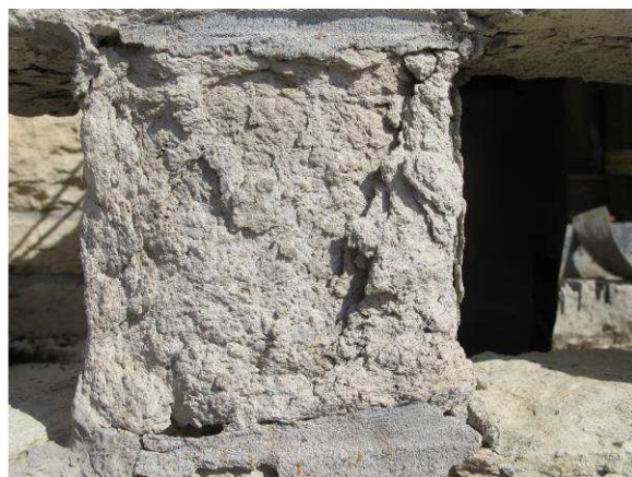
Deteriorating limestone at balcony rail
