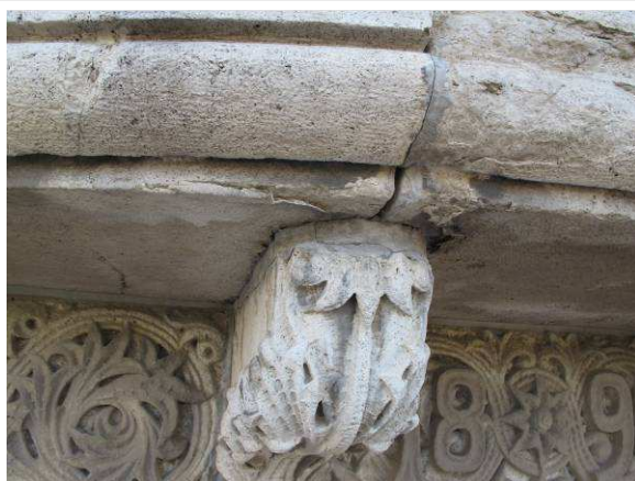
Failed joint and damaged stone above support
