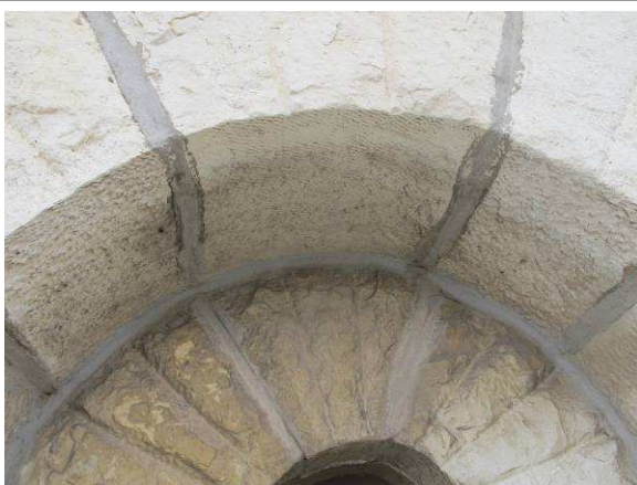
Failed mortar and stone loss at arch
