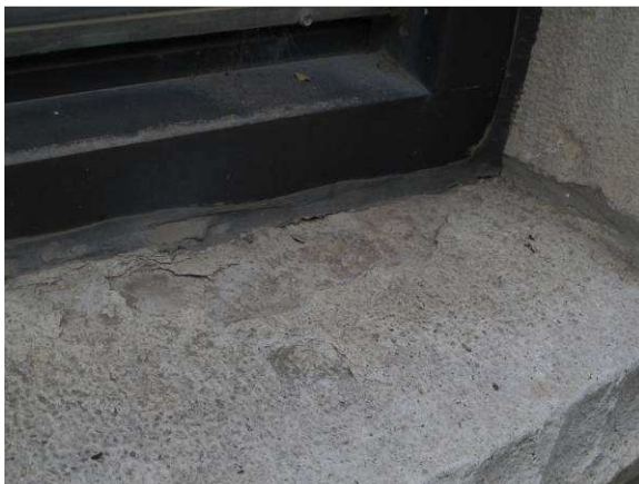
Deteriorating window ledge
