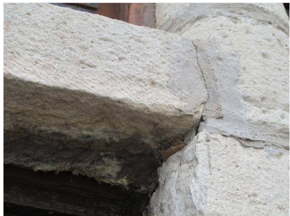
Crack in mortar at header
