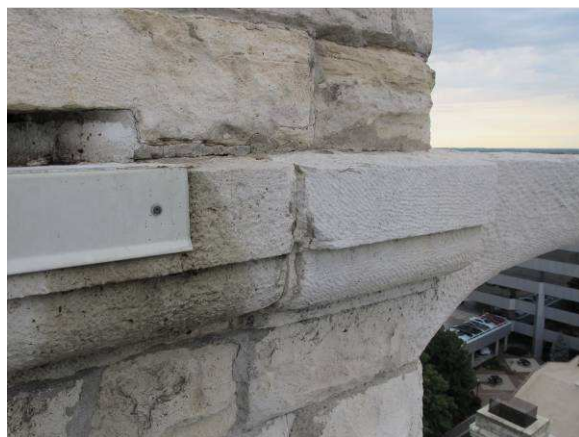
Deteriorating stone and mortar
