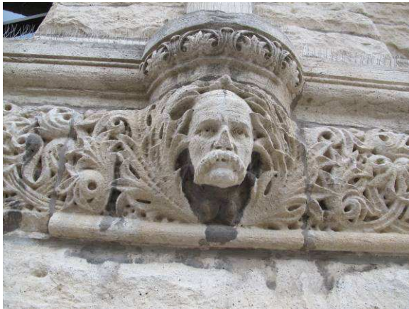
Poor mortar installation
