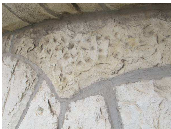
Loss of stone detail
