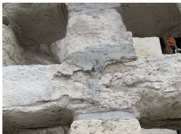
Failed mortar and damaged stone
