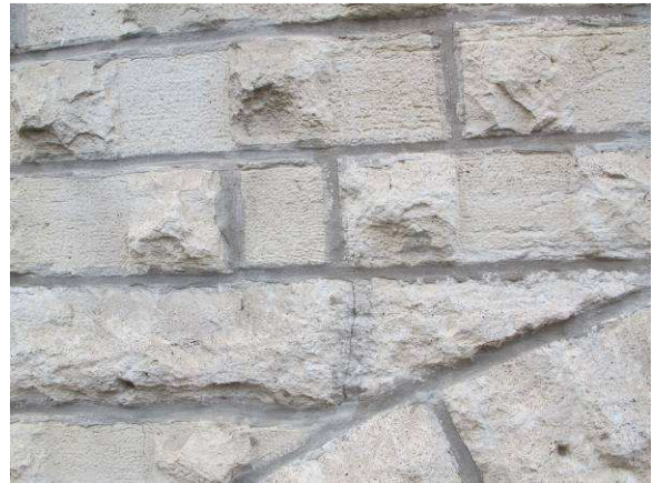
Separated mortar joints
