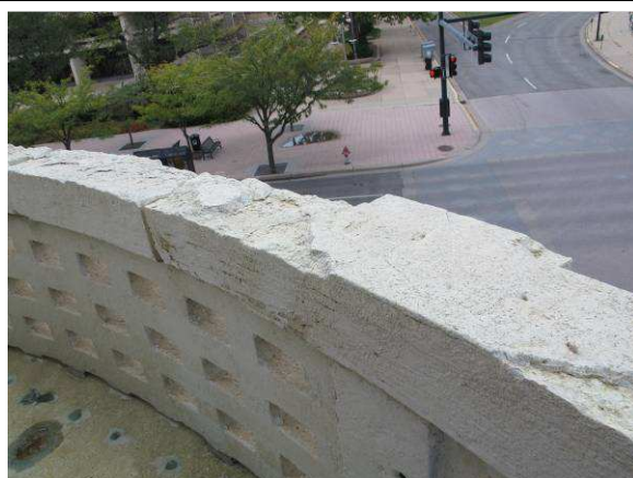
Deteriorated balcony rail
