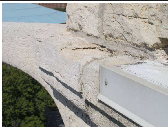
Deterioration at top of stone
