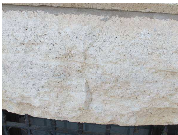
Cracked header stone
