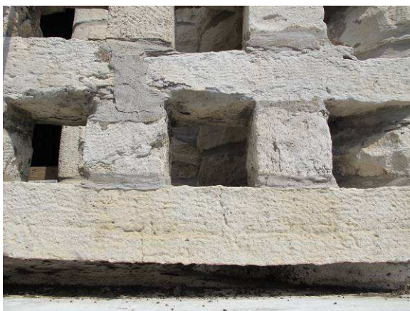
Poor repairs and deteriorating stone at balcony
