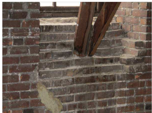
Repaired crack below window
