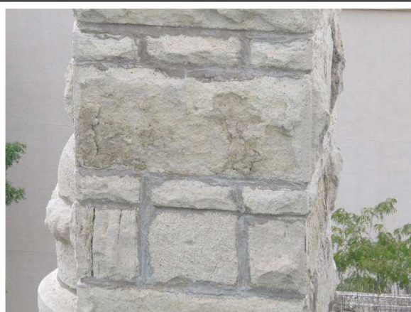
Deteriorating stone at chimney
