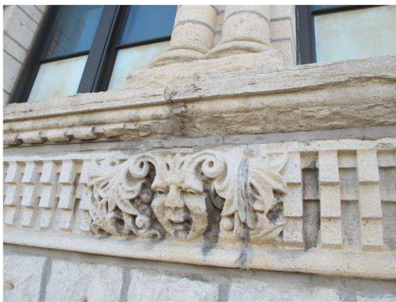
Deteriorating stone and poor mortar installation
