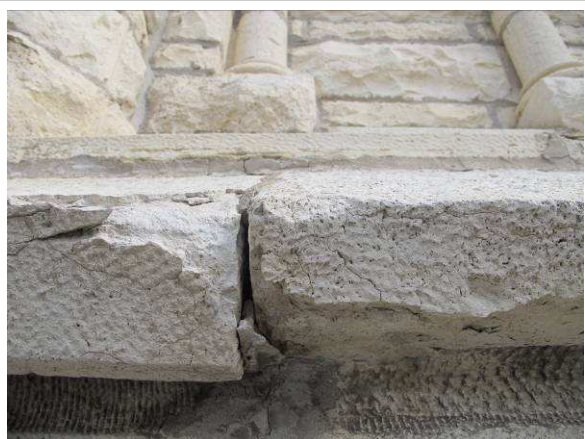
Failed mortar joint and spalled stone
