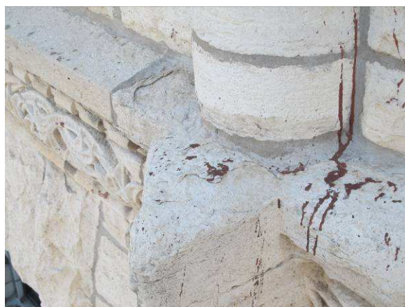
Spalling stone above entry
