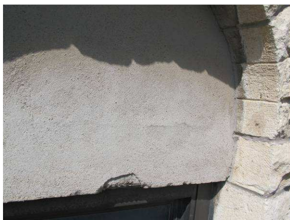
Damaged cement board
