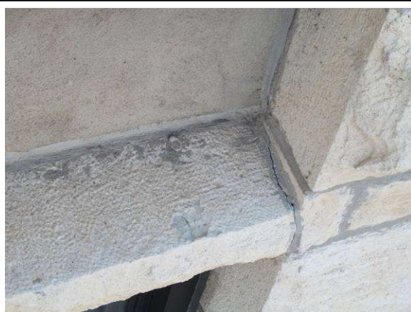
Failed mortar joint at header
