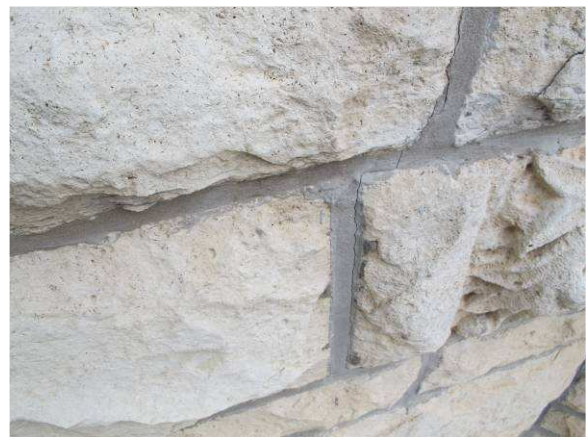
Cracked mortar joint
