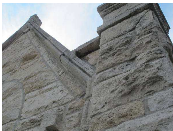
Broken stone above addition
