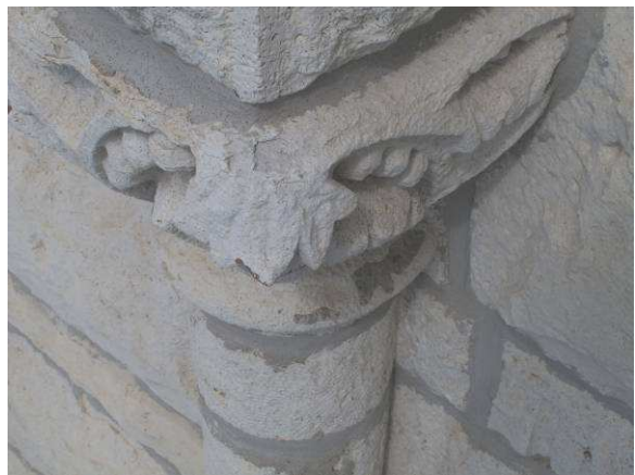
Poor mortar installation
