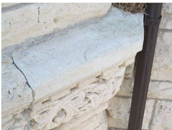
Open skyfacing joint
