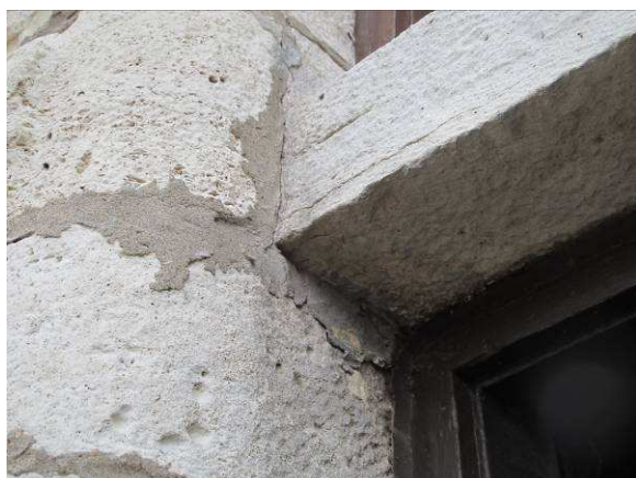
Poor mortar installation
