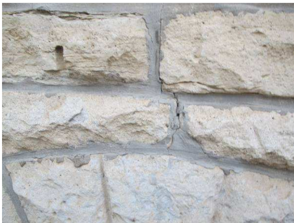
Crack running through joints
