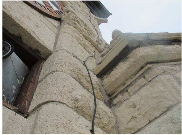
Decaying wood and missing mortar
