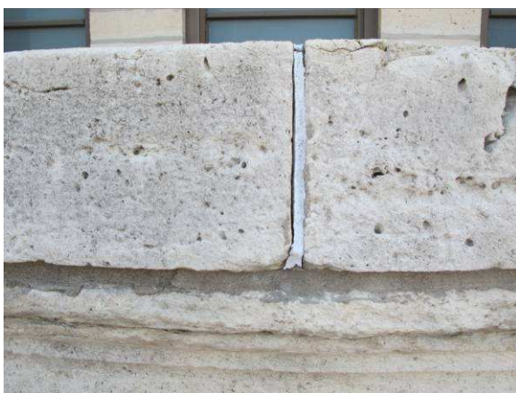
Separated joint and deteriorated stone at balcony
