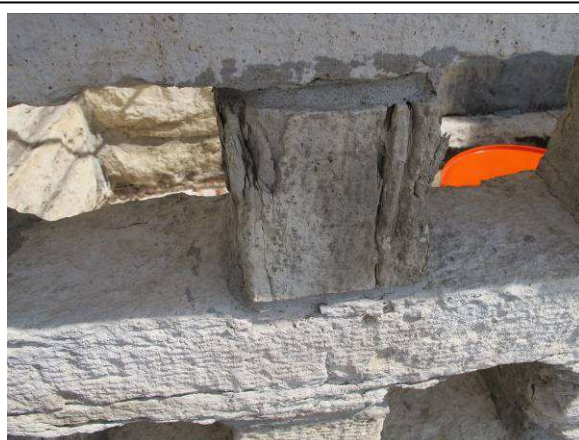
Failing stone at balcony
