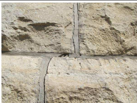
Separated and missing mortar
