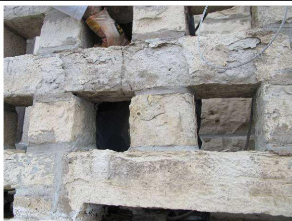
Delaminating stone at balcony
