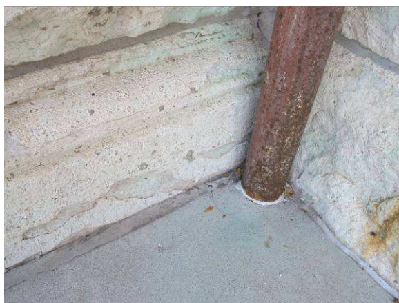
Failed sealant and deteriorating stone
