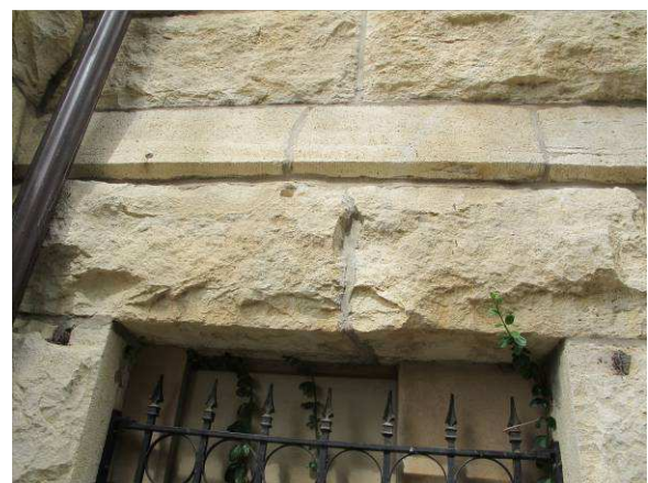
Cracked stone above window
