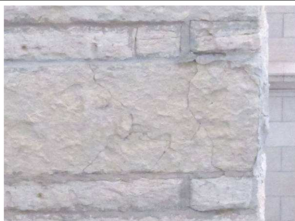
Deteriorated stone in chimney
