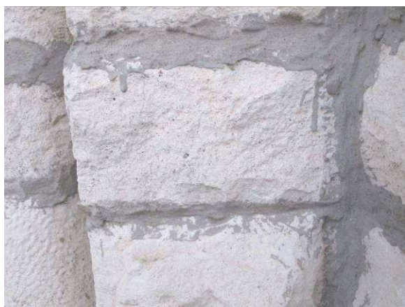
Poor mortar installation
