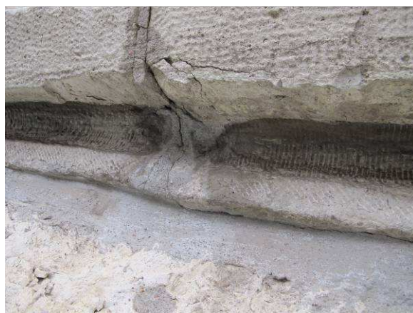
Failed mortar joint and deteriorated stone
