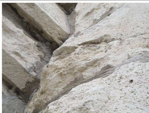
Poor mortar and failing stone
