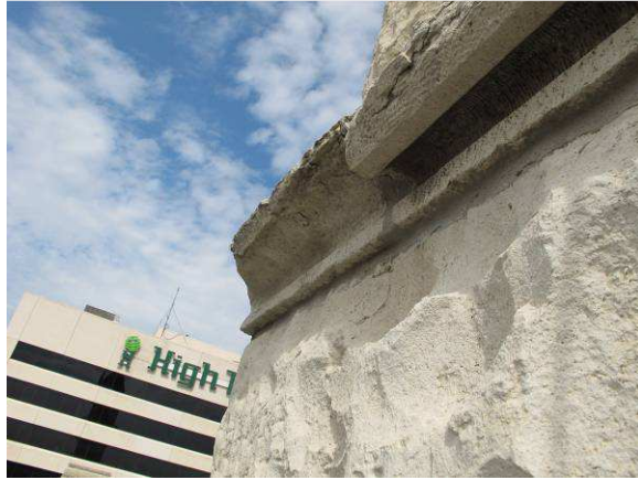
Spalled and delaminating stone
