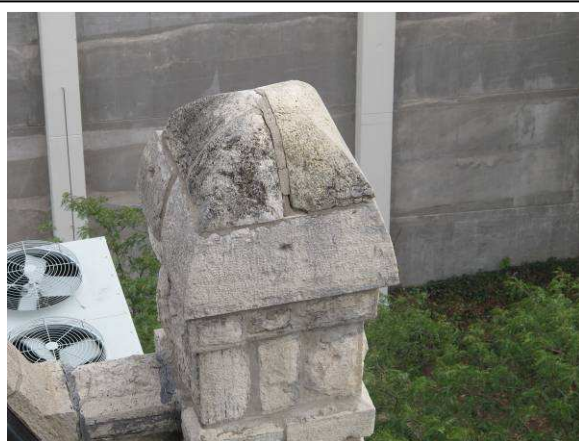
Failed mortar in spire
