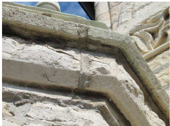
Separation at mortar joint
