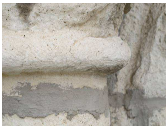
Poor mortar installation
