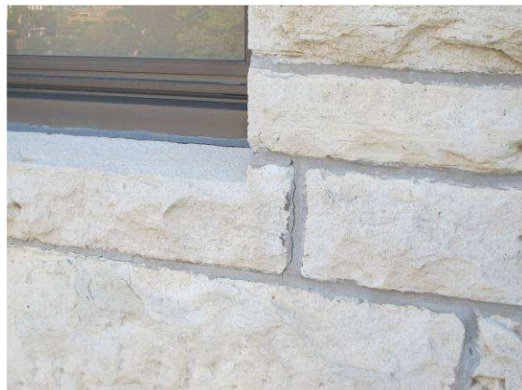
Cracked mortar joint
