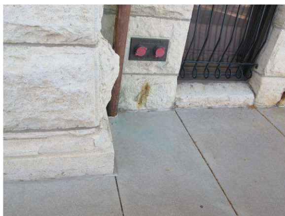
Damaged stone at grade
