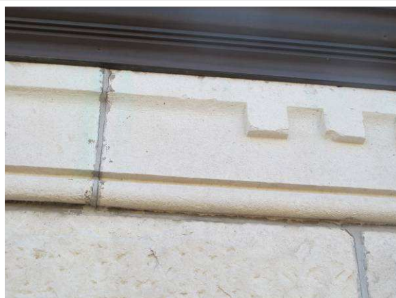
Debonded vertical mortar joints
