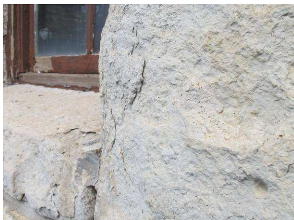
Deteriorating stone and wood window frame
