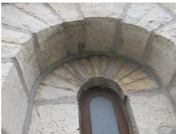
Poor mortar and stone damage at arch
