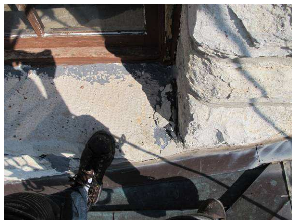
Wood window and ledge in need of treatment
