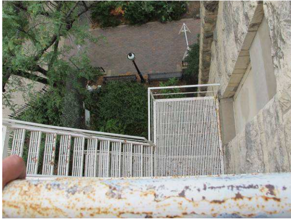
Painting failing on exterior fire escape
