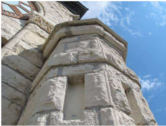
Poor mortar installation
