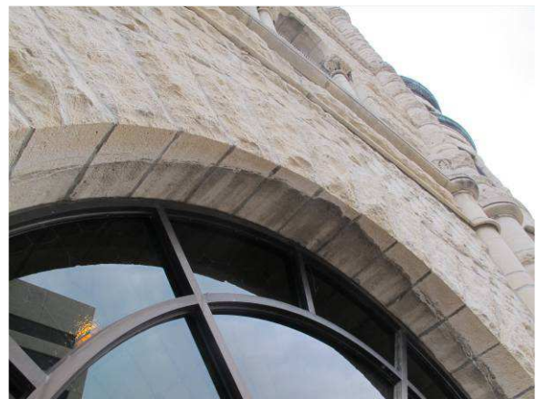
Evidence of water damage above arch
