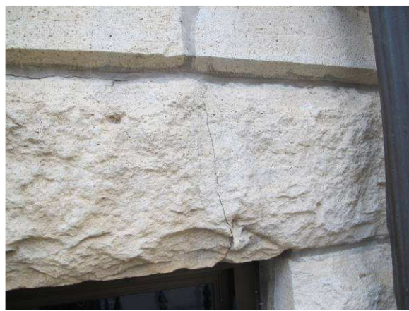
Cracked header stone
