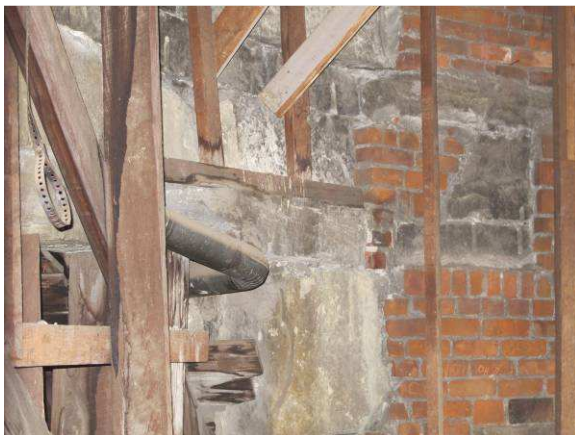
Evidence of smoke damage
