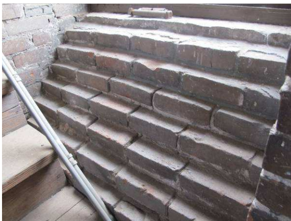
Missing mortar in interior brick wythes
