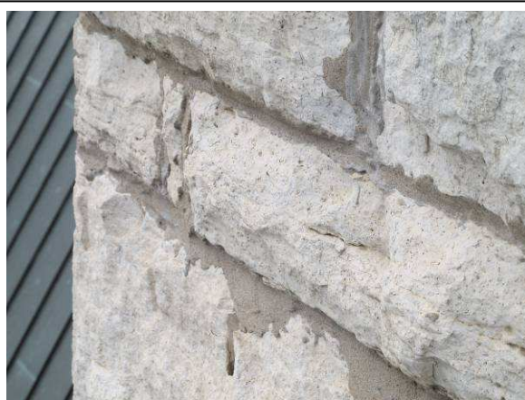
Poor mortar installation
