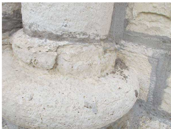
Deteriorating column base
