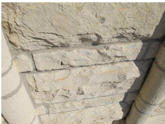
Deteriorated mortar and spalling stone
