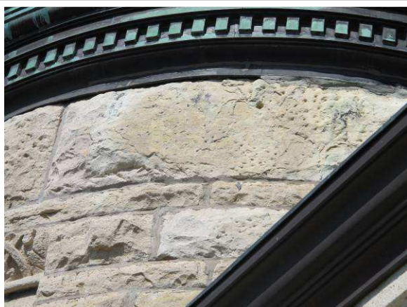
Loss of stone detail
