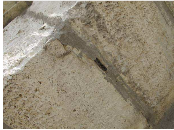
Open mortar joint
