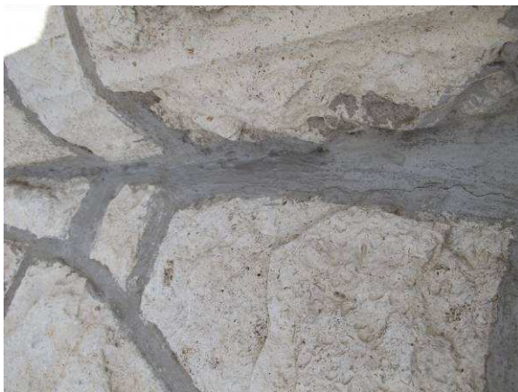
Poor mortar installation
