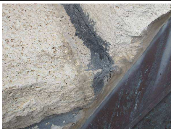
Failed caulking above flashing
