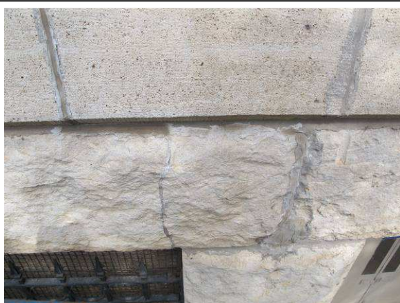
Cracked stone at window opening
