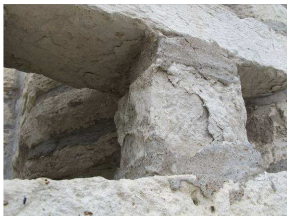
Deteriorated limestone at balcony
