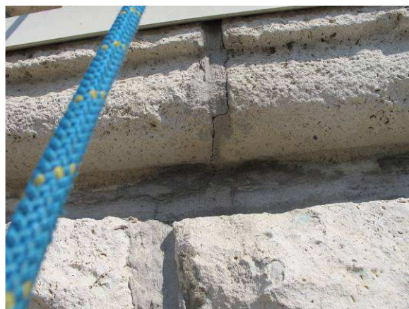
Mortar separation above arch
