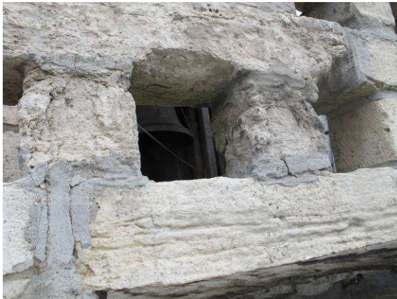
Deteriorating stone and poor mortar installation
