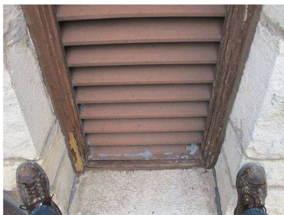
Deteriorating wood window and caulking
