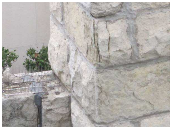
Close up of stone damage
