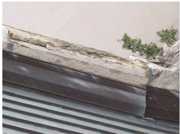
Close up of deteriorating stone
