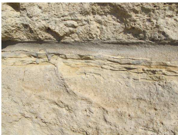
Delaminating naturally bedded stone
