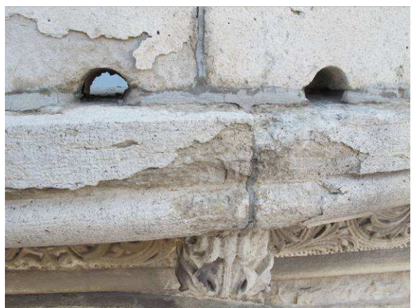
Deteriorated stone at balcony
