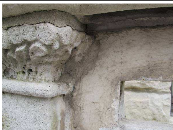
Poor mortar installation
