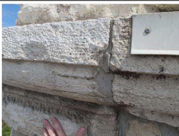
Deteriorated mortar joint
