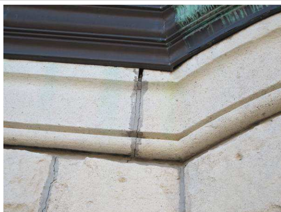
Failed mortar joint
