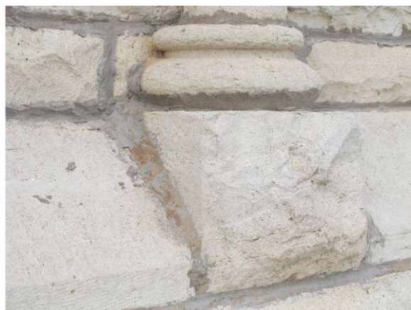
Failing mortar installation
