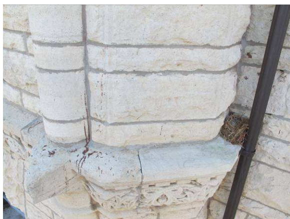
Spalling stone above entry
