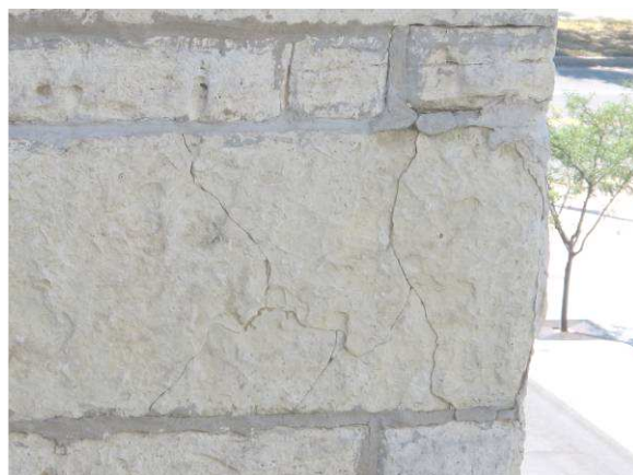
Close up of deteriorated stone
