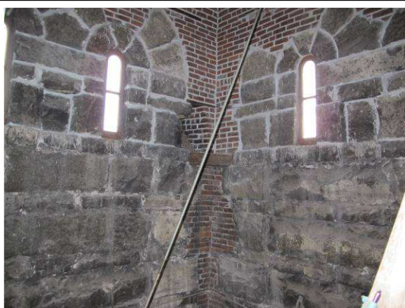
Mix of brick and stone evidence of smoke damage
