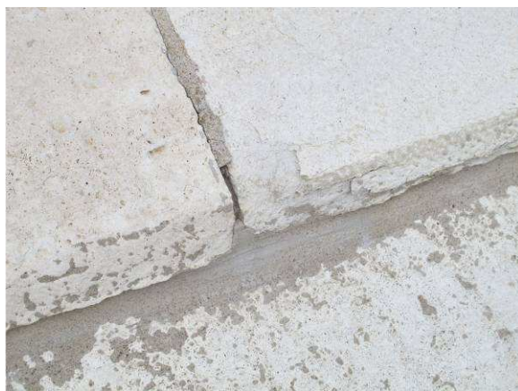
Missing mortar and stone
