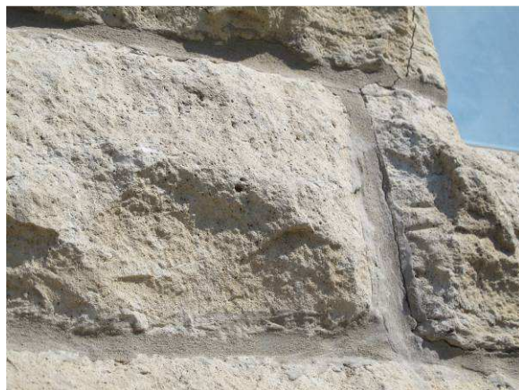
Debonded mortar joint
