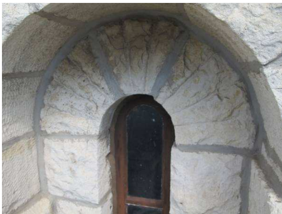
Poor mortar installation at arch
