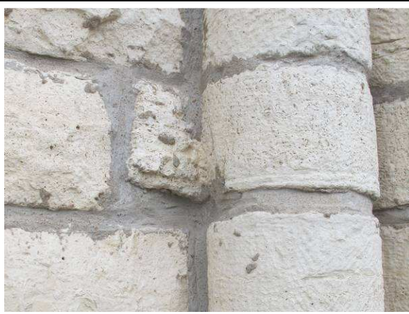
Poor mortar installation
