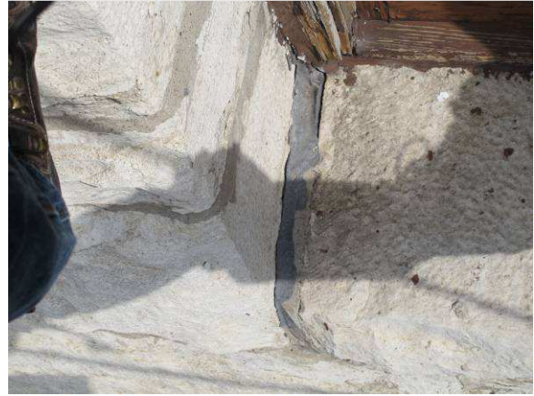
Separated caulk at window
