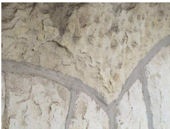
Deteriorating stone above arch
