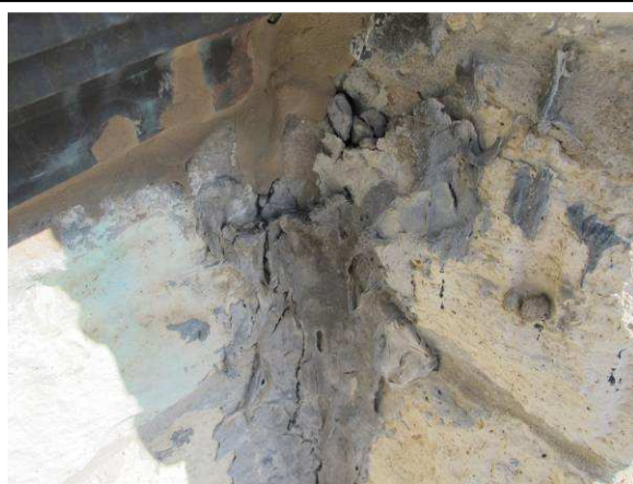
Failed caulking near flashing
