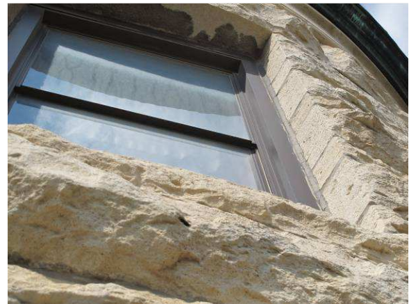
Water damage on underside of window header
