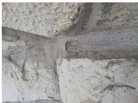
Failing mortar joint
