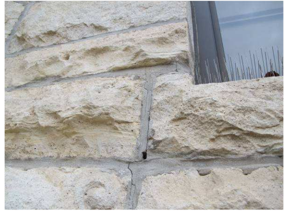
Missing, cracked and separated mortar
