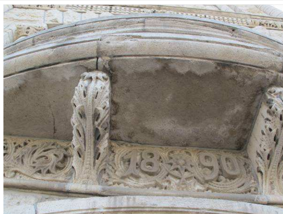
Failed joint and damaged stone above support
