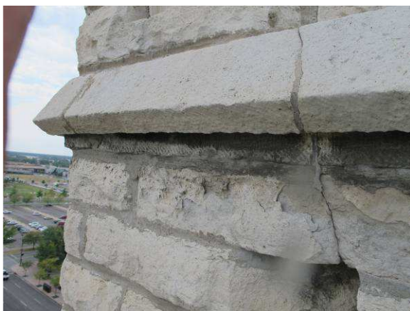
Vertical mortar separation and crack in stone
