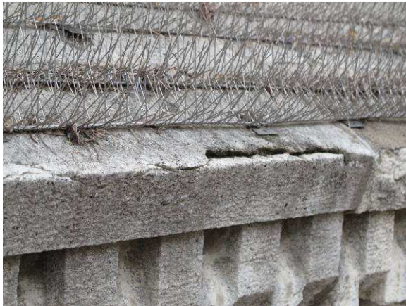
Spalled stone above dentil
