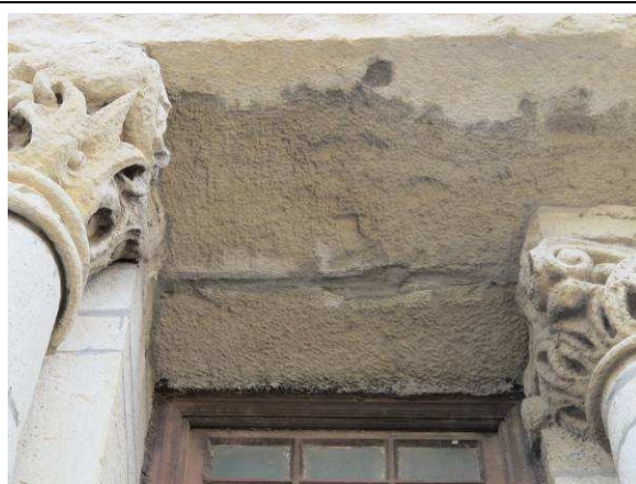
Deteriorating stone above columns
