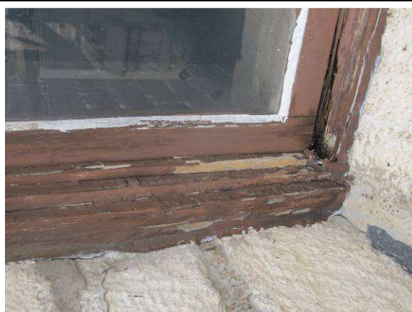
Deteriorating wood window and stone ledge
