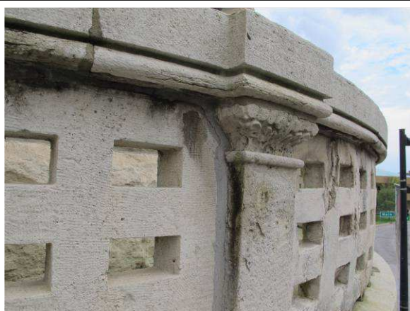
Deteriorating balcony stone
