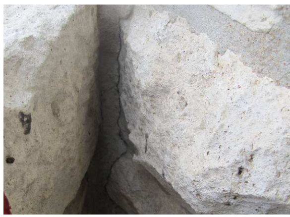
Separating mortar at corner of balcony
