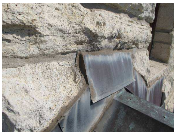
Questionable flashing detail
