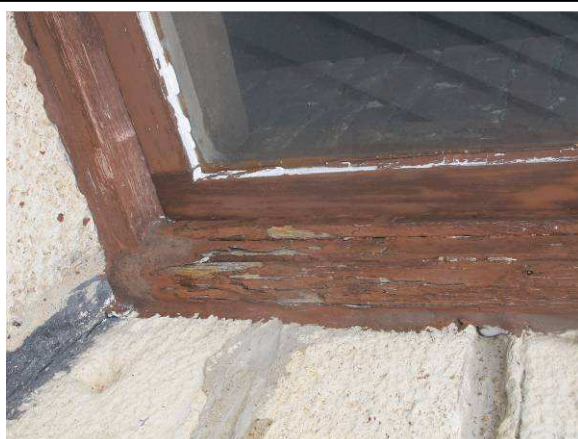
Deteriorating wood window and stone ledge
