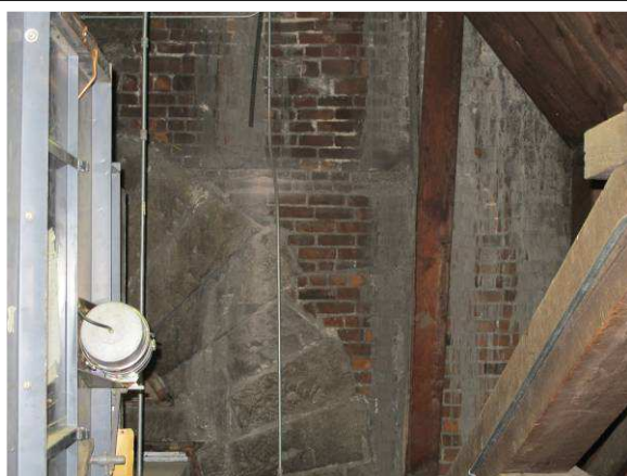
Smoke damage evident on stone
