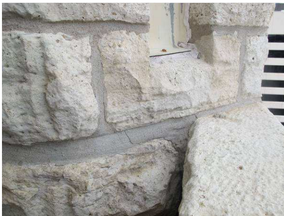
Vertical crack in mortar joints
