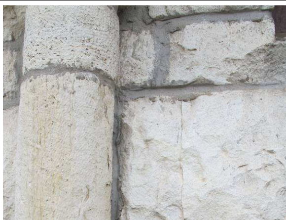
Poor mortar installation
