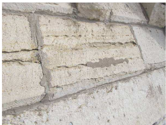
Failing stone and mortar below columns
