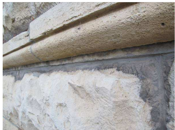
Poor mortar installation below spalled stone
