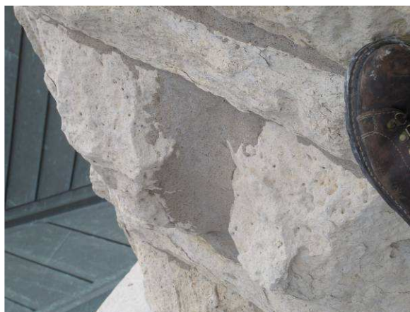
Poor stone patch
