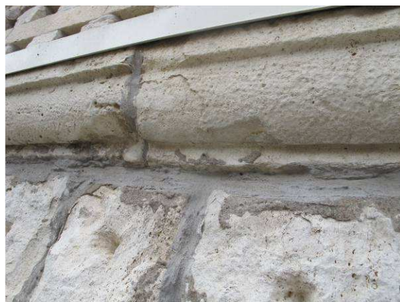
Poor mortar installation and exfoliating stone
