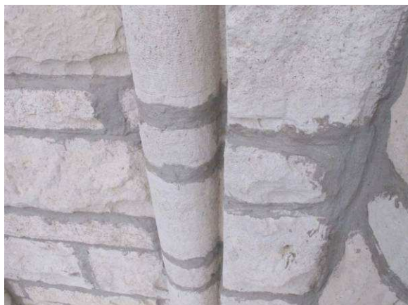
Poor mortar installation
