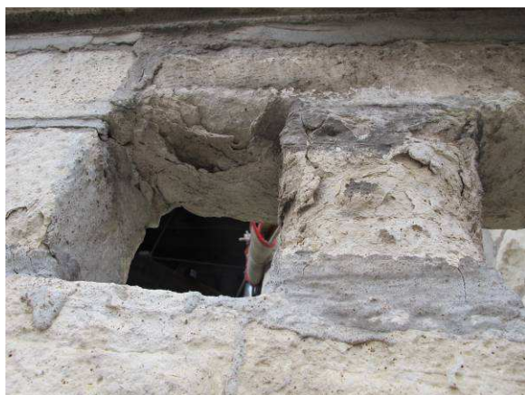
Deteriorated limestone at balcony
