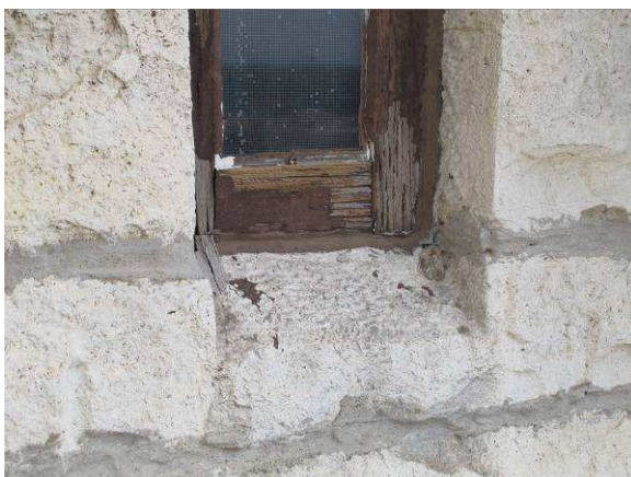
Deteriorating wooden window and ledge
