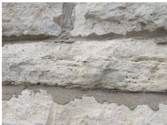
Poor mortar installation
