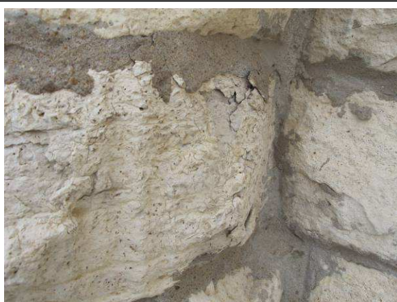
Poor mortar installation and deteriorating stone
