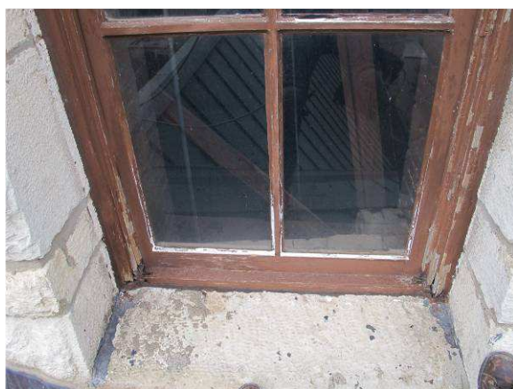
Decaying wood window
