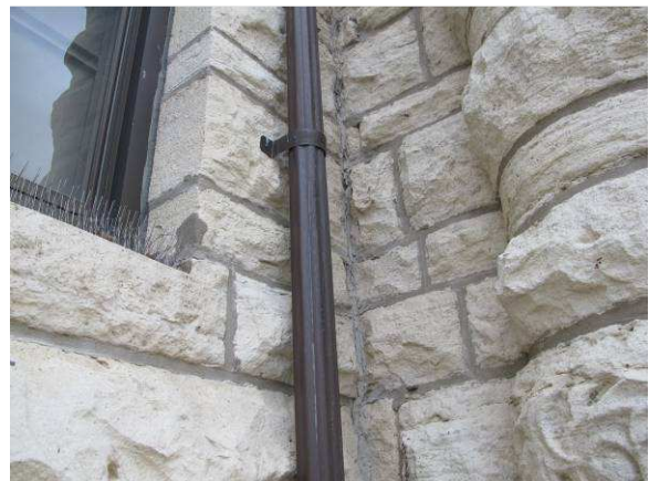
Poor mortar installation at return
