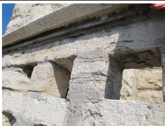
Poor quality repair at balcony rail
