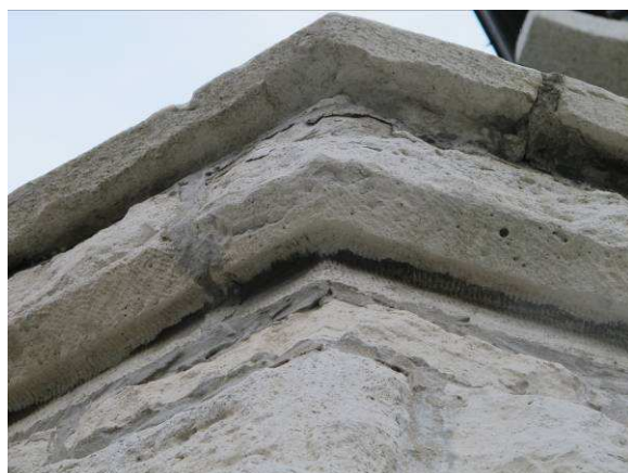
Poor mortar installation
