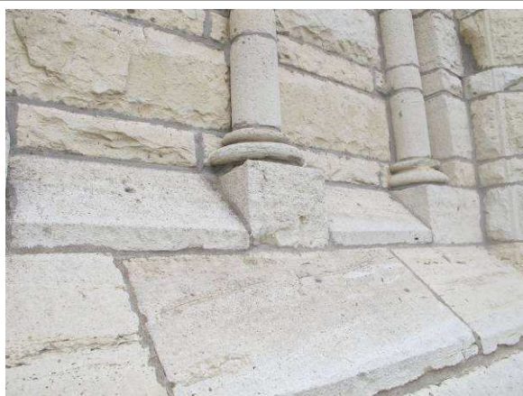
Deteriorating stone below columns
