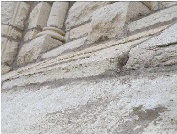
Failing mortar below columns
