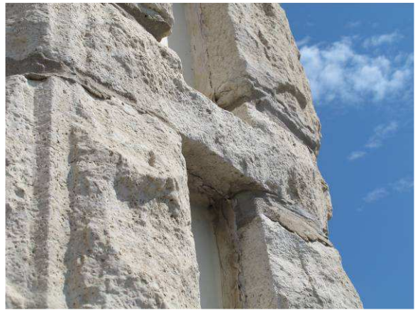
Spalling stone and poor mortar
