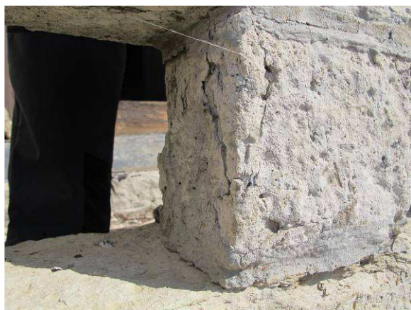
Deteriorating limestone at balcony rail
