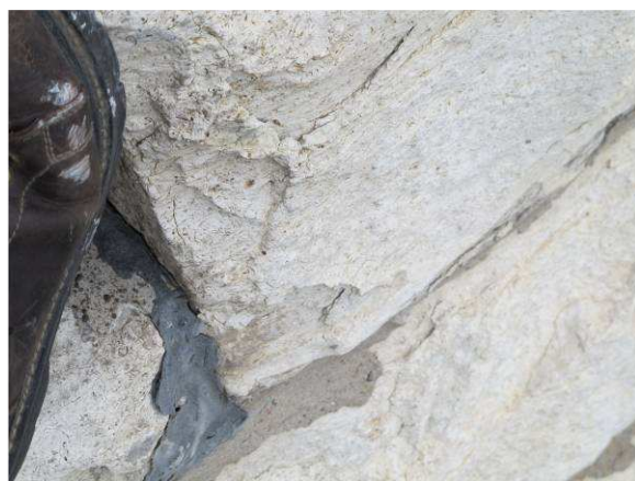
Deteriorated caulking and stone
