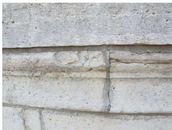
Separated joint and deteriorating mortar
