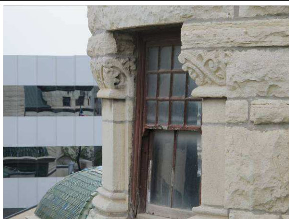
Deteriorating wood window
