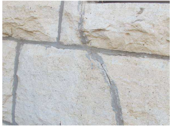
Failed repair of cracked stone
