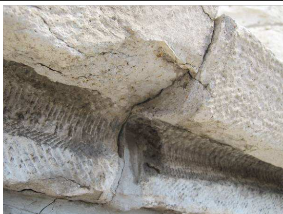
Mortar loss and stone deterioration
