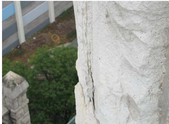
Spalling stone at NE corner of tower
