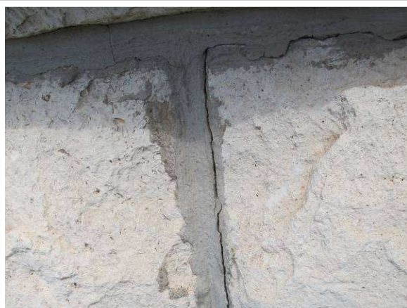
Separation at mortar joint
