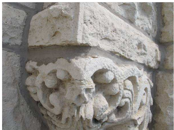
Poor mortar installation
