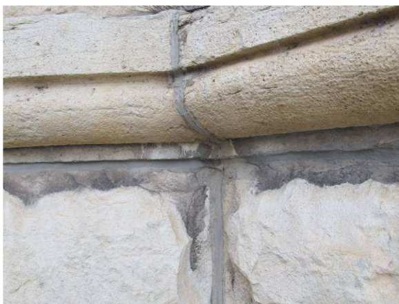
Poor mortar installation
