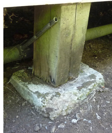
Deteriorated Post on Pad
