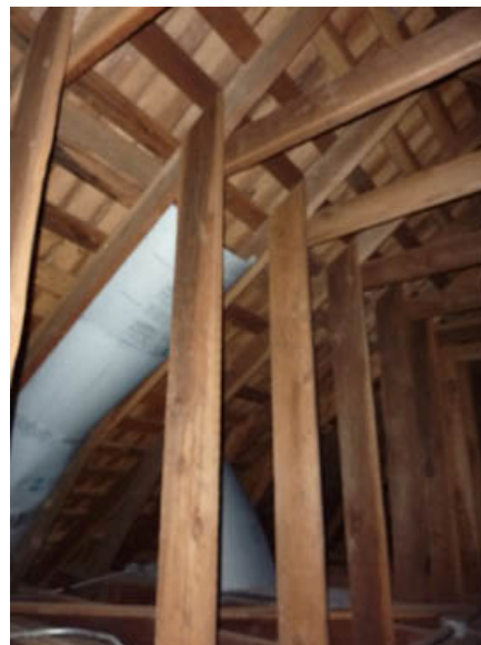
Attic Framing Over Hall Note Metal Drip Catcher
