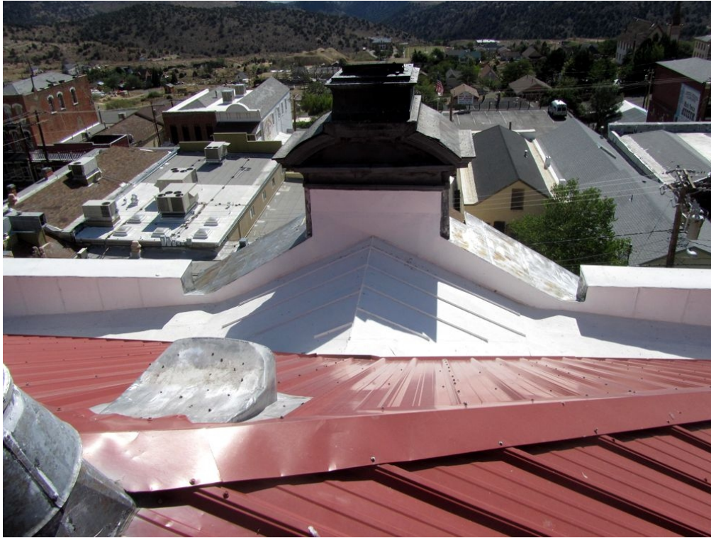
Photo 1. Back of tall parapet on the east side of the building. This requires bracing.
