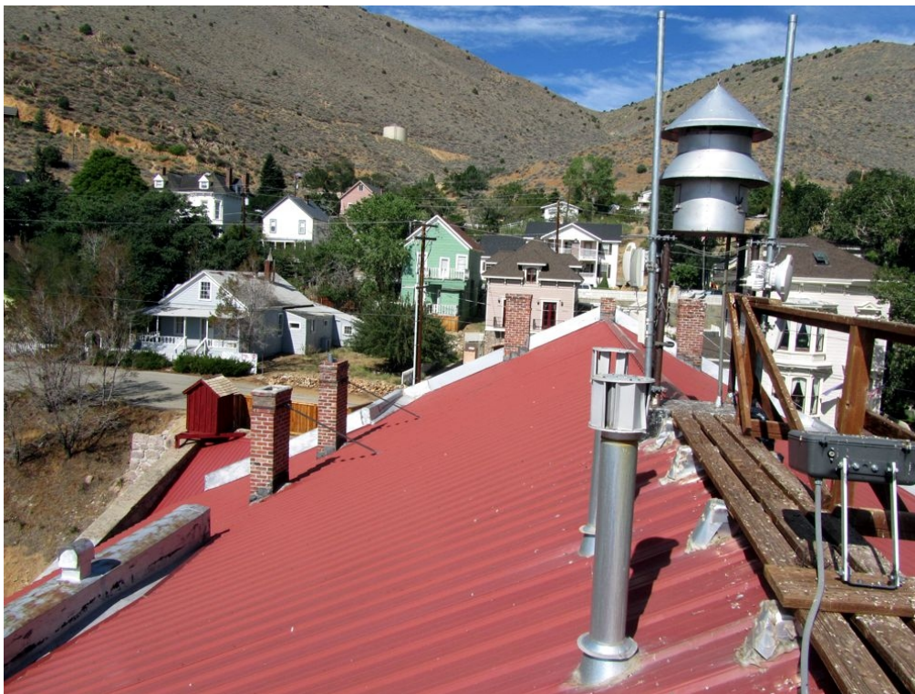
Photo 2. View west. Chimneys require additional bracing.
