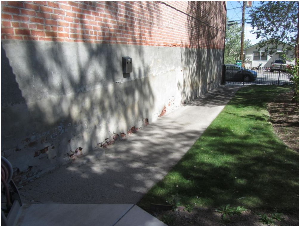
Photo 4. South wall. Brick deterioration at the base and at the top of the applied cement plaster. Repointing of brick joints and some brick replacement is needed.
