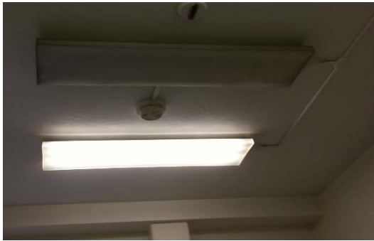
Figure 17: Typical dormitory lighting, originally one light was installed, but a surface raceway was used to install additional lighting in the space.
