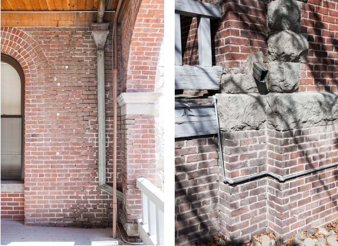
Figure 33: East wall of porch showing route of existing drainpipe, leader head and downspout. Note water damage to brick wall. Figure 34: Downspout outlet for the porch's east drainpipe. Image Source: IS Architecture, March 2015.
