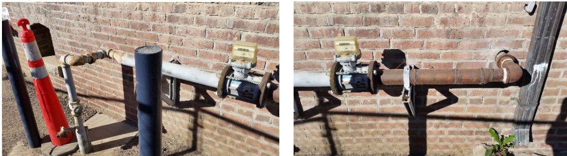
Figure 15: Natural Gas Piping – East Side of Building
