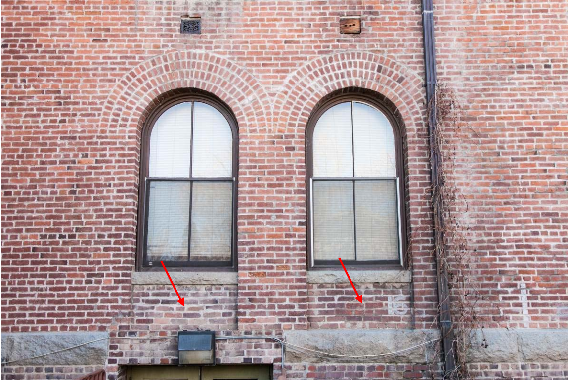
Figure 44: Overview of various condition issues related to the decorative grille vents on the north façade of Lincoln Hall. Upper left grille appears to be loose. The upper right grille is missing, but the opening is intact. Two decorative grille vent openings below the windows have been in-filled with brick. Image Source: IS Architecture, March 2015.
