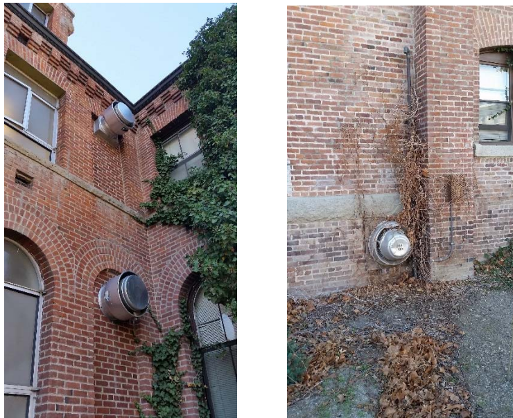
Figure 10: Restroom Exhaust Fans – North side of Building
