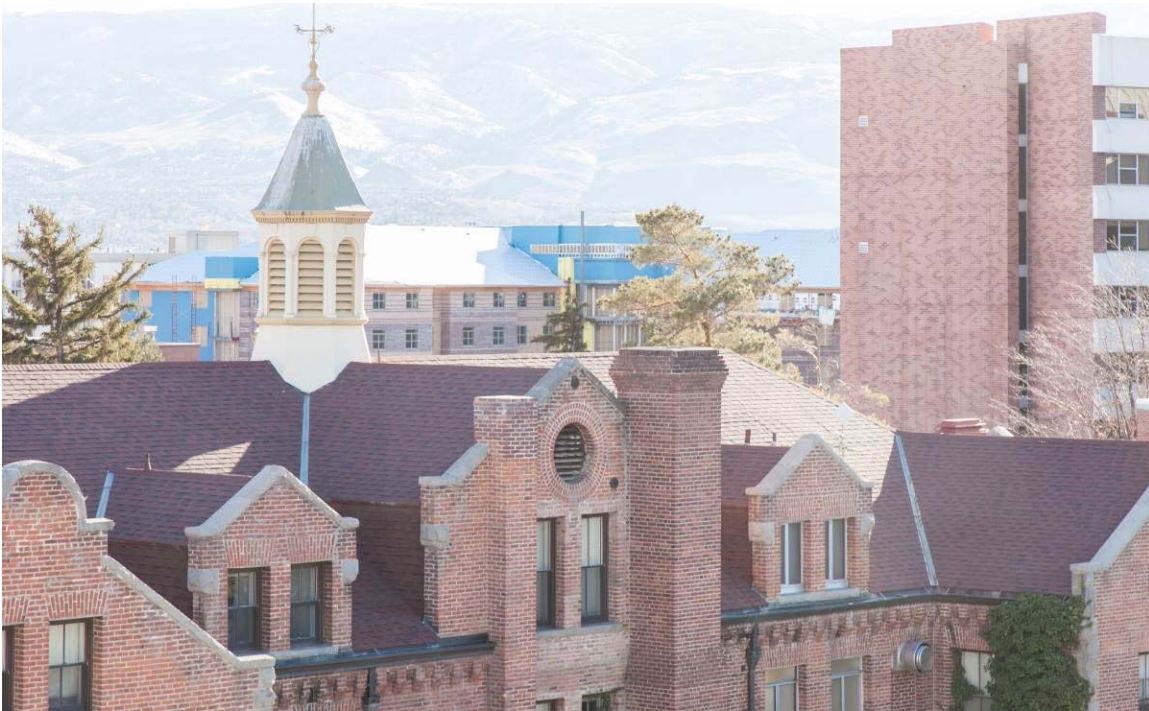
Figure 27: View southwest of roof. Note that valley flashing at right of frame appears to be rusting. Image Source: IS Architecture, March 2015.
