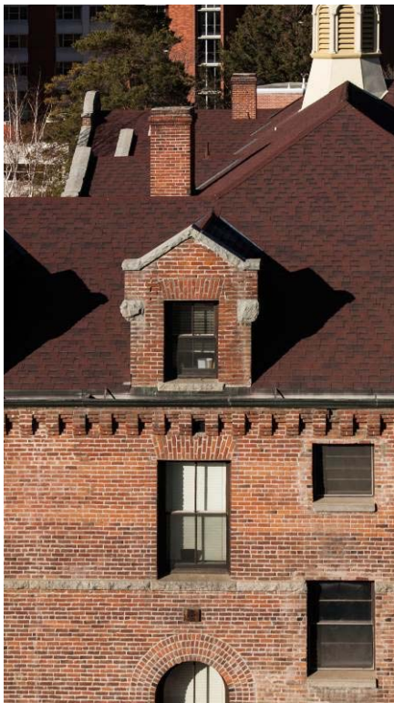
Figure 53: Detail view of east façade showing mortar loss at dormer. Image Source: IS Architecture, March 2015.
