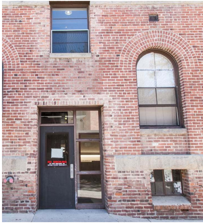
Figure 54: Detail view of west façade showing mortar loss at basement level. Image Source: IS Architecture, March 2015.
