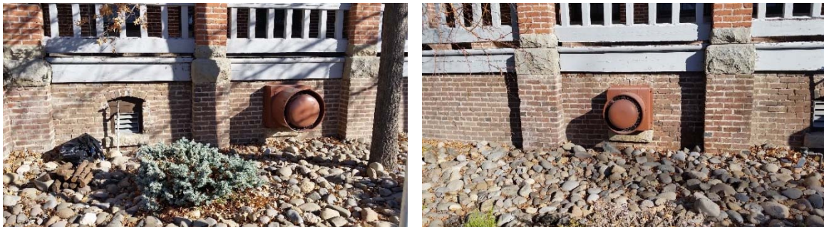
Figure 8: Basement Area General Exhaust Fans – South Side of Building.
