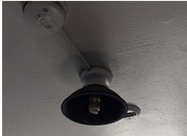
Figure 18: 3 rd floor dormitory surface mounted light fixture with modern CFL lamp. Surface raceway used to service fire alarm device.
