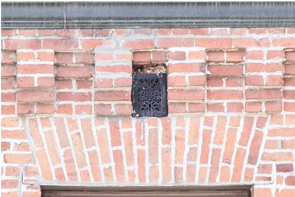
Figure 72: Detail view of decorative grille vent opening on west facade. The grille has become loose and wildlife appears to be nesting in the wall cavity. Image Source: IS Architecture, March 2015.
