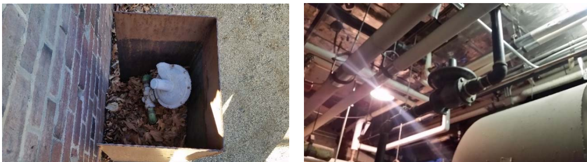
Figure 16: Natural Gas Piping – Generator and Boiler Room
