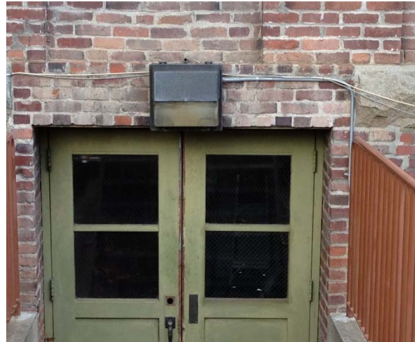
Figure 20: Typical building mounted exterior light with surface mounted raceway shown on the right side of the fixture.
