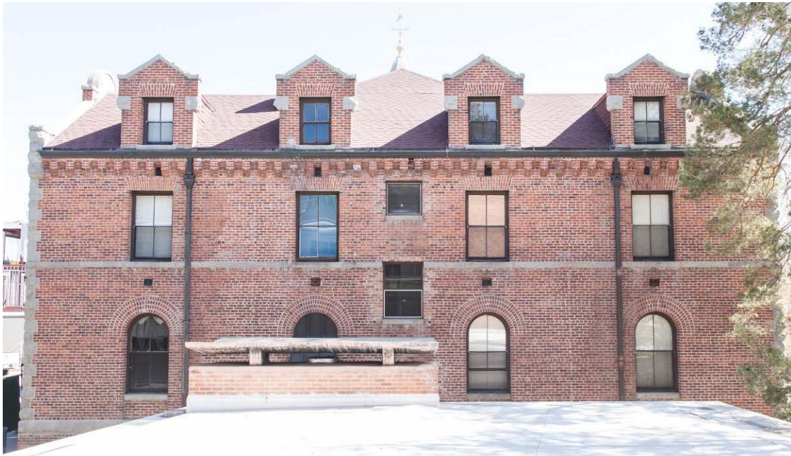
Figure 65: View east of west facade. Note the detracting blue material hung in the windows. Image Source: IS Architecture, March 2015.
