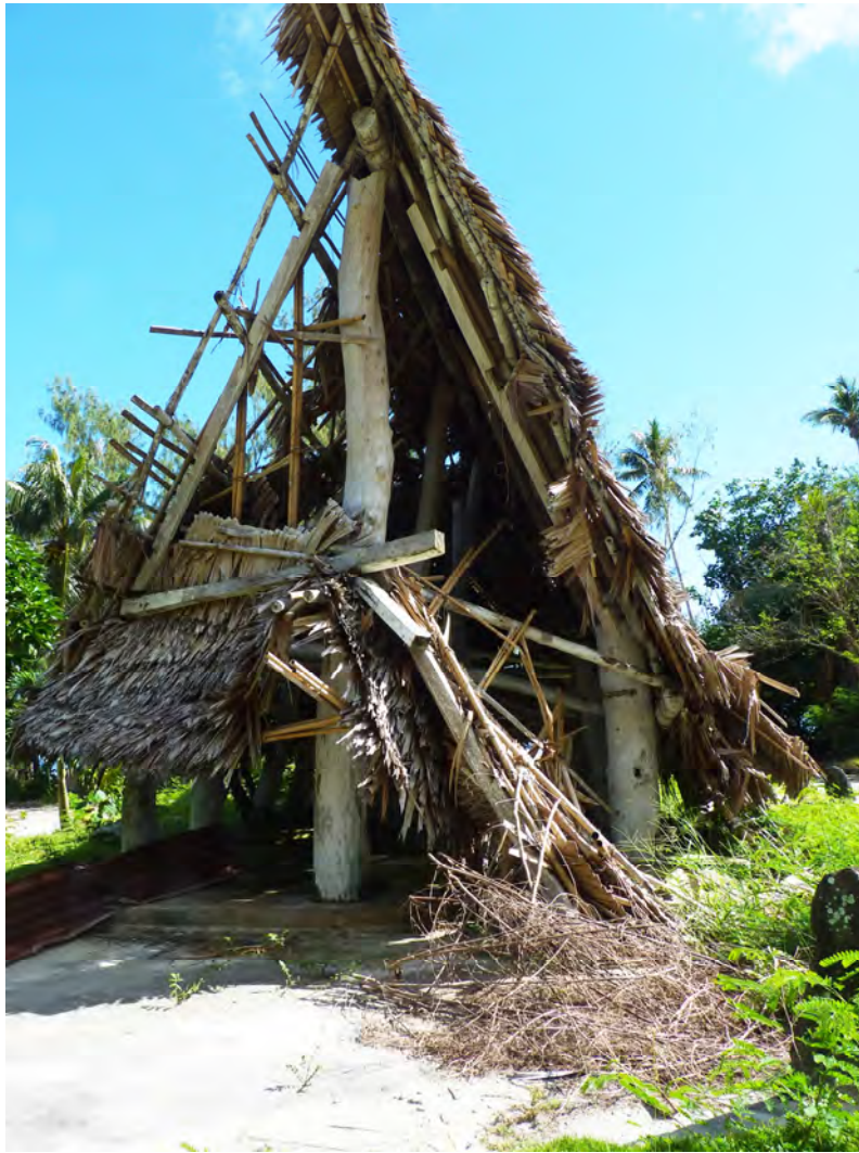
Photo 2. Extreme storm damage to Fitesuwa Men's House in Anoth Village, Gilman Municipality.
