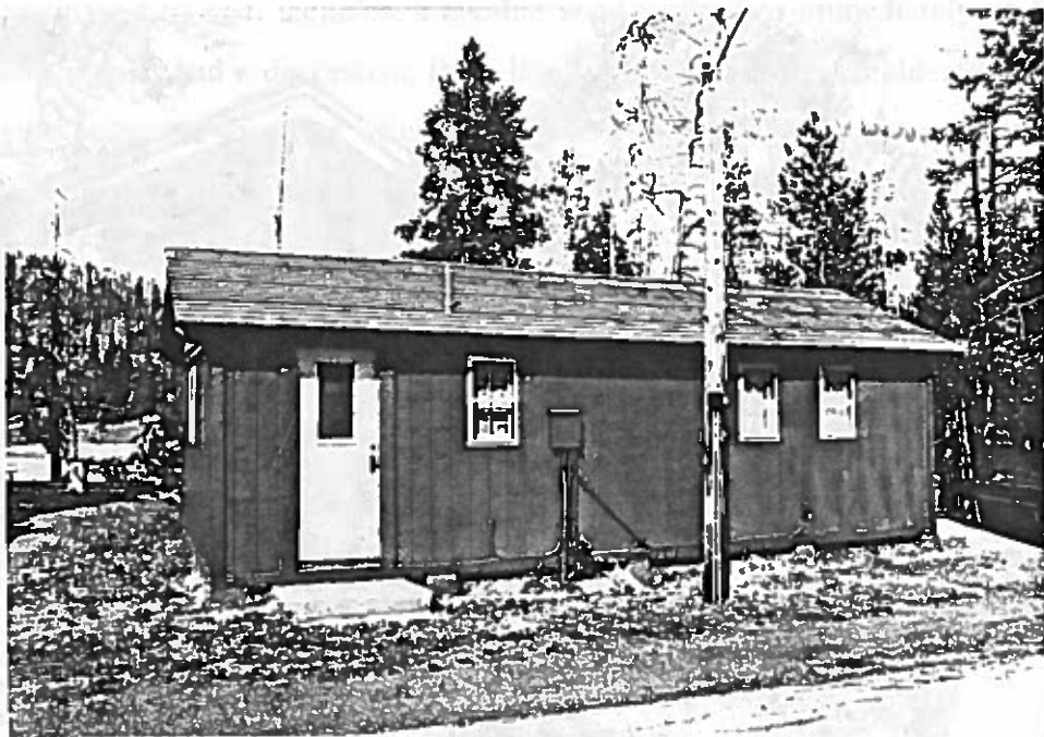
Figure 188: Looking north at a managers cabin. The texture 111 plywood paneling is starting to come apart (possible delamination) on the corners.
