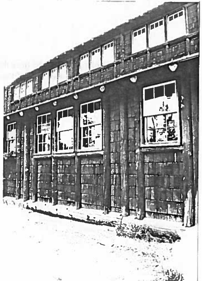
Figure 82: Looking west at a typical section of log-out wall on the east side of the Rec Hall. Note the weathered base log and sills and sash of the windows. Also the grade at this point allows water to flow under the building.
