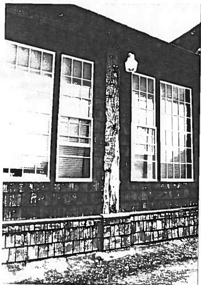
Figure 42: Looking east at one of the log columns on the west side of the Lodge. Note the missing bark at the base. Water from the roof runs down on the light fixture and back into the bark on the log. Water running down to the base is rotting the bark and base of the log.
