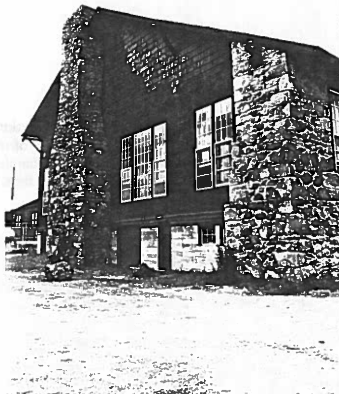
Figure 61: Looking southeast at the north end of the Lodge building. Note the shingles that were replaced and never stained to match. The top of the chimney has separated from the roof leaving an opening at the top. Water pours down into the interior.
