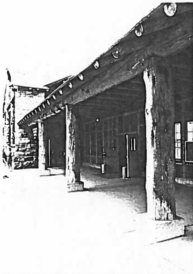
Figure 109: Looking northeast at the covered walkway on the west side of the building. Note the weathered and rotted areas on the base of the columns.
