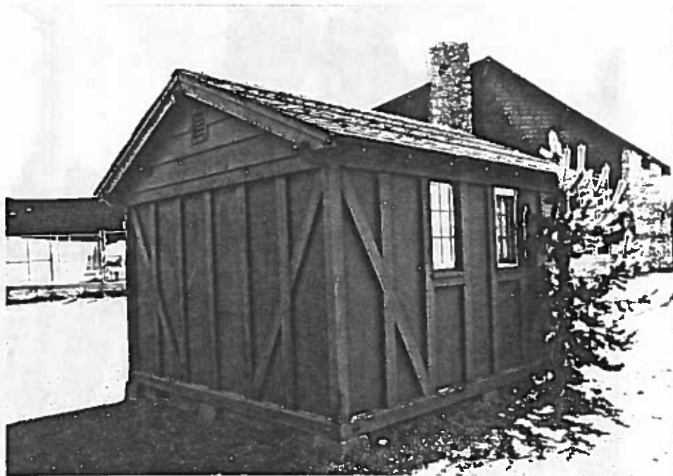
Figure 163: Looking south at a typical frame-out single cabin (#114). There is a missing screen on one of the windows and there is some weathering in the sill plate.
