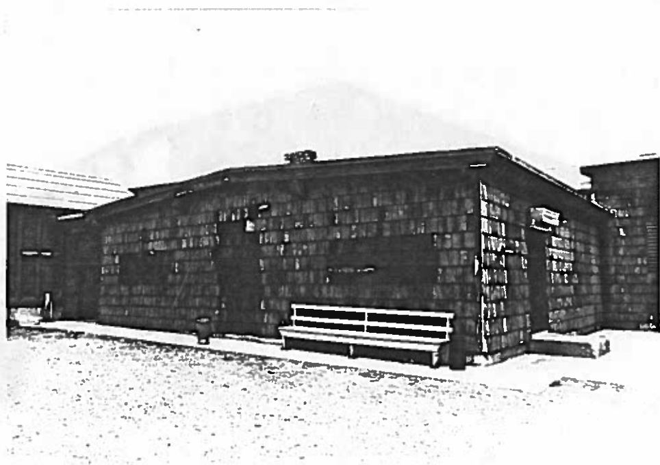
Figure 72: Looking west at another infill building with infilled windows. Note the different stains.
