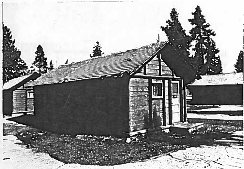
Figure 181: Looking southeast at a typical log-out duplex cabin (#238-239). Note the broken roof shingles and deteriorated ridge board.
