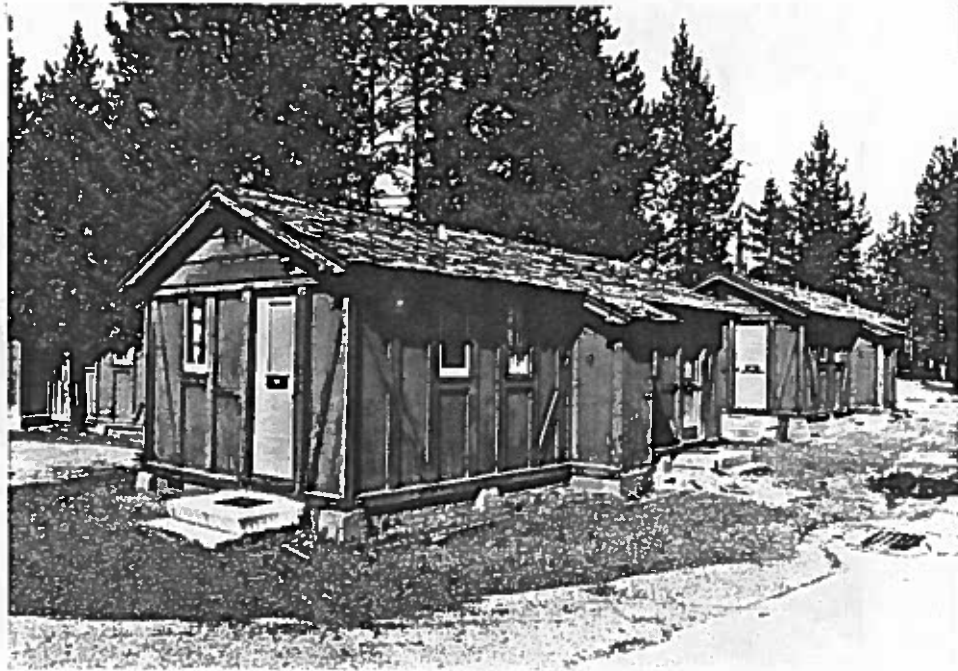
Figure 164: Looking northeast at a typical frame-out duplex cabin (#161-162). The roof is very poor on this cabin which is typical of about 60% of the cabins. Note the added bathroom.
