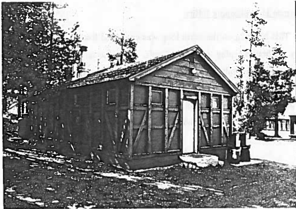
Figure 219: Looking northwest at the lower loop restroom/shower building. The building is in good condition with the exception of the concrete stoop which is deteriorating badly.
