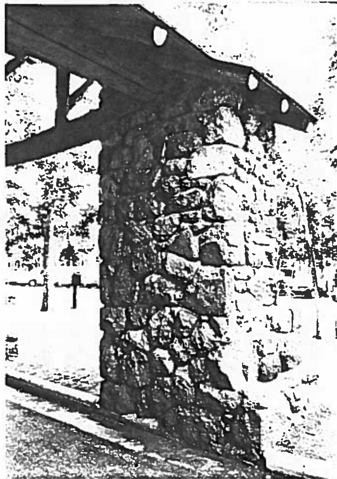
Figure 107: Looking southeast at a stone pier on the porte-cochere. There is minor mortar loss on base of the pier.
