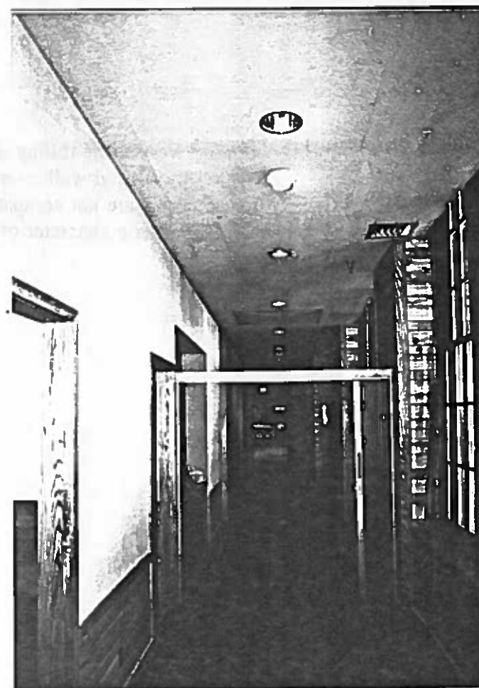
Figure 134: Looking south at the hallway along the west side of the building. Note the incompatible materials, especially the vinyl wall covering, doors and lighting fixtures.
