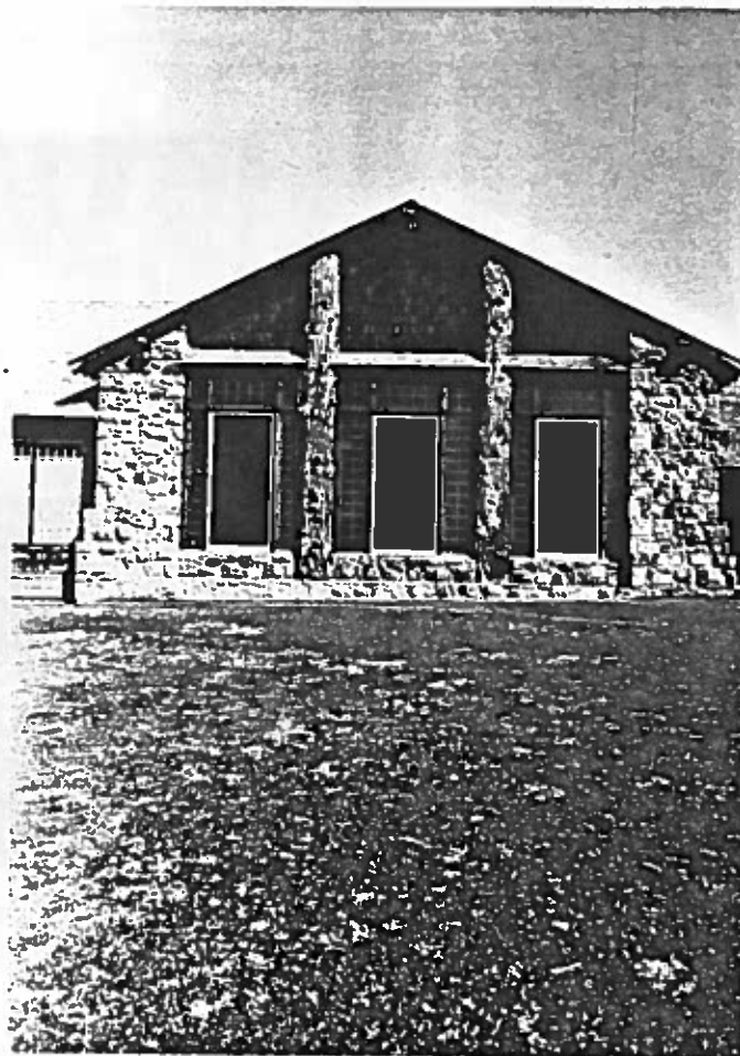
Figure 35: Looking east at the main windows in Old Faithful Lodge. The extended purlins have rotted on top and have been covered with a galvanized metal. The bark is loose on the log columns and has come off in some areas.
