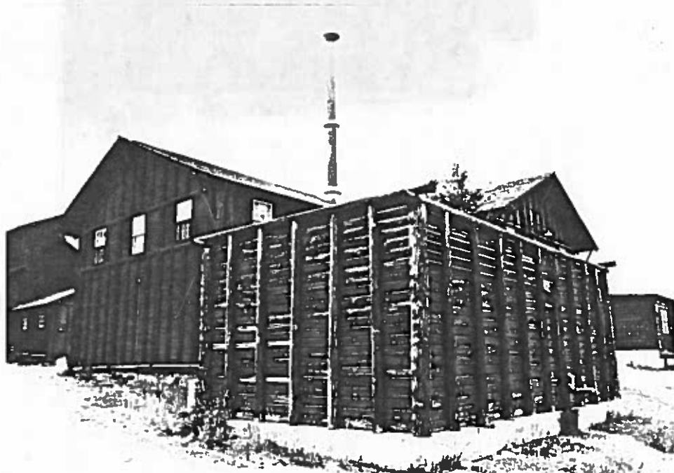
Figure 210: Looking southwest at the fuel tank enclosure at the Boiler Plant building. Note the weathered and deteriorating wood on the structure.
