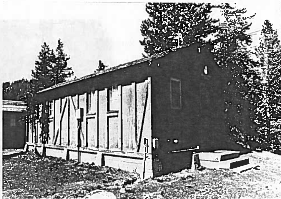
Figure 221: Looking north at the upper loop housekeeping building. The wood walls and details are weathered and dry.
