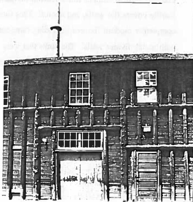
Figure 204: Looking north at the entries on the Boiler Plant building. Note the weathered wood and delamination of the plywood.
