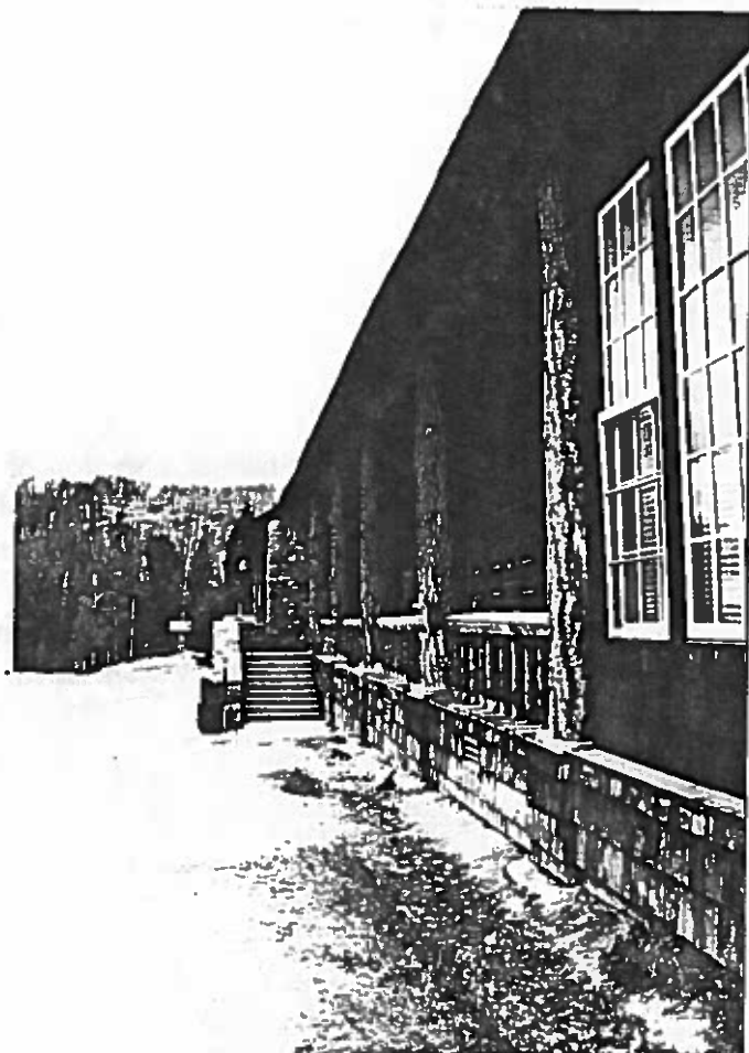
Figure 43: Looking northeast at the porch area on the west side of the Lodge. Note the weathered shingles at the base and the ditch that has been created close to the building because of roof water runoff.
