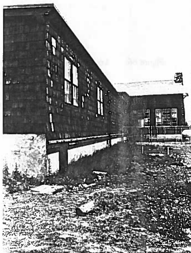
Figure 68: Looking west along the north wall of the kitchen/EDR section of the Lodge. Note the weathered wood.
