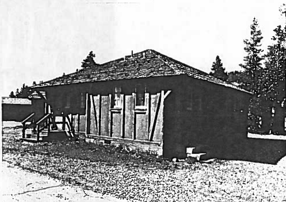
Figure 167: Looking northwest at a typical frame-out quad cabin (#110-113). Note the use of concrete and wood frame for the stoops. The roof on this structure has some bad areas.
