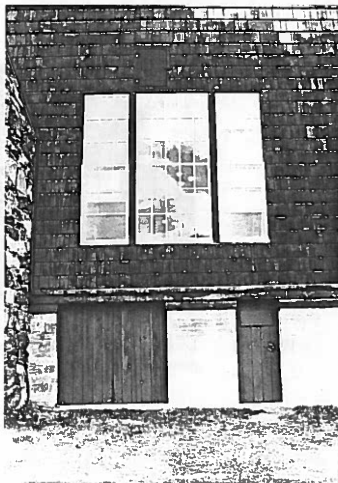
Figure 62: Looking south at the wall with a concrete base and framed wall above with shingles. Note the weathered wood and stain loss on the shingles.
