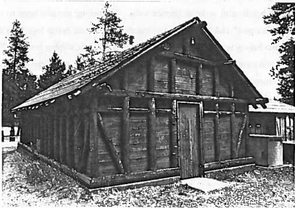
Figure 214: Looking northeast at the upper loop linen building. Note the rotted purlin tips. Also, there are some minor problems with the wood shingle roof.
