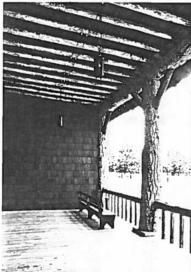
Figure 53: Looking southwest at the open porch log columns and rail. Most of the logwork is in good condition with the exception of the outer bases and railing.
