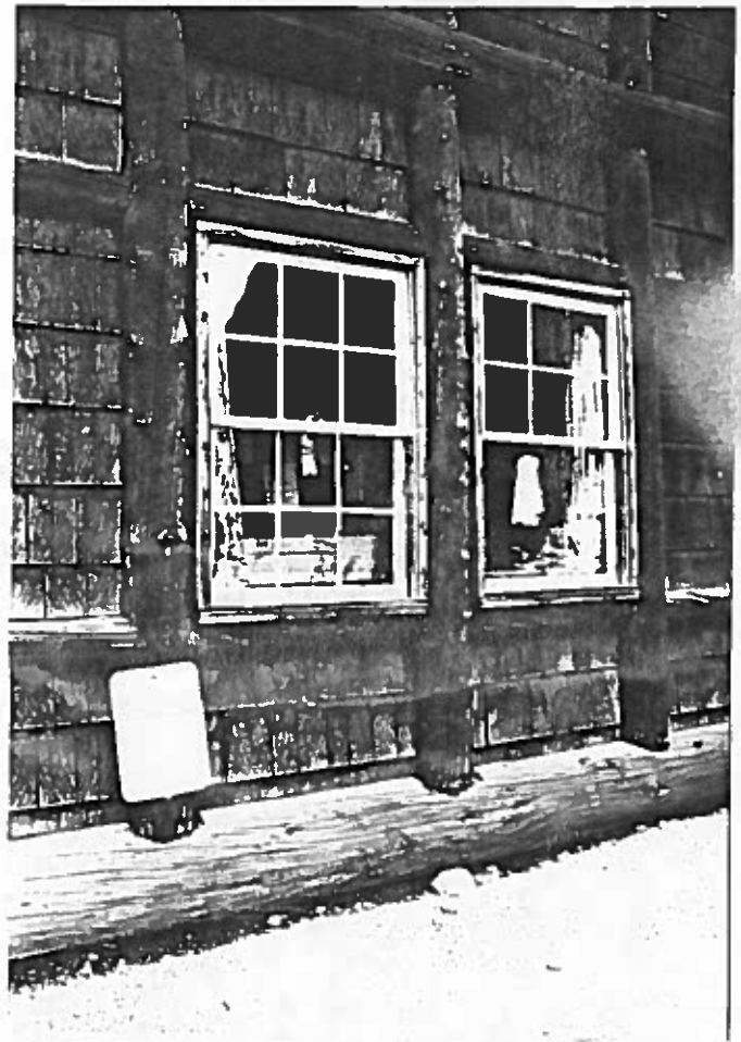
Figure 97: Looking north at the windows on the south wall of the Rec Hall. The windows are in very poor condition with rotted sash and sills, and wood trim.
