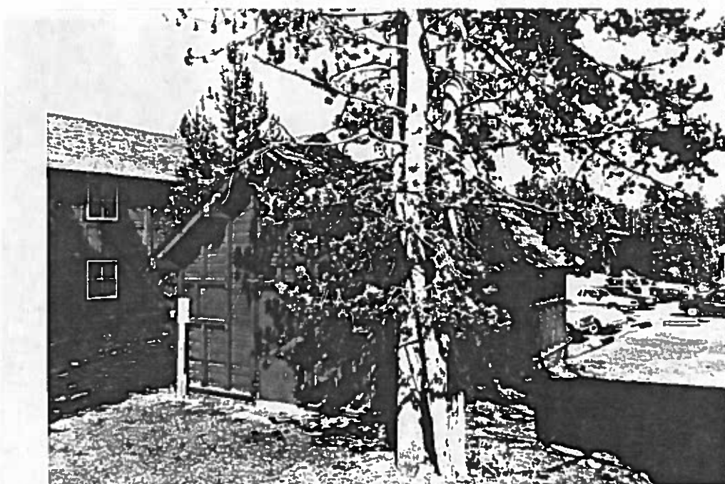
Figure 223: Looking east at the winter storage building. There are some rotted base timbers and the grade around especially the west end is poor.
