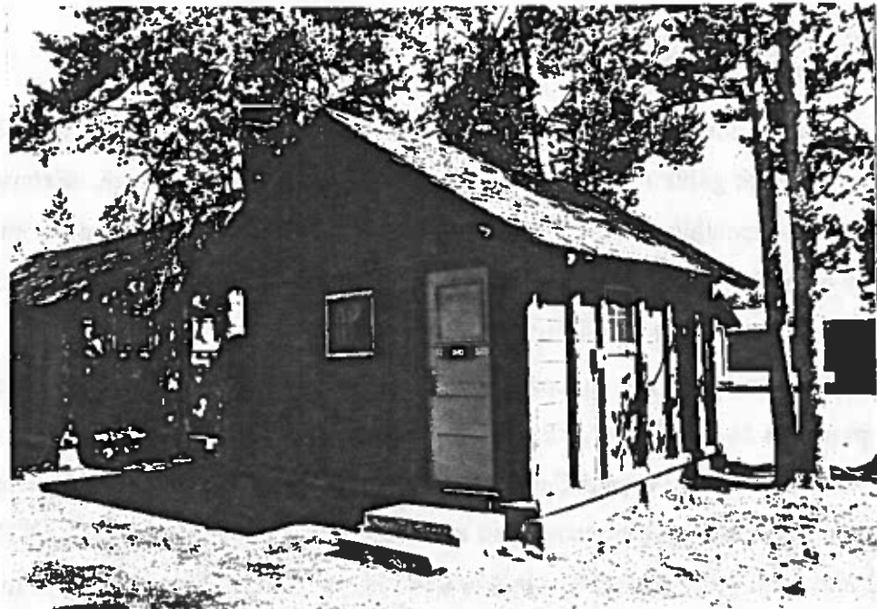
Figure 178: Looking southeast at a typical log-out single cabin (#240). Note the deteriorating wood shingle roof and the poor concrete stoop. The sill log has some rot.
