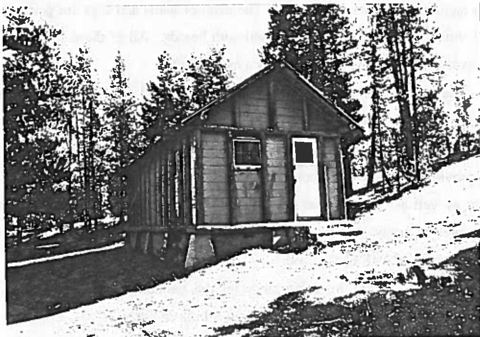
Figure 179: Looking south at a typical log-out duplex cabin (#230-231). Note the different painted boards. The roof is deteriorating and the concrete steps are in poor condition.
