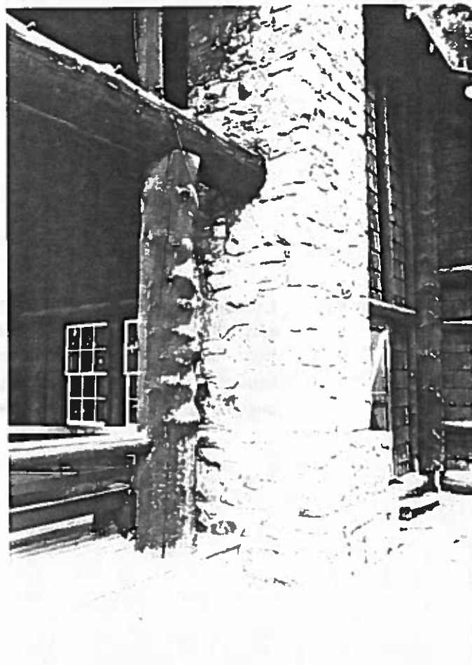
Figure 89: Looking northwest at a stone column detail on the south porch. Note the weathered base around the column and on the flooring.
