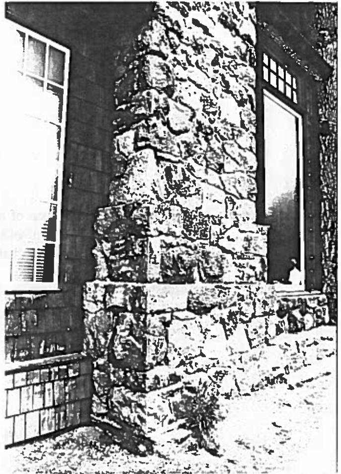
Figure 39: Looking southeast at a detail of the stonework by the main windows. Water flows into this corner of the building due to the ground not sloping away from the building.
