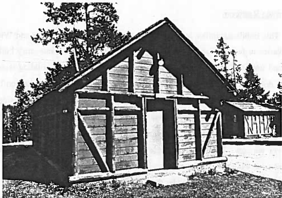
Figure 217: Looking west at the upper loop restroom/shower building. Note some sill log and purlin tip rot.
