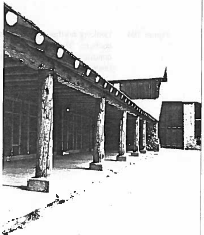
Figure 102: Looking north at one of the columns on the south side of the Lodge. The columns are weathered and there is some rot at the base. The concrete piers are also, breaking up.
