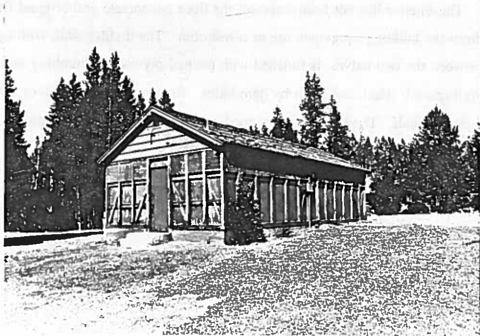
Figure 212: Looking northeast at the lower loop linen building. This frame-out building has a poor roof and there is deteriorated wood on the walls and frame. The concrete stoop is also, in poor condition.
