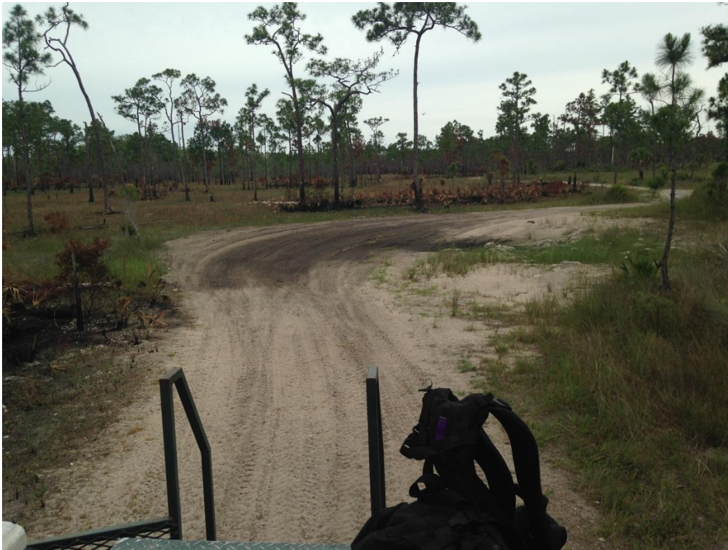
Buckskin Trail, material is bermed up and rutting has occurred
