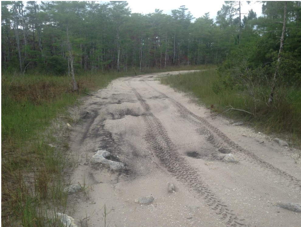
Monument Bypass Trail, widening of the trail tread and displacement of wet soils
