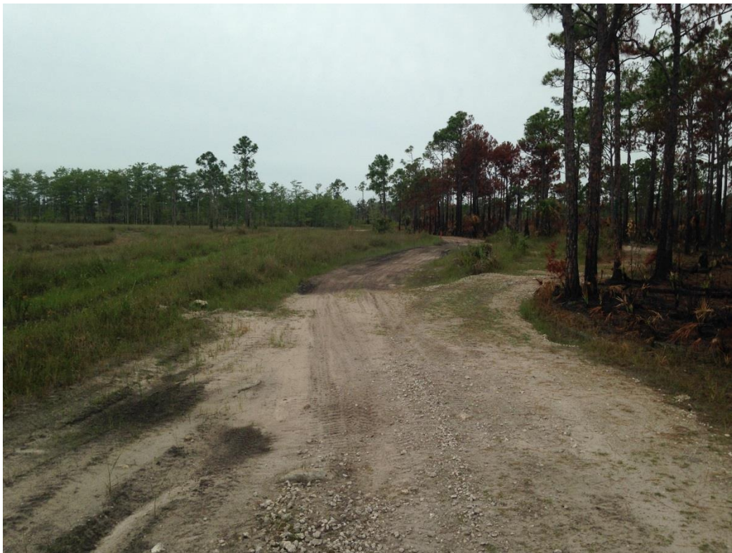
Buckskin Trail, evidence of recent maintenance and heavy traffic cutting turn, material being displaced.
