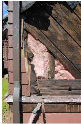
Hole in the west corner of the wall.
