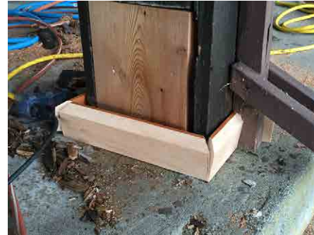
Section of column that was replaced due to rot.
