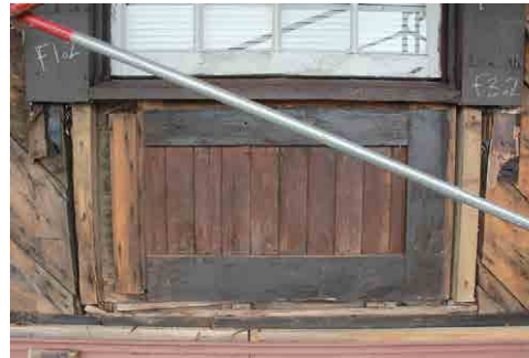
Panel that was hidden under Window F that is missing a board.
