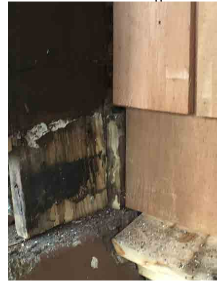
Rotten piece of porch column that will be replaced.
