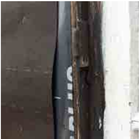
REMOVED WINDOW HINGES
