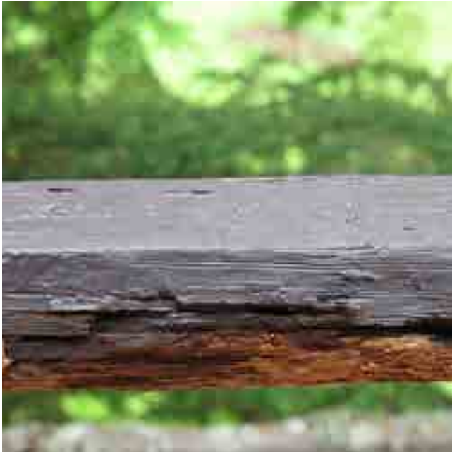
ROT DAMAGE ON WOOD TRIM
