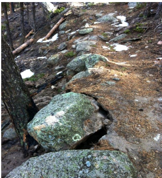
Photo 2 - Damaged Rock Wall FR-25
