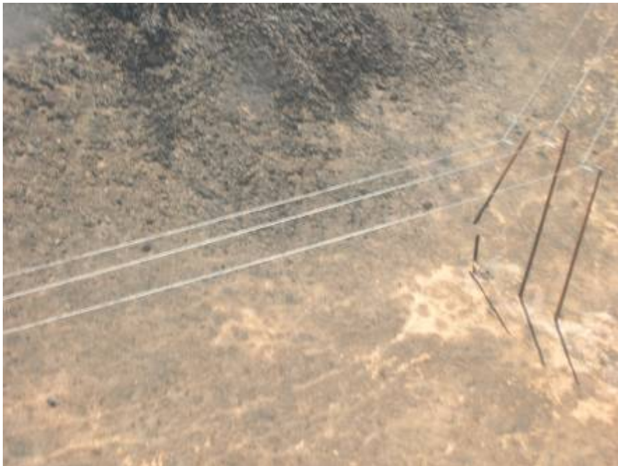
Burned utility pole above Coalpits Wash
