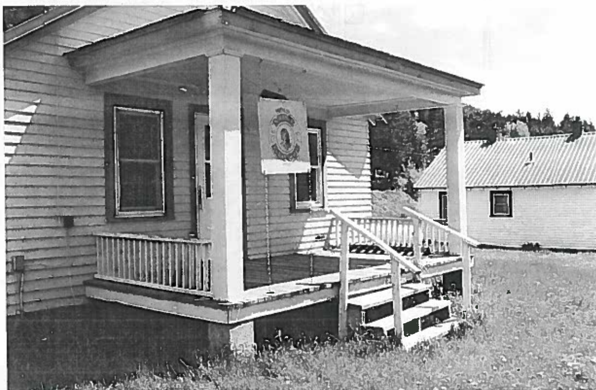
Figure 236: Looking southeast at the front porch. The porch deck has some floor deterioration but is generally in good condition.
