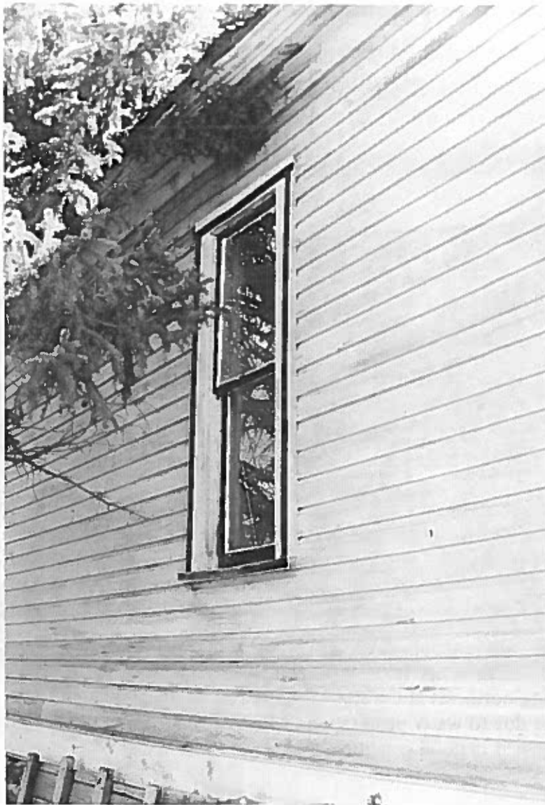
Figure 47: Looking northeast at a typical wood double-hung window on the house. Note the weathered sill, trim and wall siding.
