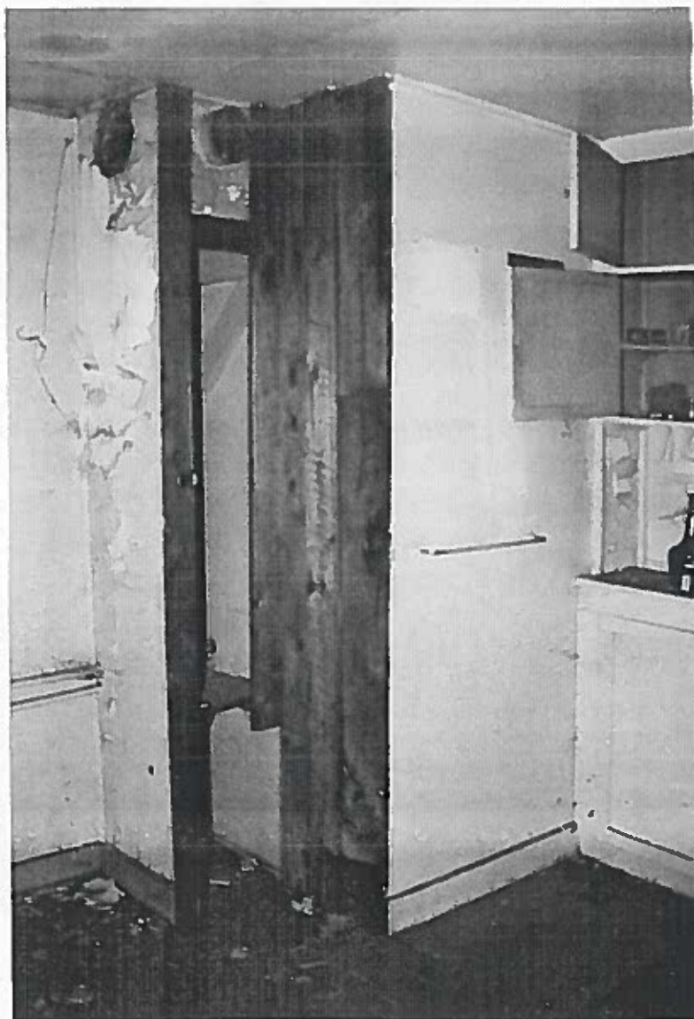
Figure 171: Looking southwest at the chimney area of the kitchen. There has been some water damage around the chimney.
