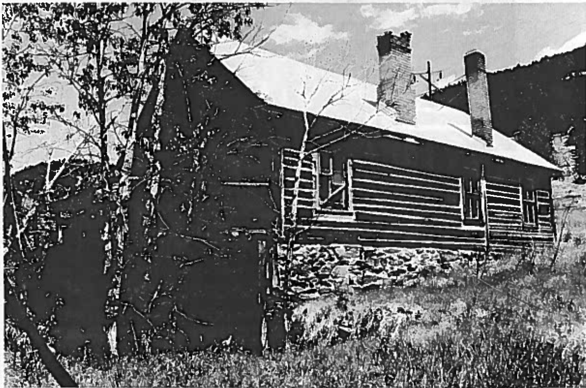
Figure 121: Looking northeast at the house. The sloped grade at this end of the house has been dug out to allow a vehicle to access the area under the deck. However this has also caused the foundation to be undermined on this end of the building where there are some settlement cracks.
