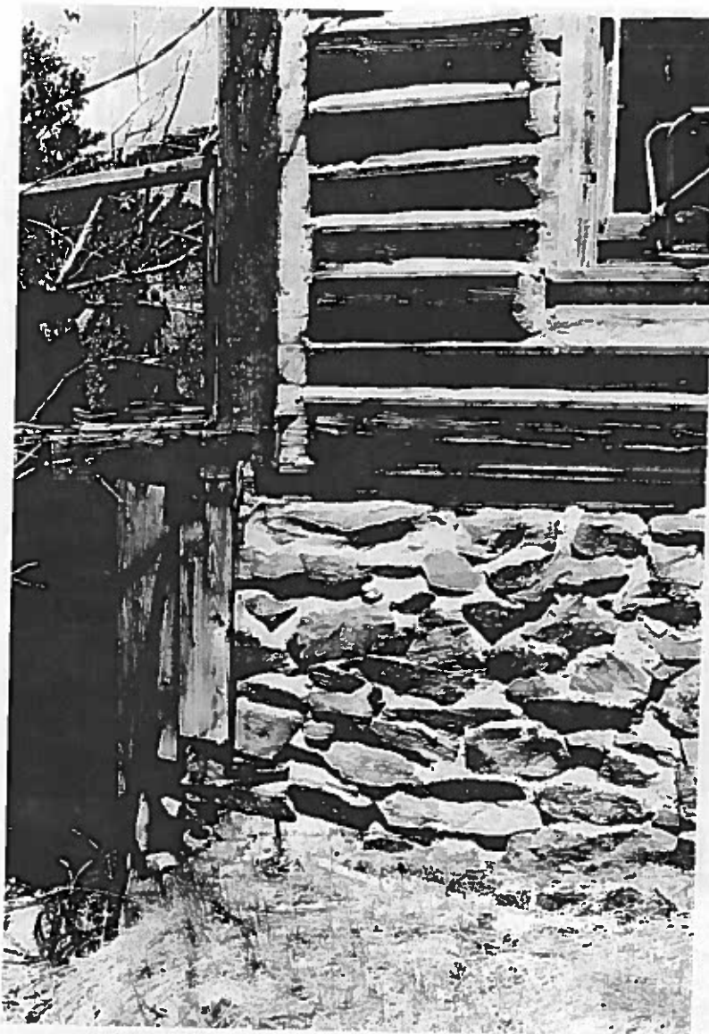
Figure 122: Looking north at a corner of the stone foundation where there is some settlement cracks.
