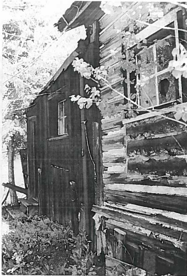
Figure 158: Looking northeast along the back of the building at the original log portion and the added frame buildings. The frame portion is in poor condition with rot at the base as well in the roof structure.
