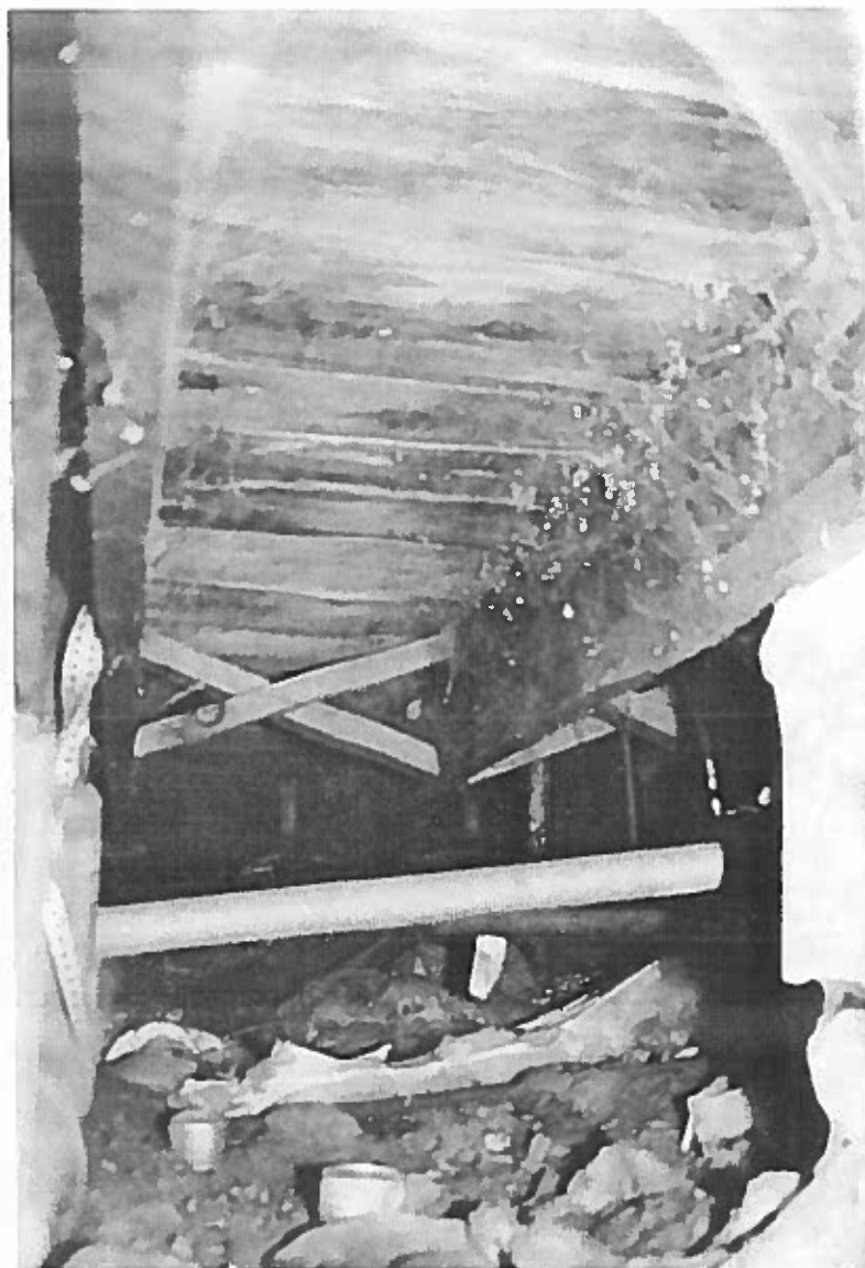
Figure 50: Looking east at the crawl space under the building. The floor joists and floor sheathing are in good condition with some minor dry rot but in most cases the materials are dry.
