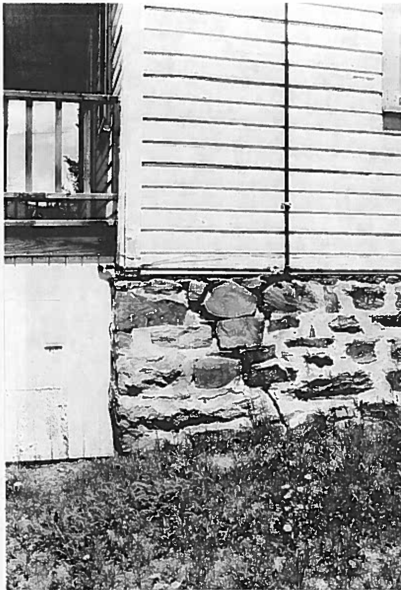
Figure 84: Looking northeast at the base foundation at the front of the building. There is some settlement in the foundation where it is cracked caused by water undermining the front of the building under the porch.
