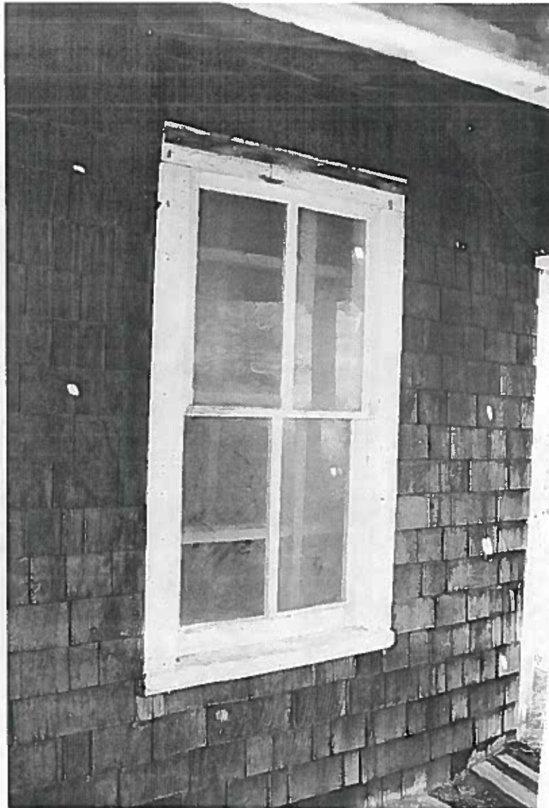
Figure 193: Looking northwest at a typical wood double-hung window under the porch. Note the weathered sill and missing glazing putty around the glass.
