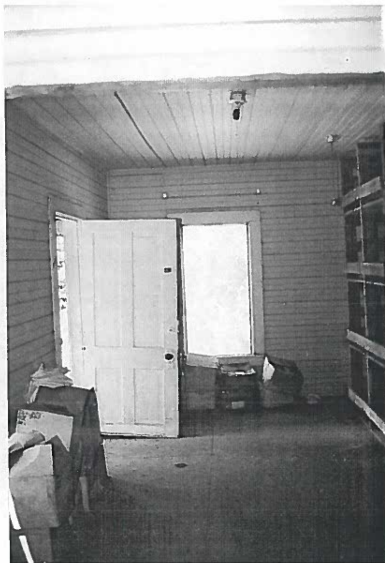
Figure 224: Looking west at the interior of the frame addition. The original floor has rotted out and is covered with a plywood sub-floor and frame.
