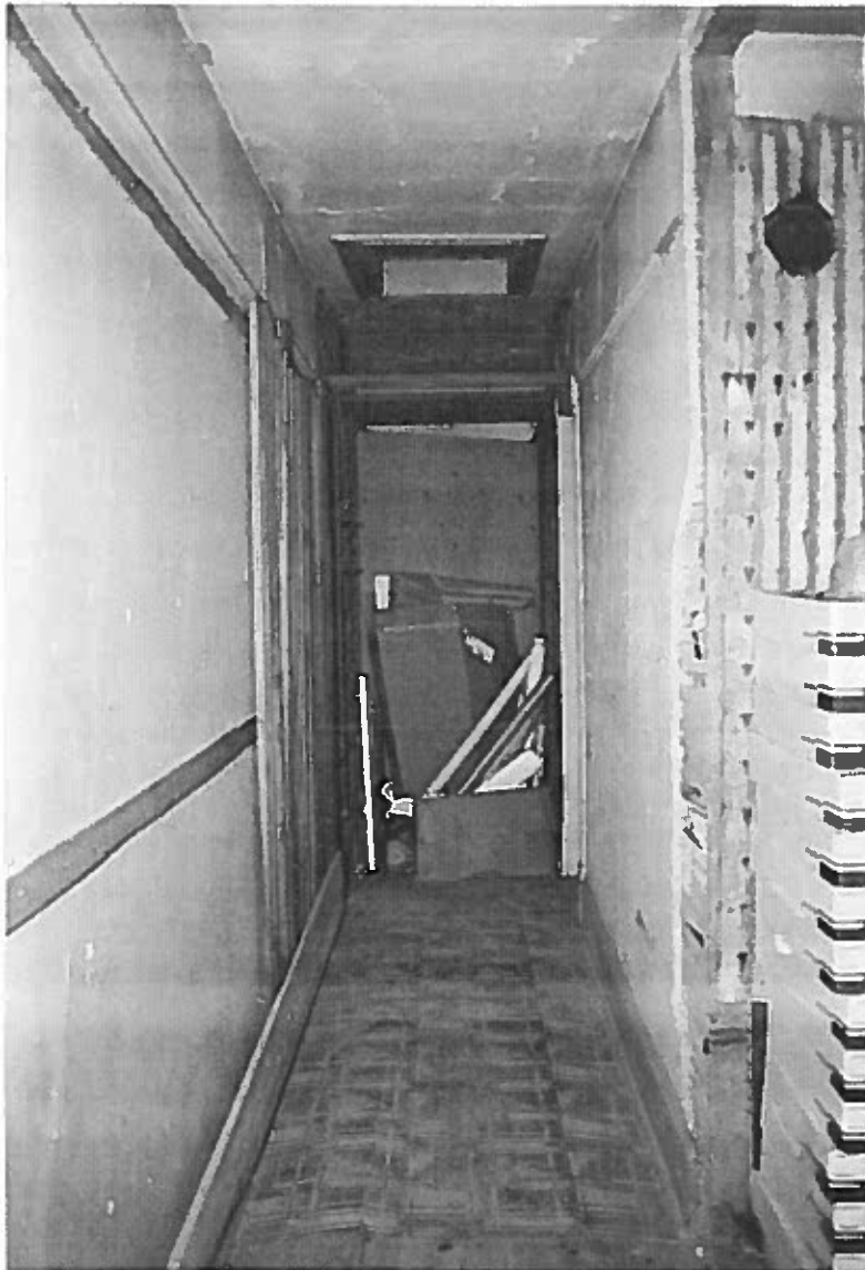
Figure 56: Looking north at the hallway through the center of the building. Both of the walls are structural especially in the center of the building because they hold up the chimney structure above. The foundation below the walls has been altered causing the walls to settle in the center.
