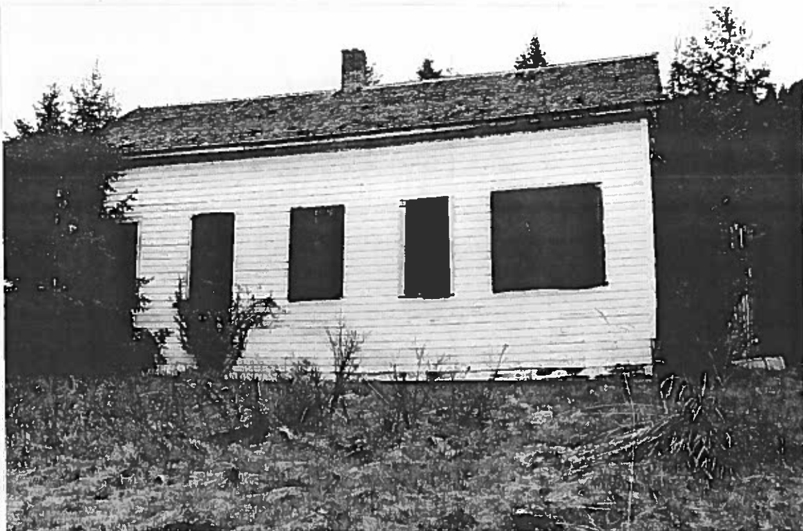
Figure 104: Looking east at the building. Note the settlement in the center of the structure. It does not appear that there is a foundation other than the wood base which appears to be rotted. The roof is in fair condition but it appears that there is potential for some water leaks.
