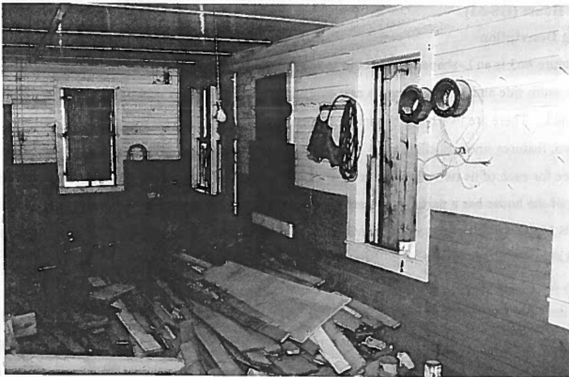
Figure 113: Looking southwest at the interior of the schoolhouse. The windows have been removed and the openings covered over. The window sash are still inside the building.
