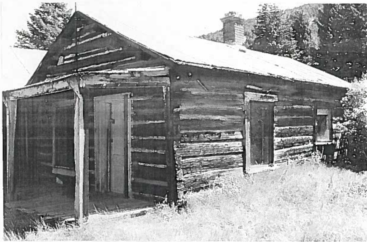
Figure 218: Looking northeast at the log portion of the building. Note the porch which is in poor condition with some rot at the base and in the columns and roof.
