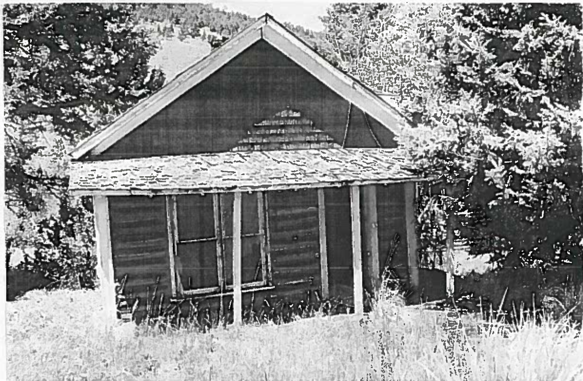
Figure 152: Looking west at the Cabin. Note the high grade at this end of the building causing water to flow onto the porch area from the adjacent road.
