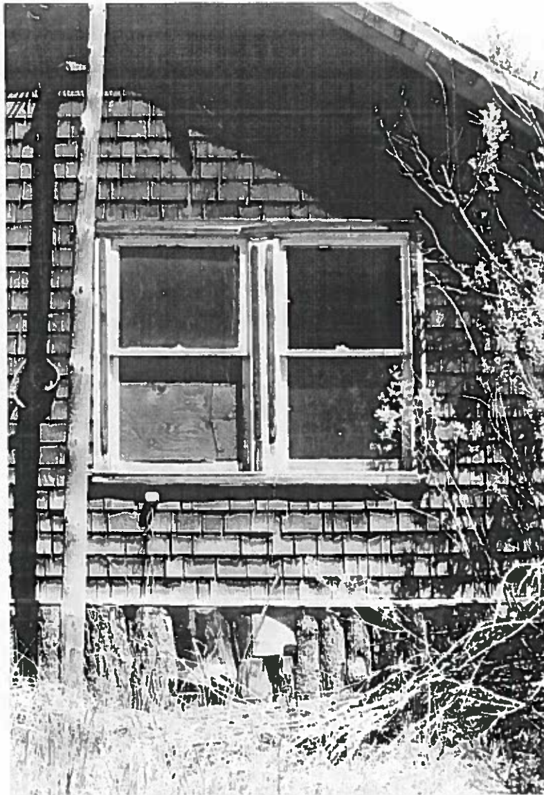
Figure 183: Looking north at a pair of wood double-hung windows typical to the building. The windows are weathered, glass is missing and the glazing is missing. Note the vertical logs that have been put around the base of the building to enclose the crawl space.
