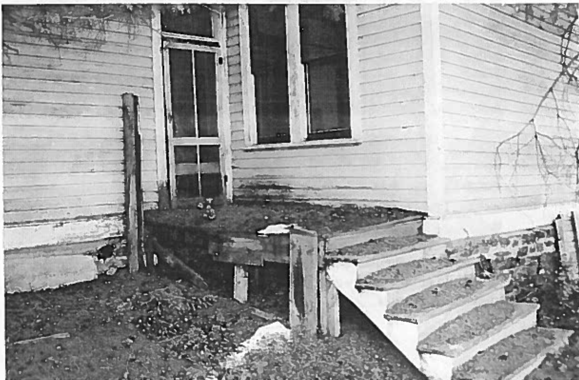
Figure 52: Looking southeast at the back porch of the house. Note the deteriorating porch and the rot along the siding and at the base of the door. The rest of the siding and trim is weathered.
