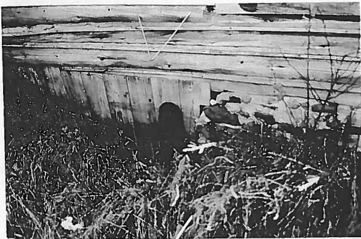
Figure 127: Looking south at the base of the north wall. The stone foundation has been removed partially for the plumbing. Because of the grade water from the roof and slope flows into the basement in this area.
