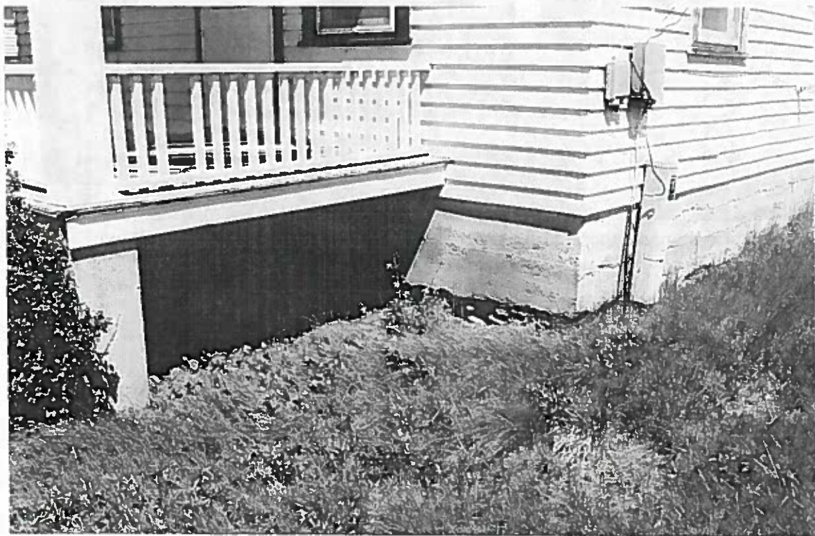
Figure 252: Looking northeast at the building. Note the undermining of the foundation on the front of the building.
