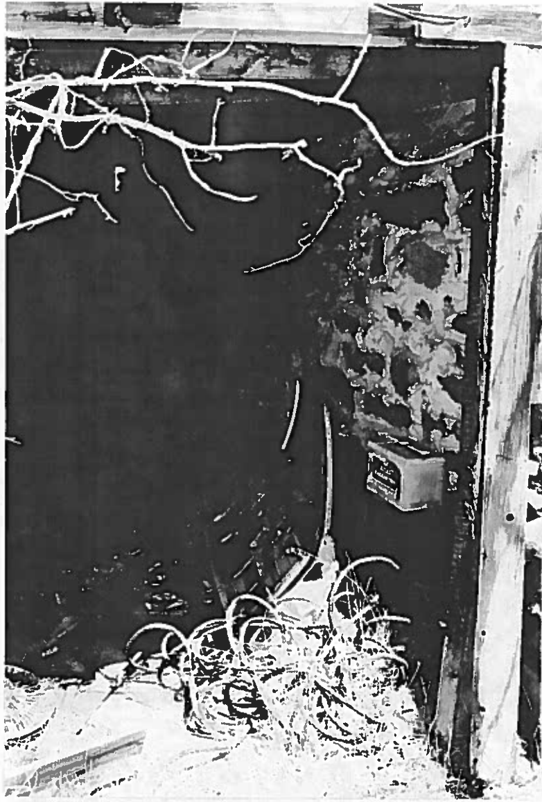
Figure 123: Looking northeast at the base of the foundation under the deck. The foundation is undermined from water coming into the basement on the north side of the building and exiting under the foundation at this point.
