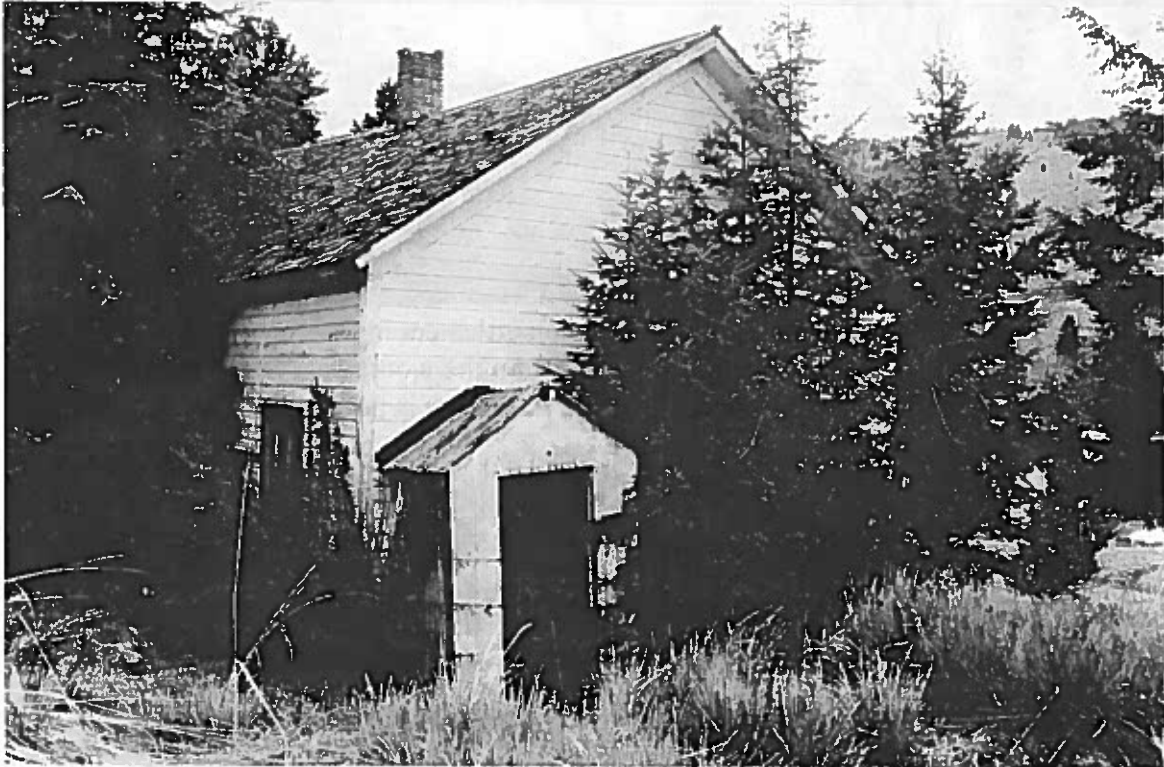
Figure 106: Looking southwest at the building. The grade around the building is causing rot in the base of the structure. The back door enclosure is deteriorating. Note the shrubs and trees against the building.
