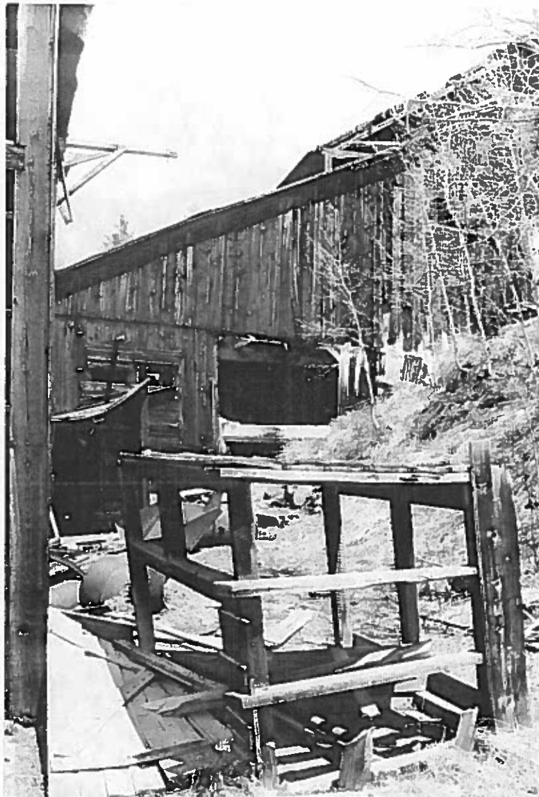
Figure 9: Looking northeast at the exterior of the floatation level of the Mill. Note the weathered wood on the siding but it appears to be dry and in good condition.
