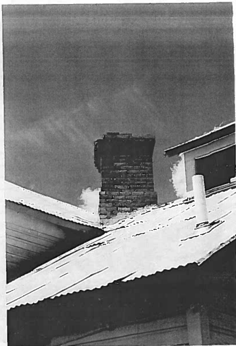
Figure 81: Looking northwest at the roof of the building. There is some brick and mortar deterioration on the top of the chimney. Some of the metal roof panels are loose.
