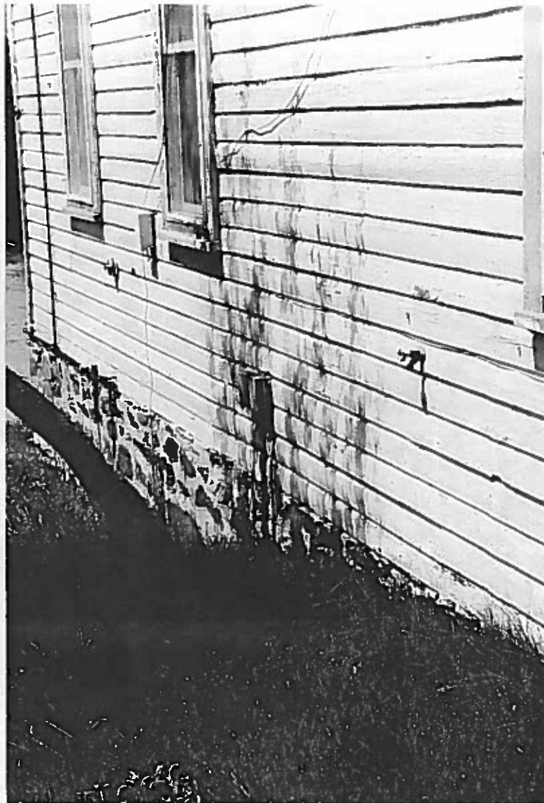
Figure 82: Looking northwest at the stone foundation and wall on the south side of the building. Note some wood deterioration where the grade comes up along the base.
