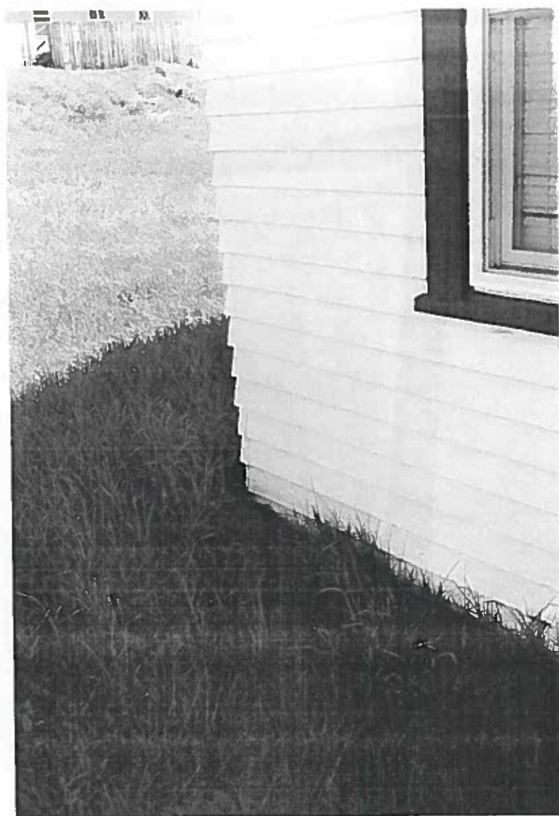
Figure 255: Looking southeast at the base of the building near the back. Note the high grade around the building at this point which is causing some deterioration of the wood materials.
