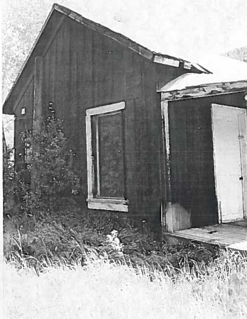
Figure 222: Looking northeast at the wood frame addition. The upper part is in good condition but the base of the building is rotting out.
