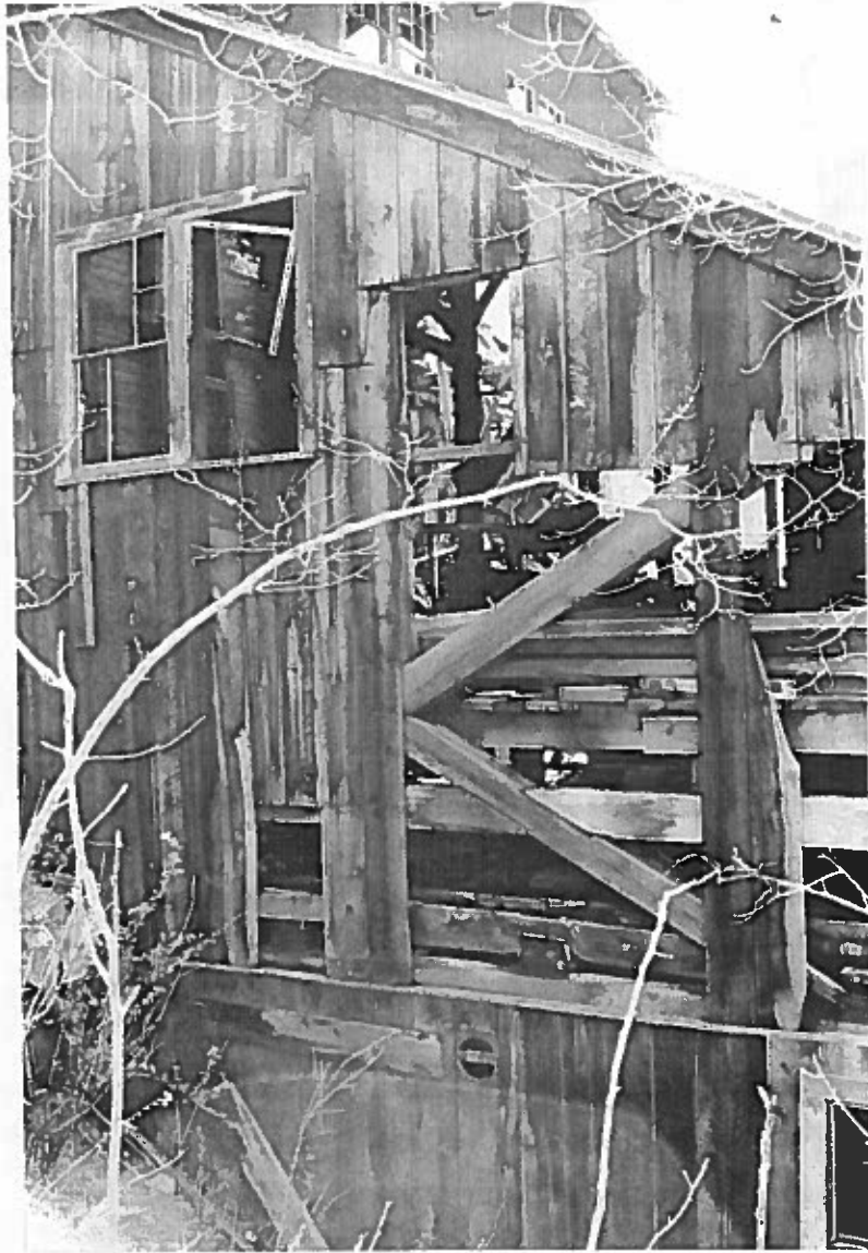
Figure 16: Looking south at the north side of the Mill at the floatation level.. Note the missing siding that was removed from the building. The windows are in poor condition.
