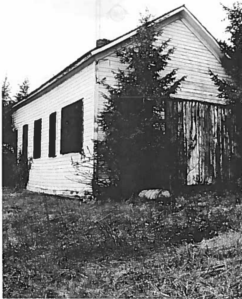
Figure 103: Looking northeast at the Schoolhouse. Note the deteriorated siding and the trees along the foundation and siding.
