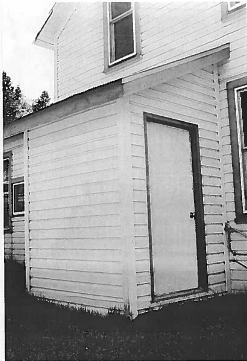
Figure 72: Looking southeast at the shed roof addition. There is a concrete slab at the base but the wood materials on the slab are rotted.
