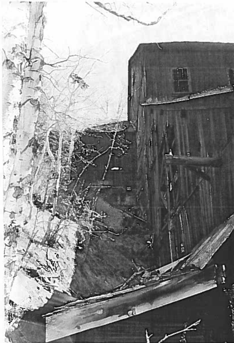
Figure 15: Looking east up along the north end of the Mill. Note the slope of the grade into the side of the building which is causing some deterioration of materials due to the water penetration.
