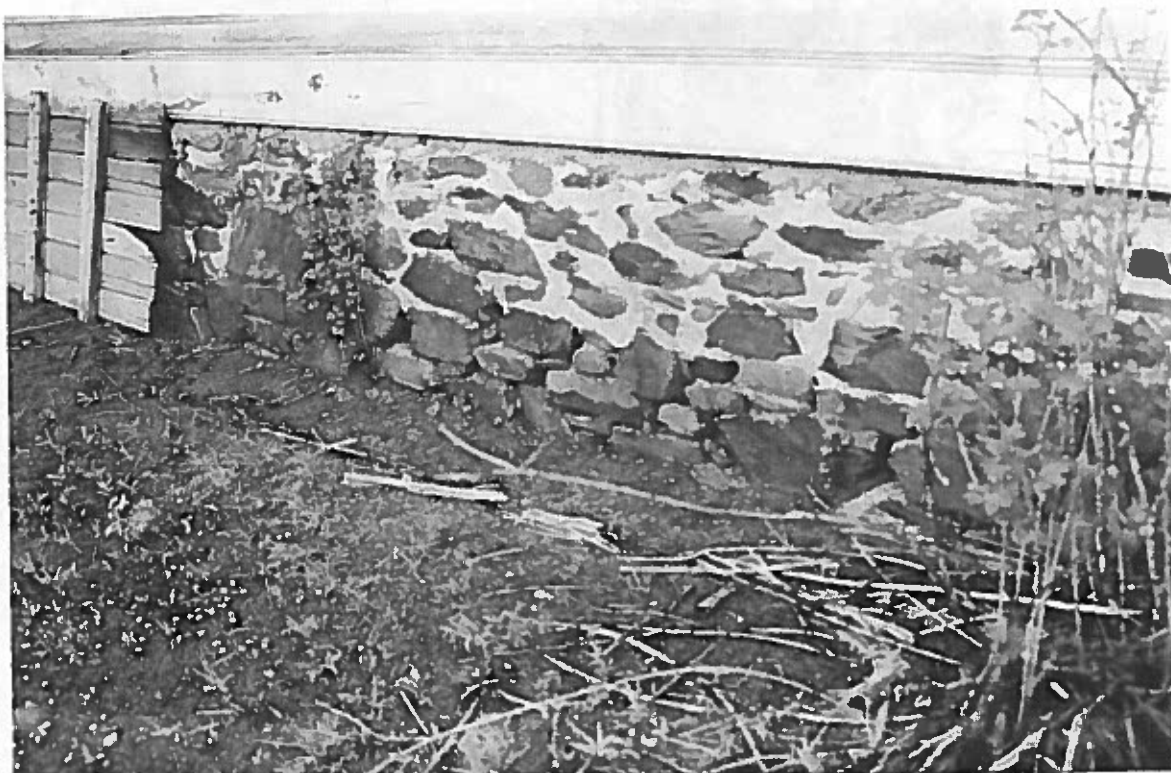
Figure 48: Looking northeast at the stone foundation of the building. Note the missing mortar at the base due to water penetration. Most of the foundation with the exception of the northeast corner is in good condition.
