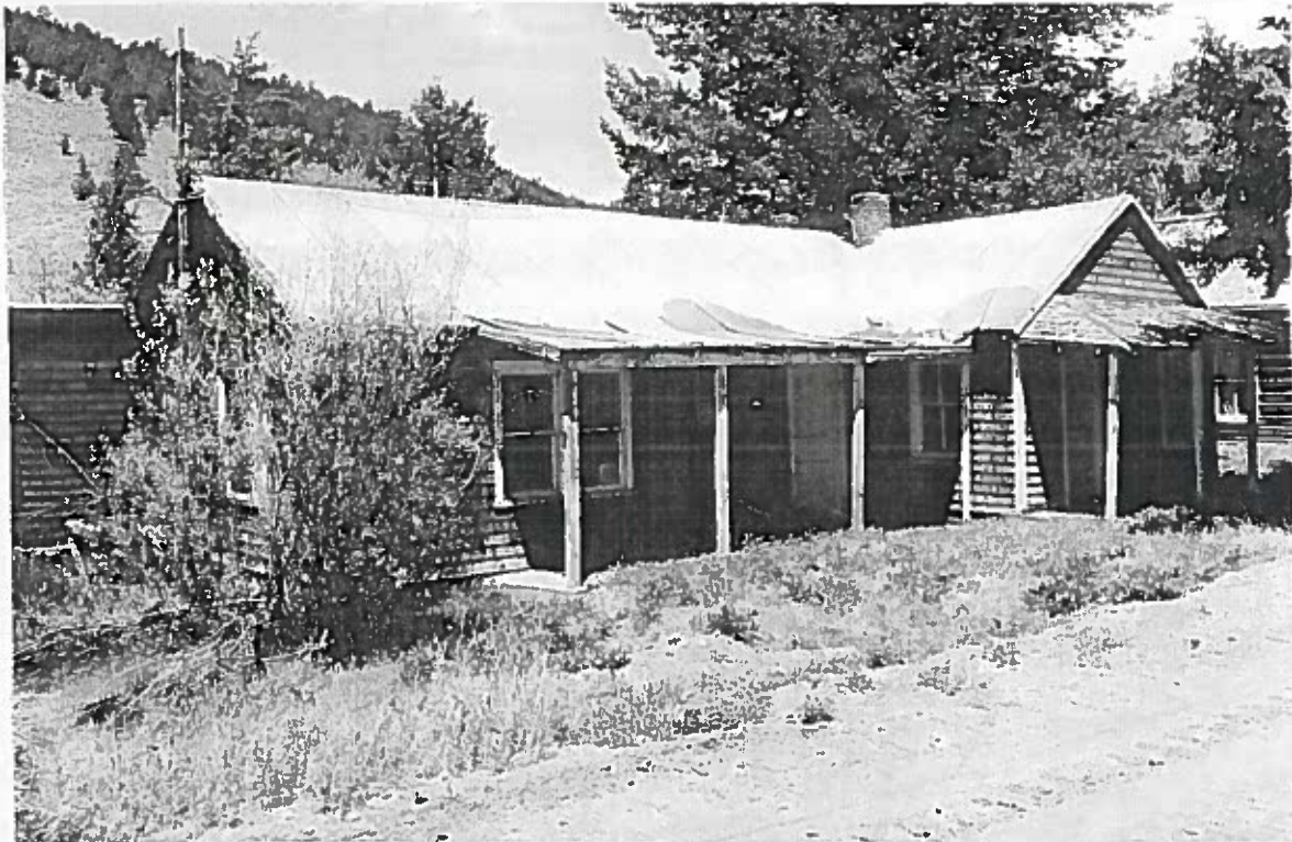
Figure 180: Looking northwest at the Cabin. Note the metal roof which is coming apart on the lower shed roof over the porch.
