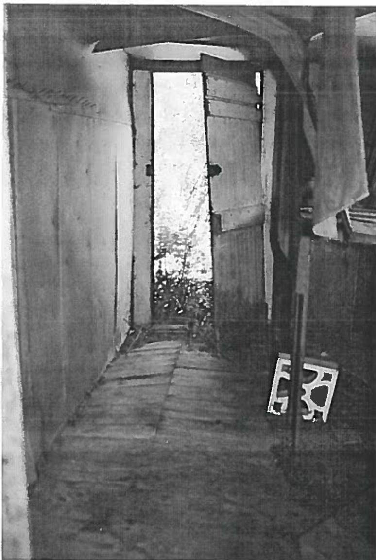
Figure 231: Looking north at the north wood frame addition to the building. Note the buckled floor built on grade. The walls are a thin frame with a hardboard siding.
