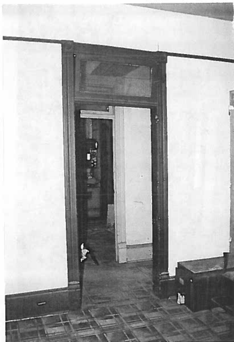
Figure 61: Looking east at the doorway to hallway from the northwest room. Note the settlement to the right of this wall also.
