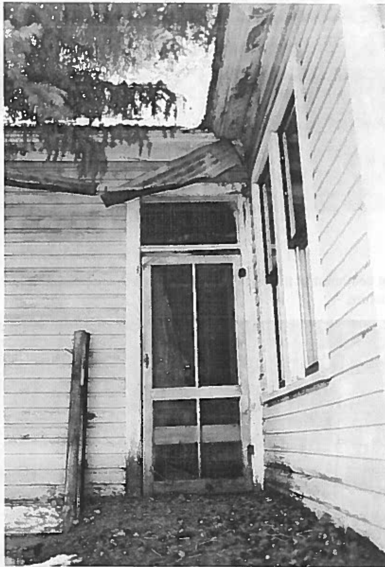
Figure 53: Looking east at the back door. Note the failing gutter along the eave and the rotted soffit due to some previous roof leaks.
