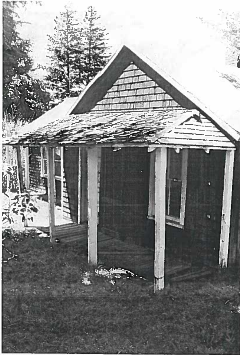
Figure 191: Looking southwest at the Cabin. Note the wood shingle roof over this porch structure which is in poor condition in some areas.
