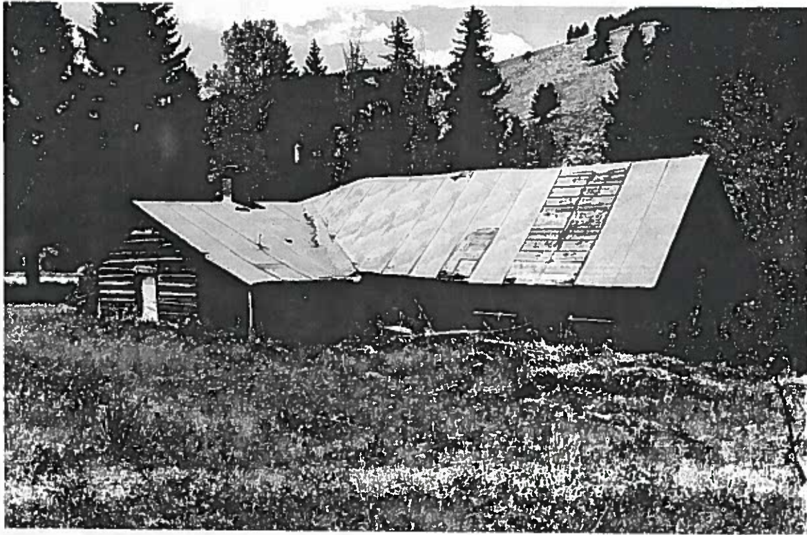
Figure 213: Looking southwest at the Cabin. Note the missing sheet asphalt on the roof, to the right. Also the grade slopes towards the building in this area.
