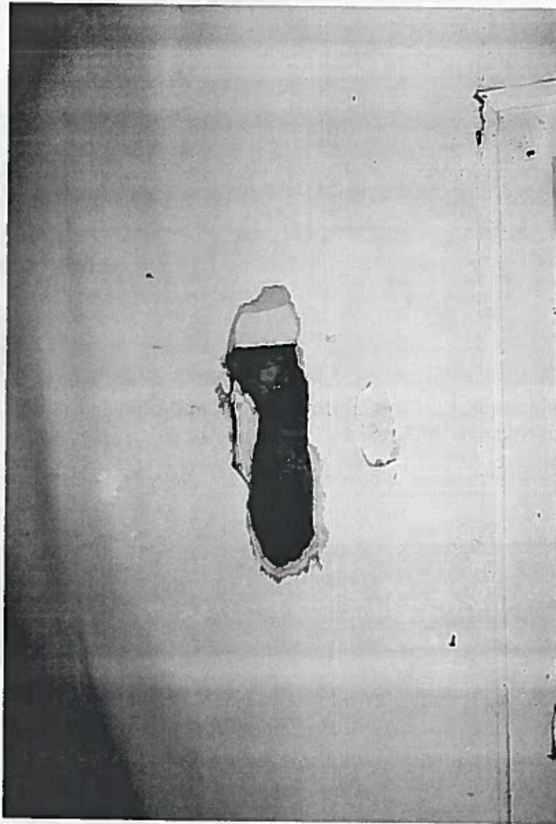
Figure 141: Looking northeast at the hole in the wall. Note the logs under the sheetrock.
