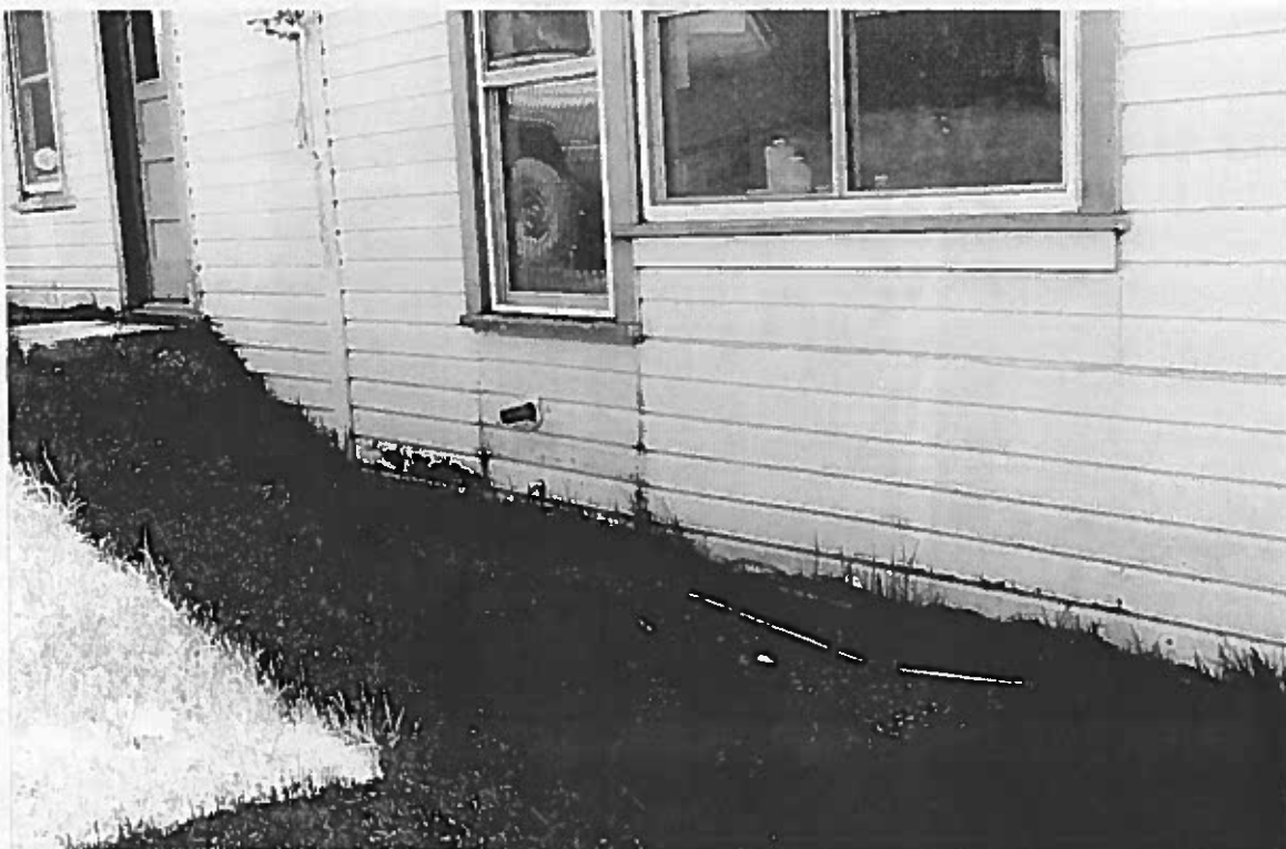
Figure 74: Looking southeast at the north wall. Note the rotted siding and base.
