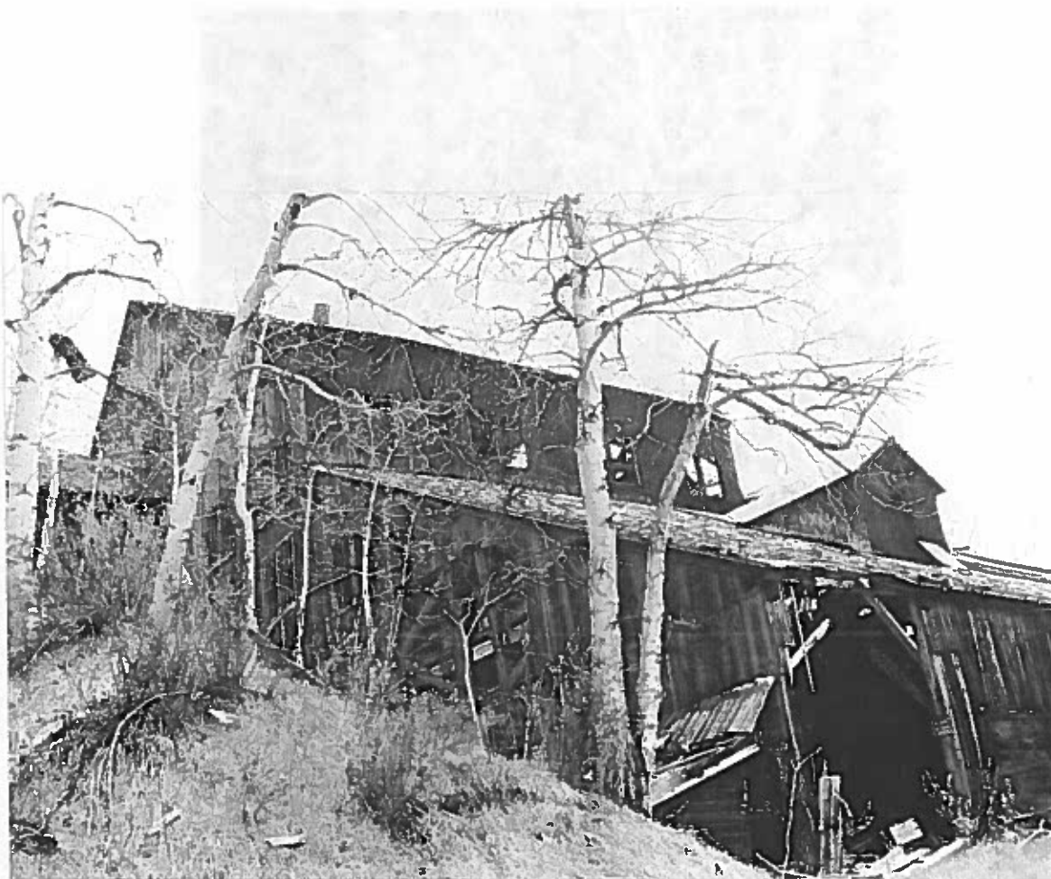
Figure 14: Looking southeast at the lower end of Mill. Note the poor condition of the wood shingle roof. Many of the shingles are loose and deteriorating.
