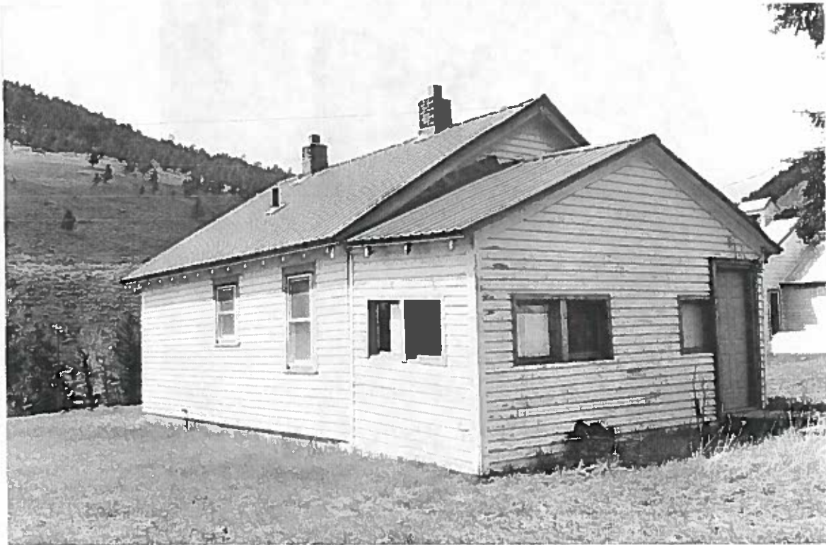
Figure 239: Looking northwest at the residence. Note the high grade around the base of the addition and the deteriorating paint on the walls.
