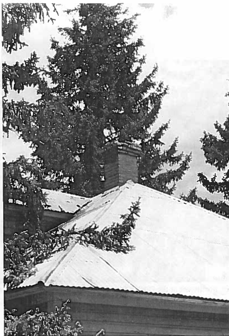
Figure 41: Looking northwest at the roof of the building. Note the galvanized metal roof which was put over the original wood shingle roof for protection. The upper part of the chimney is deteriorating and some of the mortar is missing.
