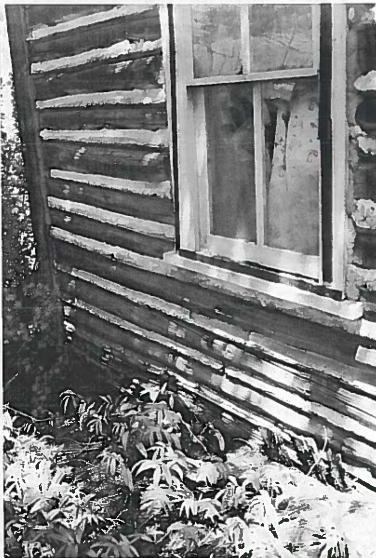
Figure 155: Looking northwest at a section of the log wall. Most of the log work is in good condition and some of the daubing is in good condition. However note the rotted sill log and the grade change along the building.
