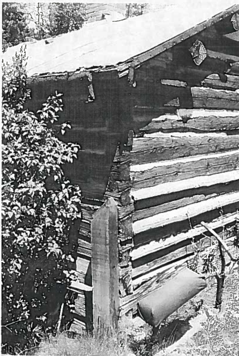
Figure 217: Looking northwest at a corner notch on the building. Generally with the exception of the base logs the wall logs are in good condition. Note the damage on the edge of the roof sheathing.
