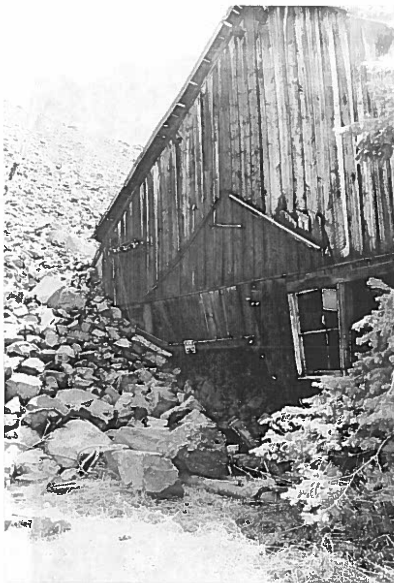
Figure 20: Looking southeast at the upper end of the Mill. Note the rock from the creation of the upper parking lot that has crushed the end of the building.
