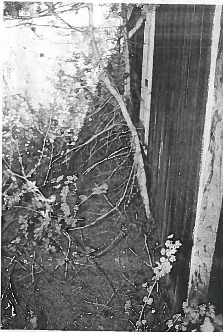
Figure 189: Looking east along the wall of the additions onto the original building showing the buildup of materials and trees where the surfaces are rotting because of water penetration.
