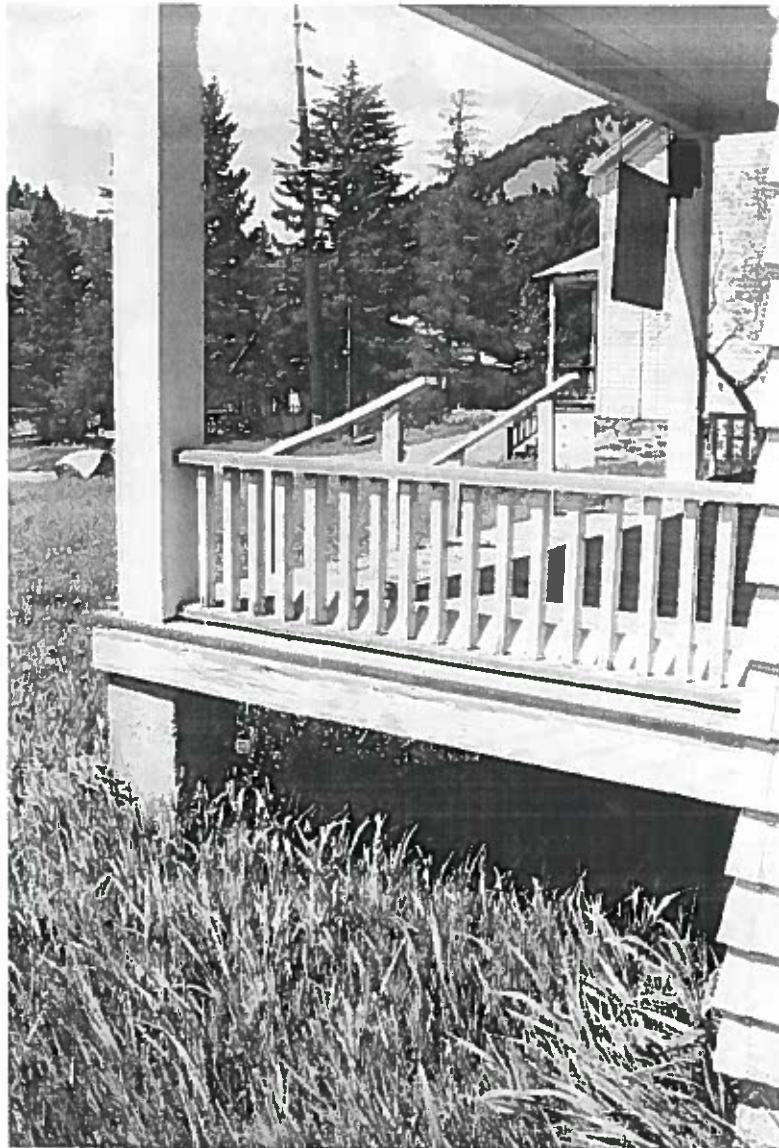
Figure 242: Looking northwest at the front porch. The base of the railing and base of the porch is weathered.
