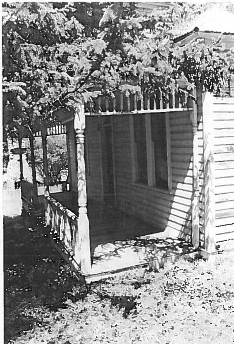
Figure 42: Looking west at the porch of the building. The structure is rotted due to the high grade around this end of the building. The turned columns, railings, and roof are in good condition.
