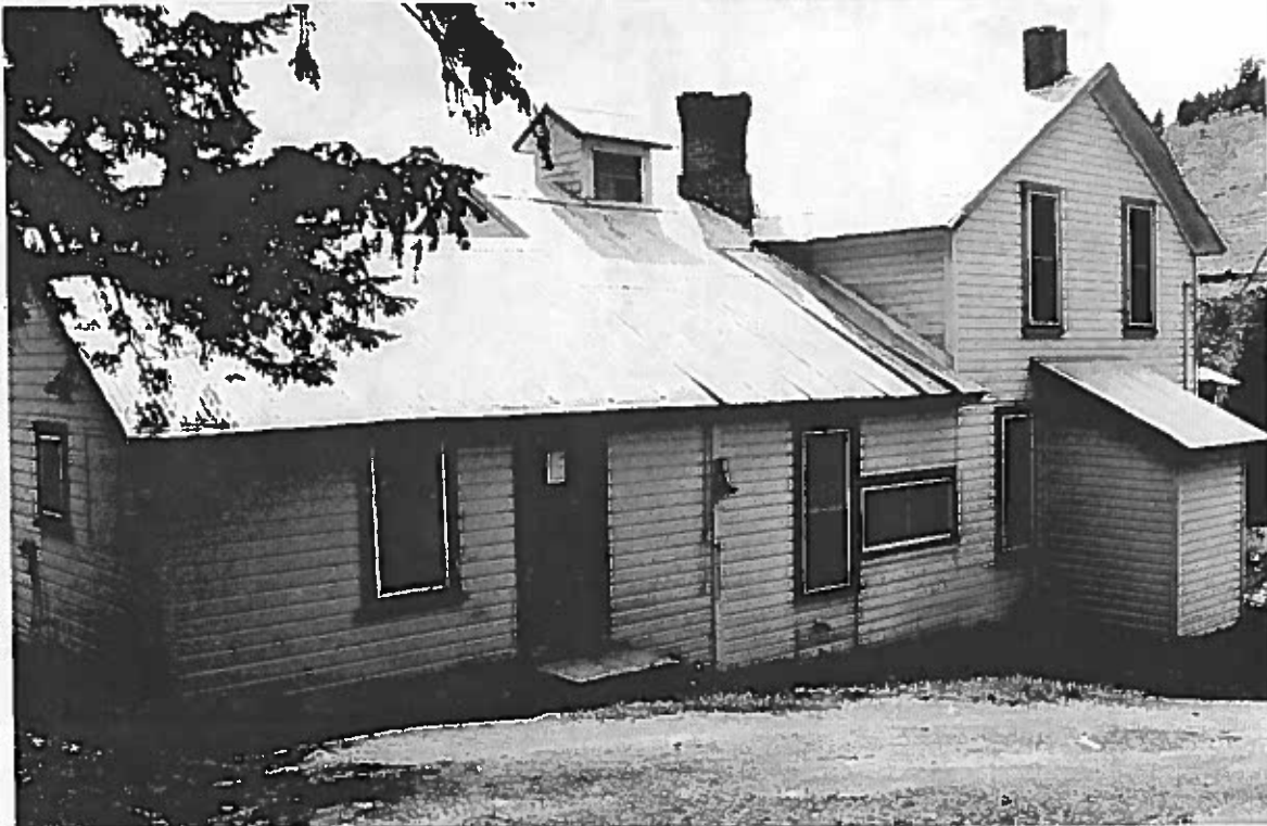
Figure 77: Looking southwest at the building. The metal roof is generally in good condition with the exception of some loose panels.
