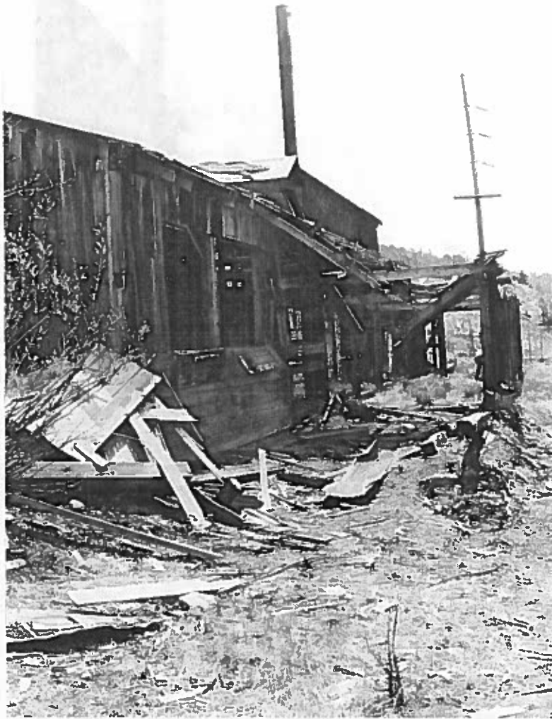
Figure 12: Looking south along the lower end of the Mill. Note the sections of collapsed roof and beams.
