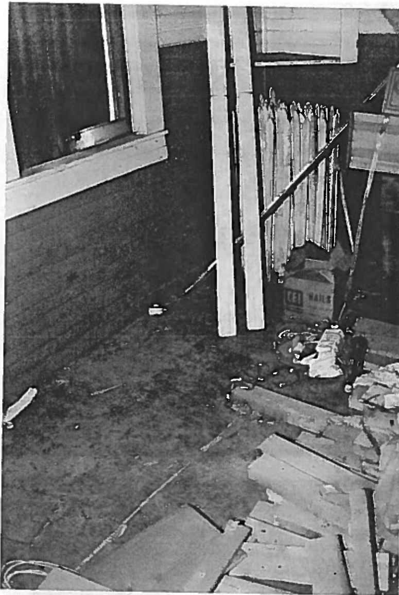
Figure 111: Looking northeast along the base of the walls. There is some deteriorating floor boards in this area.
