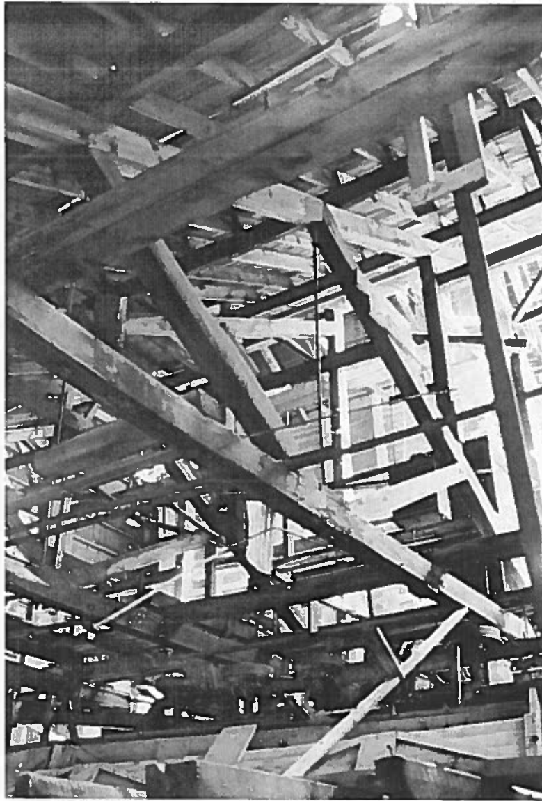
Figure 32: Looking east at the wood truss structure over the stamp and ball mill area. These trusses also appear to be in good condition with the exception of the south end that have collapsed.
