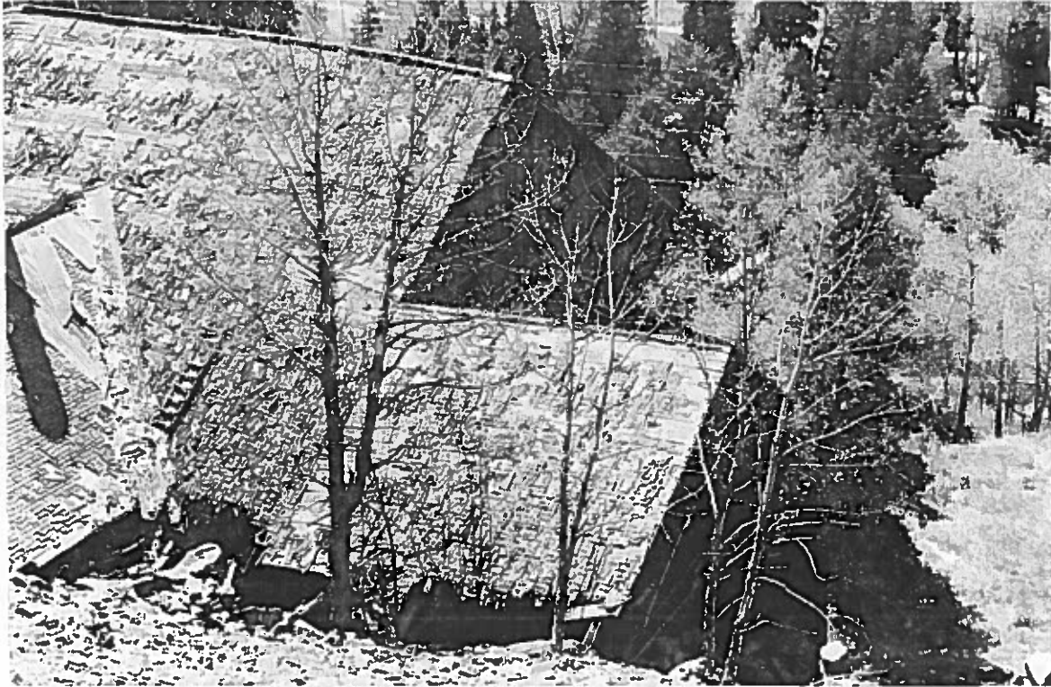
Figure 21: Looking southwest at the roof of the Mill from the upper parking lot. Note the missing and deteriorated wood shingle roof. The eave of the roof has been crushed from the rock.
