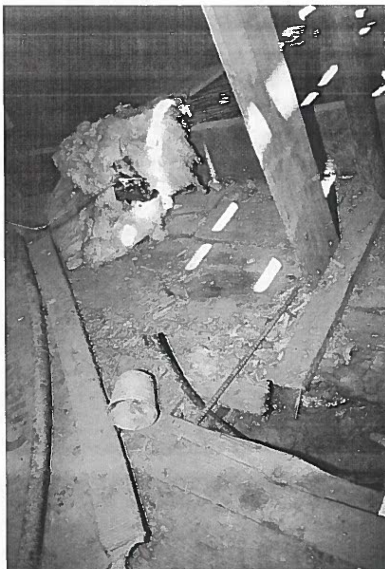
Figure 232: Looking west at the rotted wood floor in the north addition.
