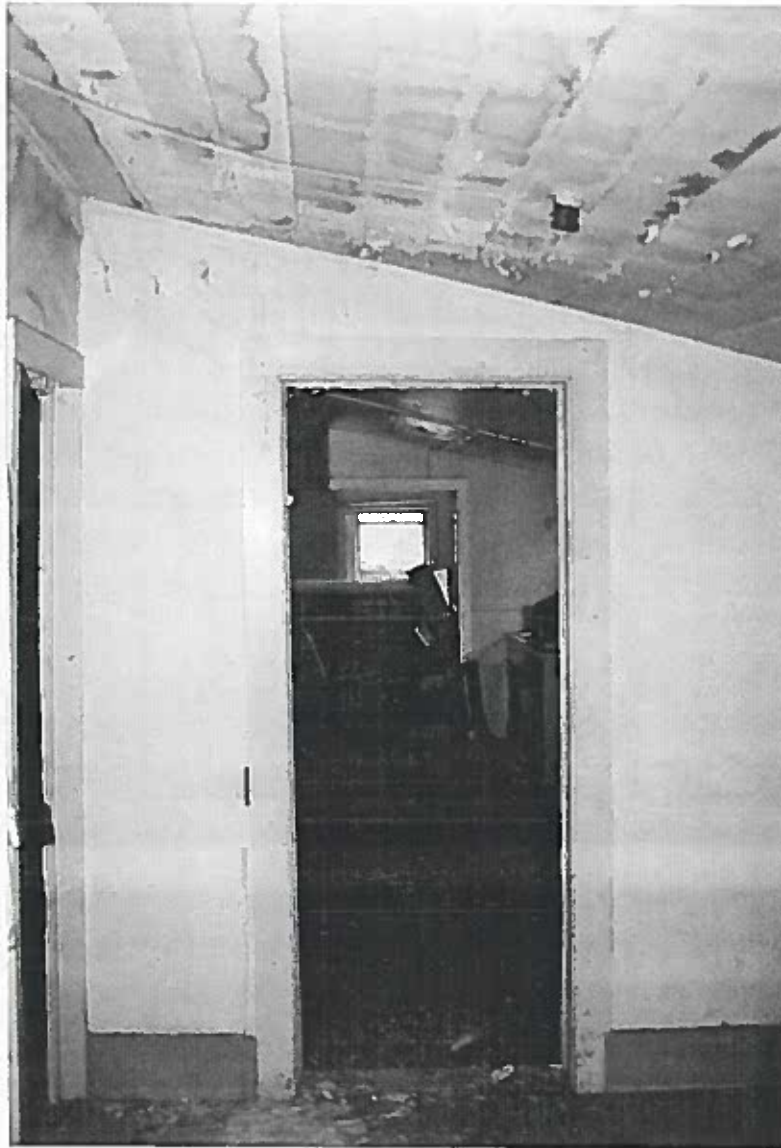
Figure 204: Looking south at the back bedroom. Note the water damage on the ceiling from the leaking roof. The roof appears to have been covered and there is no moisture penetration at this time.
