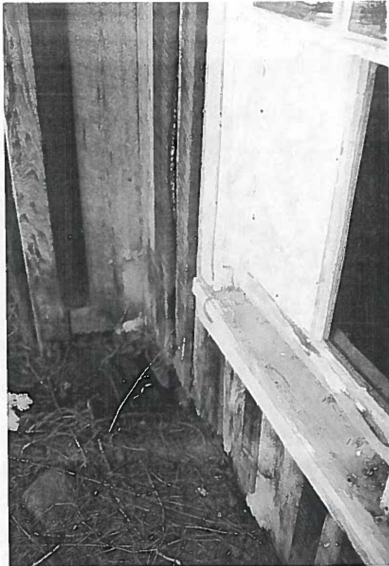
Figure 188: Looking southeast at the base of the frame additions to the Cabin. Note the rotted wood board and batten siding on the ground where there is no foundation. Also note the weathered window.
