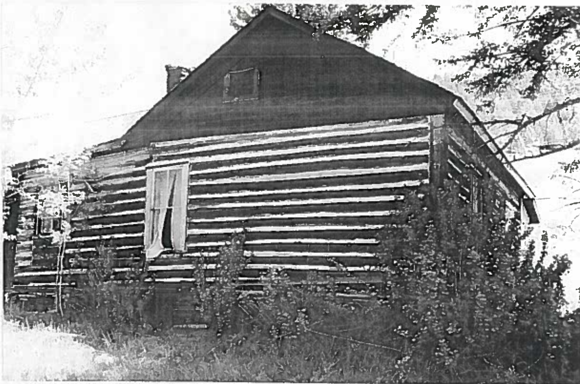
Figure 156: Looking northeast at the back of the building. The log work and gable end shingles are in good condition. The brick chimney has loose bricks and missing mortar.
