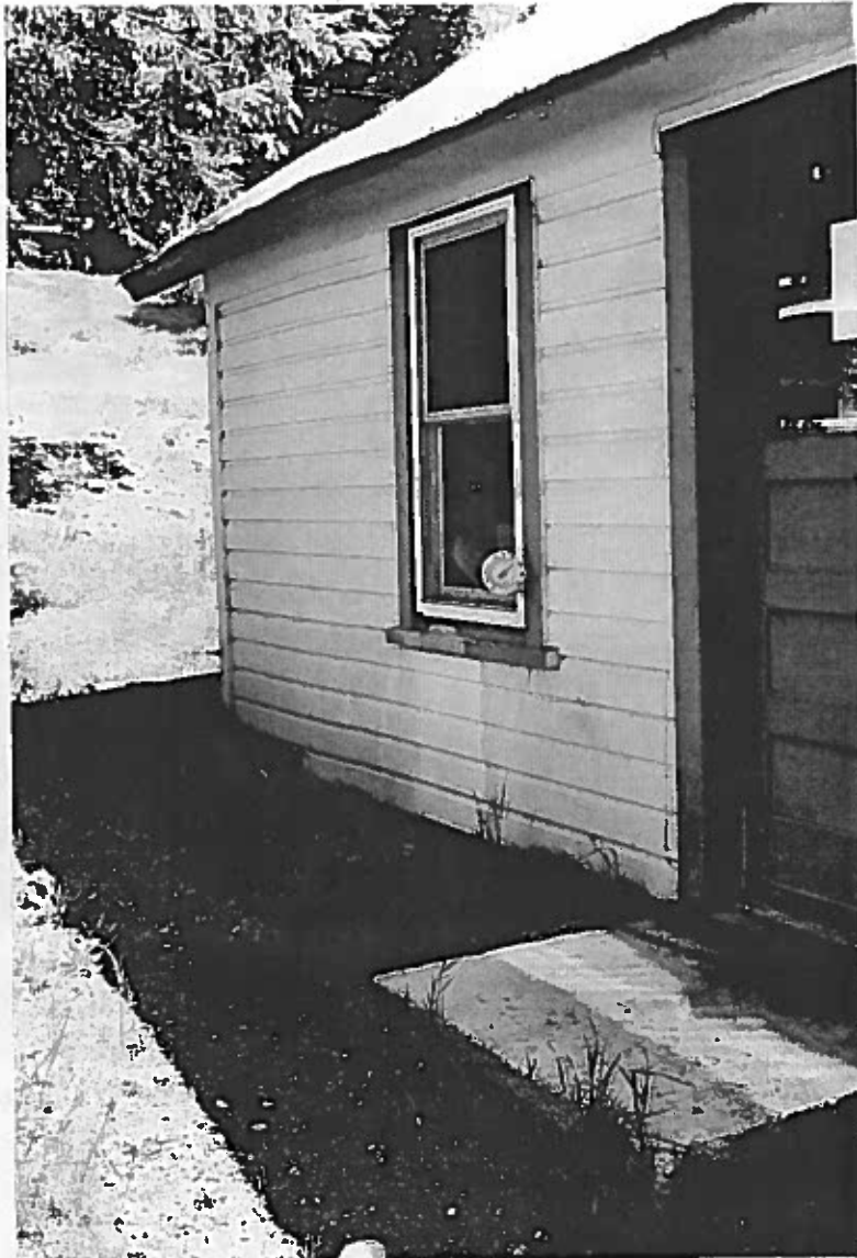
Figure 76: Looking southeast at the back door and window. Note the high grade against the building.
