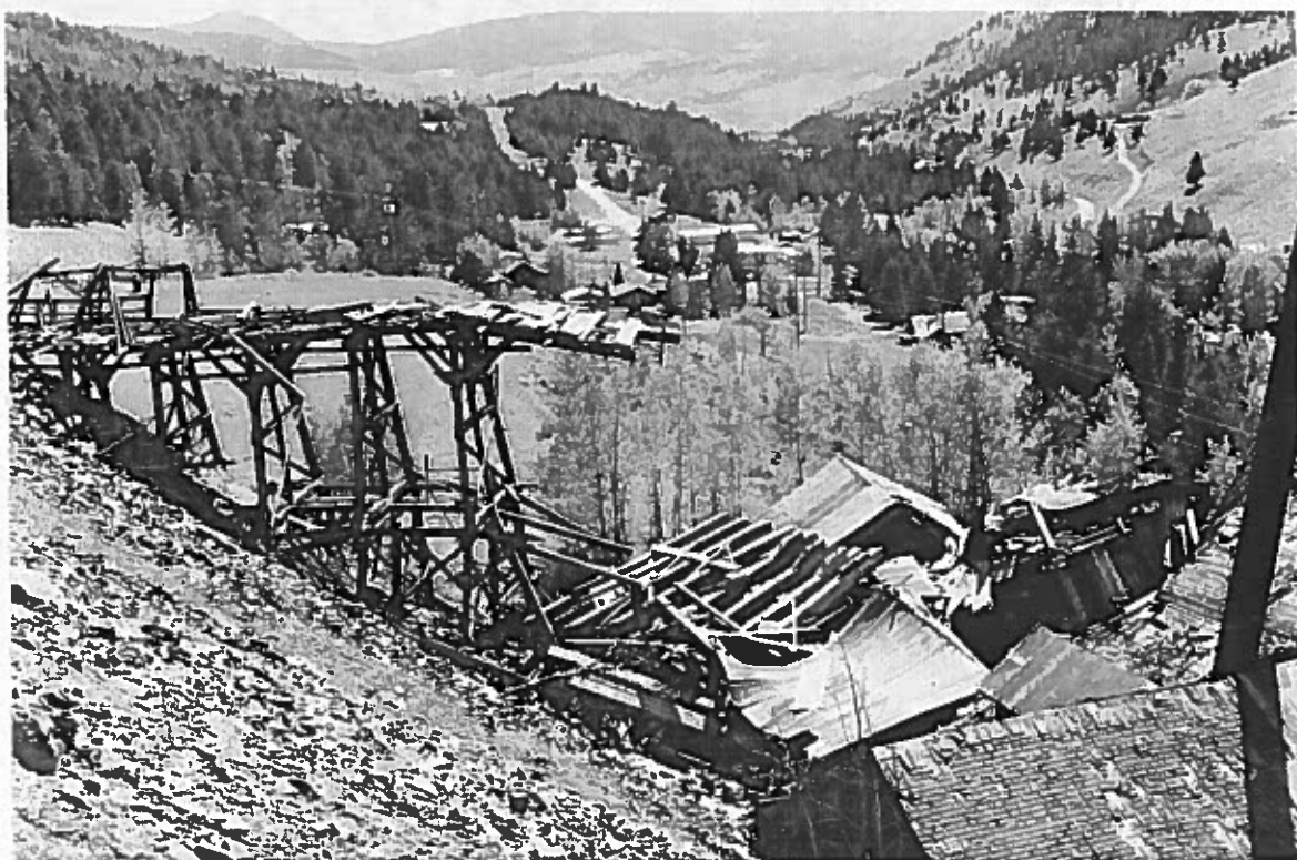
Figure 25: Looking southwest at the tramway and the collapsed ore bin area.
