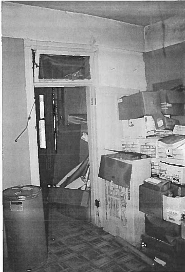
Figure 60: Looking northwest at the doorway to the hallway from the kitchen. The wall is settling to the left from the heavy chimney and limited support below.
