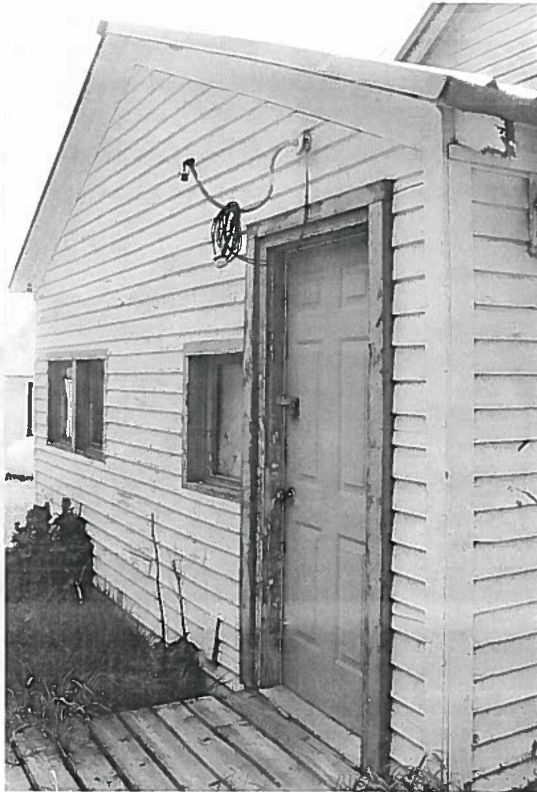
Figure 240: Looking southwest at the back door of the addition. This is a metal paneled door. Note the weathered wood frame around the door.
