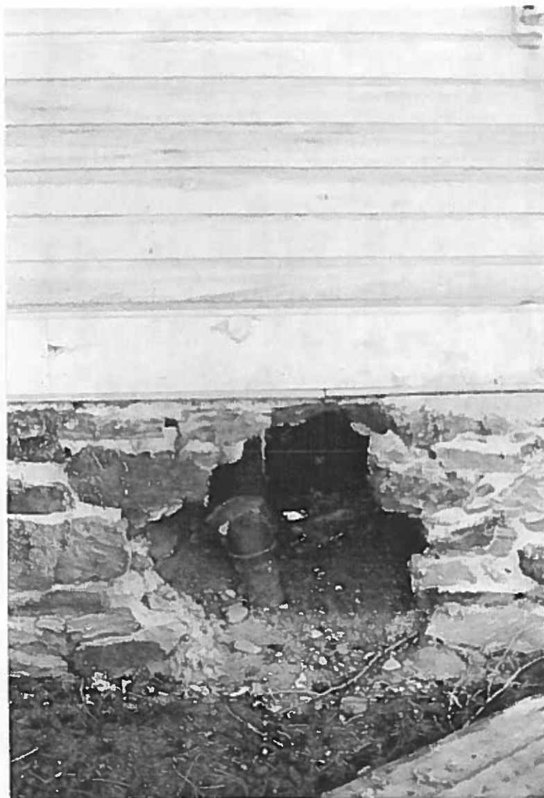
Figure 49: Looking east at the hole in the foundation on the west side where a later drainage system was added. Note the pipe in the opening. As the piping goes through the center foundation walls a large area of the stone foundation was removed causing the chimney structure to settle.
