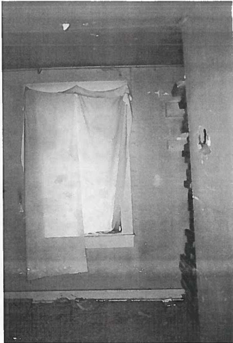
Figure 169: Looking west a the middle bedroom. Note the plaster deterioration due to vandalism.
