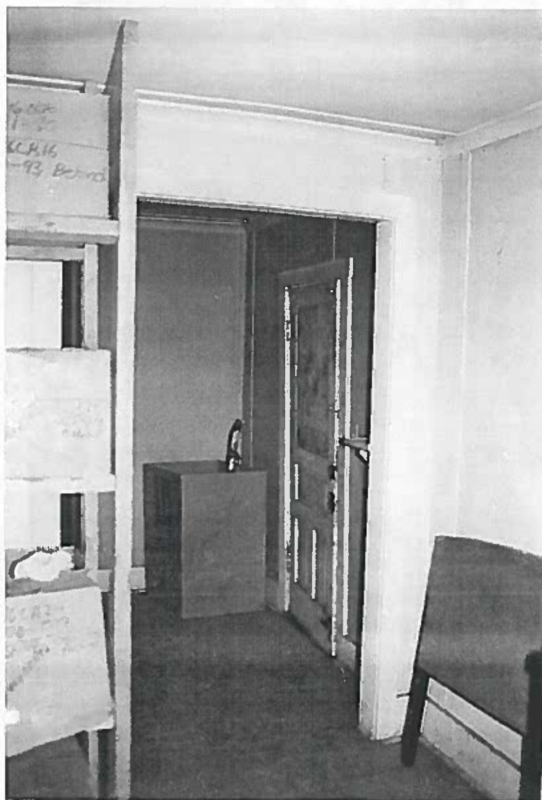
Figure 195: Looking northeast from the living room at the front entrance door into the vestibule. The door is weathered with some rot at the base. Plywood covers the glass area.
