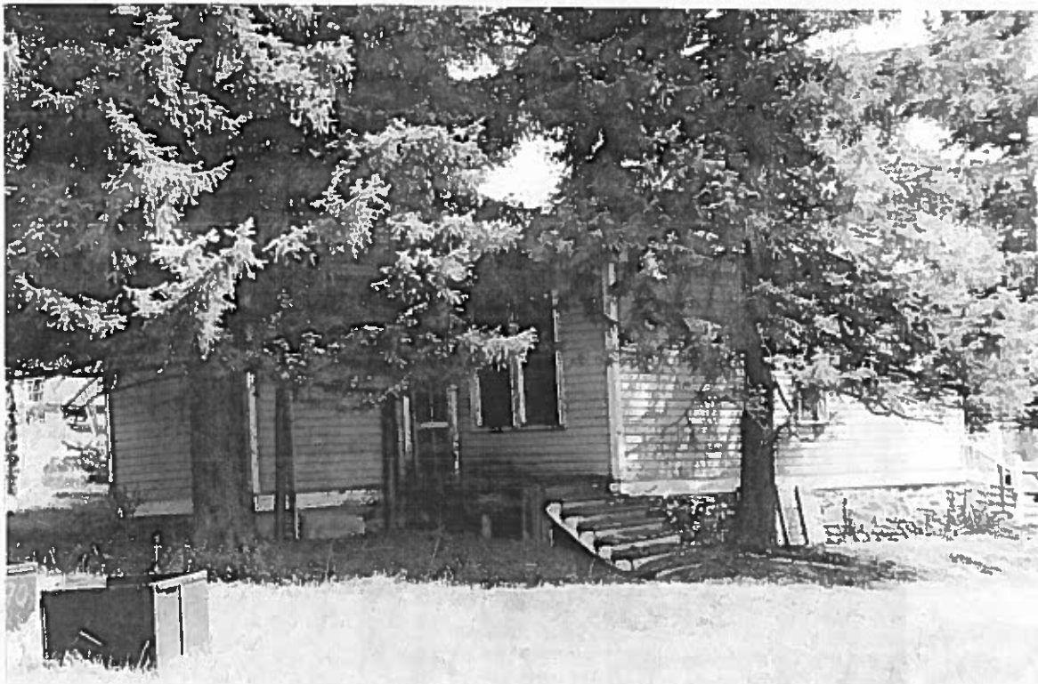
Figure 51: Looking southeast at the Bush House. The trees are causing some damage to the roof of the structure.
