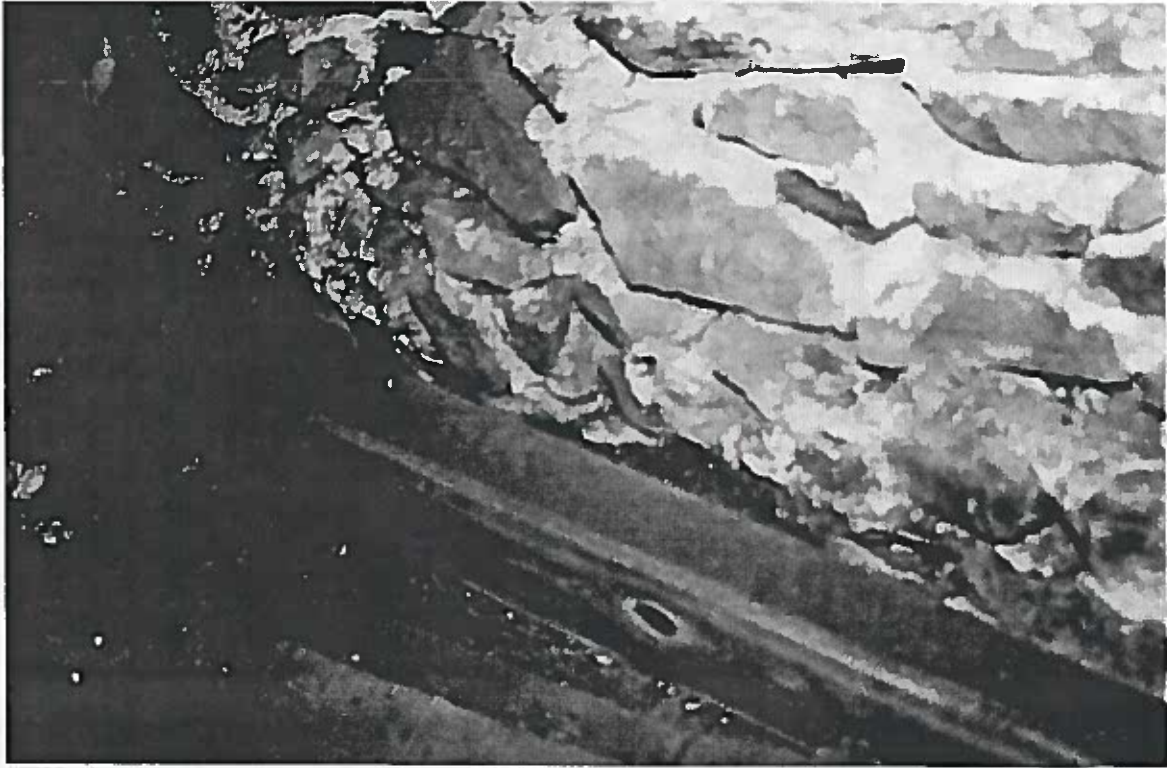
Figure 131: Looking west at the area of the foundation that is undermined because of the water flowing through the building.
