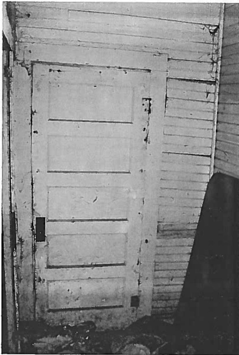
Figure 112: Looking north at the back door to the building. The door is worn and there is some rot at the base.
