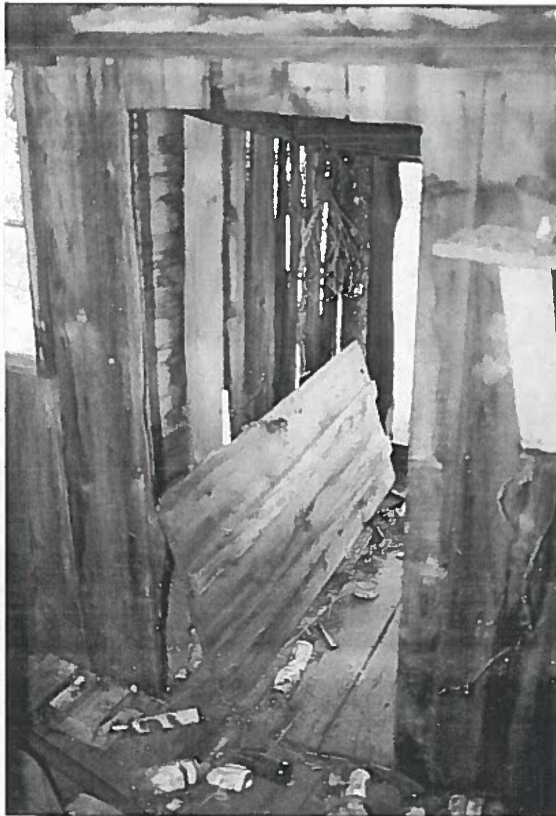
Figure 177: Looking north at the frame addition. Note the rotted floor boards, missing or removed doors, and open areas in the walls.
