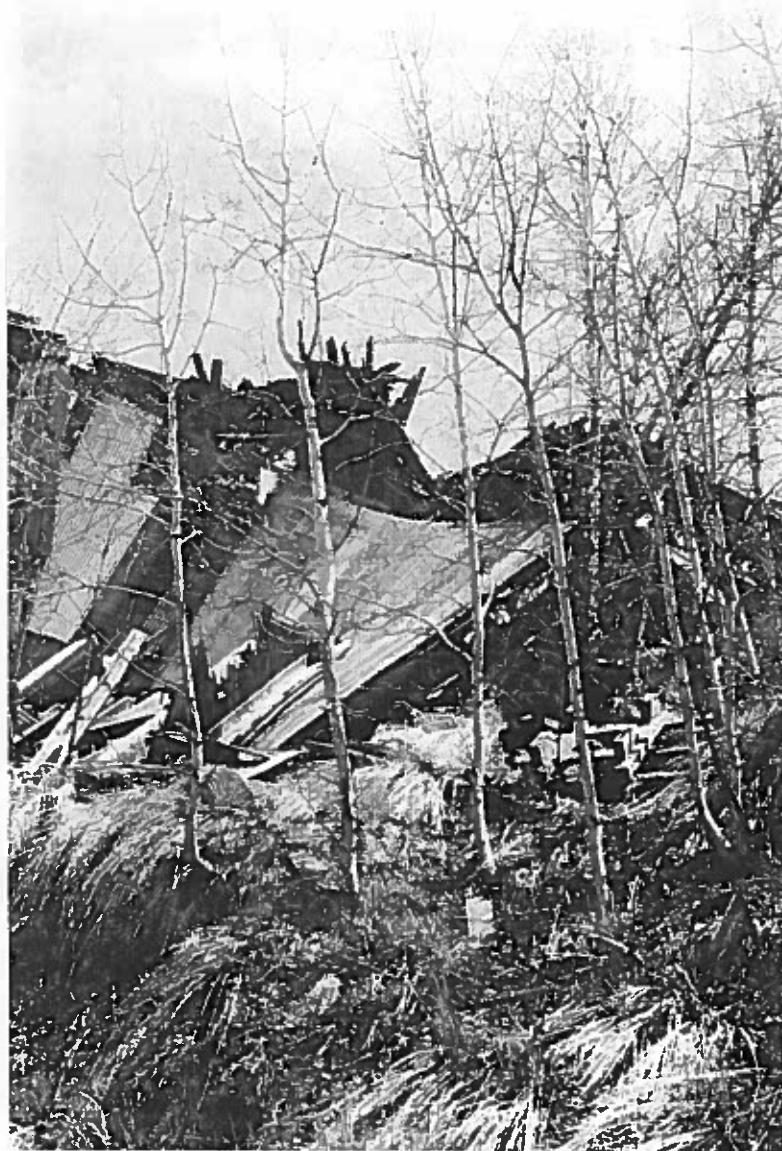
Figure 10: Looking east at the collapsed ore bin area of the Mill. Most of the roof structure and the top of the ore bins have collapsed on the south end of the building.
