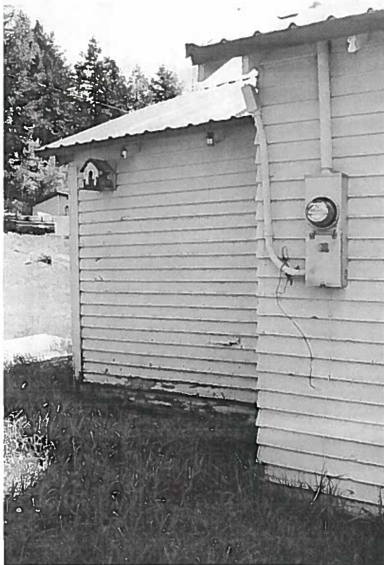
Figure 237: Looking southeast at the back addition to the residence. Note the rotted base materials because of the high grade around the back of the building.
