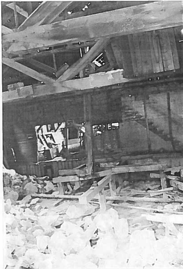
Figure 36: Looking south towards the upper boiler room on the upper end of the Mill. The rock is from the base for the parking lot that has rolled into the structure. The center section of the structure appears to be in good condition.
