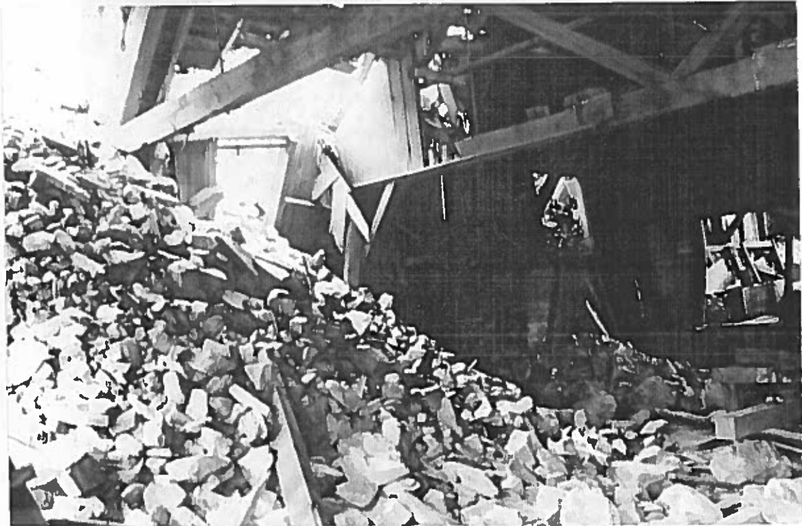
Figure 35: Looking southeast at the crushed wall on the upper end of the Mill when the rock was placed here for the parking area above. The main wall was pushed in and off its foundation.
