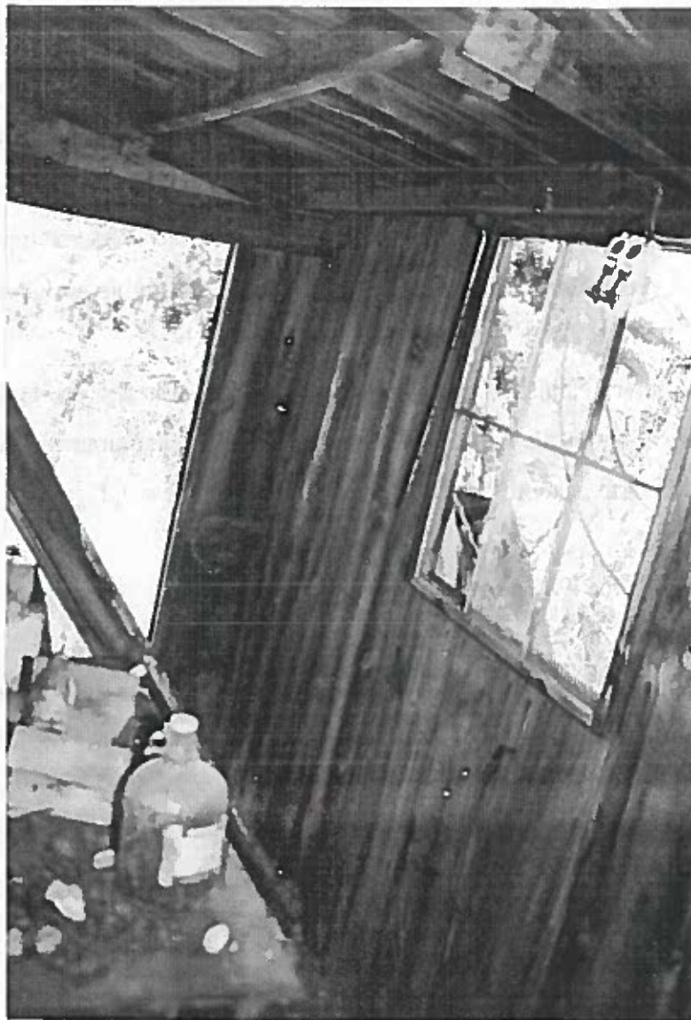
Figure 178: Looking northeast at a section of the frame addition. The base of the walls are deteriorating and the window is in poor condition.
