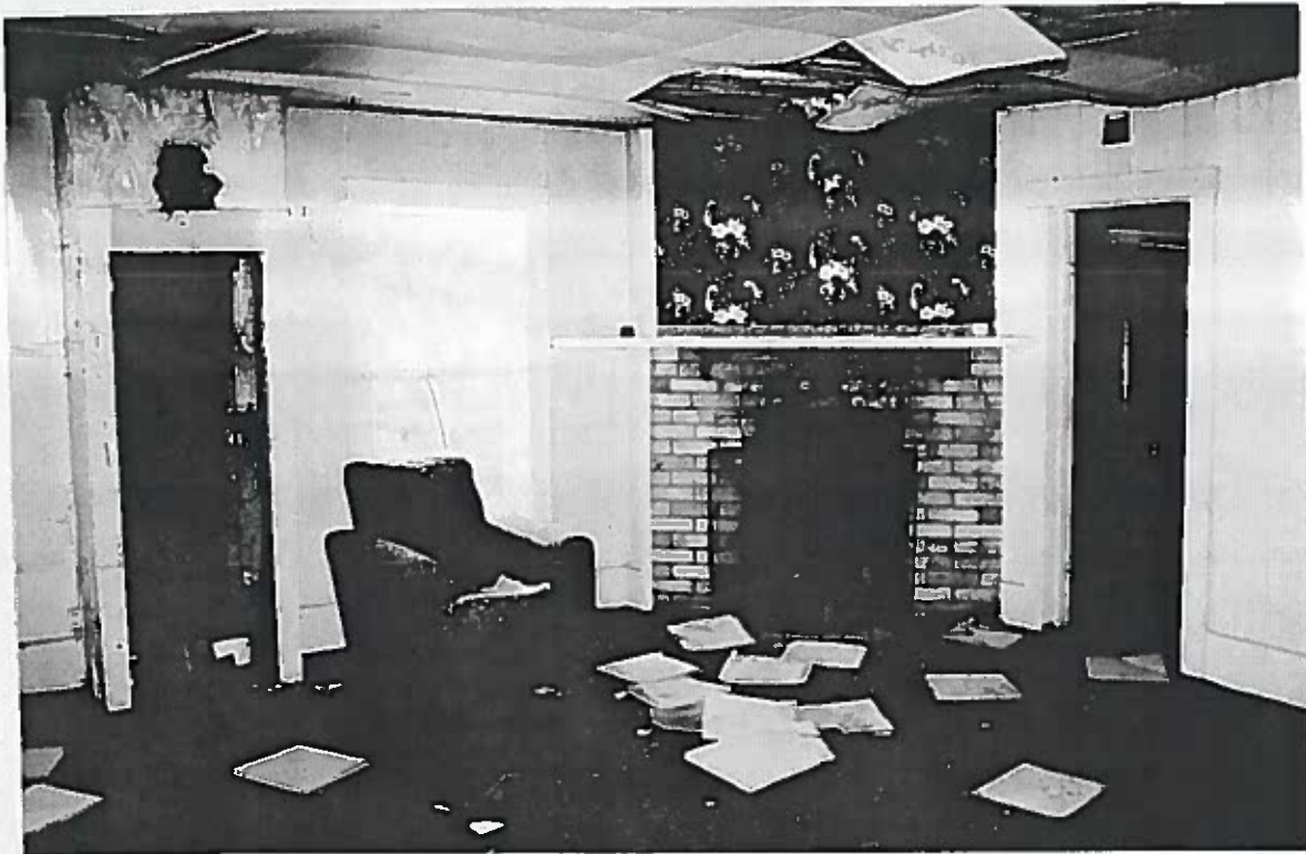
Figure 137: Looking southwest at the living room and fireplace. Note the newer materials that have been added to the walls and ceiling. Original wall and ceiling paper exists under the newer materials.
