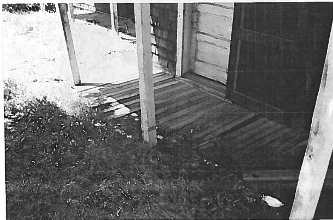
Figure 192: Looking southwest at the porch floor which is deteriorating badly because of the buildup of earth around the base and drainage of water from the road. Note the rotting bases of the columns also.
