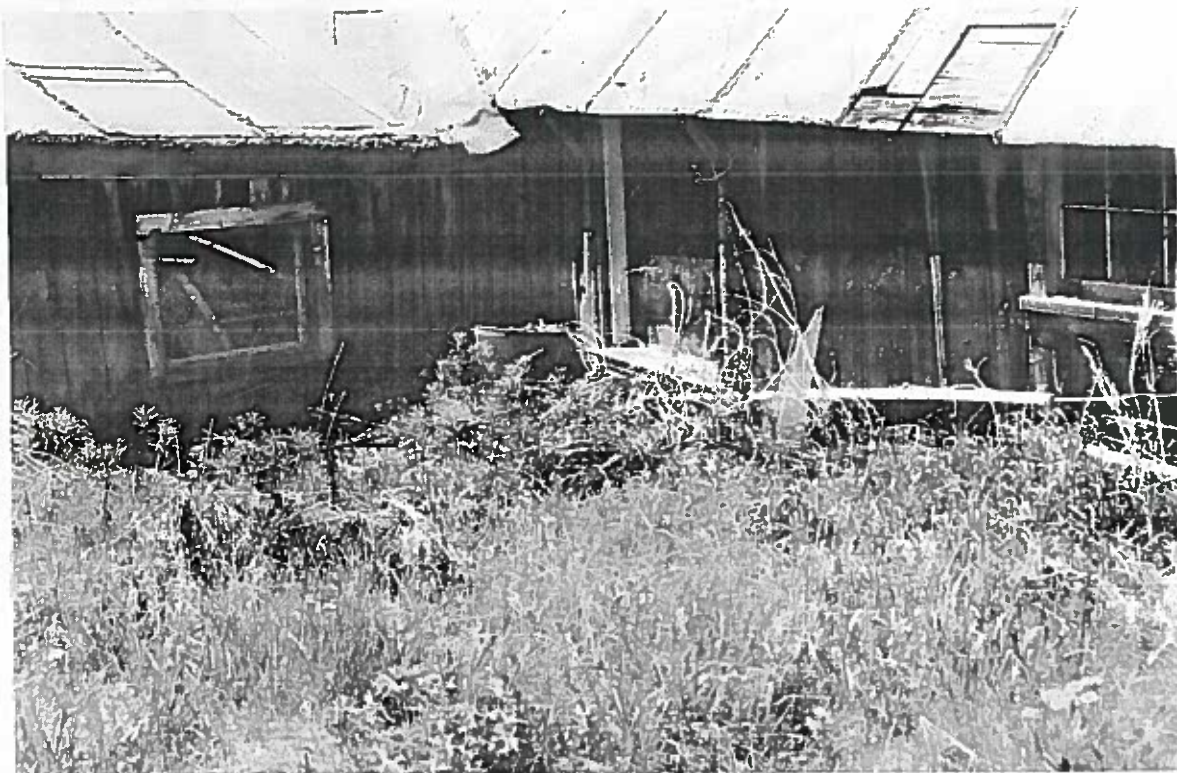
Figure 215: Looking southwest at the intersection of the frame addition and the original log building. Note the deteriorated roof sheathing and the high grade around the building.
