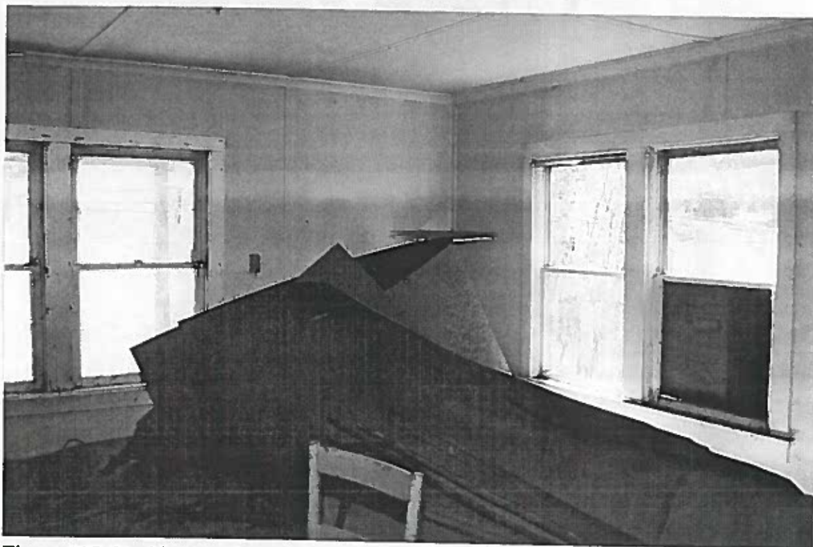
Figure 197: Looking southeast at the windows in the front room. There is some water damage along some of the sills and bottom sash of the windows as well as one piece of glass missing.
