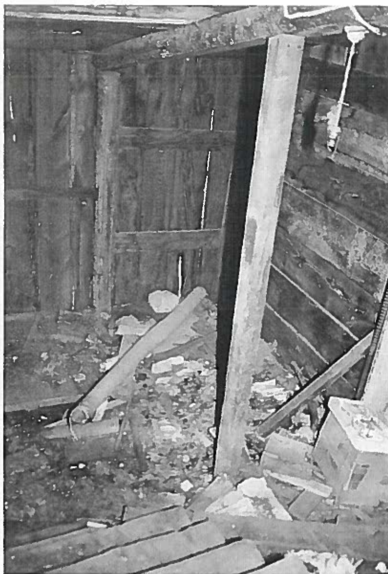
Figure 210: Looking west at the lower level of the frame addition. The wood floor is rotted out and the base of the structure is rotted. Additional posts have been added to help keep the roof intact from snow loads.
