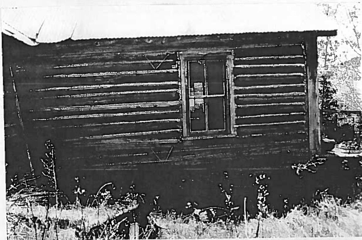
Figure 126: Looking south at the north wall of the house. The log walls and wood in the windows are weathered but in good condition. The daubing has hair line cracks but in most cases is still intact.
