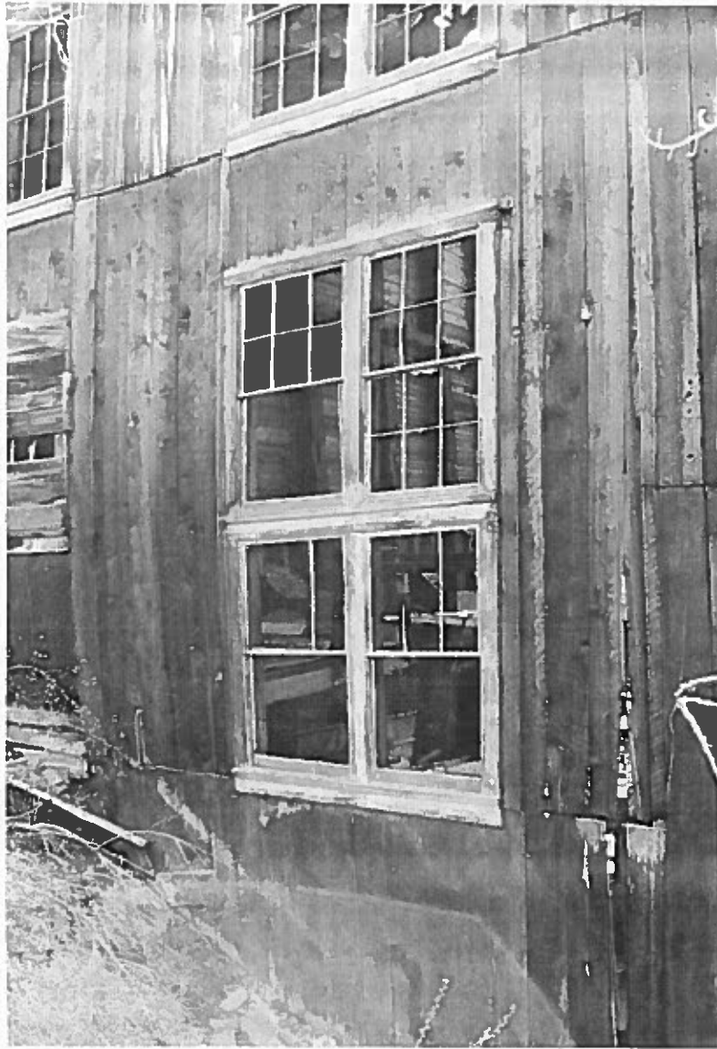
Figure 18: Looking southeast at the details of the windows on the north wall. Note the missing glass and weathered wood.
