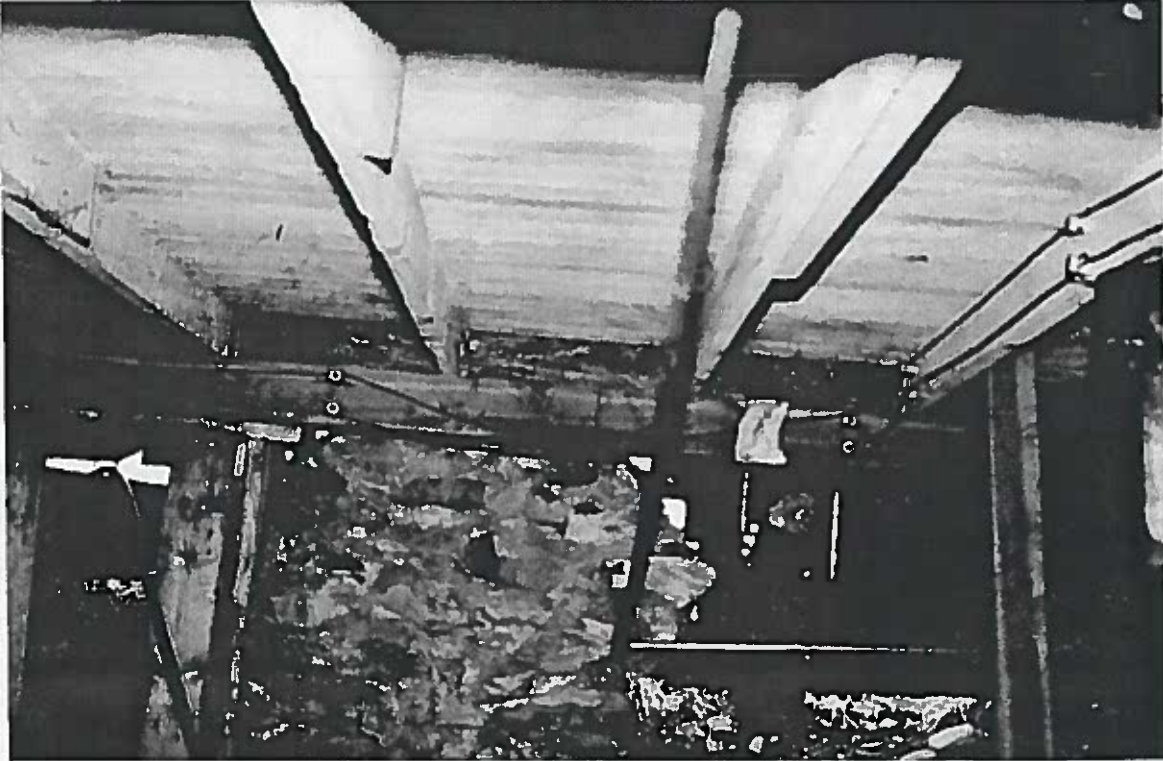
Figure 133: Looking north at the foundation and the areas where the water penetrates into the structure. Note the area to the right where the slope drains water directly into the basement.
