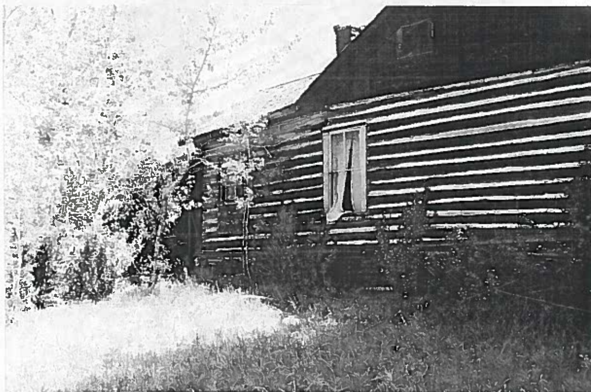
Figure 157: Looking northeast at the back of the building. The trees and shrubbery are too close to the building causing moisture buildup along the base.
