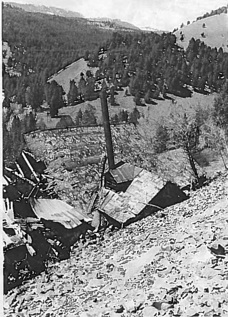
Figure 23: Looking northwest at the roof of the upper part of the Mill. Note the collapsed area around the ore bins to the left.
