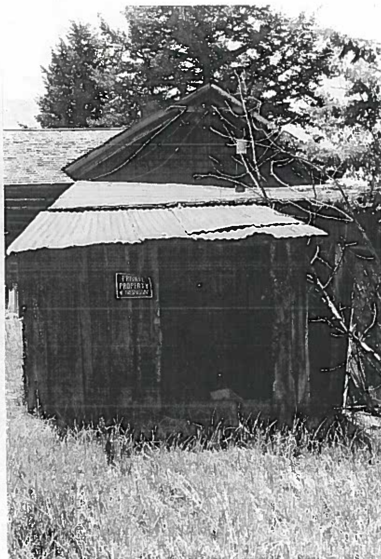
Figure 160: Looking south at the frame addition to the building. Note the wall missing and high grade around the structure.
