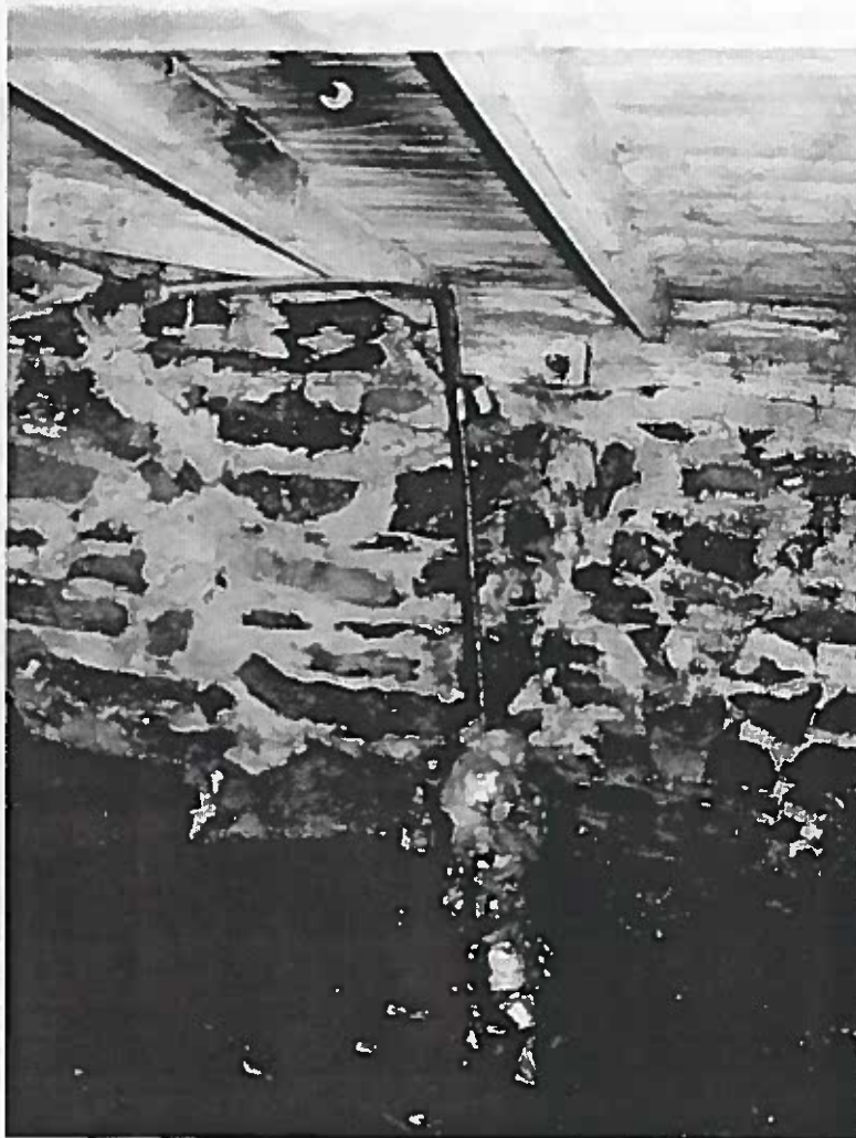
Figure 132: Looking south at the water line along the stone foundation for the fireplaces. There are some cracks in this wall due to settlement.
