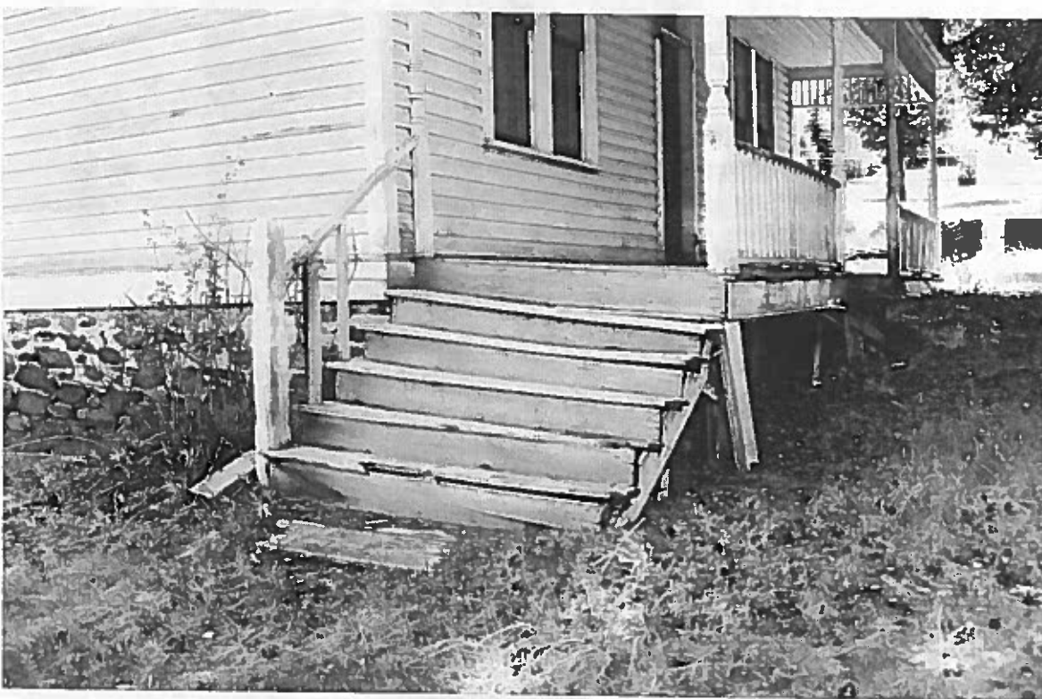
Figure 46: Looking east at the front porch and steps of the building. Note the deteriorating steps on this end of the porch. The support on the corner of the porch is also moving out.
