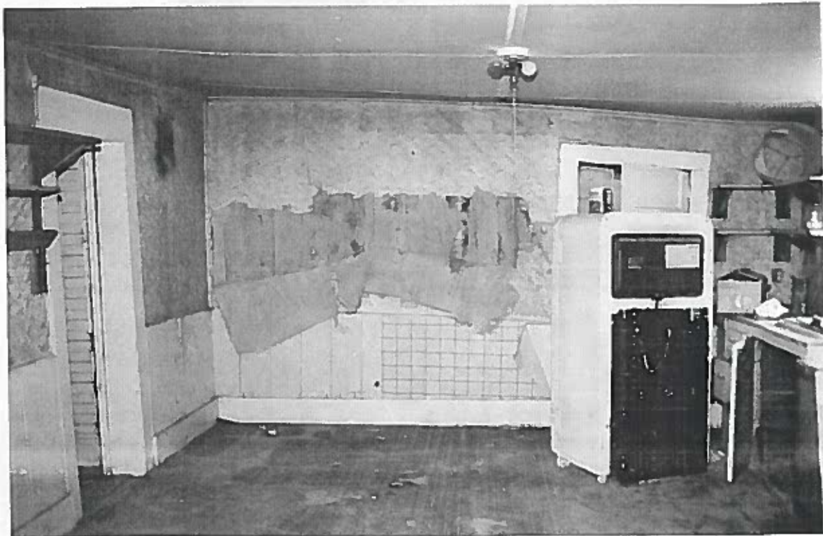
Figure 226: Looking north at the back wall of the original log building with its original layers of wall paper and newspapers. Generally the materials are in fair to good condition.
