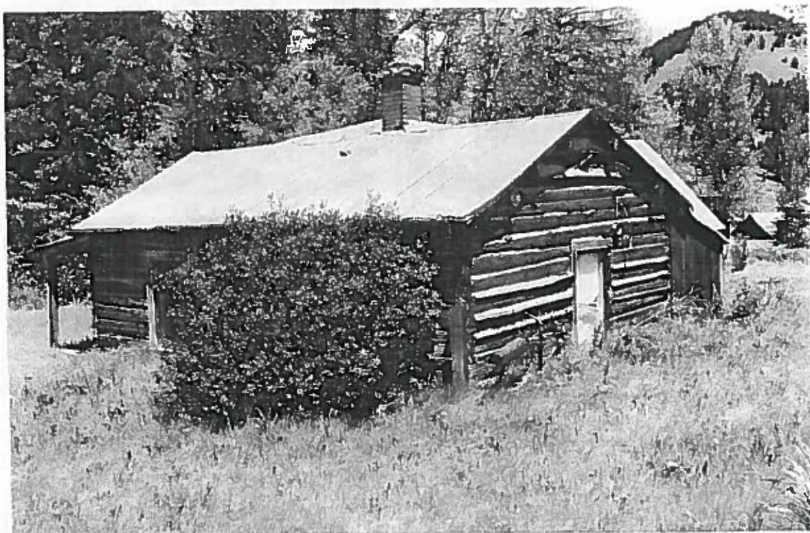
Figure 216: Looking northwest at the building. Note the high grade around this end of the building against the log work. The bottom sill log and at least one to two wall logs are deteriorated and rotted. The top of the brick chimney is also deteriorating.
