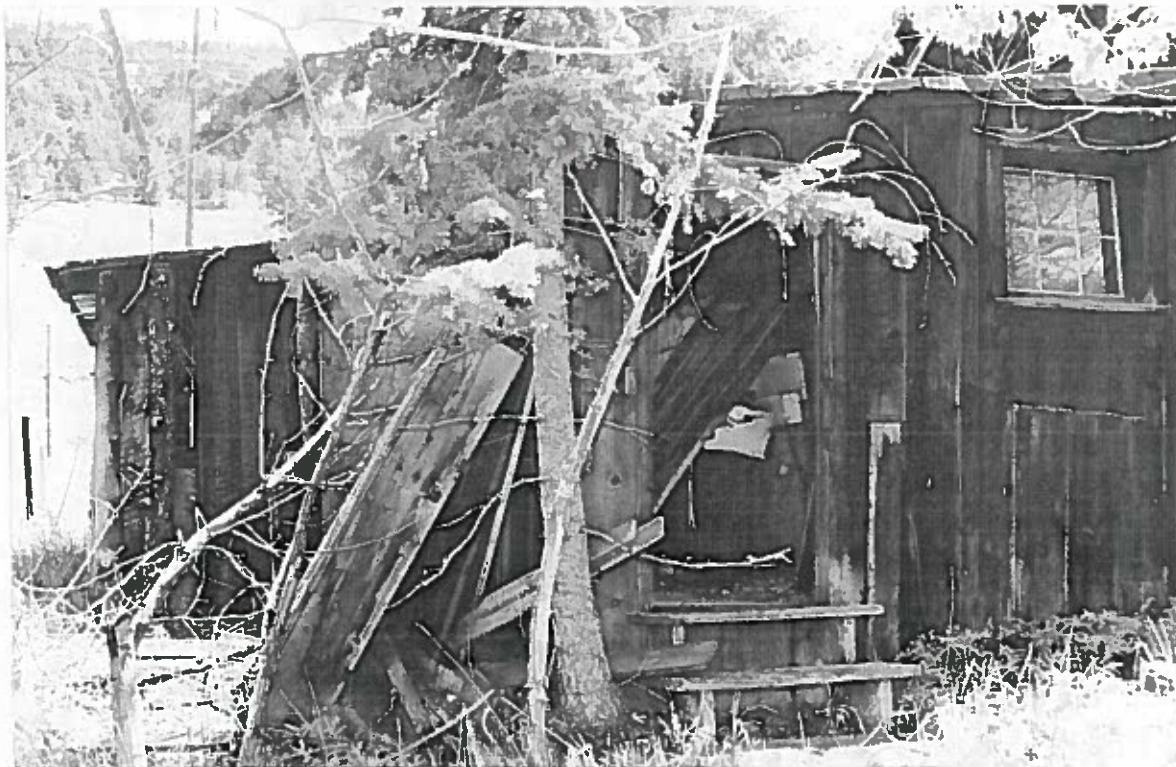
Figure 159: Looking east at the frame addition to the building. Note the collapsed area, missing walls and doors and settlement in the structure.
