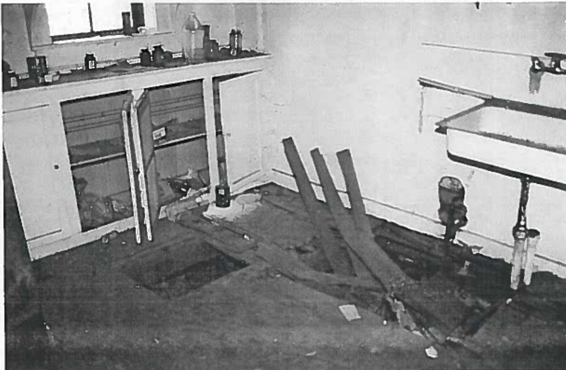
Figure 173: Looking northwest at the kitchen. Note the holes in floor where the wood has been cut out.
