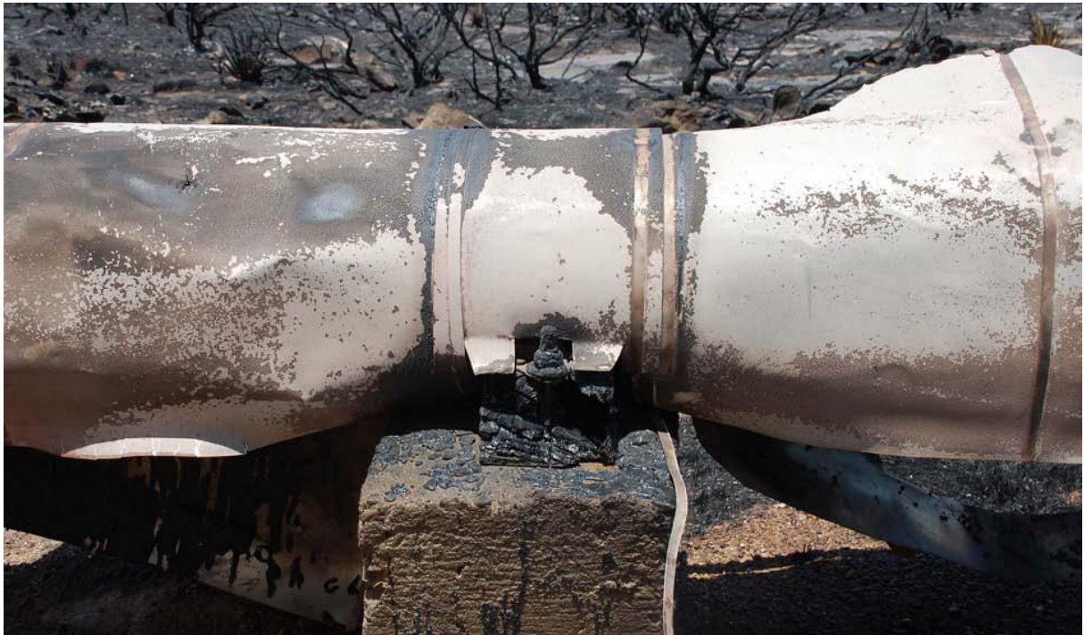
A section of the park's 8" surface-constructed water main showing charred pipe support blocking and lost restraint strap with exposed insulation underneath.
