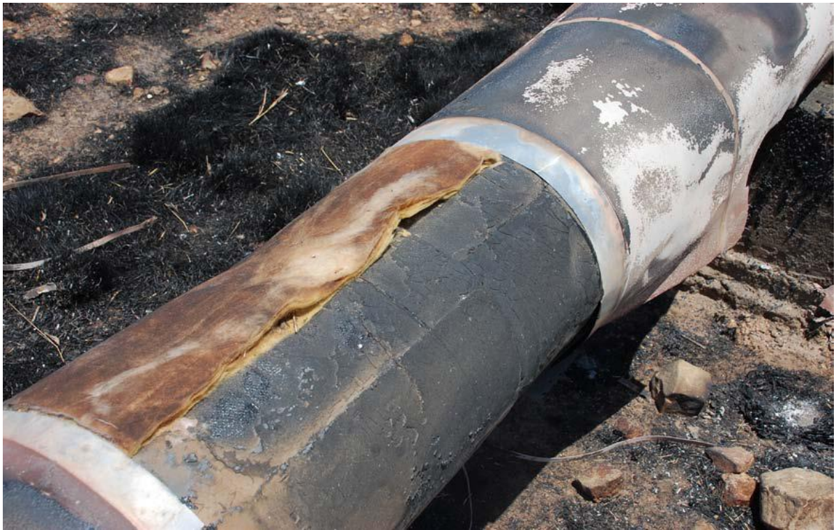
A section of the park's 8" surface-constructed water main showing exposed friable asbestos.
