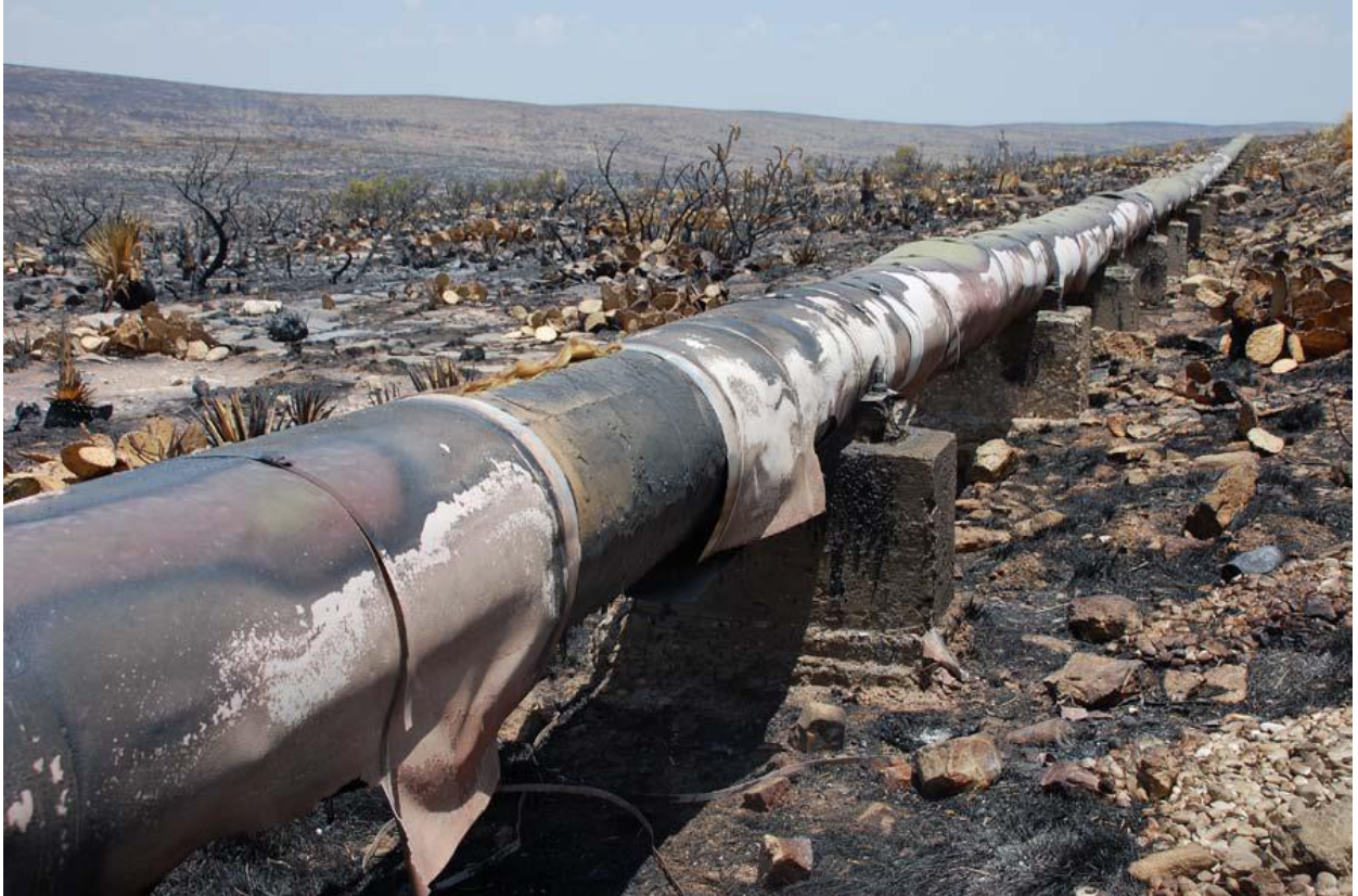
A section of the park's 8" surface-constructed water main showing melted insulation covering and strap
