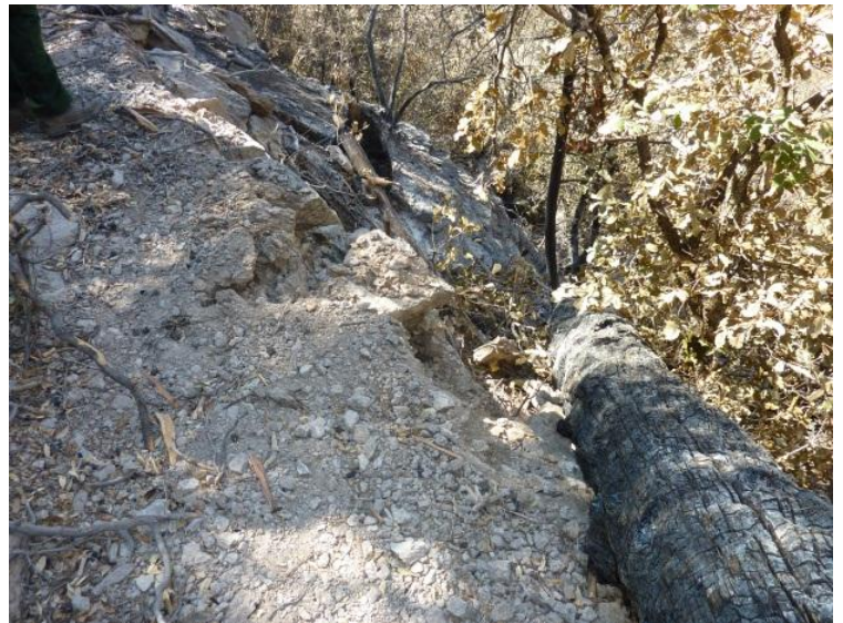
Damaged rock retaining wall on Mushroom Trail
