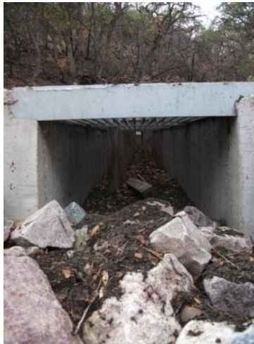
Debris/sediment in grate of 3 rd Low Water Crossing
