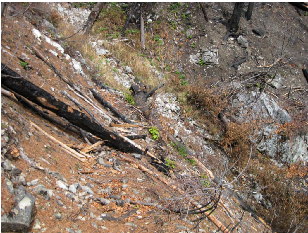
Photo 7. Boulder Creek trail with windfall, rockfall, and tread damage
