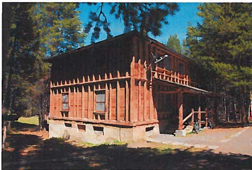
Figure 21: Looking northeast at the building. The roof is in fair condition and is winter-kept during the heavy snow loads. Note the poor drainage and grade at the corner.
