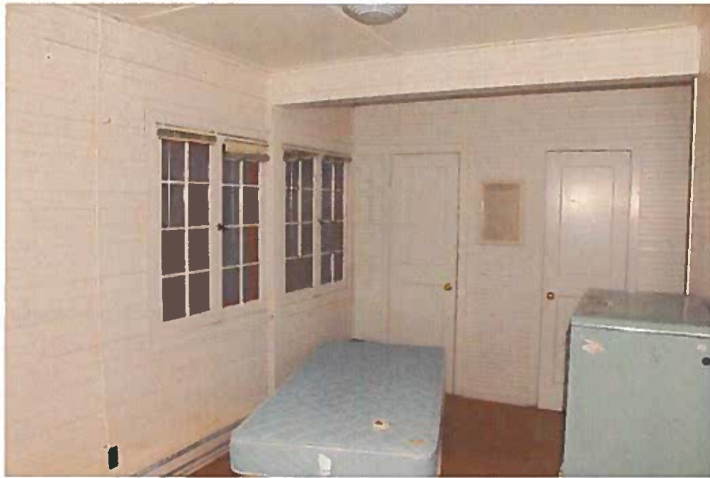
Figure 90: The windows have some missing muntins with some larger glass pieces installed in the larger opening.
