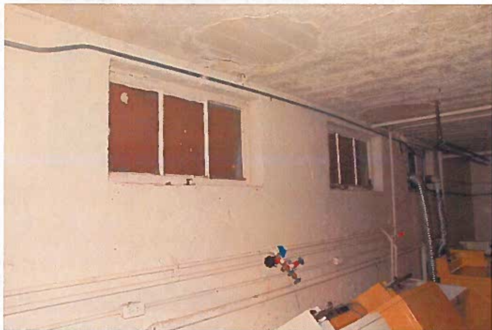
Figure 37: The steel sash windows are in fair condition with some loss of paint and some deteriorating putty.
