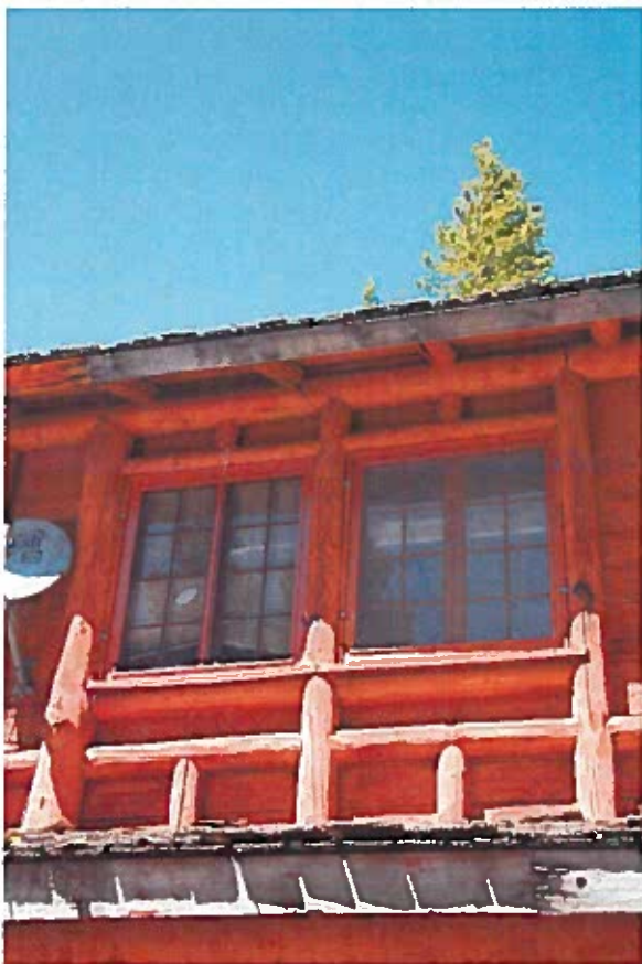
Figure 28: Looking north at a typical window above the porch roof. Water penetrates into the area below the window. Note the weathered fascia.
