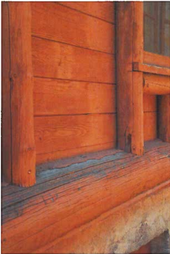
Figure 29: Looking northeast at a typical sill log on the front of the building. Note rot in the base of the columns, the weathered log, and dry wood sheathing.
