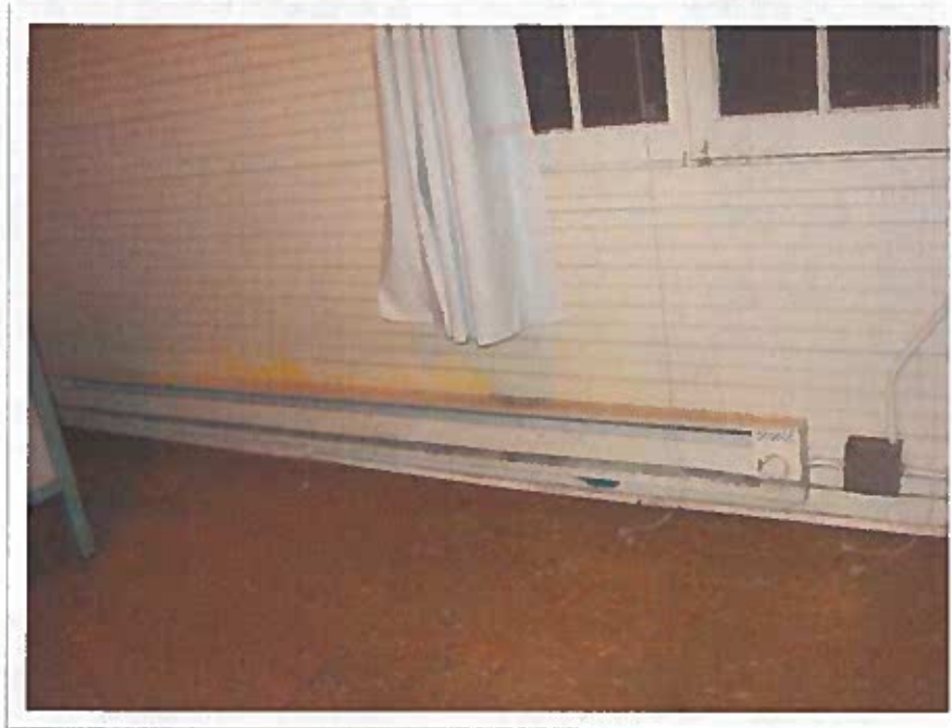
Typical Electric Baseboard Heat
