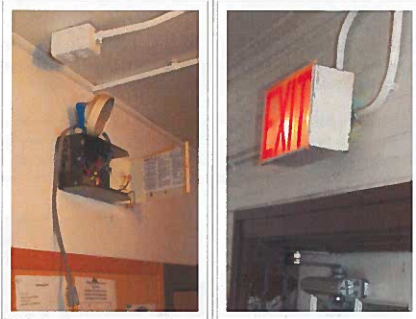
Emergency Lighting Unit (left)
