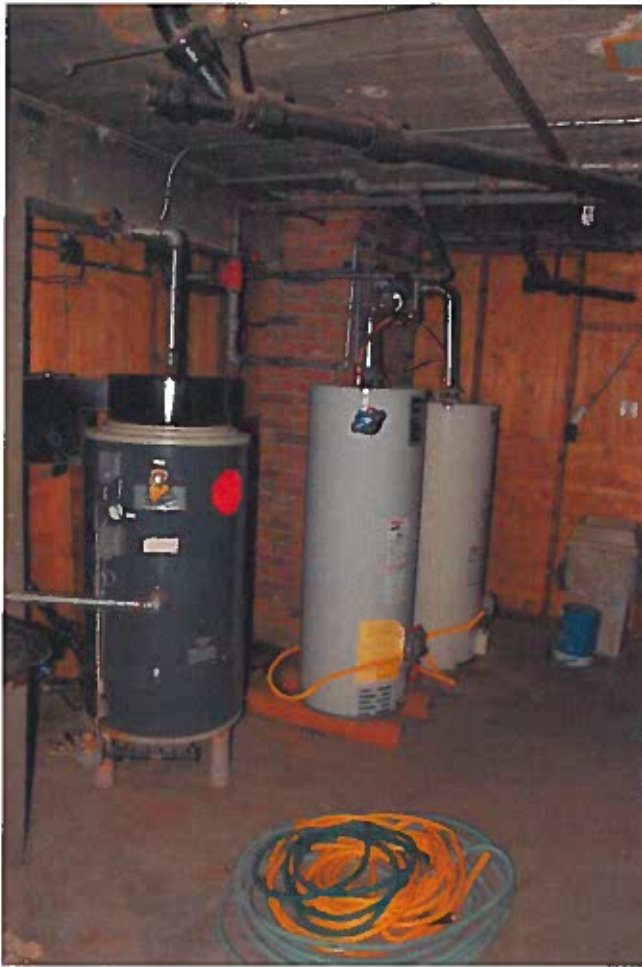
Figure 42: Note the domestic hot water heaters. The piping and electrical conduit is not well organized.
