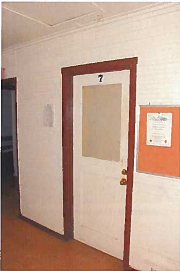
Figure 78: Typical wood paneled door with half-glass lite covered over from the room side.
