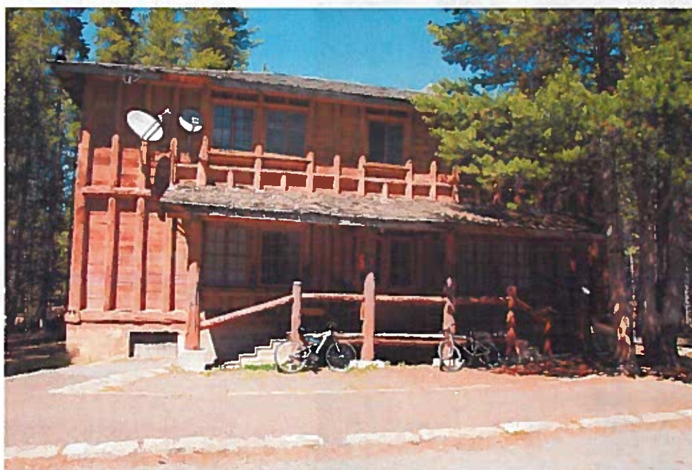
Figure 22: Looking north at the porch at the front of the building and porch railing. Part of the railing has deteriorated and has been removed.
