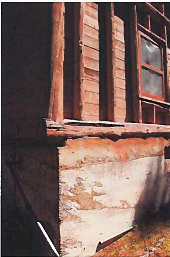
Figure 20: Looking southeast at the concrete foundation. There are some minor horizontal cracks in the foundation wall. Also note the rotted sill log.
