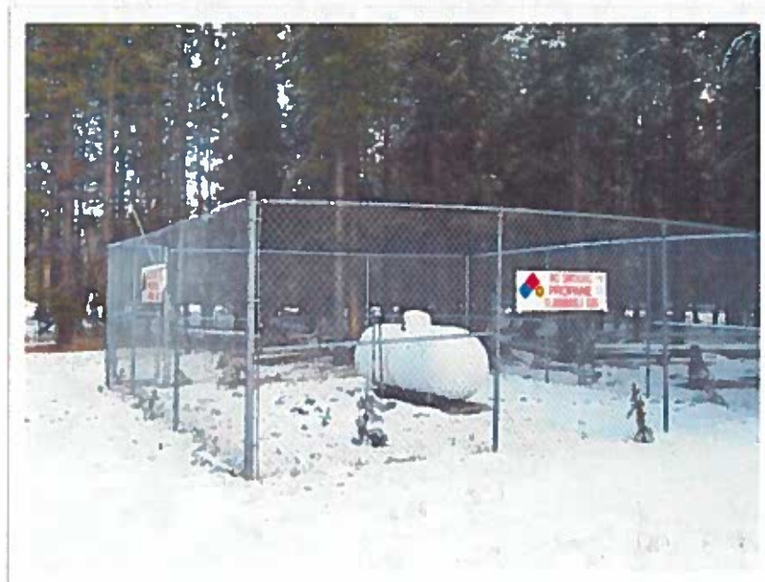
Propane Tank Servicing Facility
