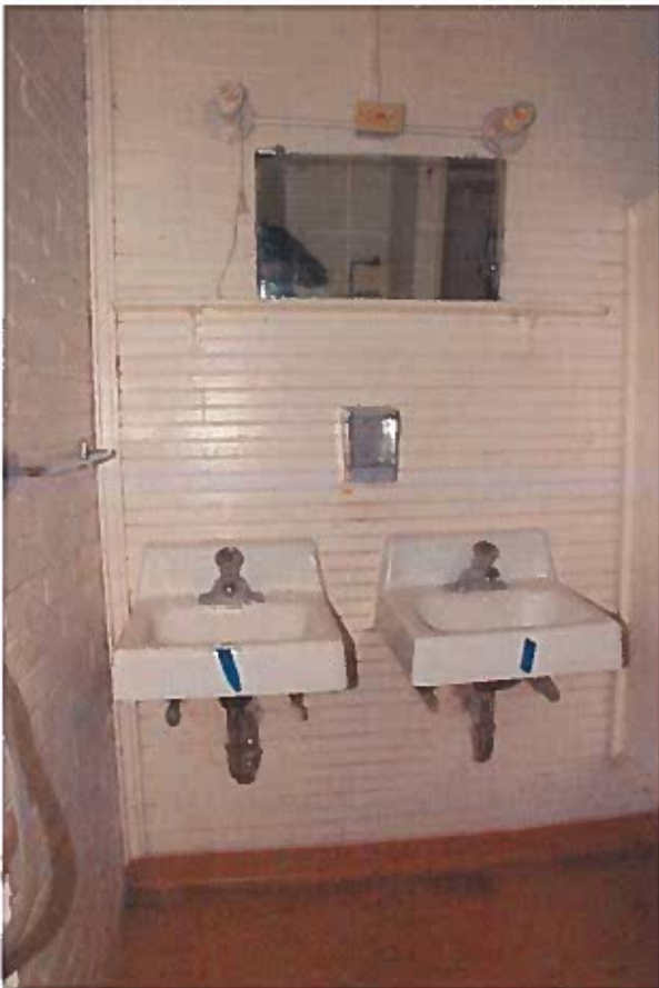
Figure 48: The bathroom fixtures are in fair condition. The bathroom needs to be redesigned to meet ADA requirements and to make it more usable.
