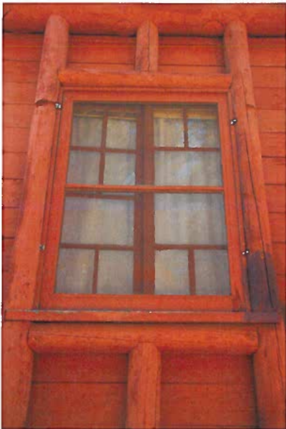
Figure 16: Looking west at a typical window and details of some of the logs. Note the weathered surfaces and some rot in the base of the columns and the weathered wood on the window, and also the missing muntins in the sash.
