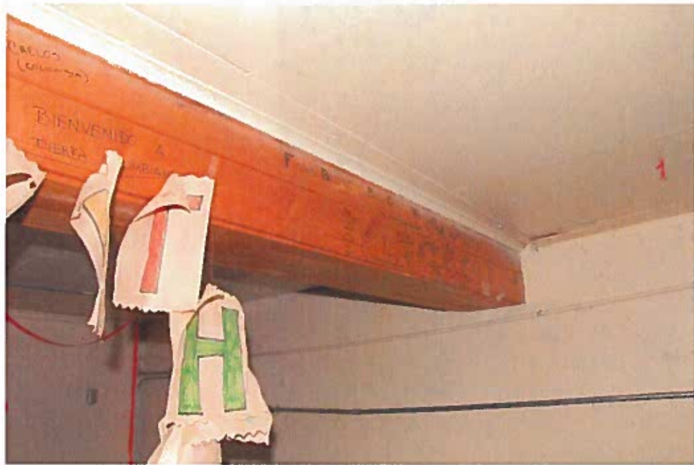
Figure 44: Concrete beam wrapped in wood.
