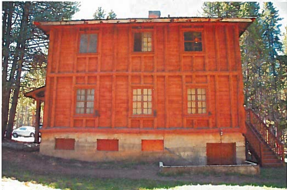
Figure 14: Looking west at log and wood sheathing that is dry and weathered. The windows have some broken panes.
