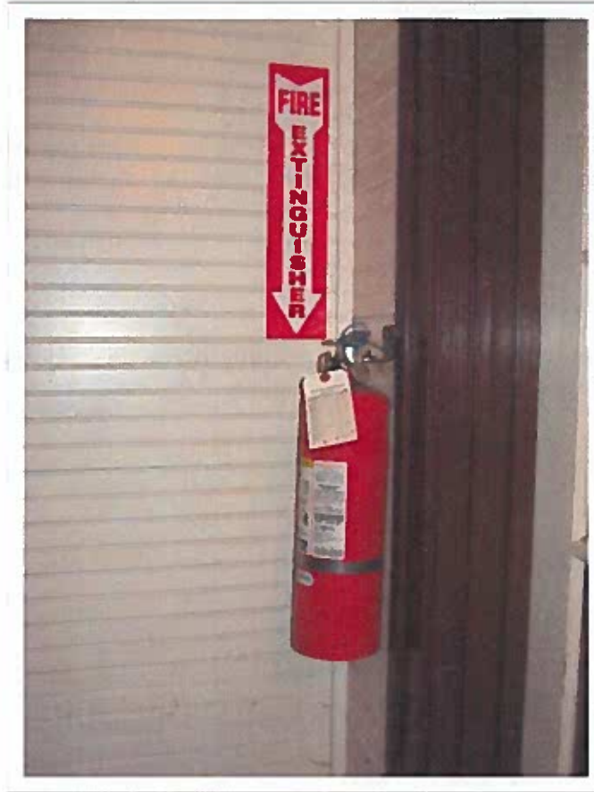
Typical Fire Extinguisher
