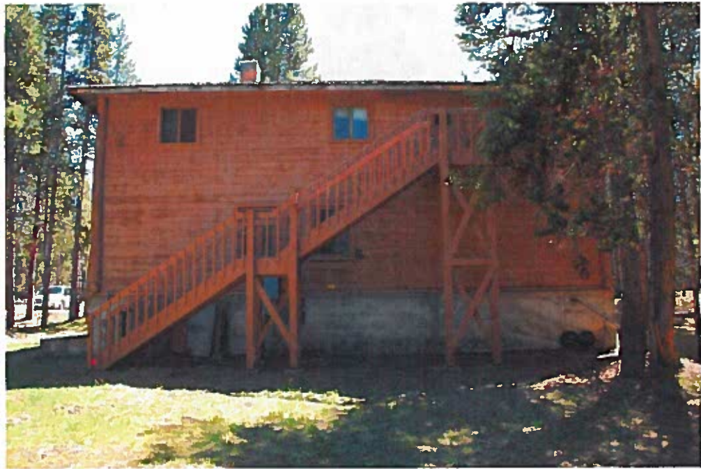
Figure 17: Looking south at the building. The stair on the back of the building is in good condition, but there are code problems with the railing. The wood sheathing on this wall is weathered.
