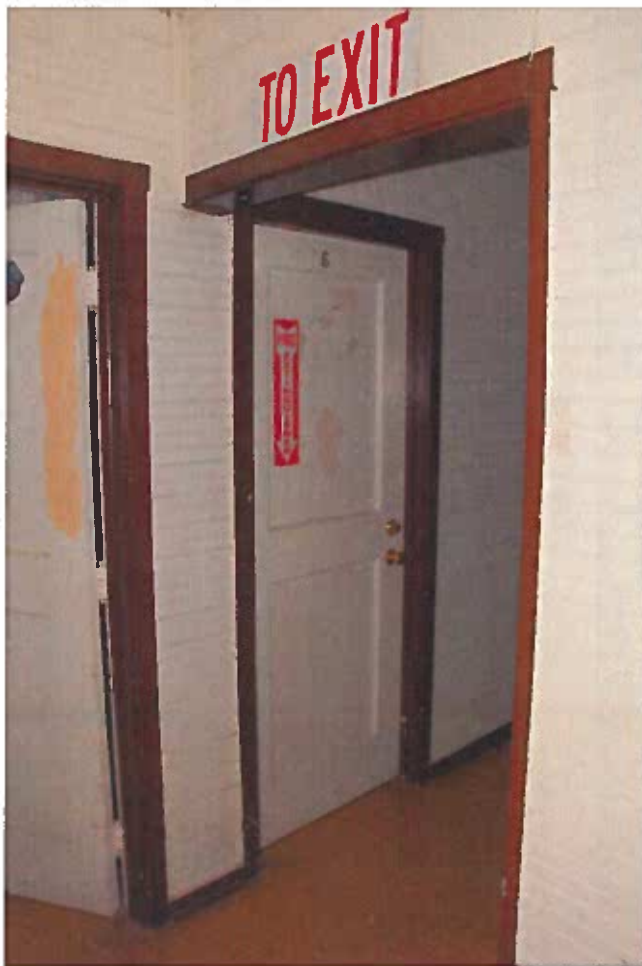
Figure 74: Typical wood paneled doors with a half lite. This door does not meet code in the fire corridor without a fire suppression system.
