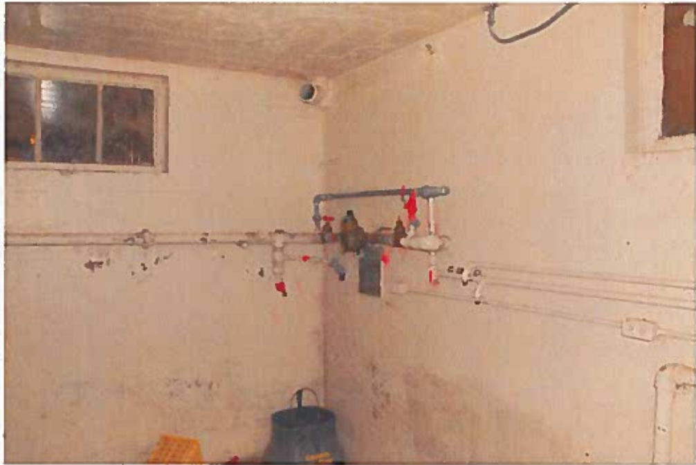
Figure 40: Water meter for the building. The plumbing appears to be in fair condition.
