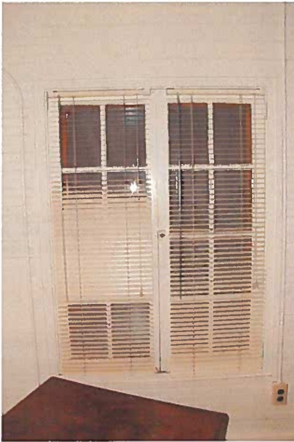
Figure 61: Generally the windows are in fair to good condition on the inside. They will have to be evaluated totally in the future.
