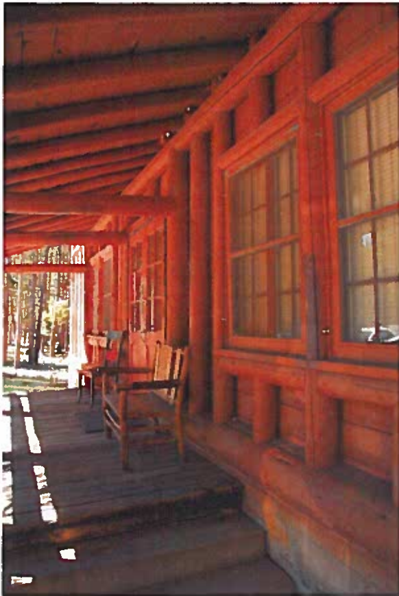
Figure 27: Looking northwest at the front porch and entrance. The porch roof has some deteriorated areas at the connection to the wall. Water penetrates into the horizontal logs causing some rot.
