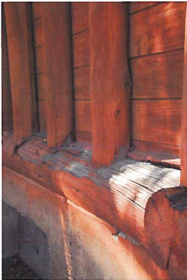
Figure 18: Looking west at a typical base log on the building. Note the weathered and cracked log. The mortar cap is loose and coming apart.
