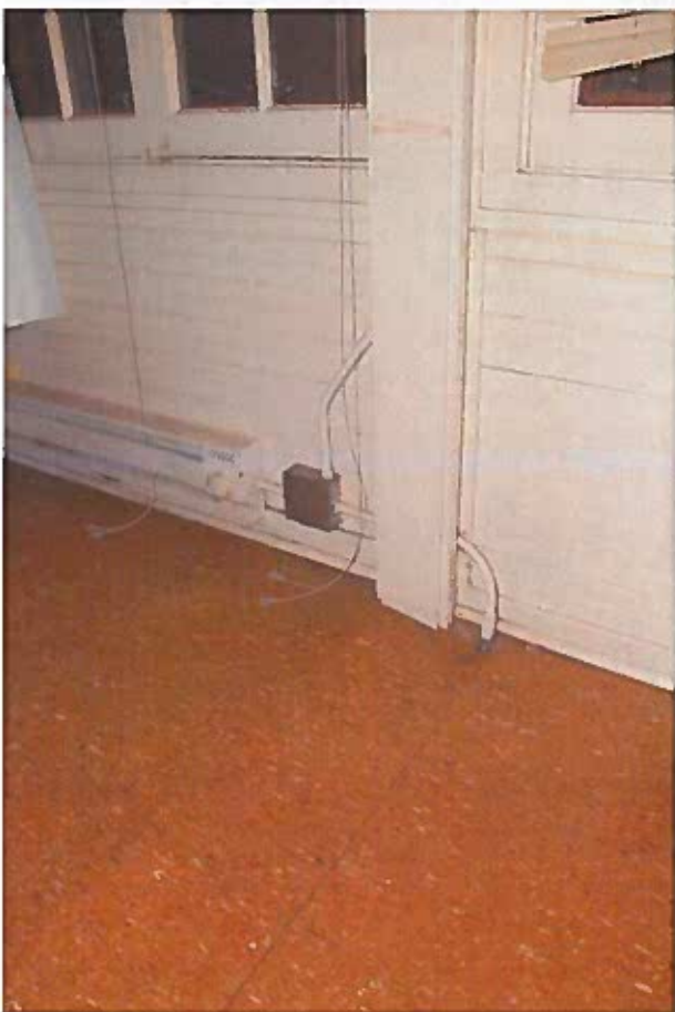
Figure 52: Note the wear on the lower part of the walls and at the base. There is some missing paint and deteriorated wood members.
