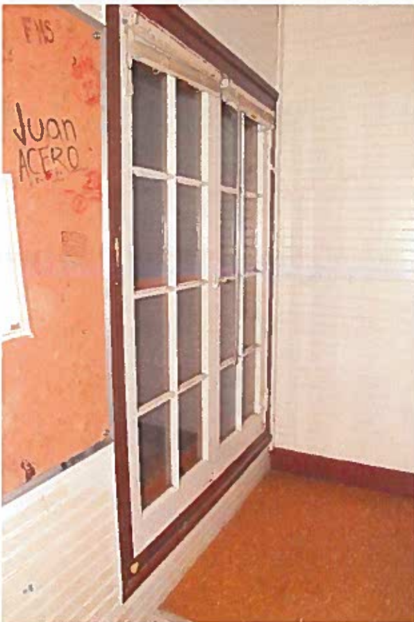
Figure 65: The hinged window appears to be in good condition on the landing but causes problems with stair for exiting.
