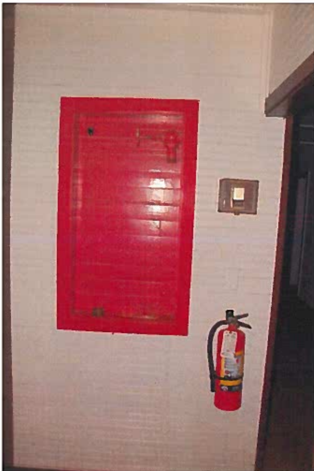
Figure 77: Fire hose cabinet and fire extinguisher.
