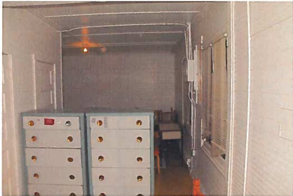
Figure 55: Note the closet doors to the left with original wood paneled doors and the wood bead board on the outer walls and ceiling. The light fixtures are poor and not very energy efficient.
