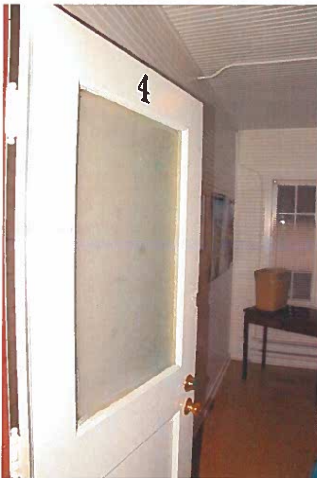
Figure 60: A typical original door on the first floor. Note the original hinges that are in good condition although loose in some cases.
