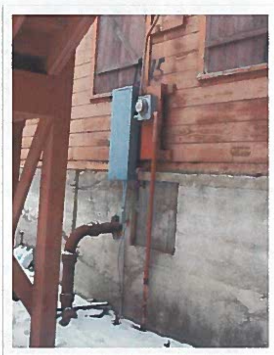
Exterior-Mounted Electrical Service
