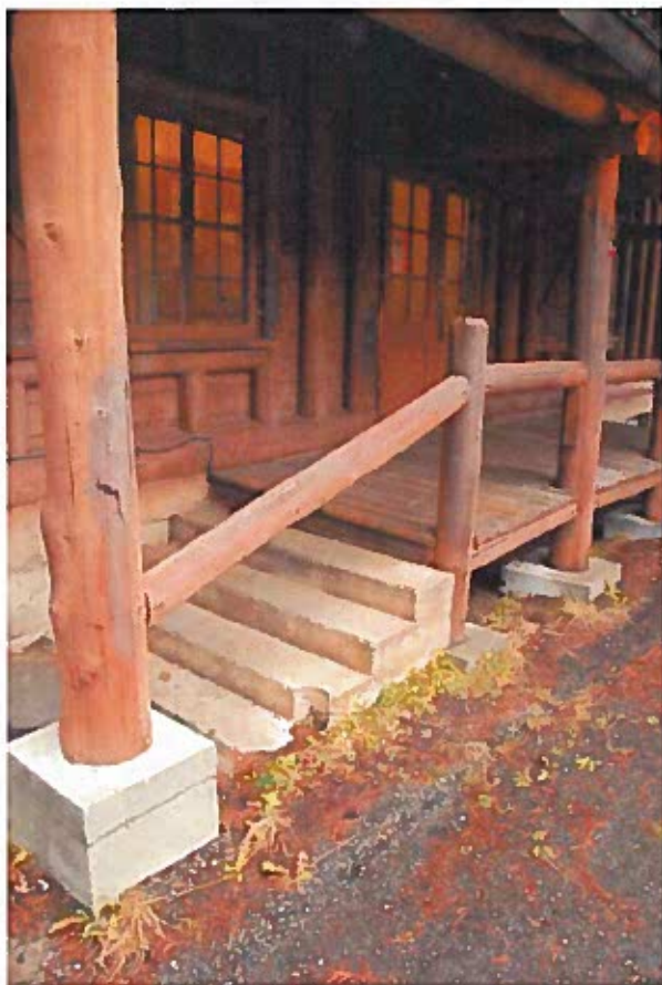
Figure 23: Looking northeast at the front porch. Note the variable heights in the risers of the steps and landing. The deck is in poor condition.
