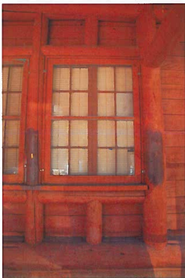
Figure 24: Looking north at a typical window next to the doorway. It is in fair condition but shows signs of weathering and some minor rot.
