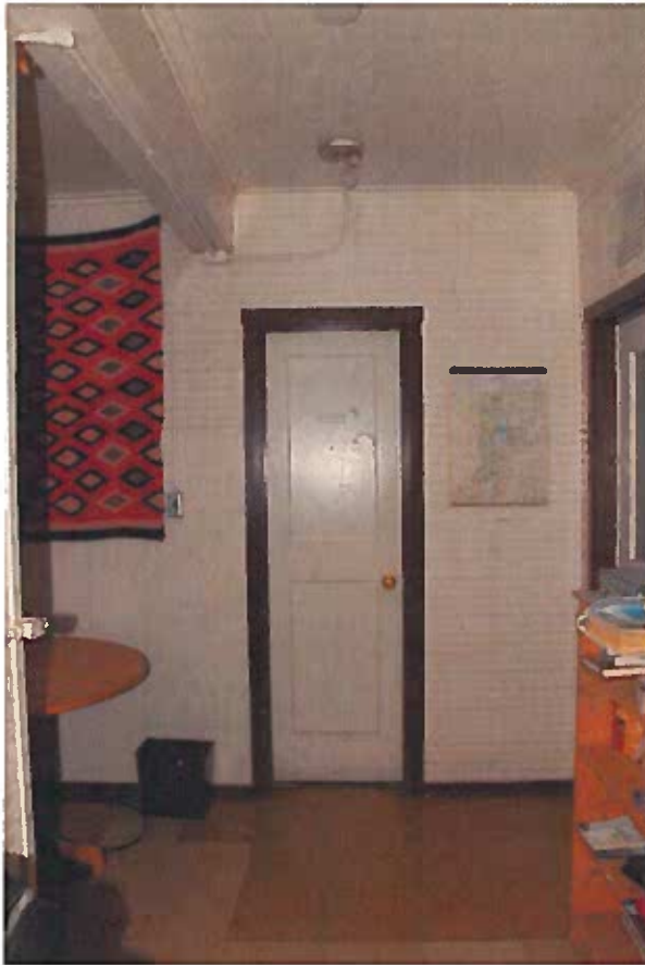
Figure 47: The original wood paneled door does not meet the width for ADA access to the bathroom.
