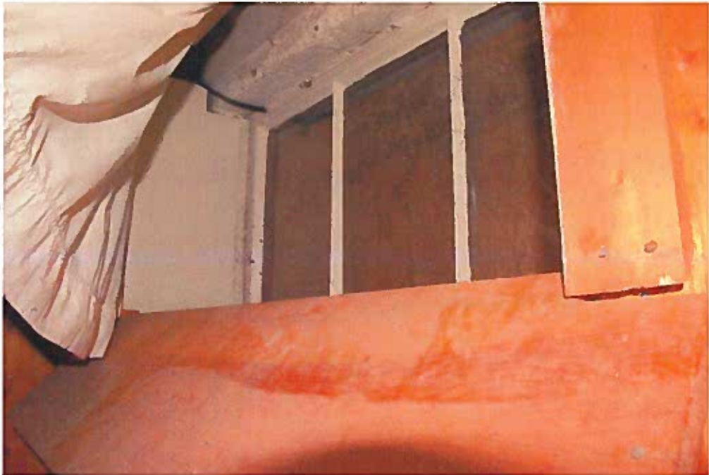
Figure 35: The steel sash windows are in fair condition with some loss of paint and deteriorating putty. There is some water leaking around the frame.
