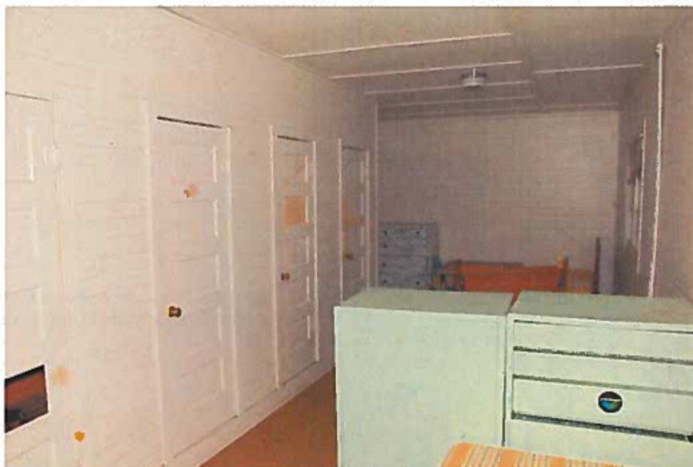
Figure 82: Note the missing panel in the door to the left. All of these doors access storage closets.
