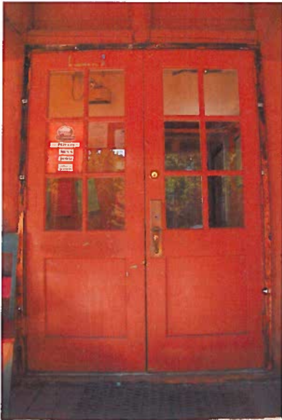
Figure 25: Looking north at the entrance. The wood paneled doors with lites are in poor to fair condition. The hinges are loose and the meeting styles have some wood damage. The doors do not close properly.
