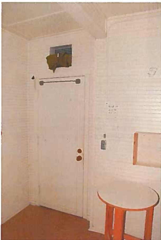
Figure 51: The wood paneled doors do not meet fire codes without a fire suppression system in the building. The ventilation screen also does not meet code.
