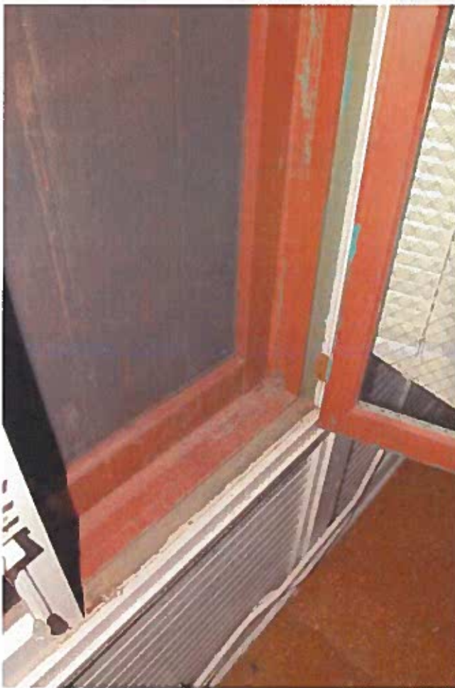
Figure 56: From the inside note some of the weathering of the windows. There is missing paint and some deterioration in the wood sills.
