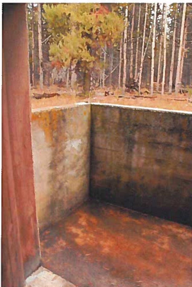
Figure 31: Looking east at the retaining wall with stair to the basement. The concrete along the outside stair is deteriorated and spalling.
