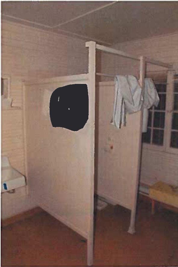
Figure 92: The partitions are in poor condition.
