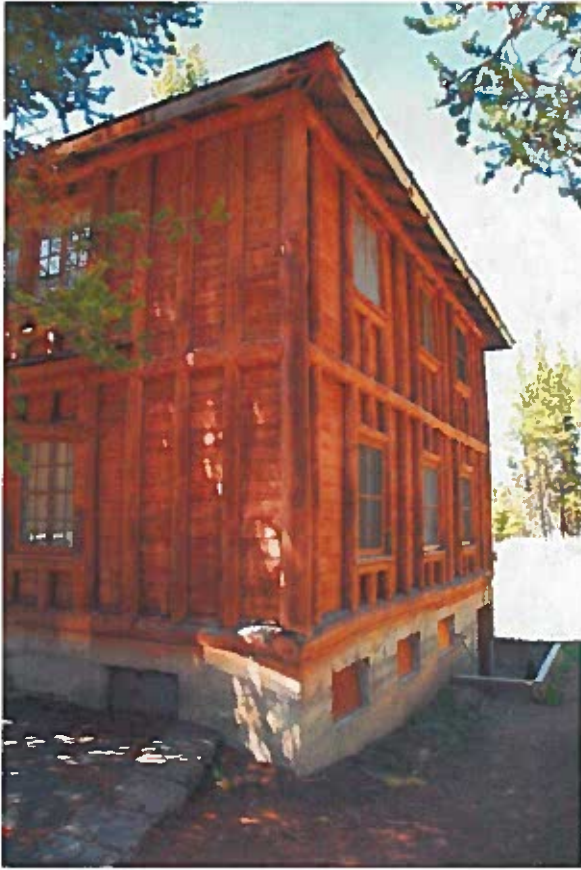
Figure 15: Looking northwest at the building and concrete stair to the basement. The stair does not meet code and there is some deterioration in the concrete walls.
