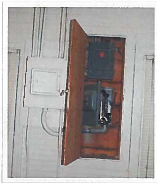
Load Centers on Main Level
