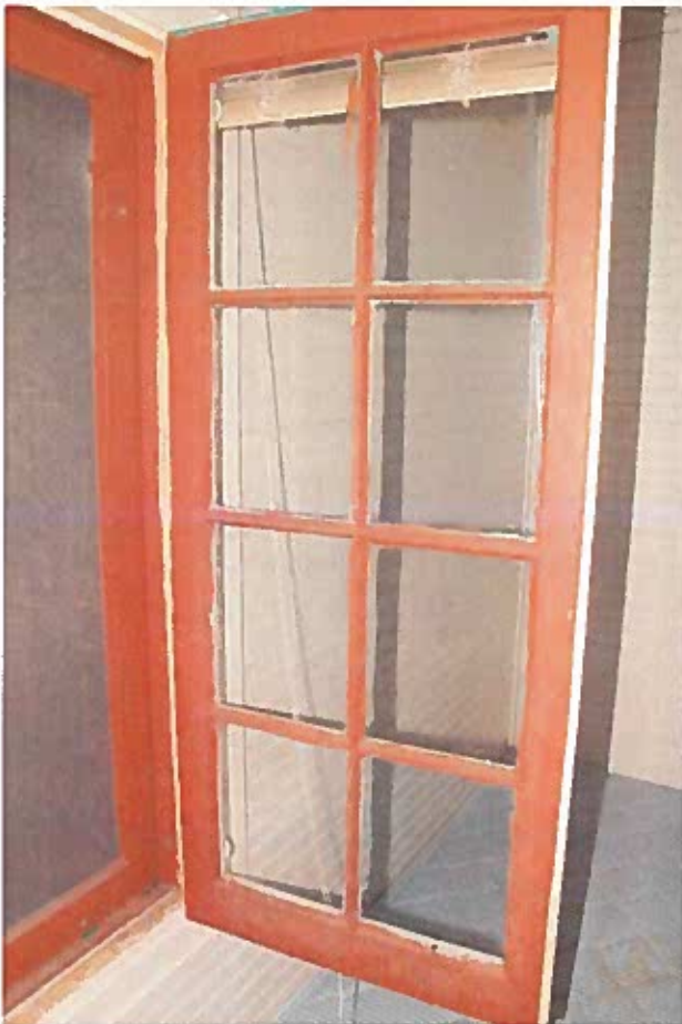
Figure 91: The window exterior shows some weathering, peeling paint and deteriorating window putty.
