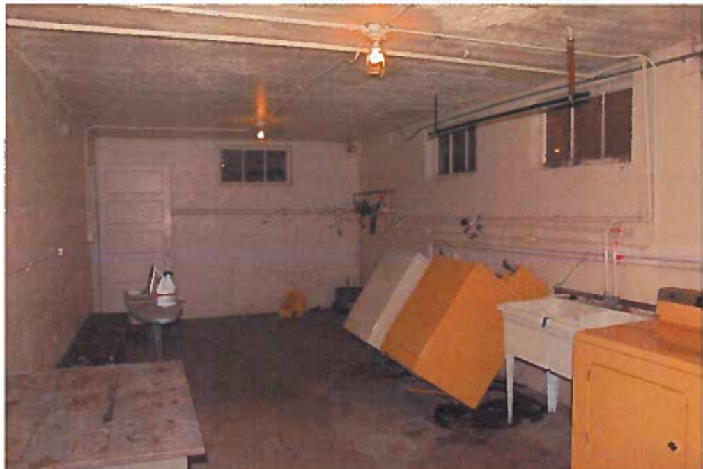
Figure 39: The laundry room has concrete walls and floor. There is some staining on the walls from the windows and from areas above.
