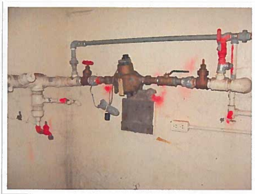
2" Domestic Water Service
