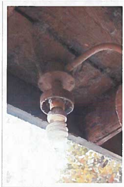
Light Fixture with Missing Globe
