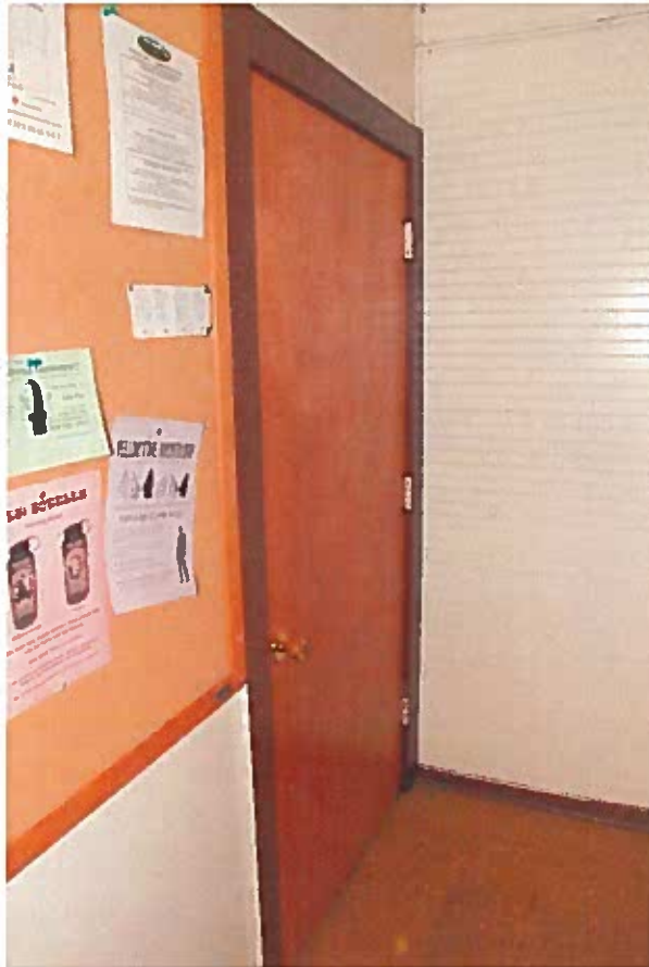
Figure 45: The interior first floor door swings into the exit corridor from the second floor.
