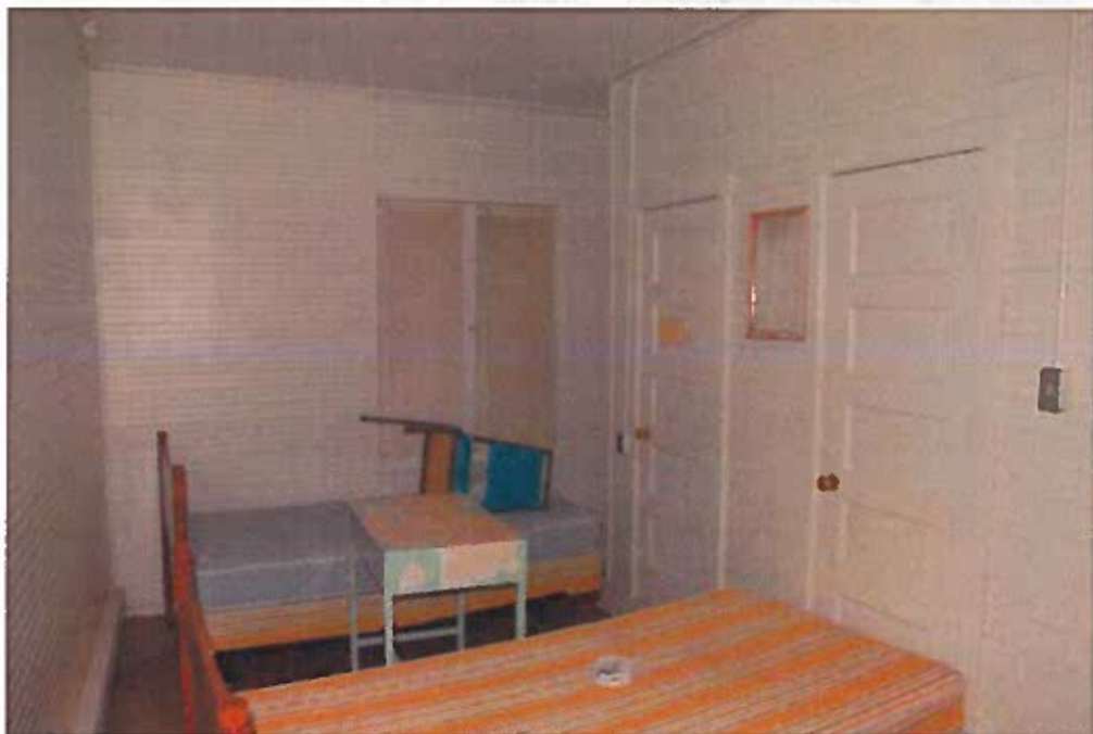
Figure 54: This room is used by several tenants and has a lot of wear on the walls and floor surfaces.
