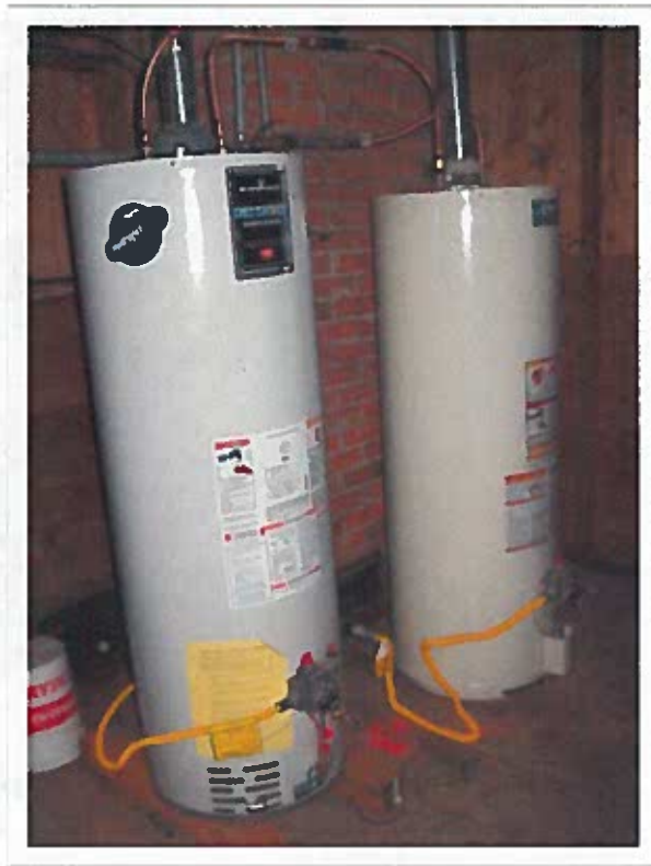
Domestic Hot Water Heaters
