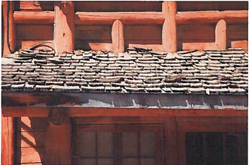
Figure 26: Looking north at the porch roof. The wood shingles are loose and missing. Note the weathered fascia.
