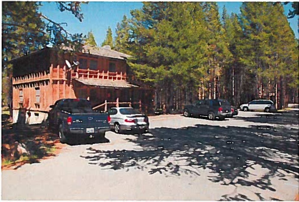
Figure 13: Looking northeast at the Dormitory. The logout walls and sheathing are dry and have some deterioration.
