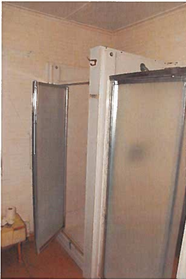
Figure 94: The bathroom showers with some mold and worn areas on the walls and door.
