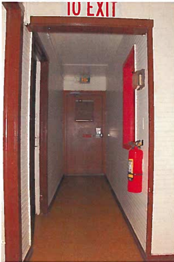
Figure 68: Note the second exit from the second floor. However the entrance to the stair corridor is too close to the main exit stair.
