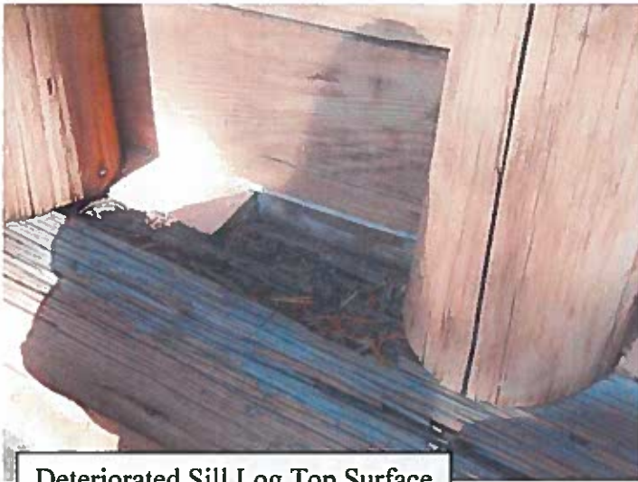
Deteriorated Sill Log Top Surface
