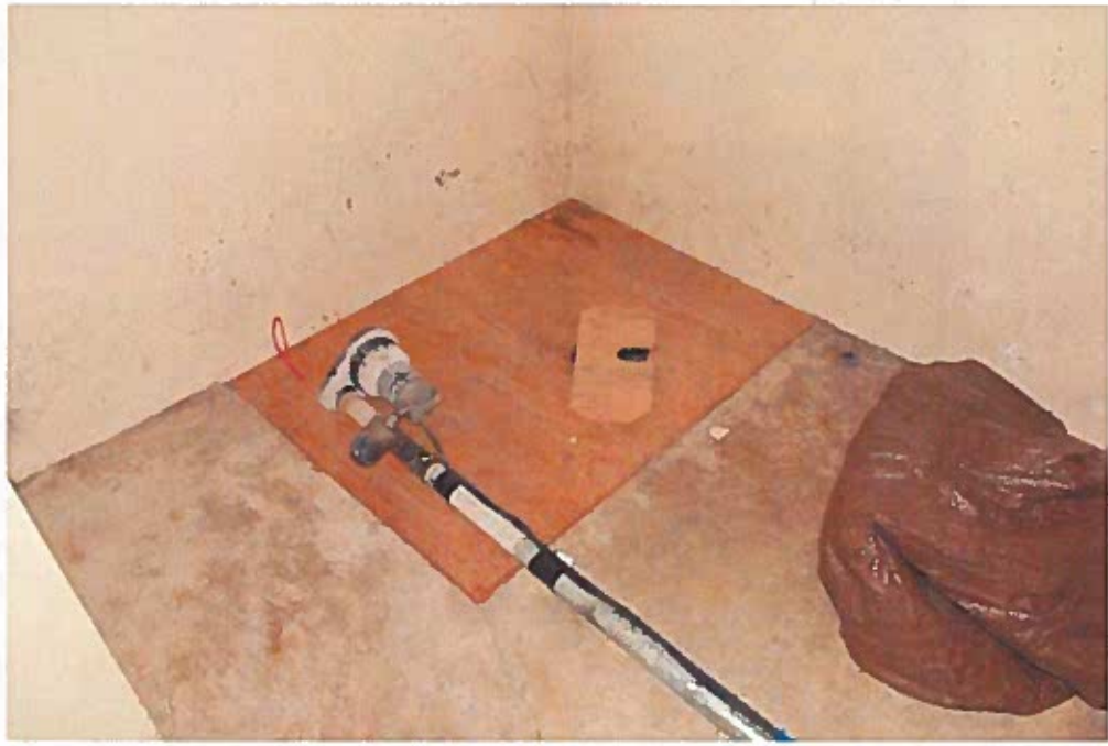
Figure 38: A sump pump is used to pull water out of the room during backup in the drainage systems in the laundry room.
