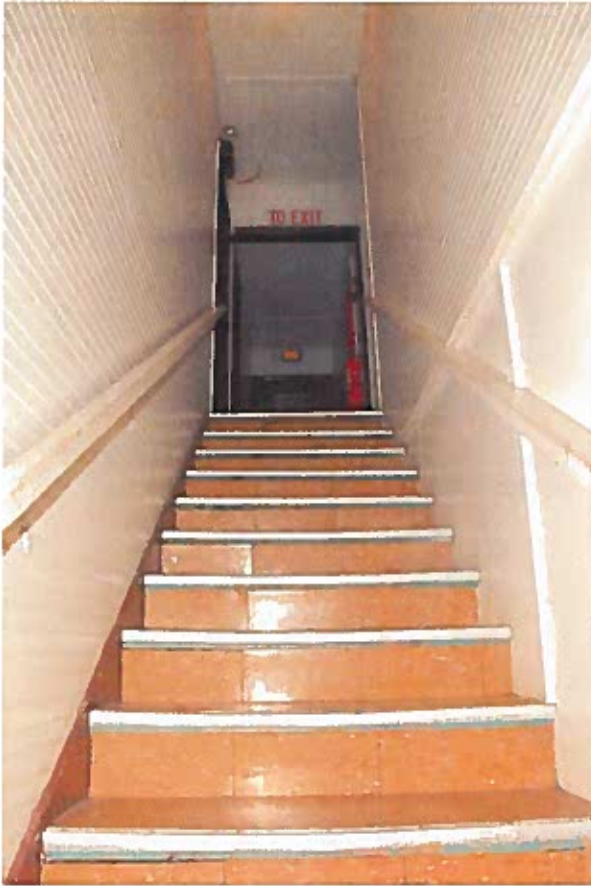
Figure 66: The stair is steep and the railings and lighting are poor.
