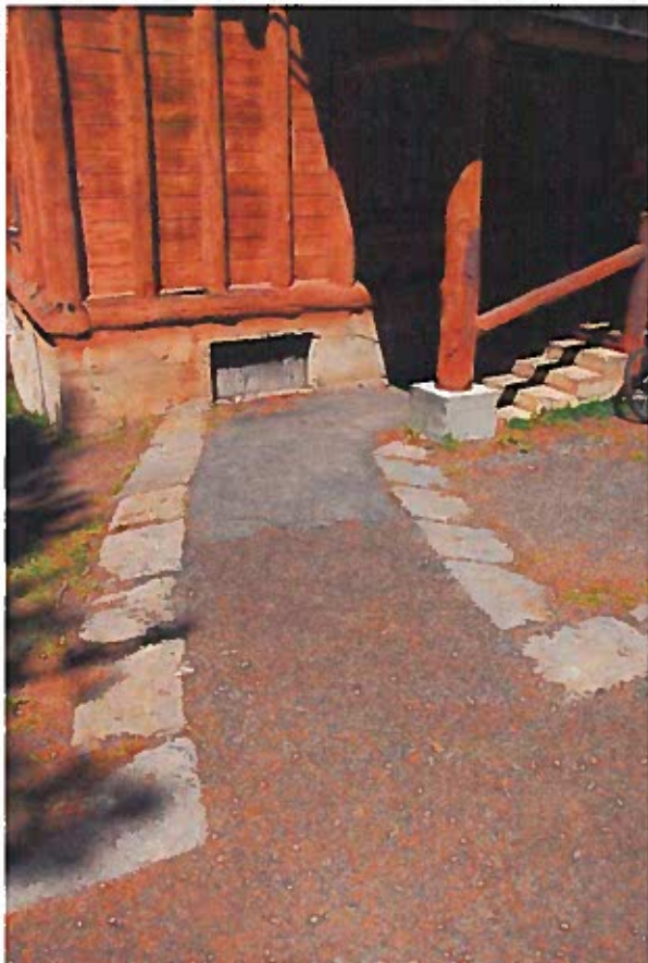
Figure 11: Looking north at the walkway to the building. Note the drainage towards the building and front steps.
