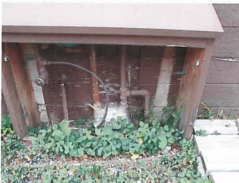
GAS METER AND CONNECTION - EAST WALL OF THE EXTERIOR OF THE STRUCTURE.
