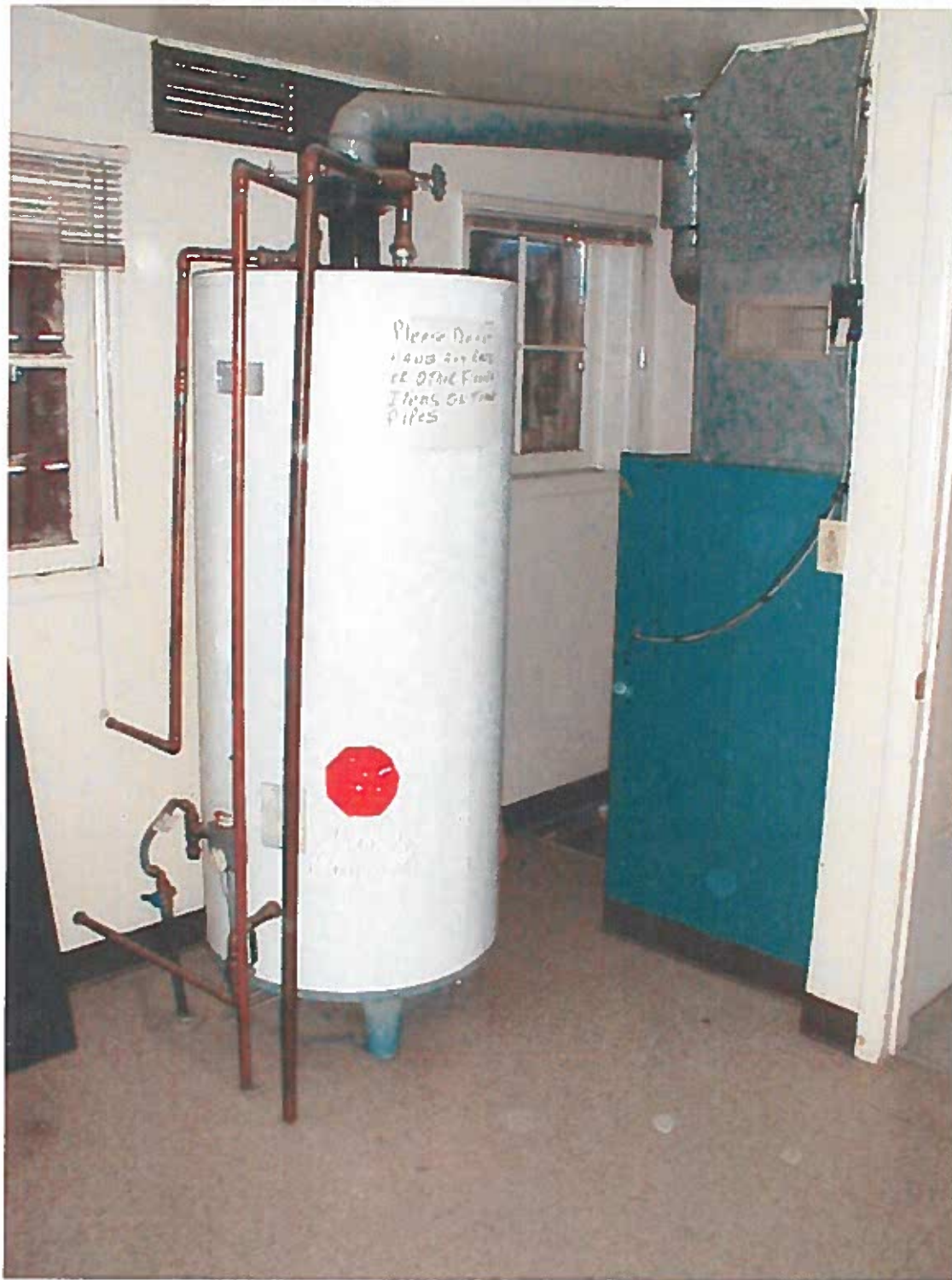
FIRST FLOOR MECHANICAL/UTILITY ROOM - LOCATED IN THE DORMITORY WING
