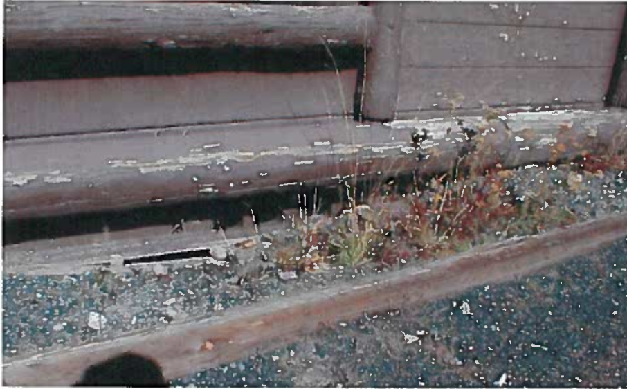
NEGATIVE DRAINAGE - SE PORTION OF STRUCTURE
