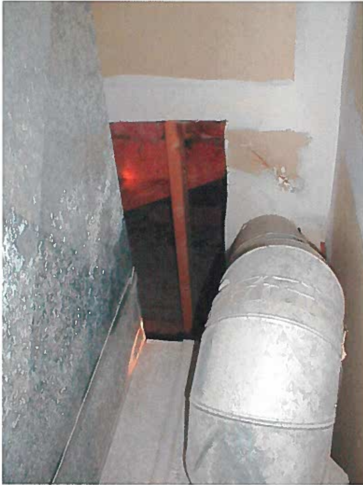
DUCTWORK FROM THE SECOND FLOOR MECHANICAL ROOM - ACCESS IS SINTO THE ROOF STRUCTURE OF THE SW ADDITION.
