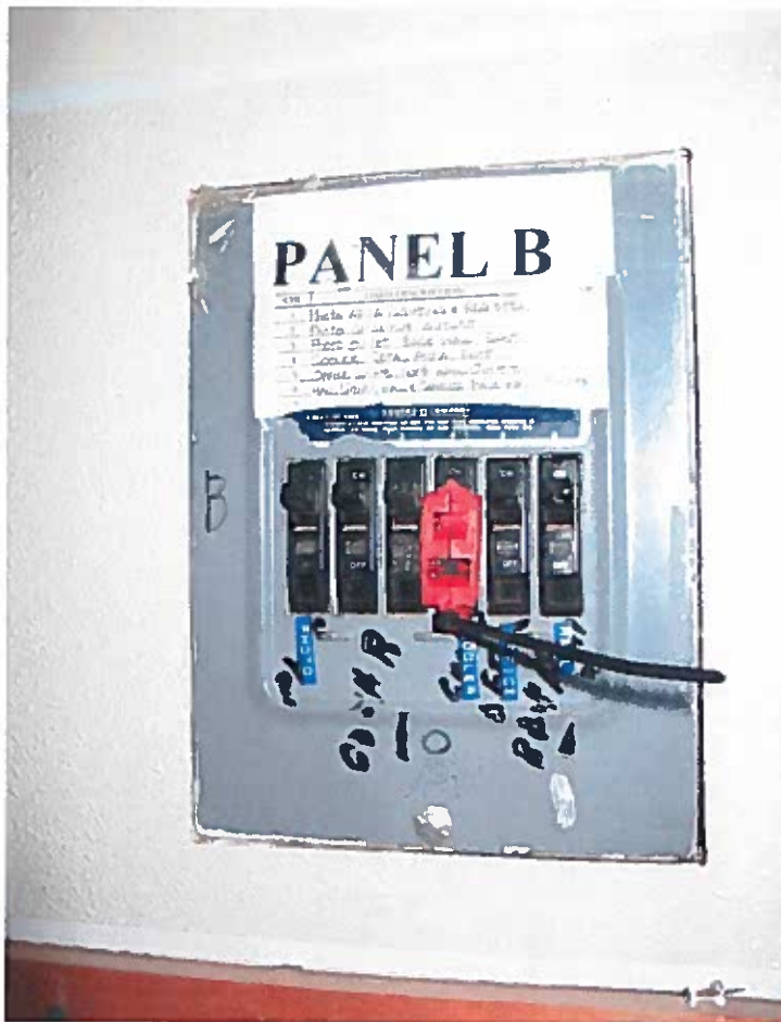
CIRCA 1971 ELECTRICAL PANEL; IT IS NOT KNOWN IF PANELS WILL REQUIRE BEING REPLACED. IT IS BELIEVED THAT THE CONDUIT AND CONDUCTORS WILL COMPLY WITH CURRENT CODES.
