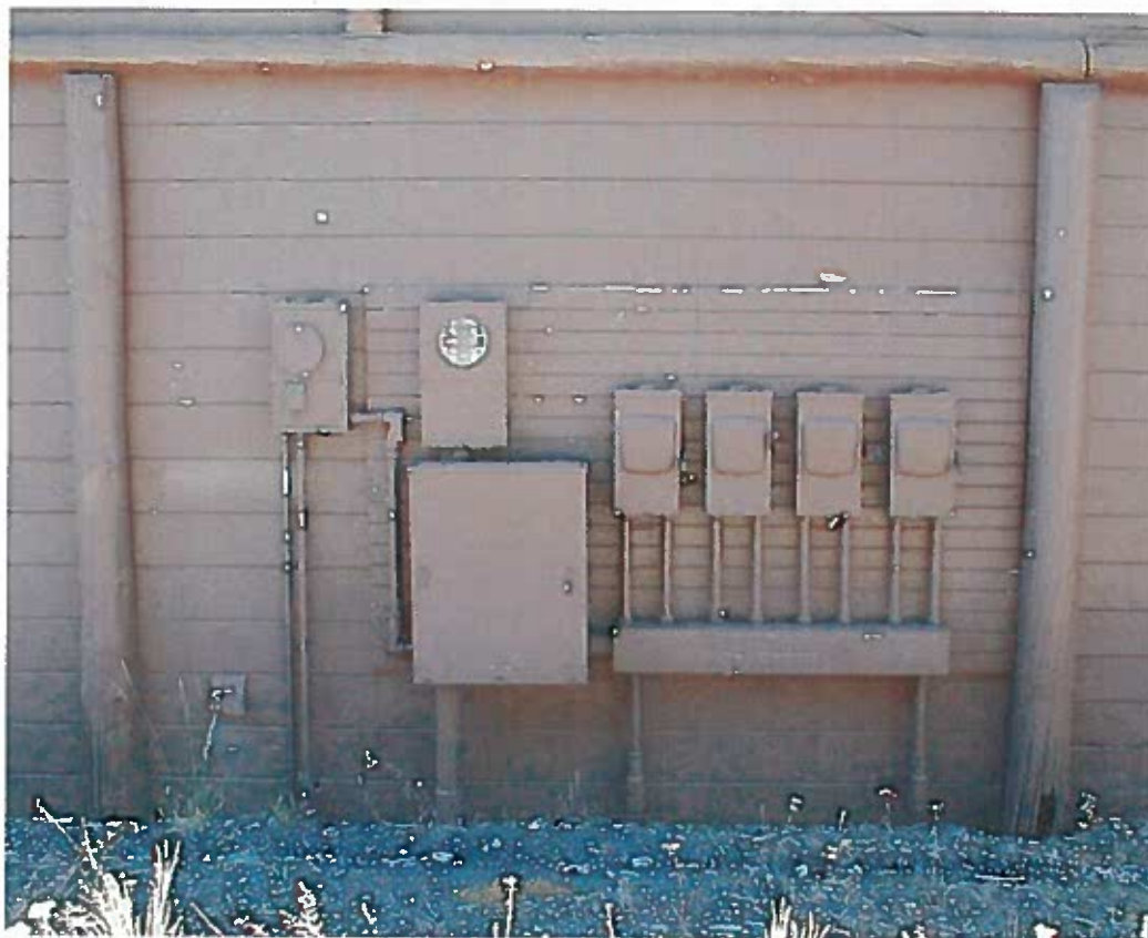
ELECTRICAL SERVICE CONNECTIONS LOCATED ON THE EAST WALL OF THE EXTERIOR OF THE STRUCTURE.
