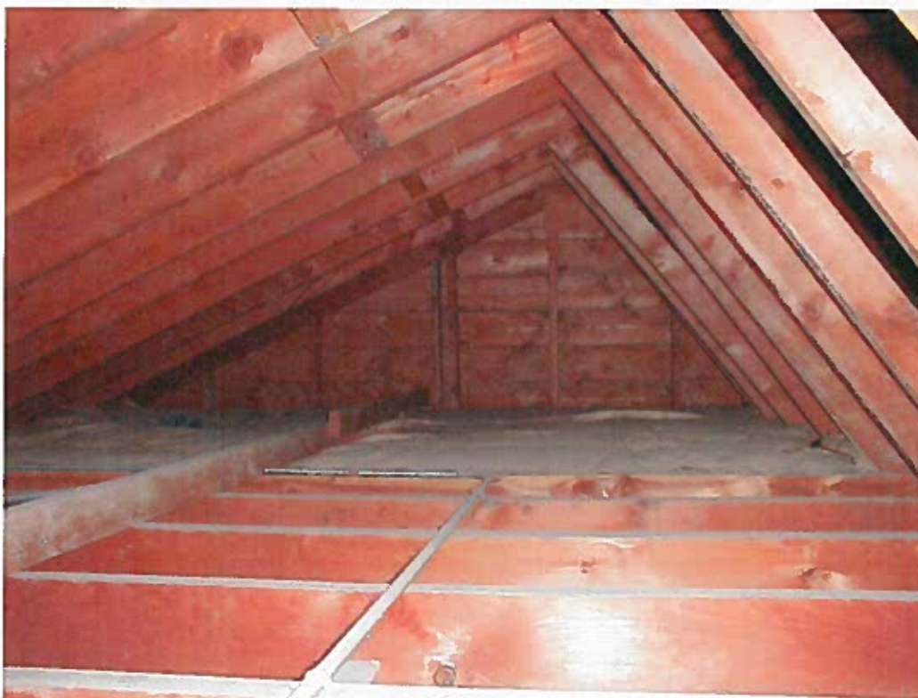
TYPICAL ROOF STRUCTURE ABOVE ORIGINAL DORMITORY WING - NOTE CONDITION OF RAFTERS, BRACES, AND JOISTS. THIS SECTION OF ROOF IS ALSO INSULATED ALTHOUGH IT IS NOT VISIBLE IN THIS PHOTO.
