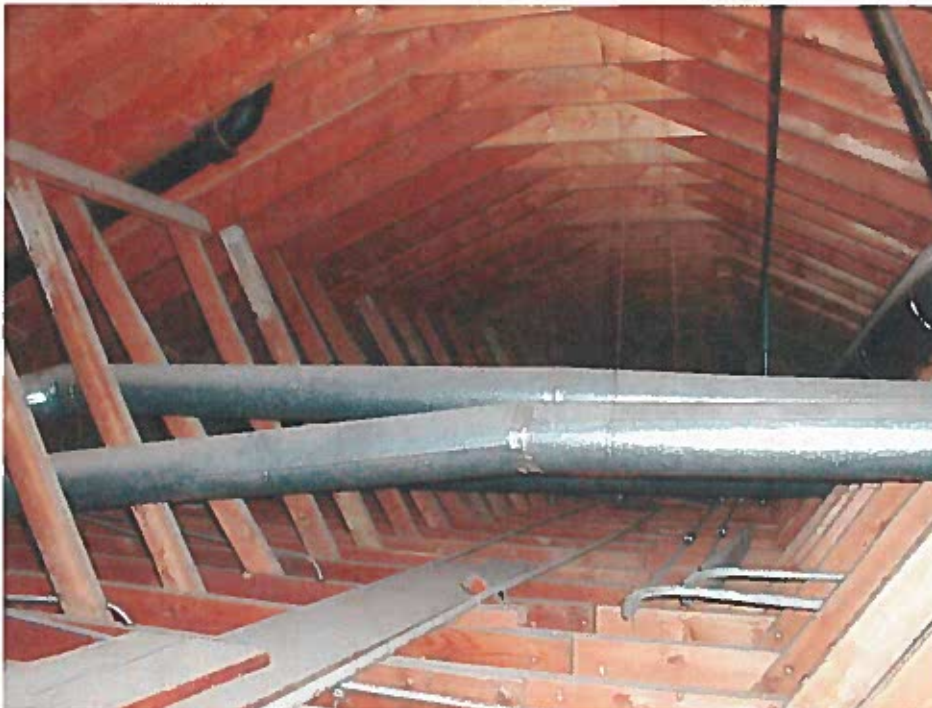
TYPICAL DISTRIBUTION DUCTWORK IN THE ATTIC SPACE OF THE DORMITORY WING.
