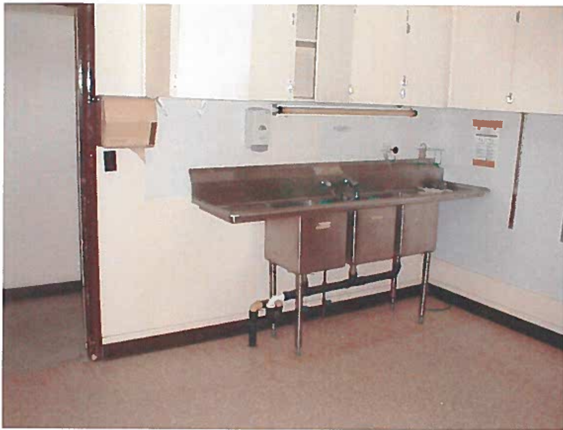
SINKS - COMMERCIAL KITCHEN AREA - SE CORNER OF DORMITORY WING; FIRST FLOOR
