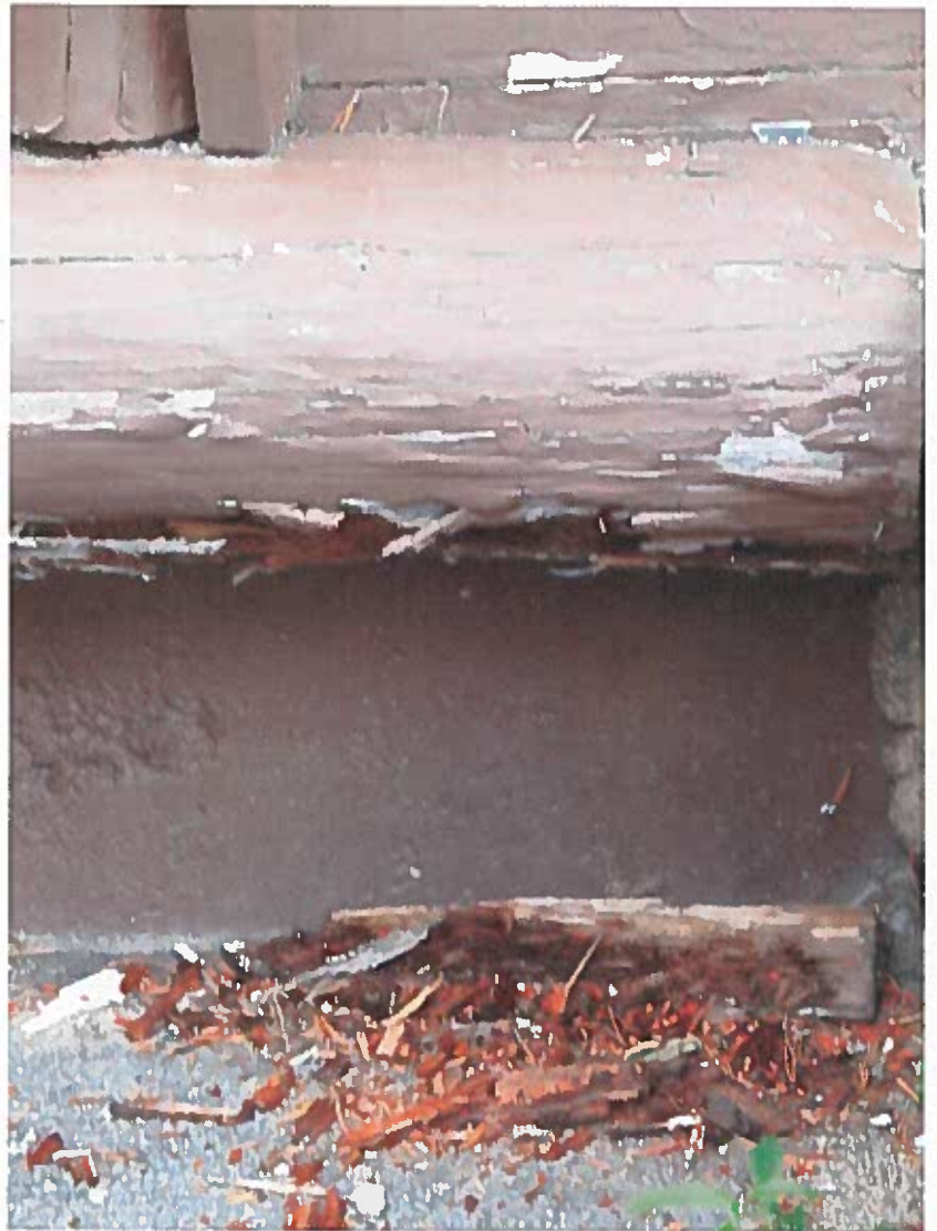
DETAILED PHOTOS OF LOG DETERIORATION IN THE APPLIED DECORATIVE SILL LOGS.
