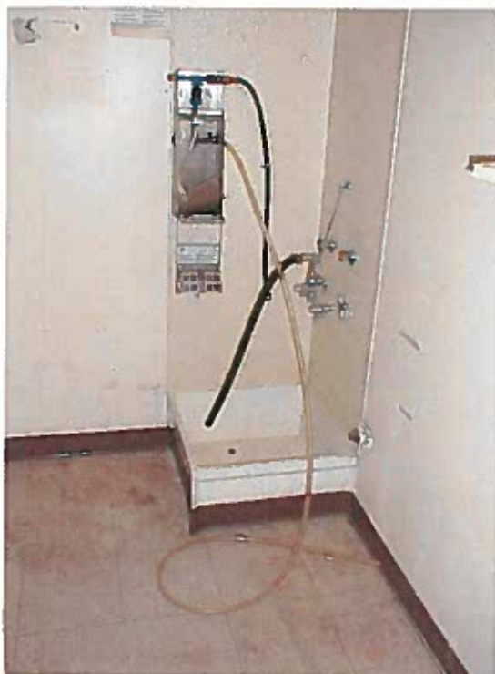
FLOOR SINK IN FIRST FLOOR MECHANICAL/UTILITY AREA.
