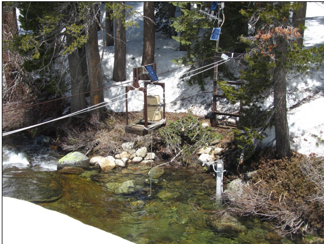
Figure 1.12. The Marble Fork above Tokopah Falls streamgage station. Cableway with auto sampler and staff plate on right bank.
