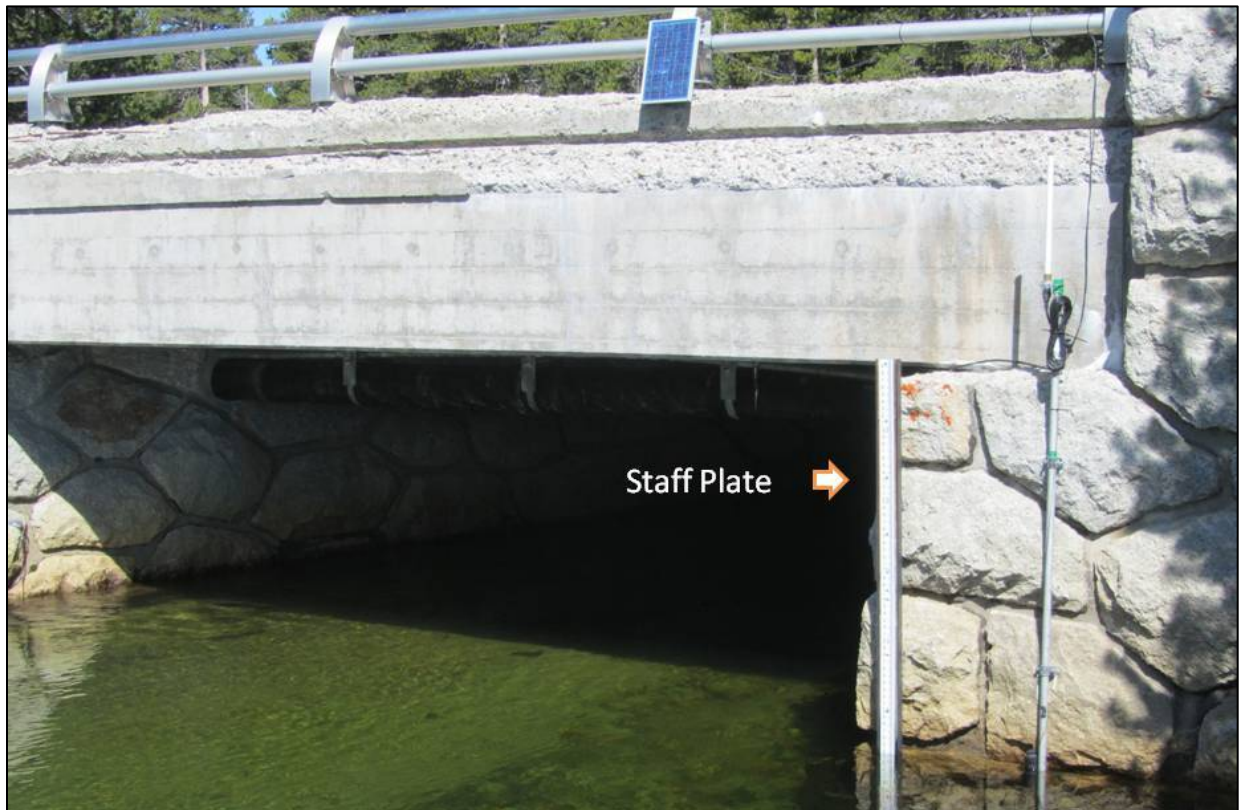
Figure 12. Typical staff gage with numerical gradations for reading water depth, the Tuolumne River at Tioga Road Bridge streamgage.
