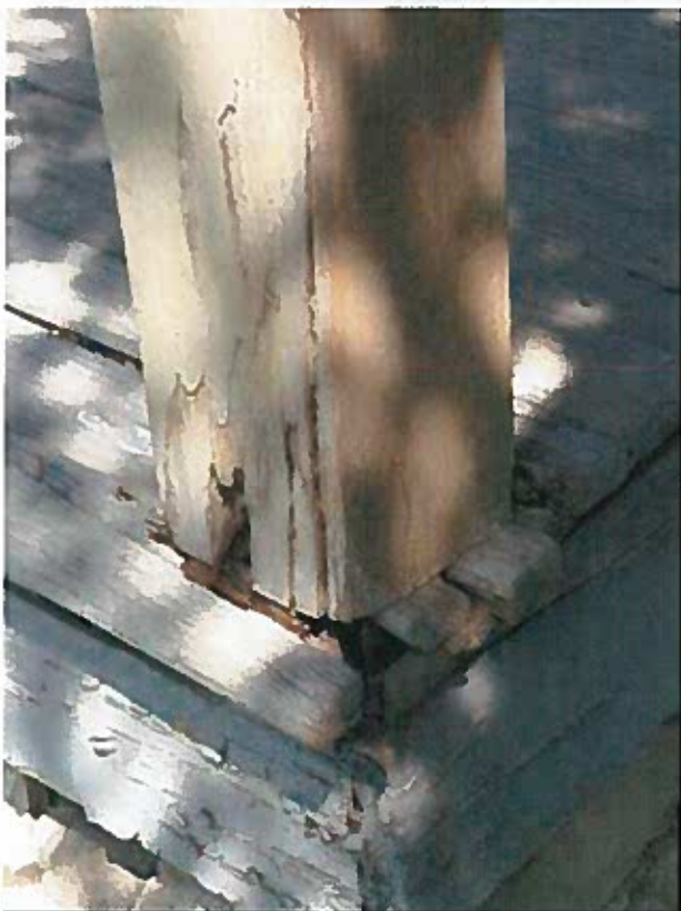
Condition at base of SE porch column. Photo Credit: Herb Dawson, NPS.
