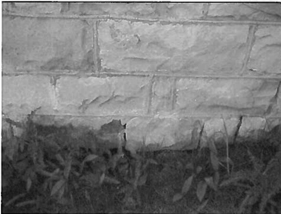
Degradation – base of north wall; east end. Photo Credit: Ken Sievert
