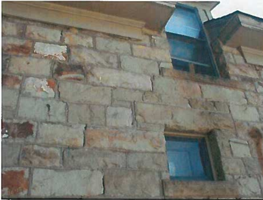
Closer view of cracks described on previous page. Photo Credit: Ken Sievert
