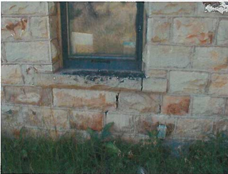
Failed mortar joints below north kitchen window; note crack in window sill. Photo Credit: Ken Sievert.
