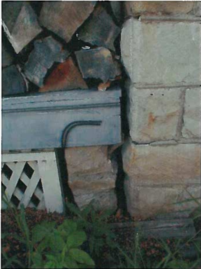
Stone porch piers along the north side of the entrance porch deck. Both piers are leaning and require stabilization. The latticework wood barrier adds architectural delicacy to the use of the structure as a place of residence, but is in need of repair. Photo Credits: Ken Sievert
