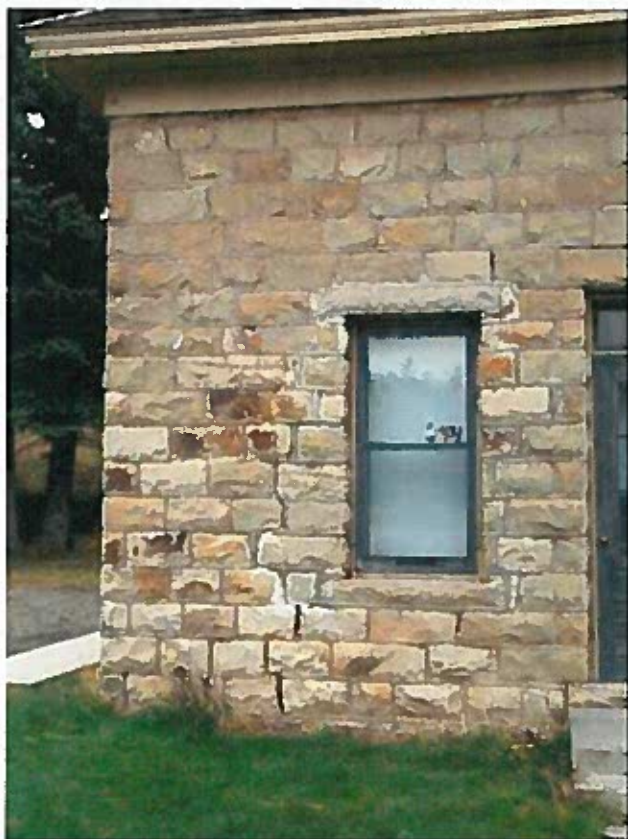
West end of south stone wall; this area of the structure exhibits the greatest amount of failed stone masonry in the building with significant cracks, spalls, and minor movement. Evidence of past repairs can be seen in some of the mortar joints in the detailed photos below, but deterioration has continued since the repairs. Photo Credits: Ken Sievert & Herb Dawson, NPS.
