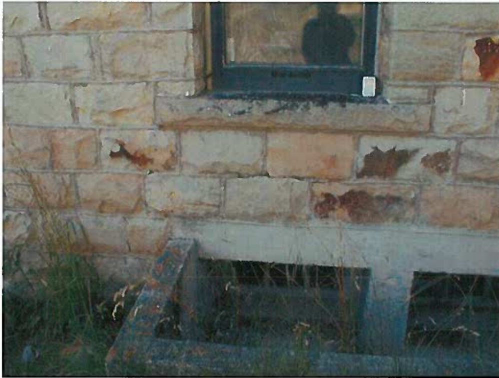
Stonework next to areaway along north wall. Note moss & lichen on concrete Areaway and window sill. Photo Credit: Ken Sievert
