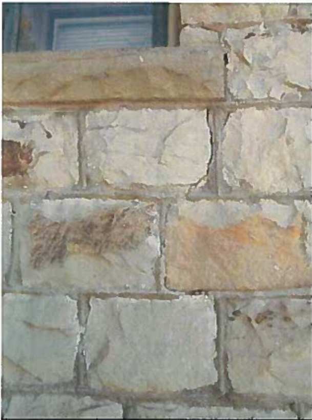
Slight crack below sill of west window; following the coursing of the stonework. Selected areas of the masonry joints have been repointed as can be seen near the bottom of the photo. Photo Credit: Herb Dawson, NPS.
