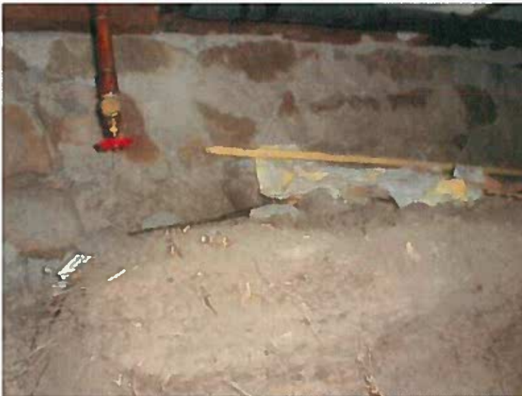
Water service adjacent to the east foundation wall. Photo Credit: Ken Sievert
