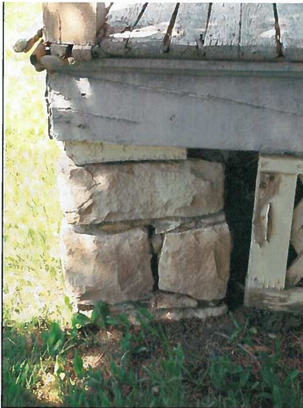
Stone porch pier at the SW corner of the entrance porch deck. The pier is rotated, fractured, and requires stabilization. Photo Credits: Herb Dawson, NPS.
