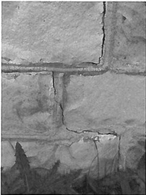
Crack at base of north wall. Photo Credit: Herb Dawson, NPS.
