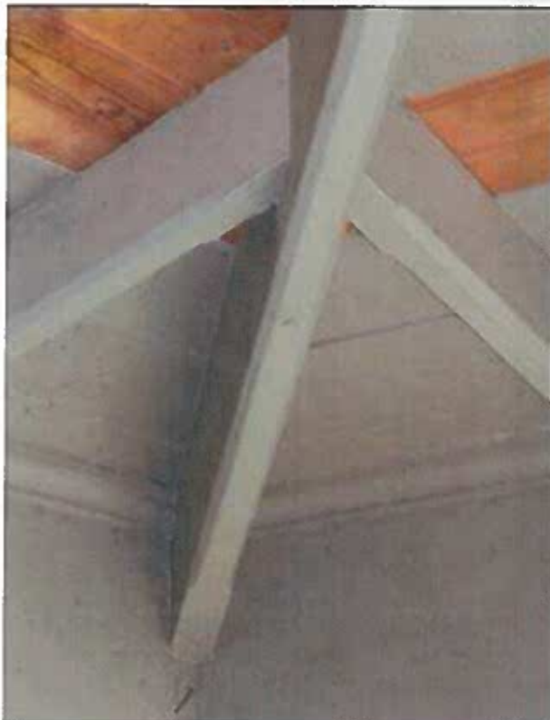
Beveled chamfers on the exposed framing members. Recently replaced sheathing boards are unpainted. Photo Credit: Herb Dawson, NPS
