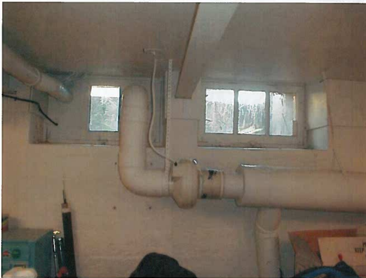
View of the north wall of the basement utility room. The pumped air system is for radon elimination from the sub-structure of the residence. Photo credit: Ken Sievert.
