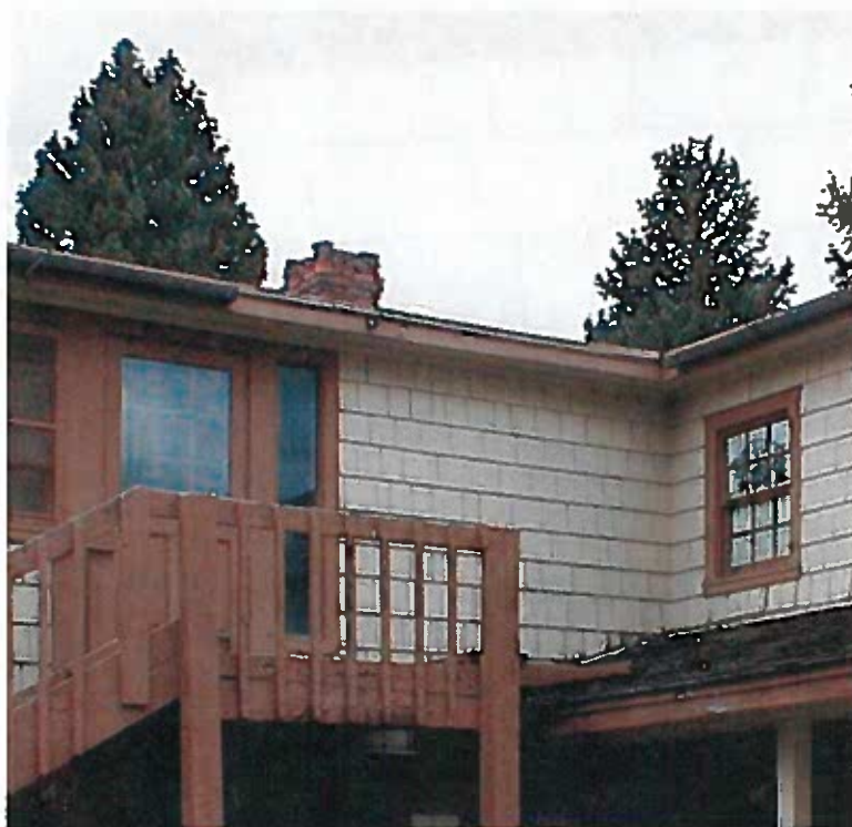
Re-entrant southeast corner; the exterior stair serves as a fire exit from the 2nd floor. Note the poor condition of the top of the brick chimney.
