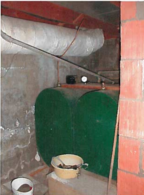
The presence of these heating oil tanks indicates that the building was once heated with an oil fired appliance. It is recommended that the tanks be removed.
