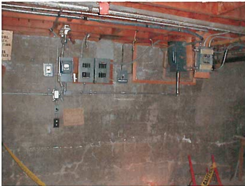
Electrical apparatus located at the south wall of the partial basement below the dormitory wing.
