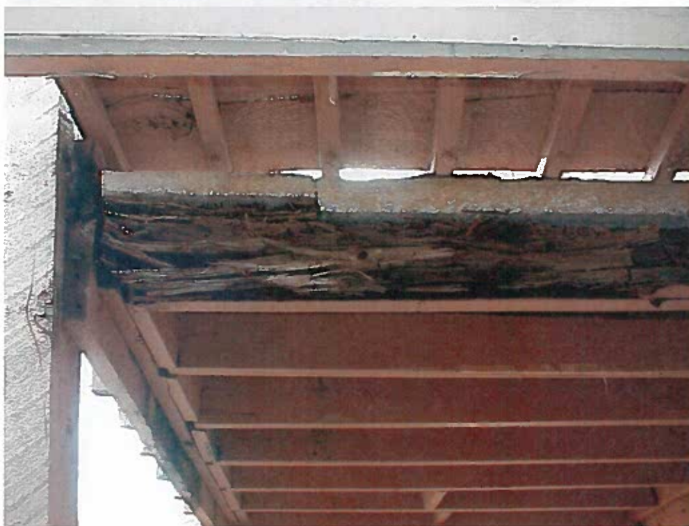
Close-up of the end (north) structural member beneath the exterior stair shown above. This member is beyond repair.
