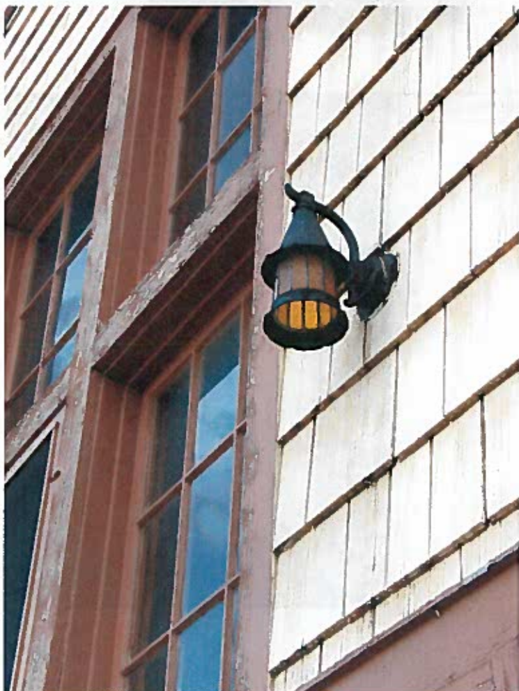
Exterior light fixture at the retail wing. It is not known if this is an original fixture; however, it is recommended that it be retained.
