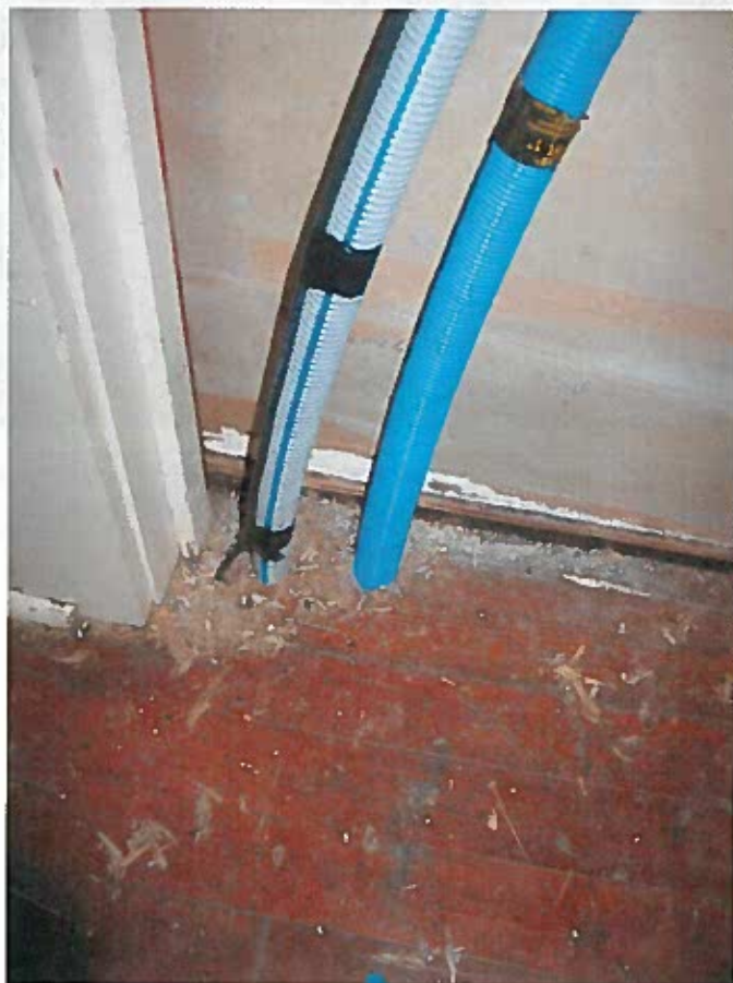
Contemporary wiring that has been intrusively installed in an abandoned doorway located in the southeast corner of room 109.
