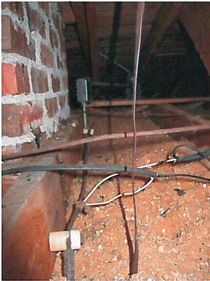
Numerous eras of electrical wiring—knob-and-tube, braided wire, romex, and metallic conduit—are evident next to the brick chimney in the attic.
