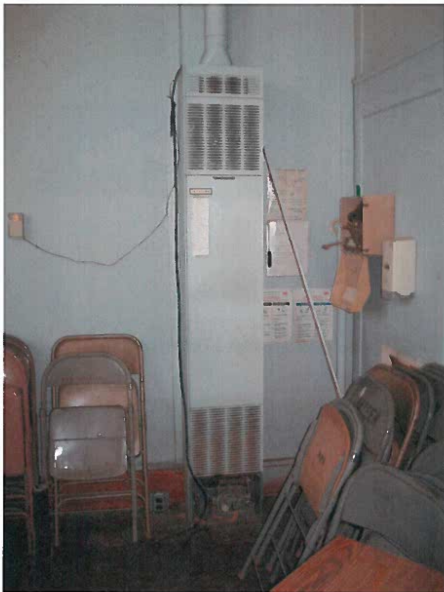
This cabinet heater is located at the southwest corner of the retail sales area; its condition is unknown but it is unlikely that it would be suitable for use again.
