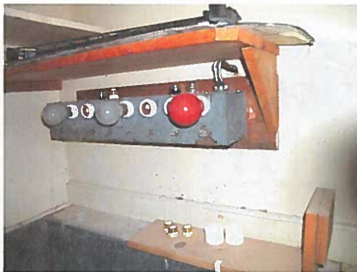
Detail of safelight control at the darkroom sink.
