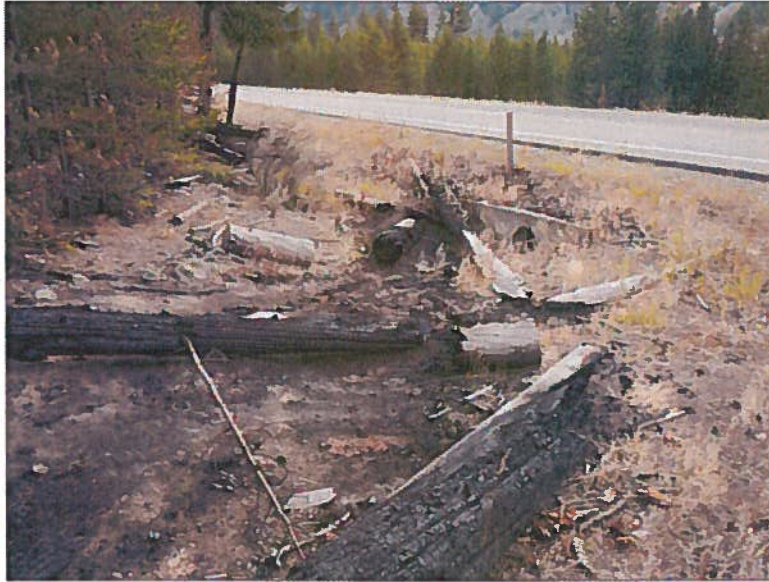
Figure 10. Floatable woody debris adjacent to a culvert.
