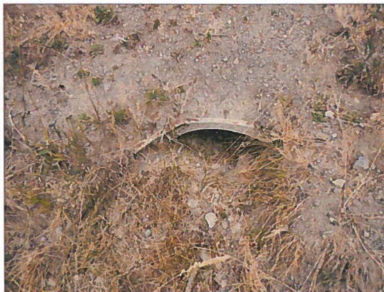
Figure 11. A plugged culvert along the West Entrance Road.
