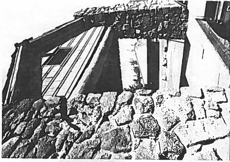
Figure 39: Looking northwest at the end of the east bay of the station. Note the missing log under the shingles, and the loose and missing stonework in the columns.
