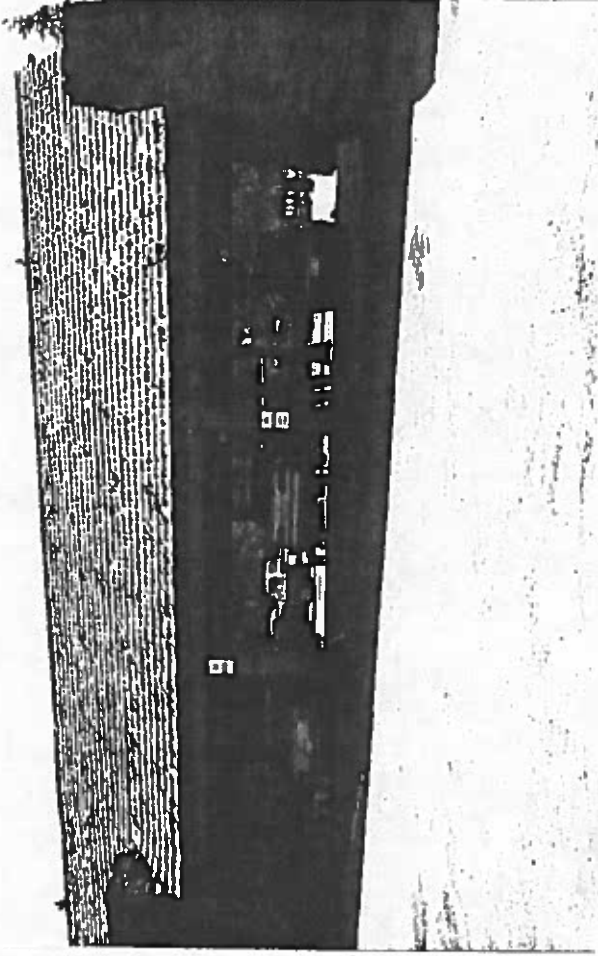
Figure 51: Looking east at the service bay of the station. Note the cupped and curled shingles on the roof.
