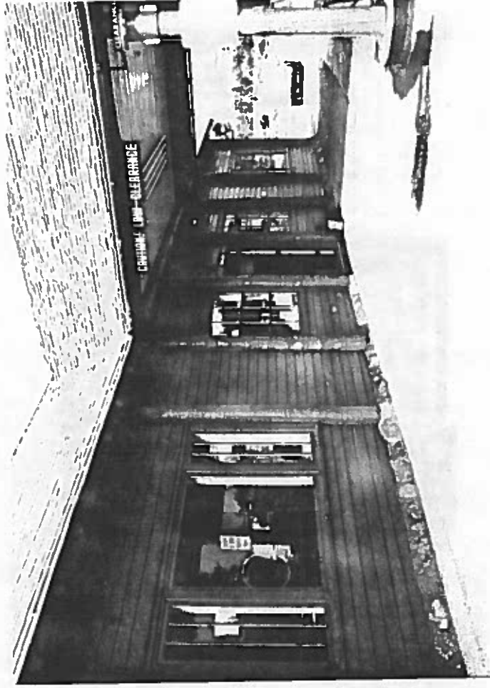
Figure 10: Looking southwest at the front of the station towards the front entrance. Note the good windows and the stone base. Also, note the rotted roof rafter and the condition of the shingles on the roof at the right.
