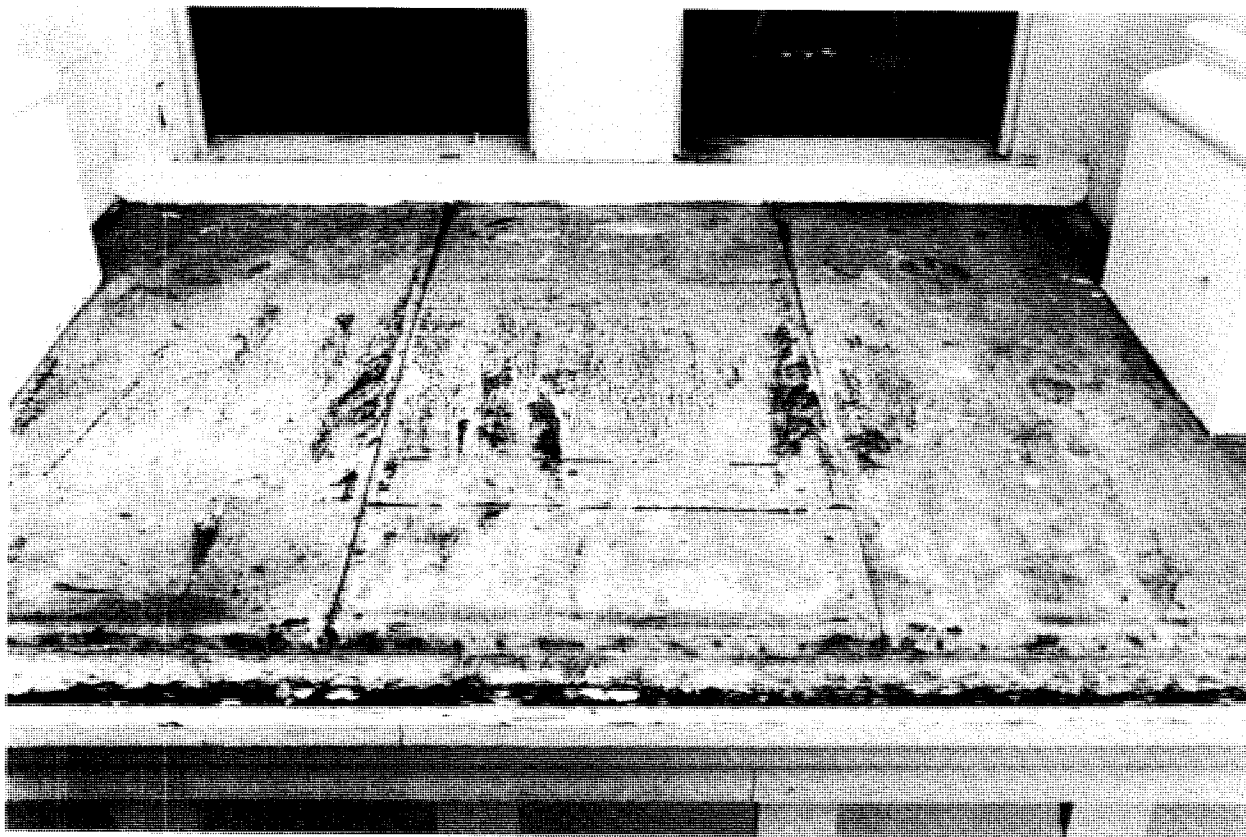
Illustration 28. Penniman House: West Facade, Flashing at Base of Center Dormer Window (1984).
