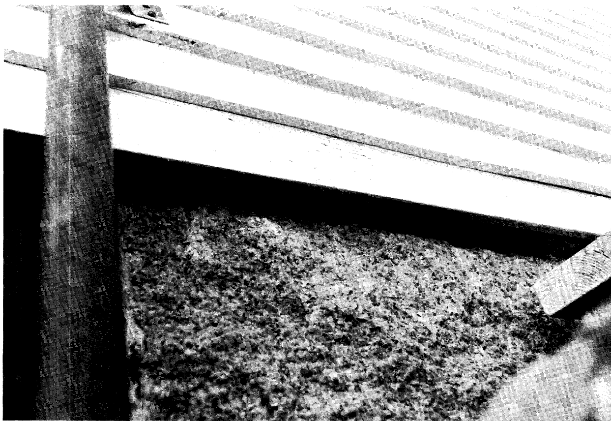
Illustration 16. Penniman House: East Facade, Showing Ends of Vertical Sheathing Boards Under Clapboards (1984).
