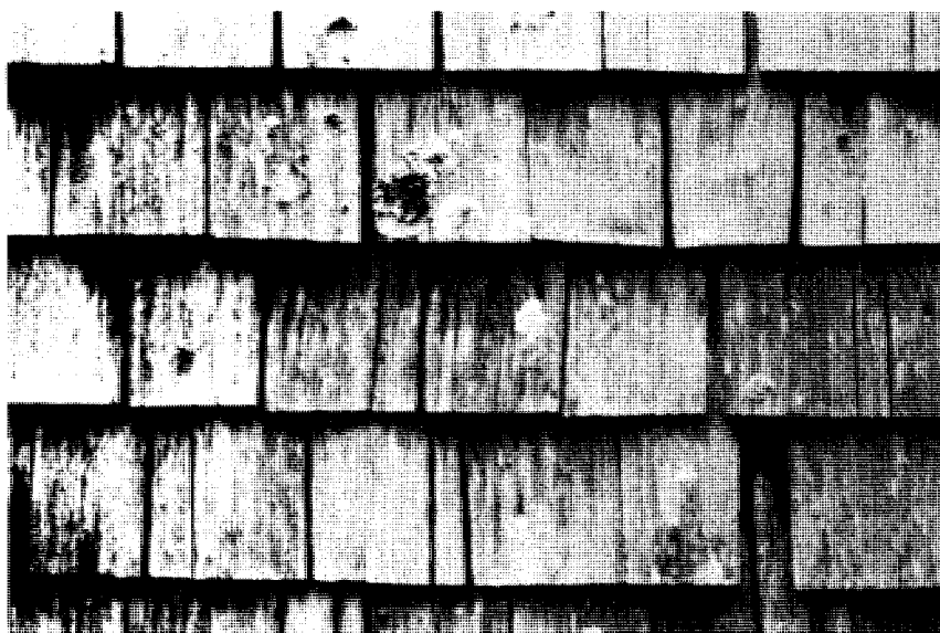
Illustration 102. Atwood-Higgins House: East-Elevation Shingles, Fungal Growth.
