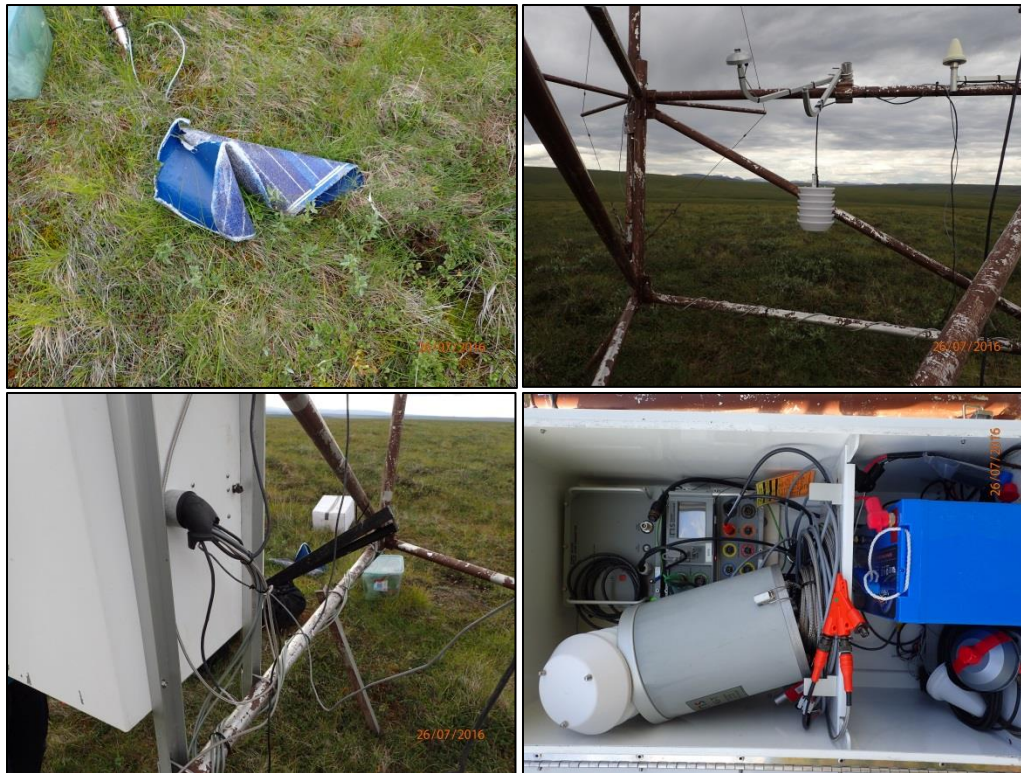
Figure 20. Noatak fire RAWS station, July 26, 2016. Clockwise from top: damaged solar panel, damaged sensors, damaged cables, replacement sensors left in enclosure at departure.
