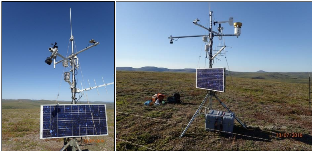
Figure 12. Tahinichok climate station July 13, 2016 shown before (left) and after (right) repairs. Upon arrival at the station, the AT-RH sensor and cable were damaged, the snow depth cable was damaged, and the tipping bucket and snow depth sensors were out of level.
