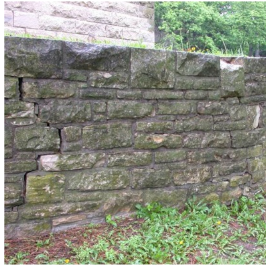
Figure 10. Stone Retaining Wall with Joint Cracking
