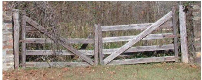
Figure 3. Missing Sections in Wood Gate
