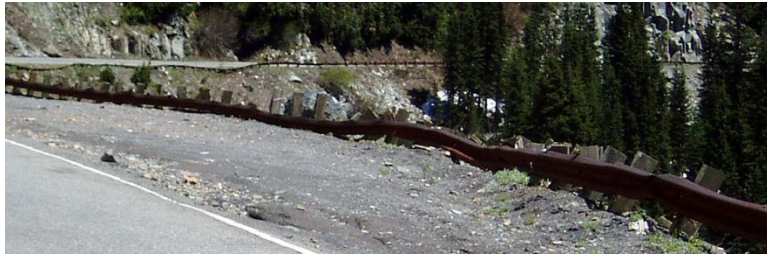
Figure 4. Guardrail and Posts Out of Alignment
