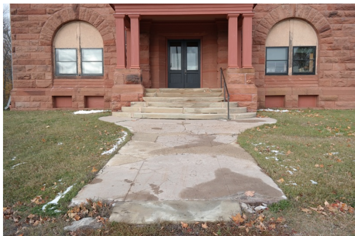
Figure 18. Cracked and Deteriorated Walkway
