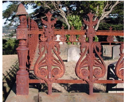
Figure 1. Corrosion of Metal Railing
