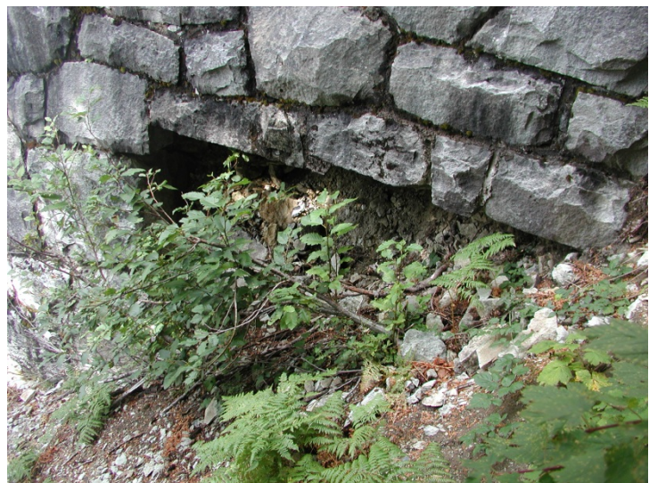
Figure 11. Retaining Wall with Stones Missing
