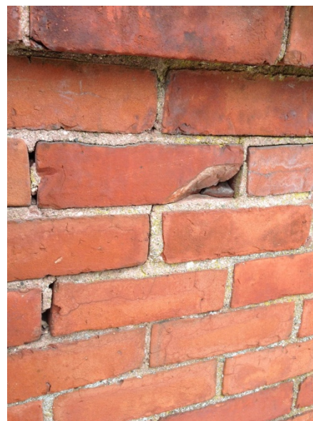
Figure 12. Brick Wall with Spalling
