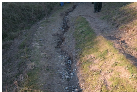
Figure 14. Eroded Trail Tread
