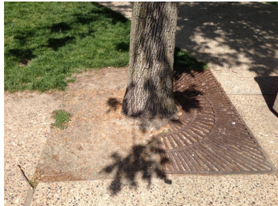
Figure 8. Partially Missing Tree Grate
