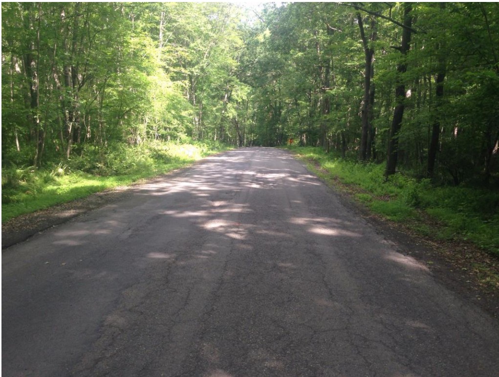
Photograph 1. Photo looking northwest at a degraded section of Old Mine Road within the project study area. P. Sharpe - June 2017. (Photo Location Map – Appendix A)
