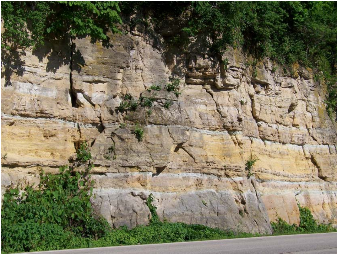
Figure 1. Cambrian Jordan Sandstone exposed in the cliff adjacent to the road leading to the monument road, north of McGregor, Iowa. Vertical fractures in the relatively horizontal strata become conduits for groundwater flow. In the winter, water freezes in the fractures and expands, causing increased pressure on the surrounding rock. When the ice thaws, the pressure is released, and weakened sandstone blocks may spall off the cliff and onto the road. Photograph courtesy of John Graham, Colorado State University. View is of the Jordan Sandstone across the road from the historical marker commemorating the old military trail used by troops in 1840 when traveling from Fort Crawford in Wisconsin to build Fort Atkinson in Iowa.
