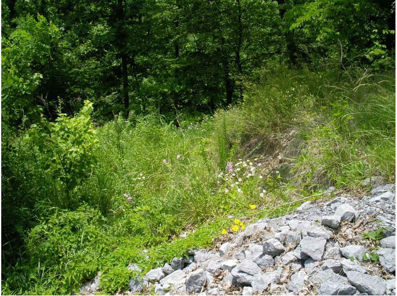
Figure 6. Area prone to slumping along Wilderness Road with rip rap installed in an effort to stabilize the slope. Photograph is by Lisa Norby (NPS-GRD).
