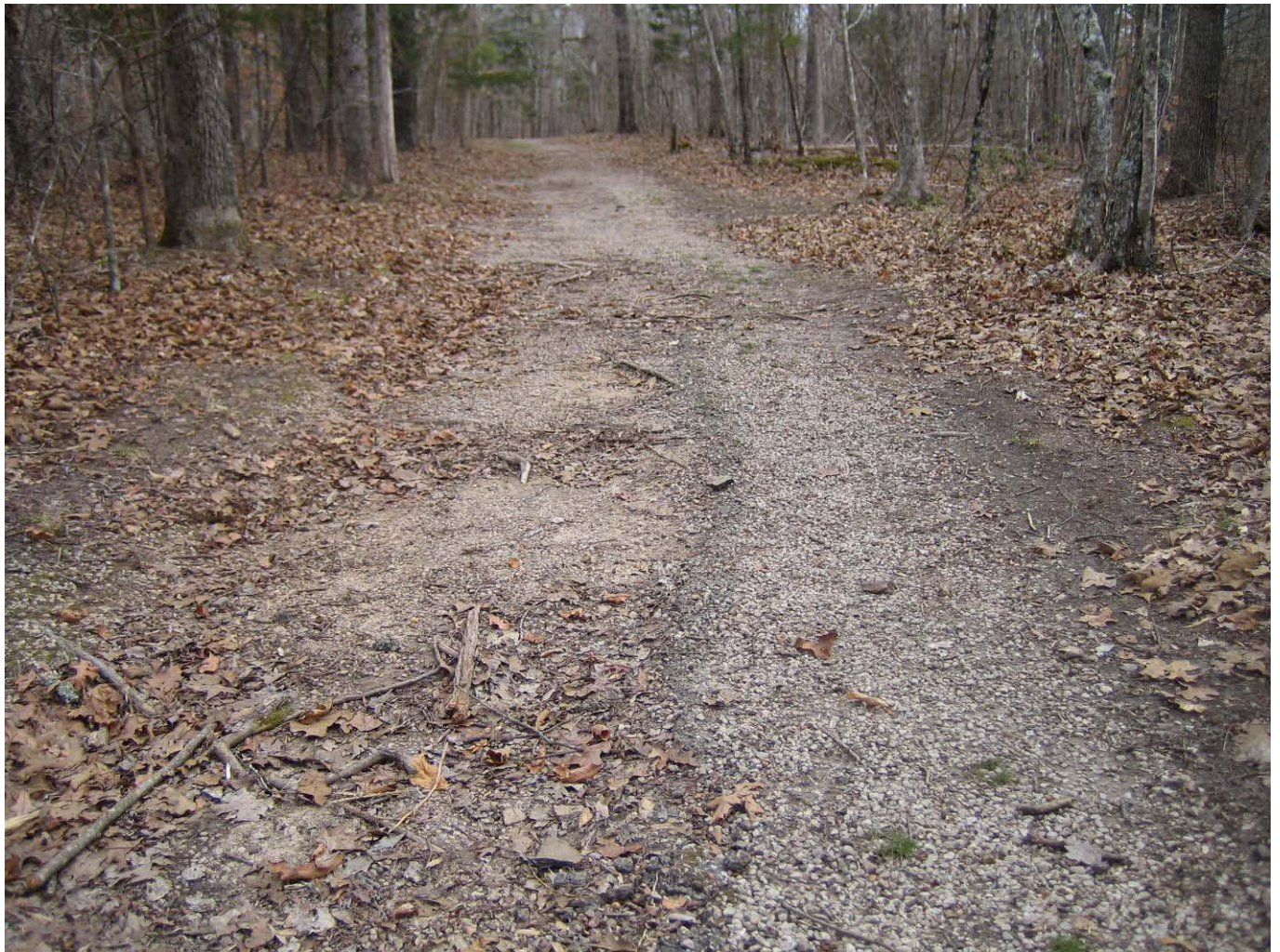
Figure 4. Erosion along a trail near Rhea Springs towards a Confederate burial trench. Note unsuccessful asphalt surface on the right side of the trail installed to improve access and curb erosion. Photograph is by Trista L. Thornberry-Ehrlich (Colorado State University).
