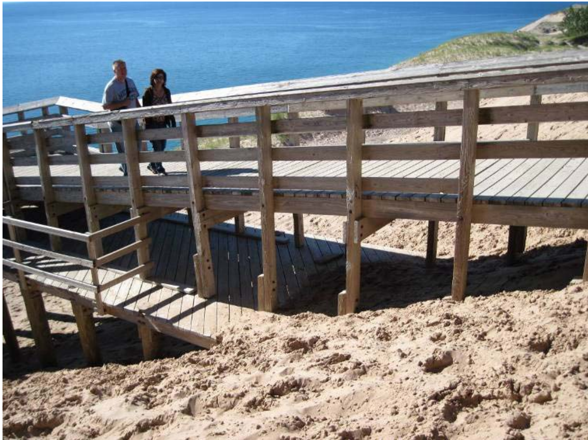
Figure 10. Windblown sand. Blowing sand periodically covers the overlook structure, and moving sand exposes posts at the Lake Michigan Overlook. Photo by Katie KellerLynn.
