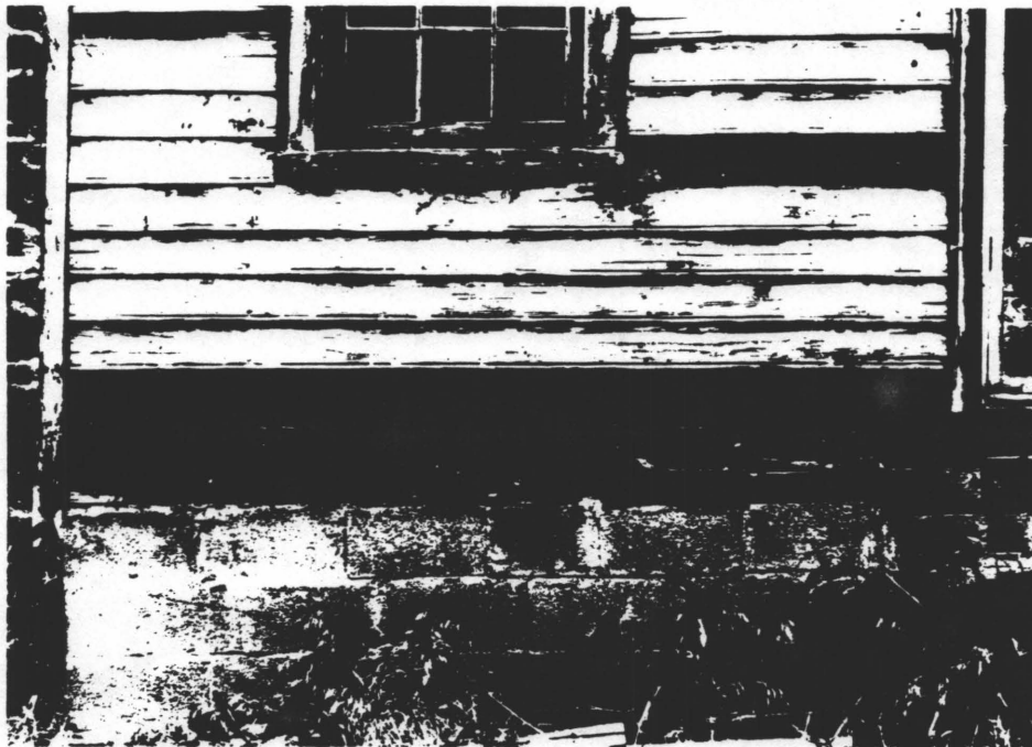
PHOTOGRAPH 10 ORIGINAL CABIN, WEST END OF THE SOUTH ELEVATION SILL. THE ORIGINAL SILL (WEST OF THE DOOR) IS UNDERPINNED BY CONCRETE BLOCK DATING TO THE 1940s.
