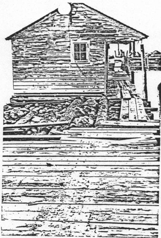
South view of the fish house and main approach to the dock. Majority of the planking needed to be replaced along with a few main log stringers.
